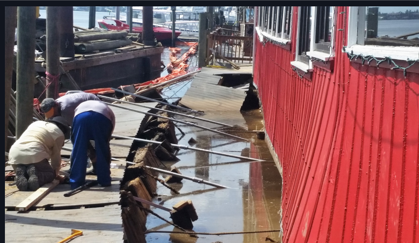
Dock damage at Tin City
