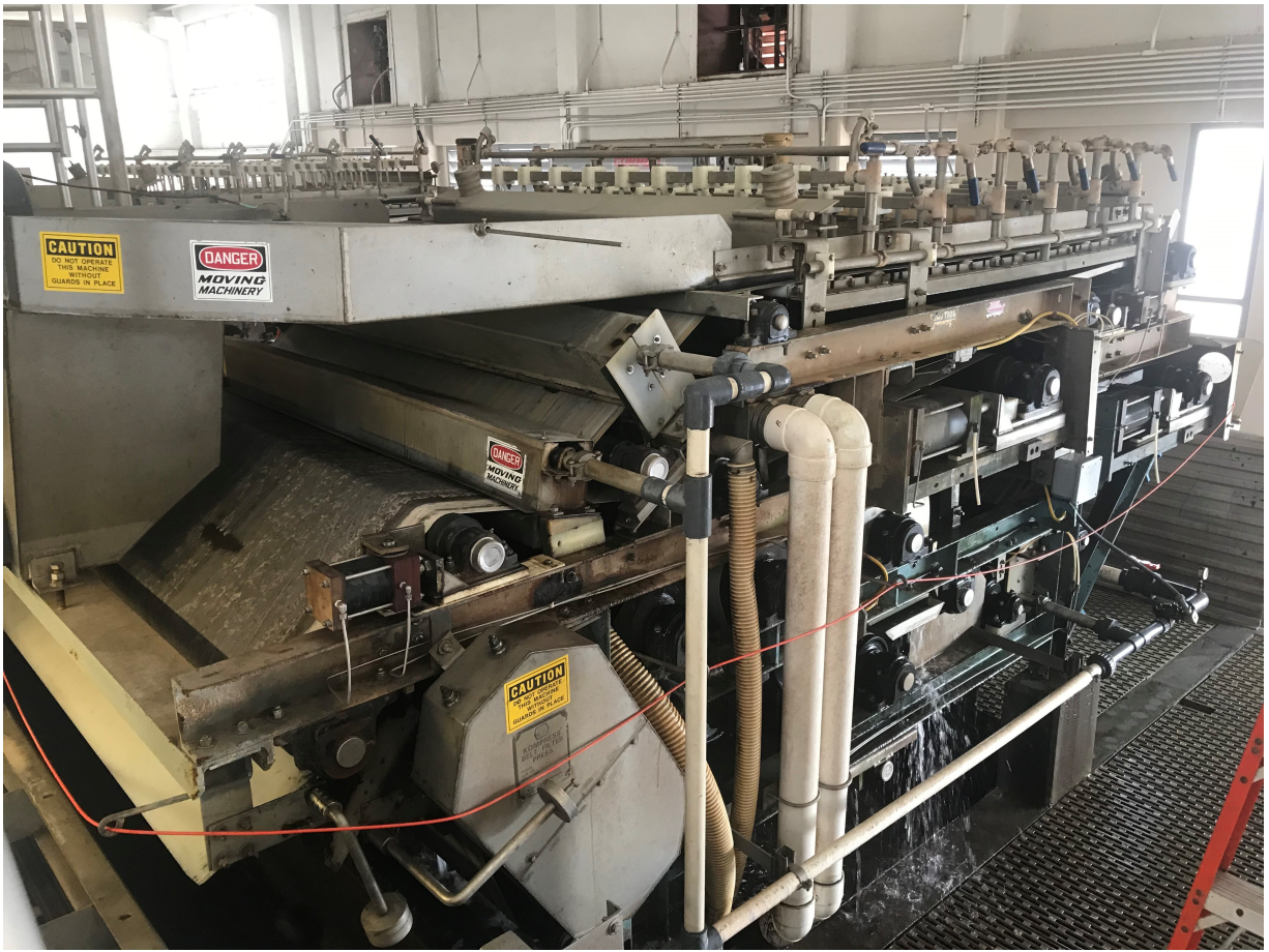
Three Belt Filter Presses
