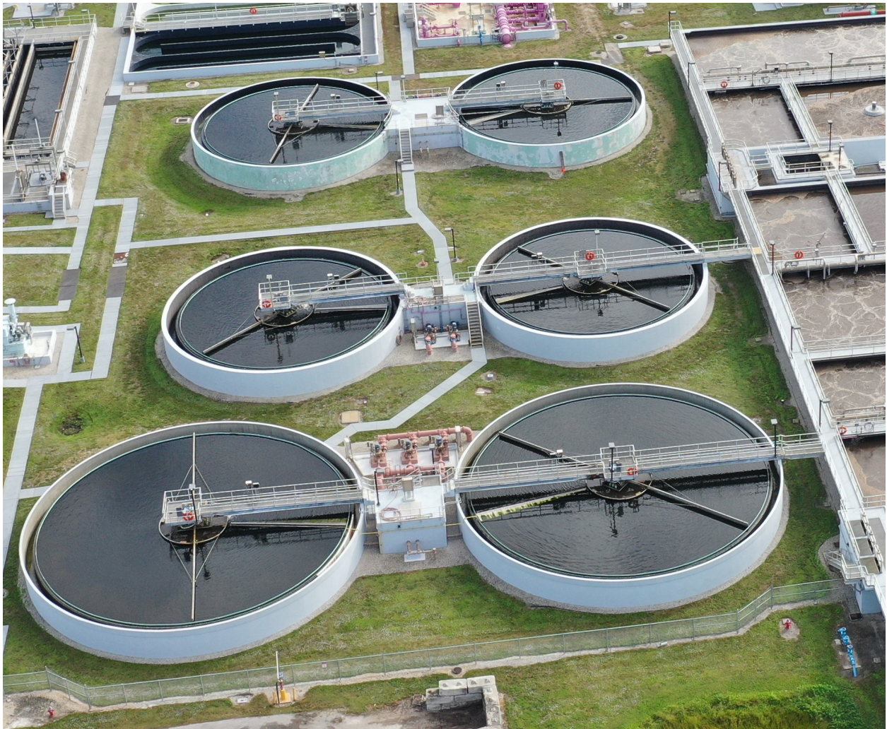
Six Final Clarifiers
