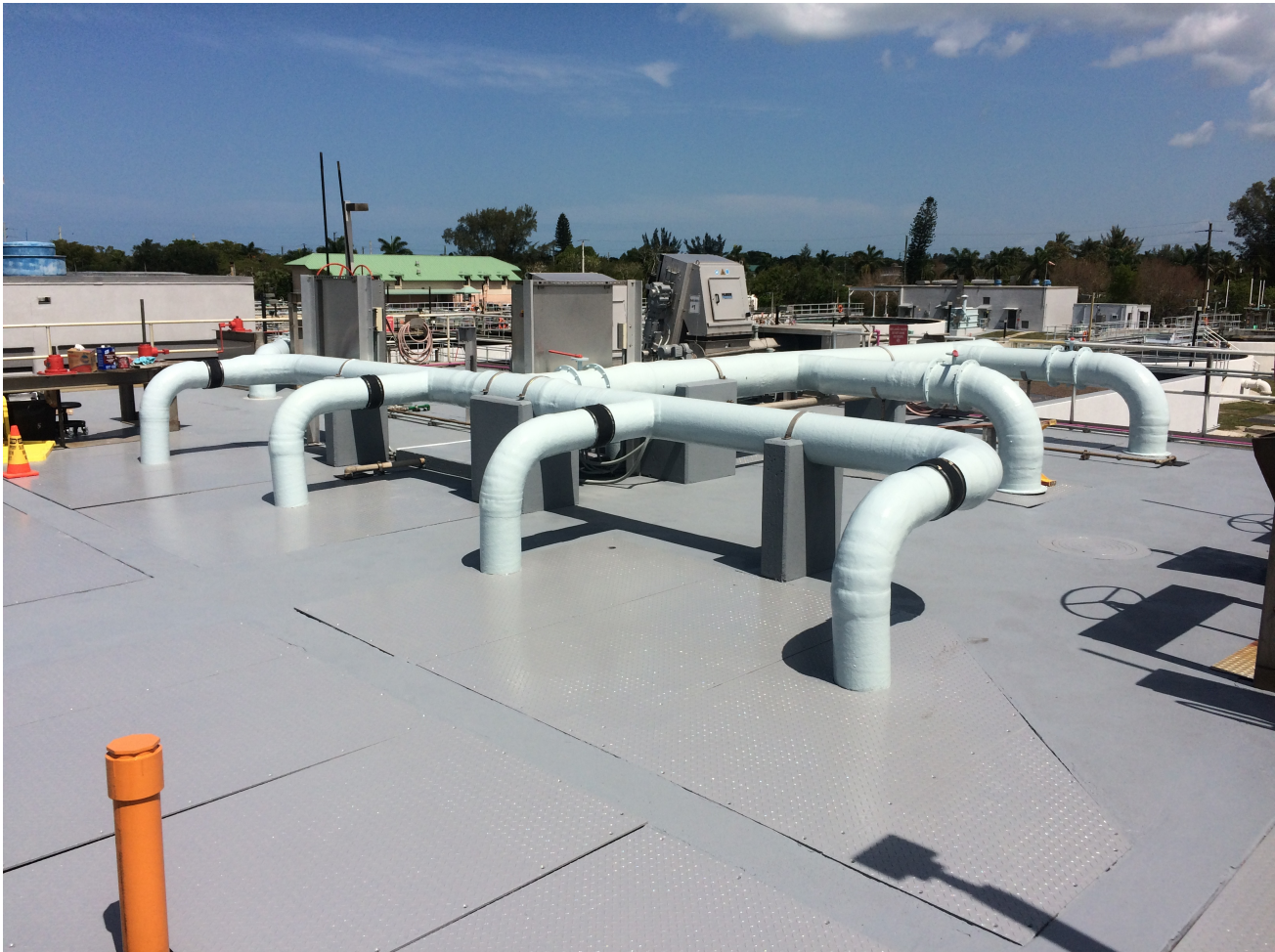
Covered Channels & Odor Control Ductwork
