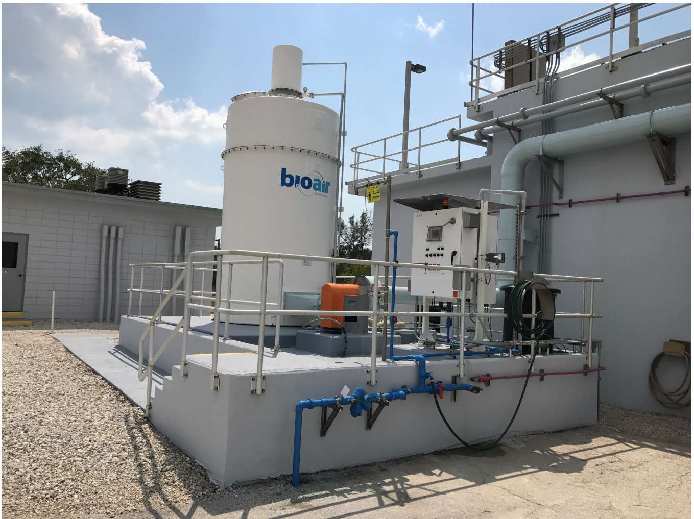
Odor Control Unit
