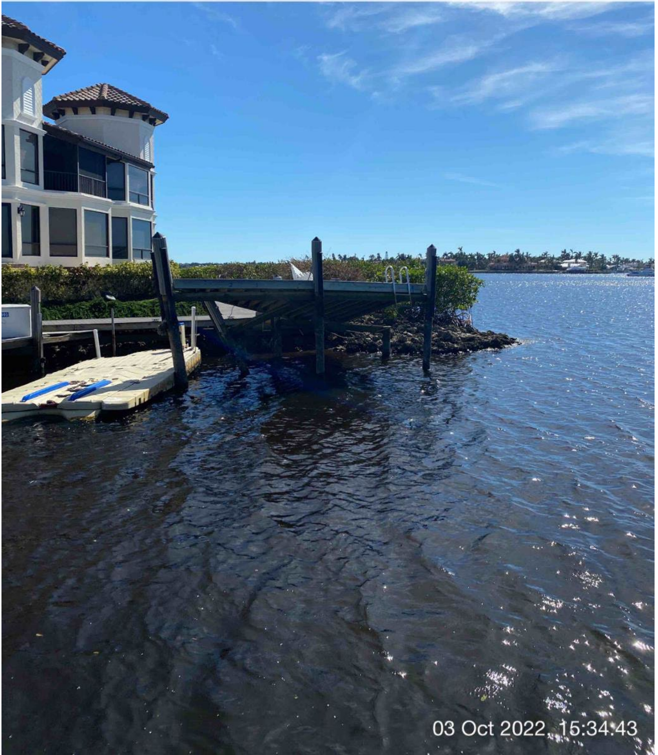
Destroyed dock at station 1+00 in Canal W-W
