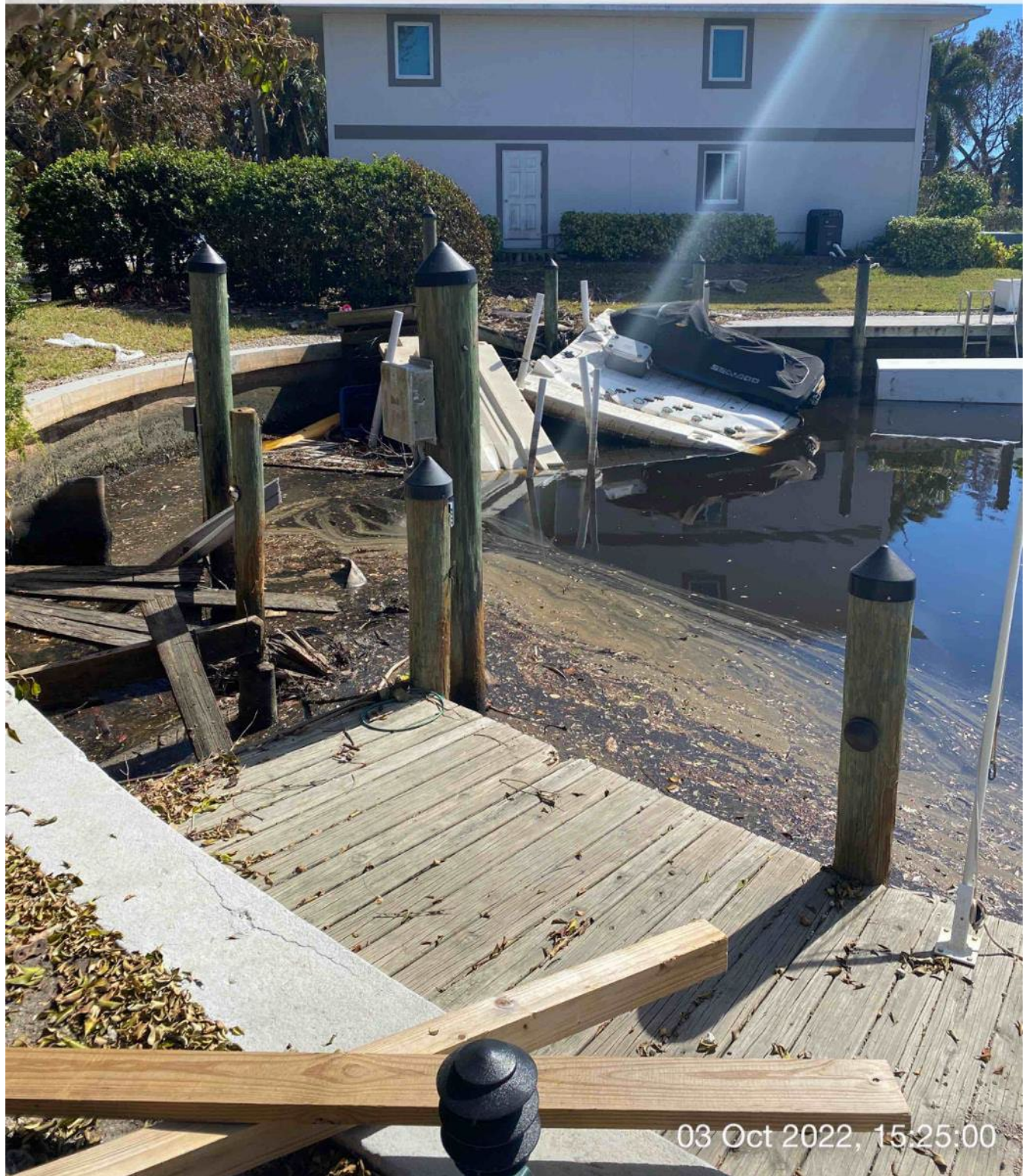
Destroyed dock and debris at station 19+30 in Canal W-W
