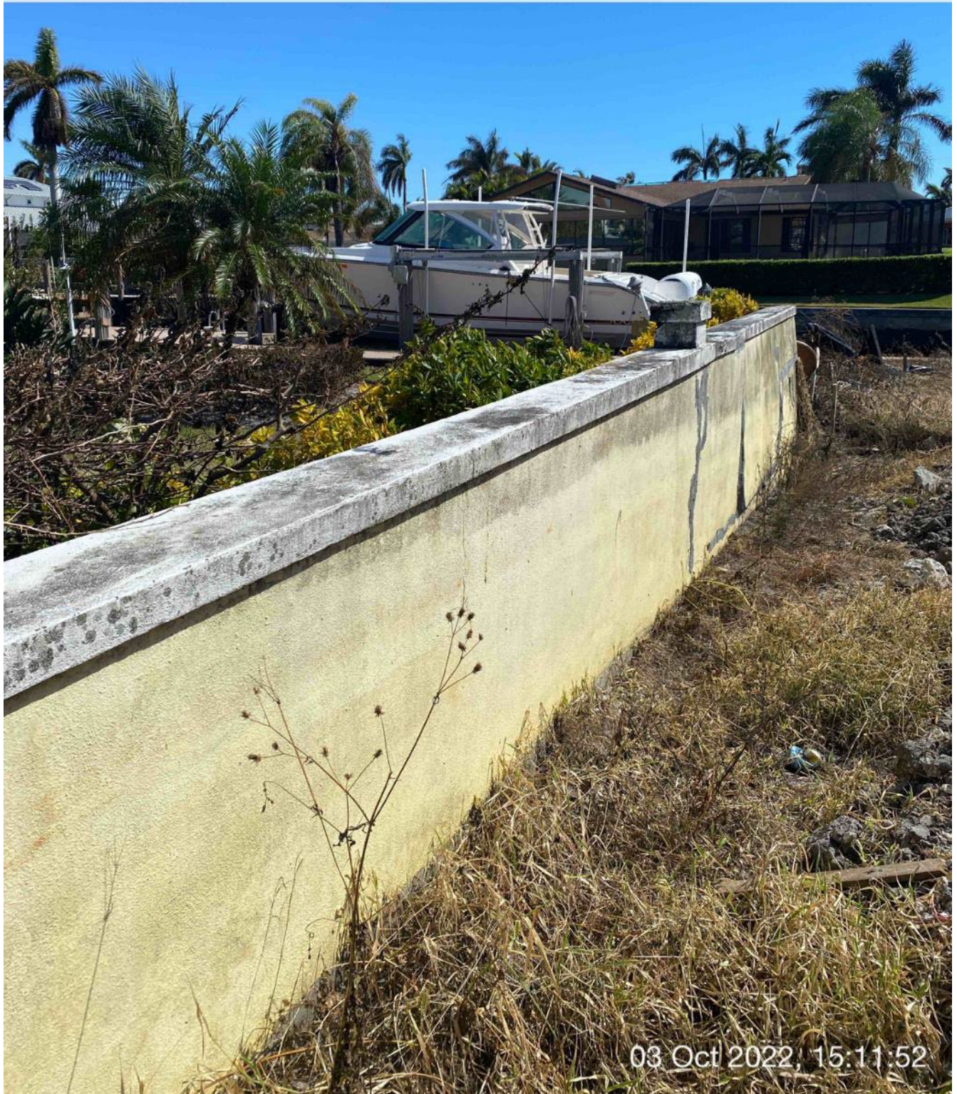
Debris and high water mark on east side wall at 1300 Curlew Avenue
