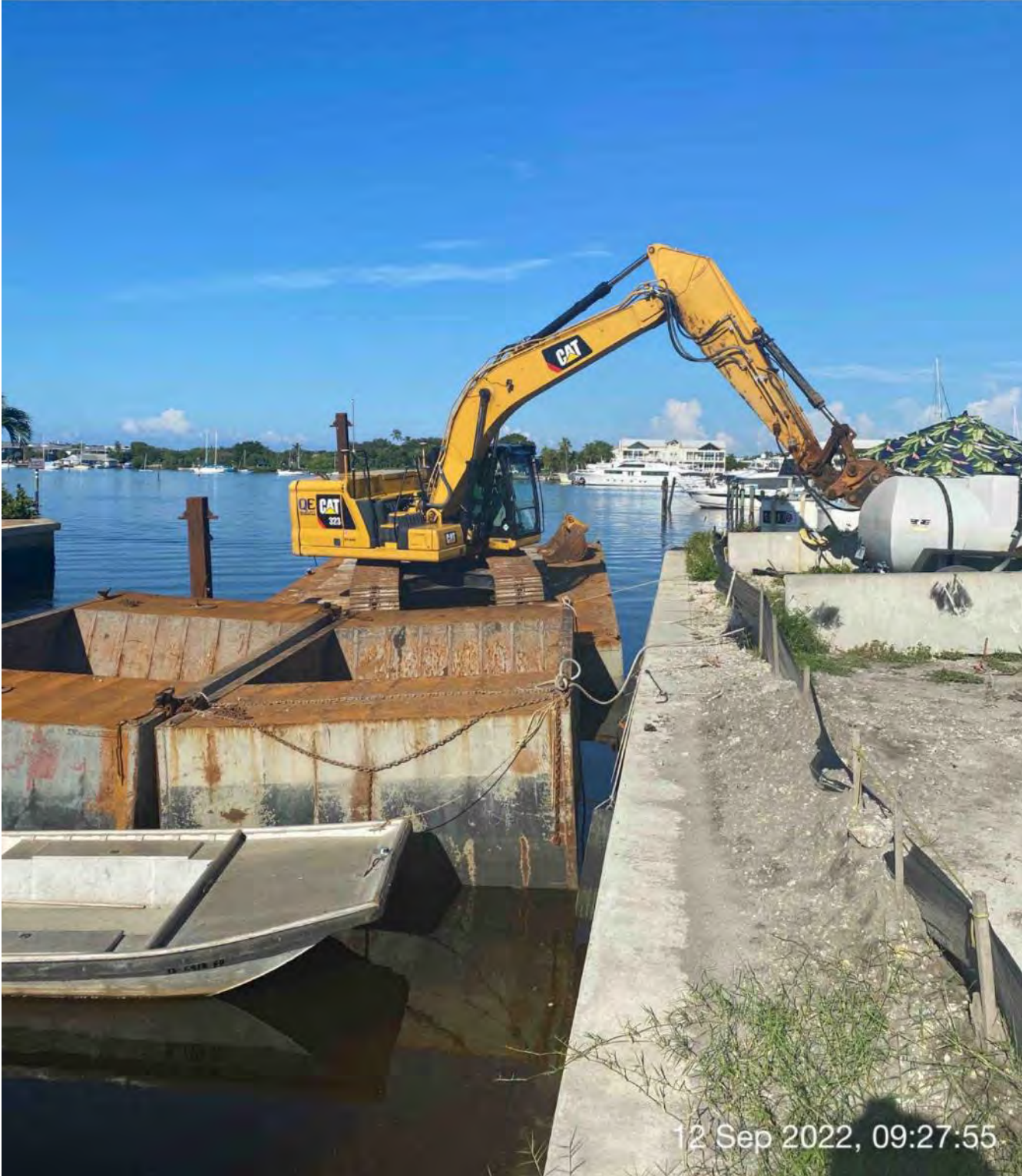
323 excavator, barge, hoppers, and support boat staged in Canal CC-CC between stations 1+00 and 2+00
