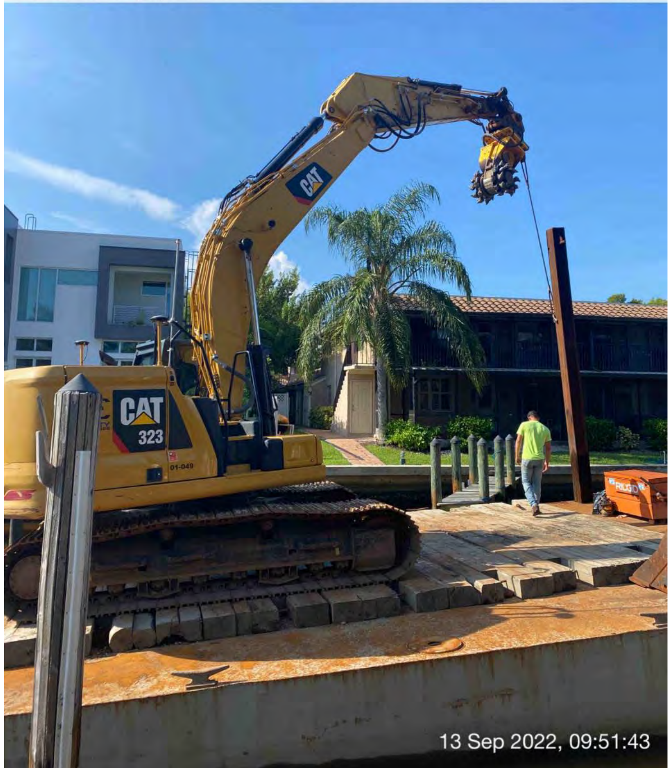
323 excavator lifting spud to allow push boat to mobilize barge at station 15+00
