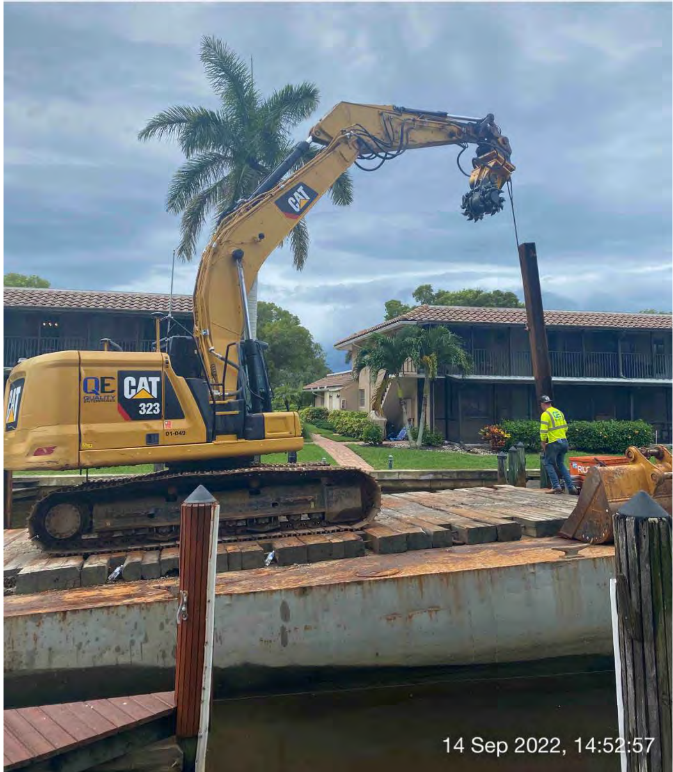
323 excavator lifting spud to allow push boat to mobilize barge at station 14+25
