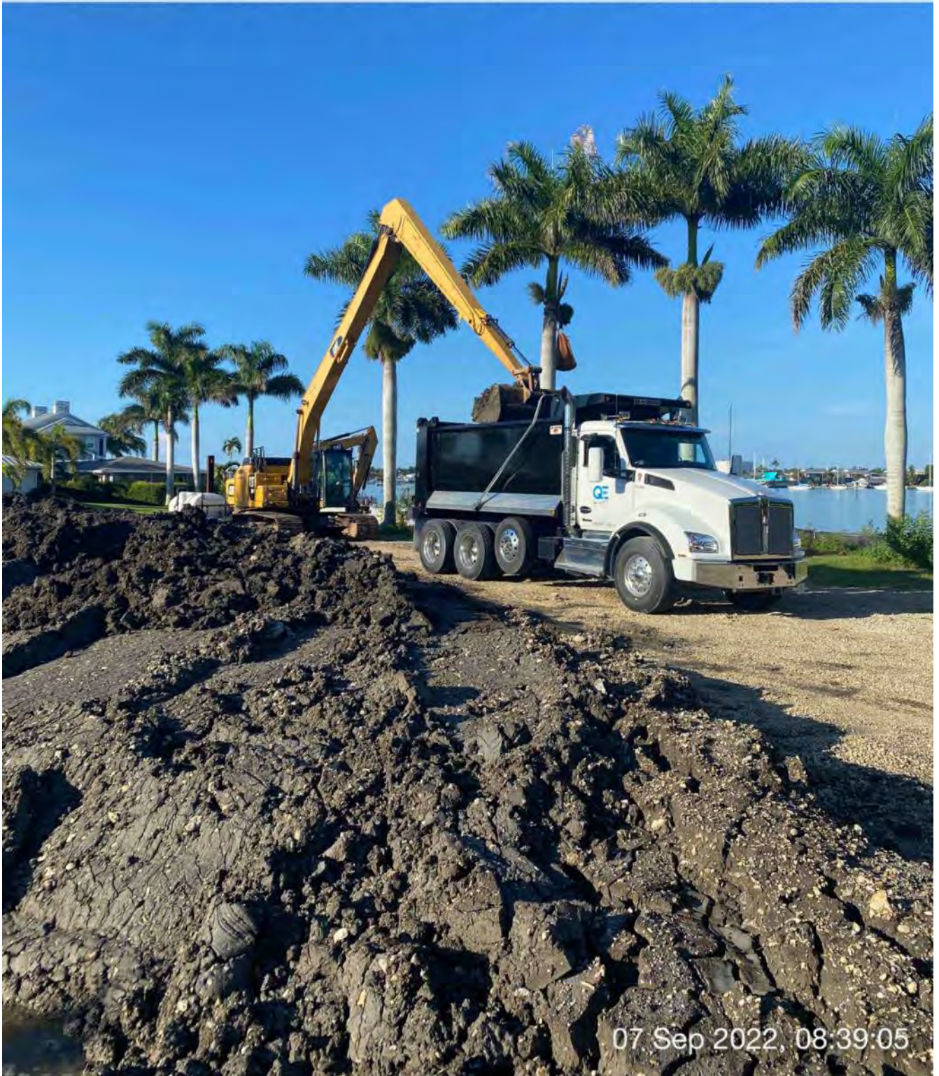
326 excavator transferring removed material form dewatering site to dump truck bed at 1300 Curlew Avenue
