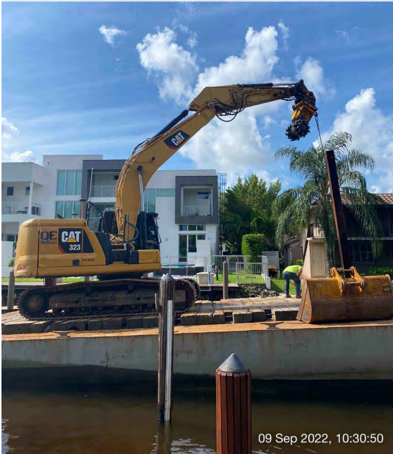
323 excavator lifting spud to allow push boat to mobilize barge at station 15+50
