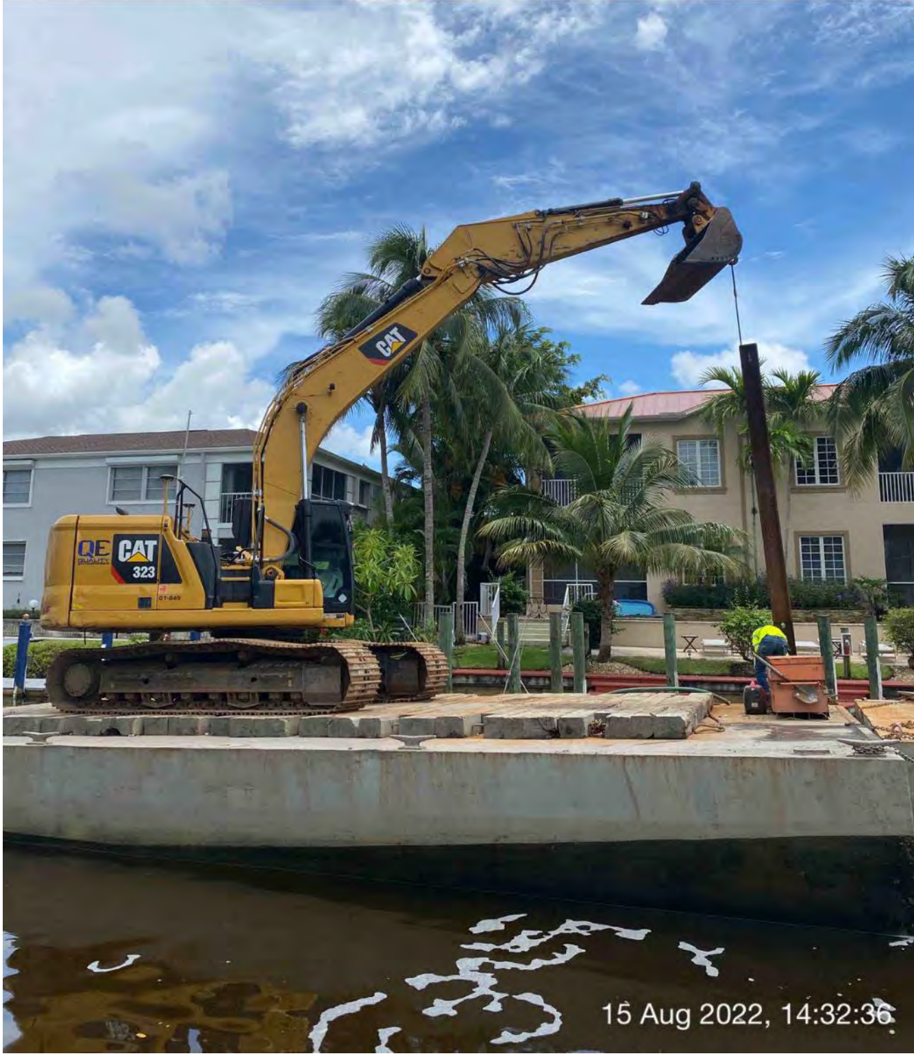
323 excavator lifting spud to allow push boat to mobilize barge at station 12+00
