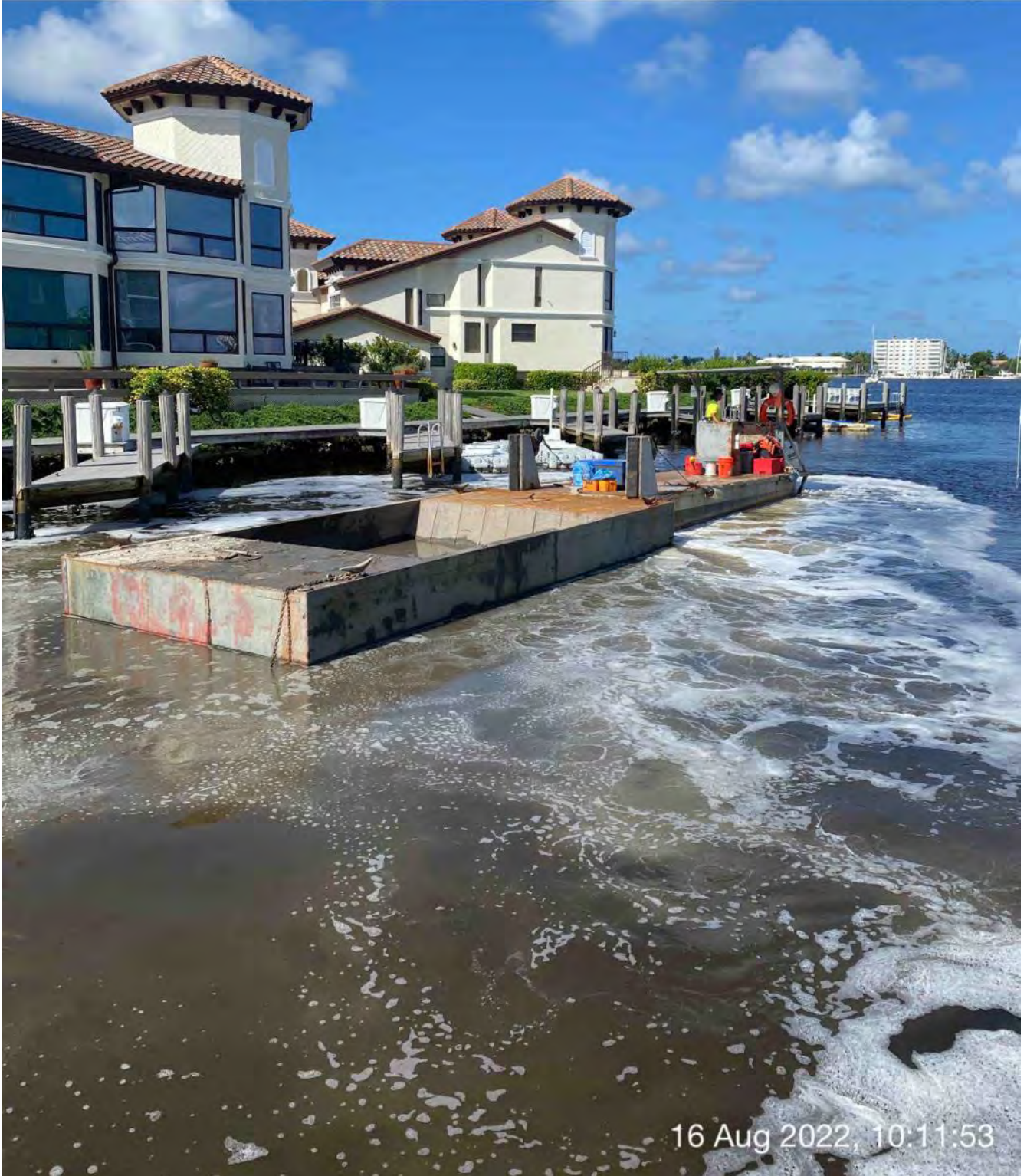
Push boat transporting full hopper of removed material from Canal W-W to Canal CC-CC
