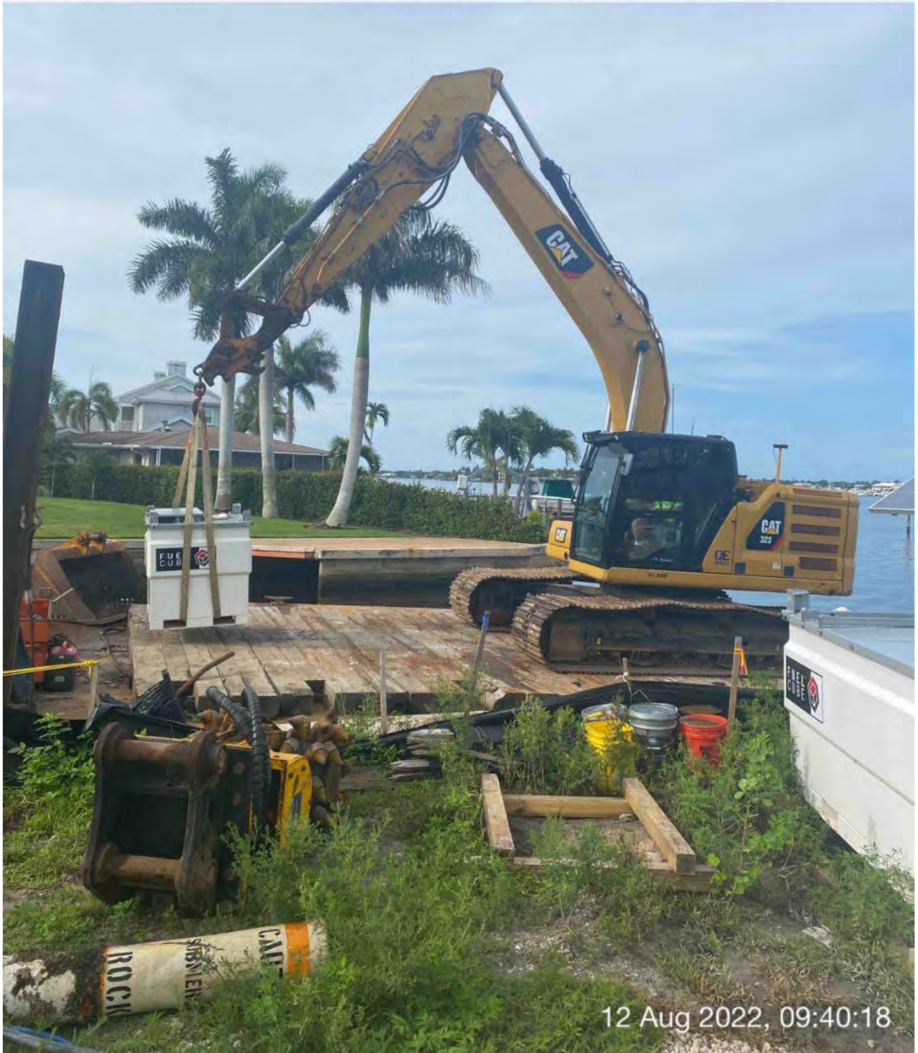
323 excavator lifting fuel cube from 1300 Curlew Avenue to barge to refuel 323 excavator
