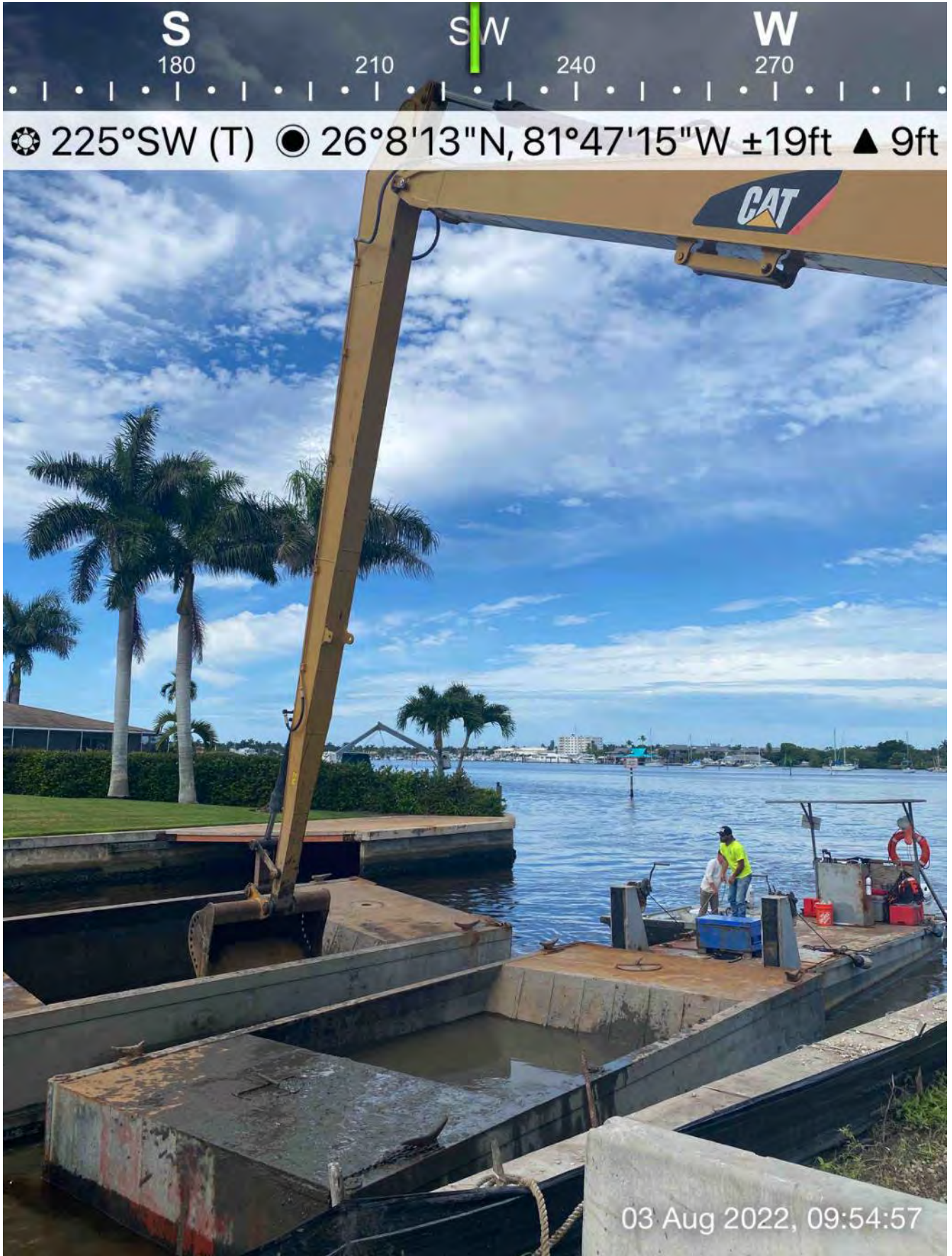
Push boat dropping off full hopper of removed material in Canal CC-CC
