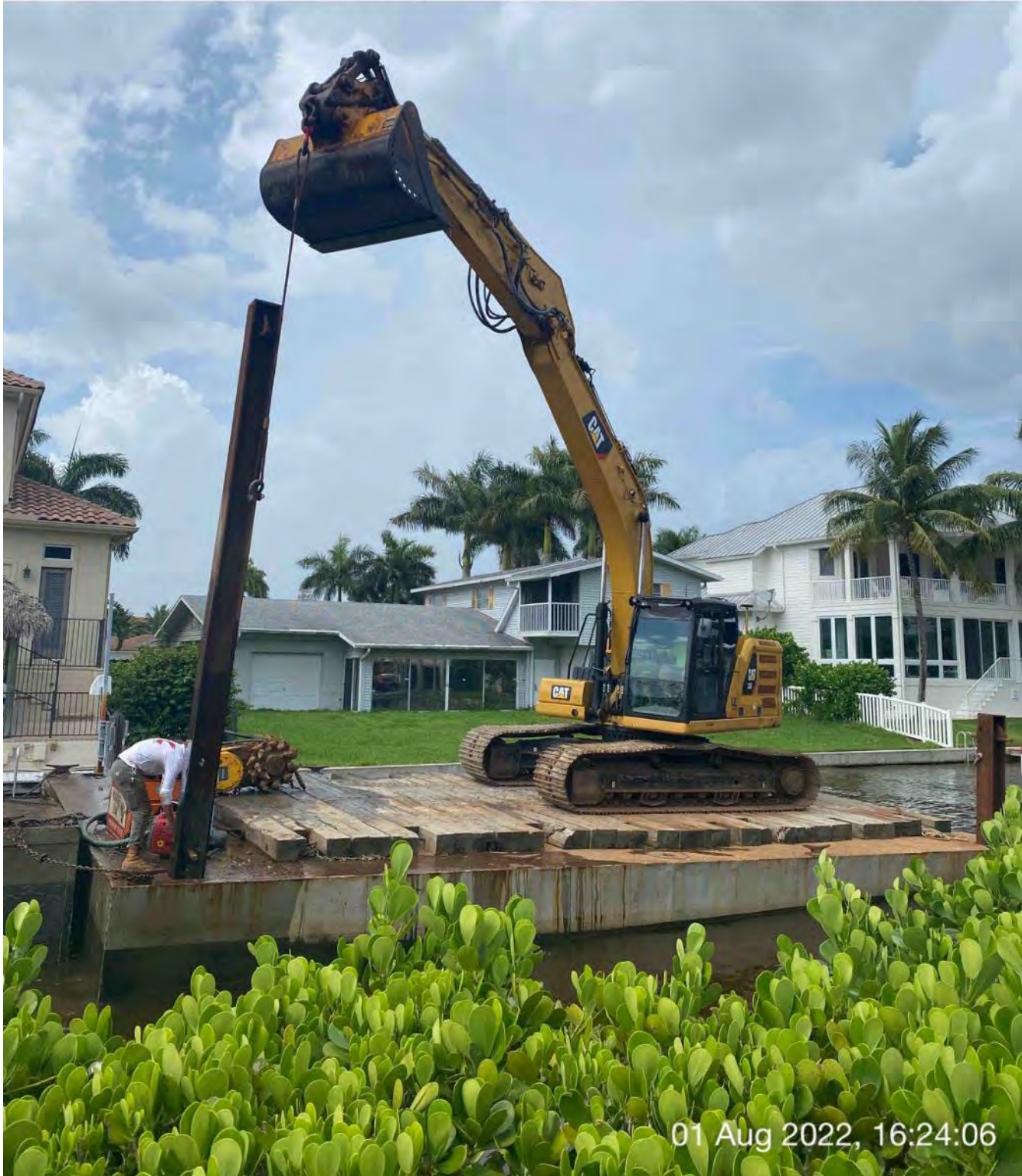
323 excavator lifting spud to allow push boat to mobilize barge at station 3+00
