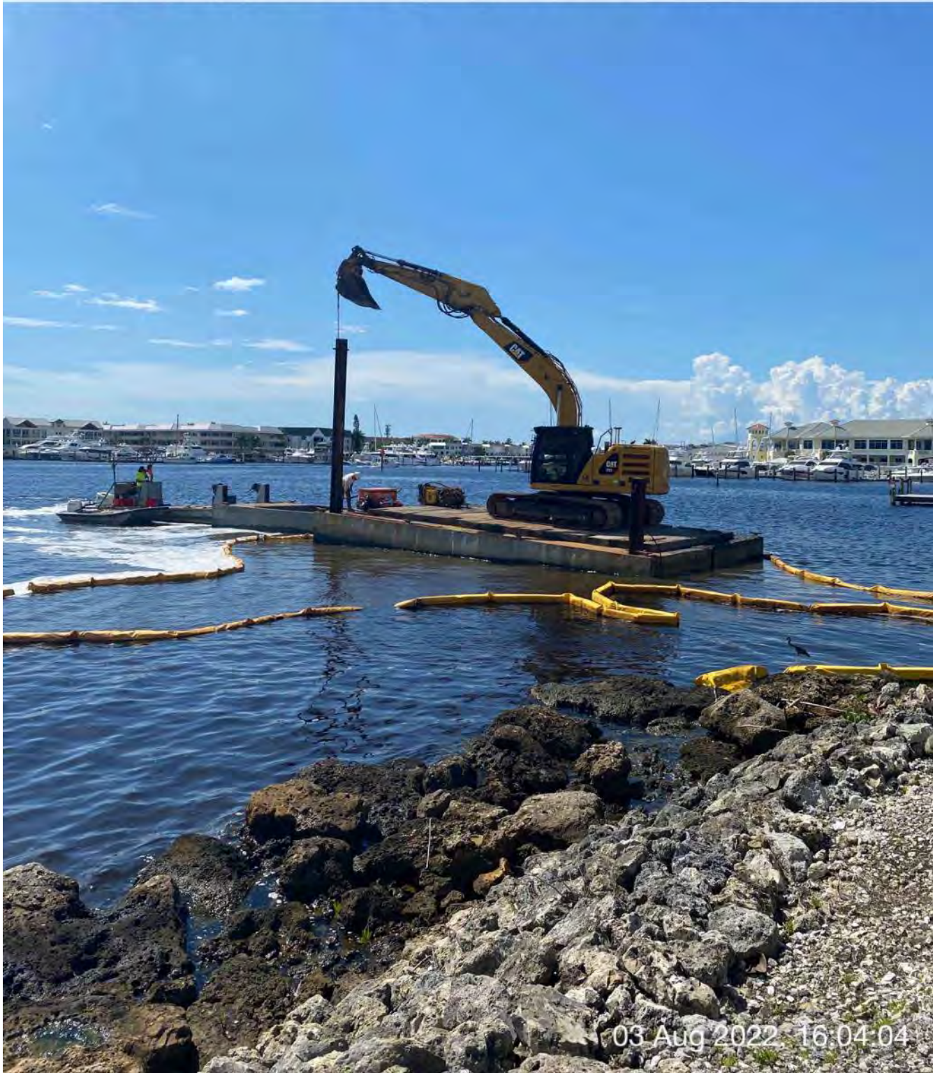
323 excavator lifting spud to allow push boat to mobilize barge at station 0+75
