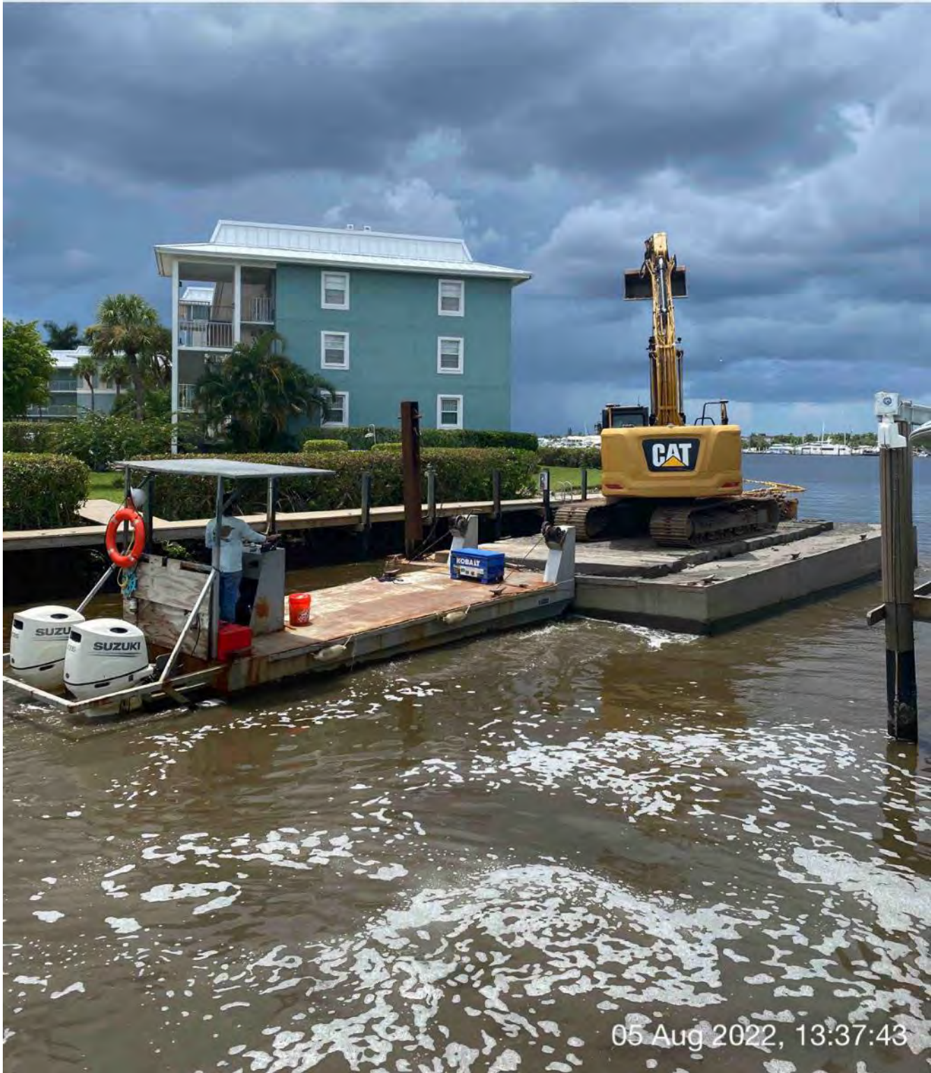
323 excavator lifting spud to allow push boat to mobilize barge at station 2+50
