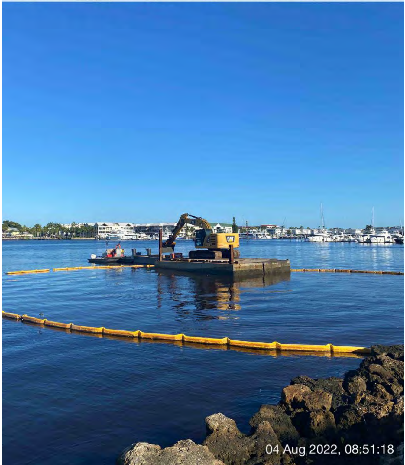
323 excavator removing material from station 0+50 and transferring to hopper in Canal BB-BB
