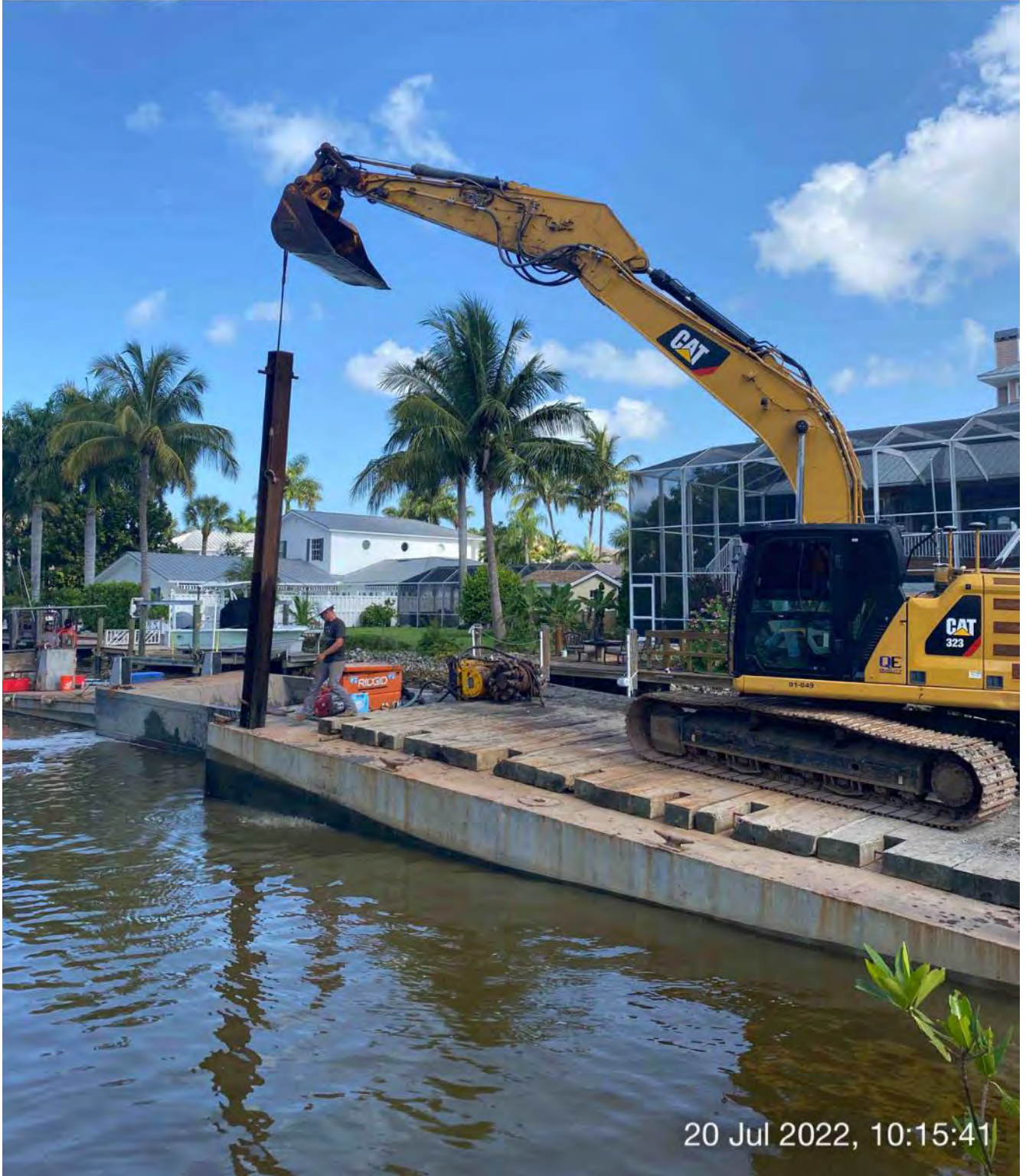
323 excavator lifting spud to allow push boat to mobilize barge at station 10+00
