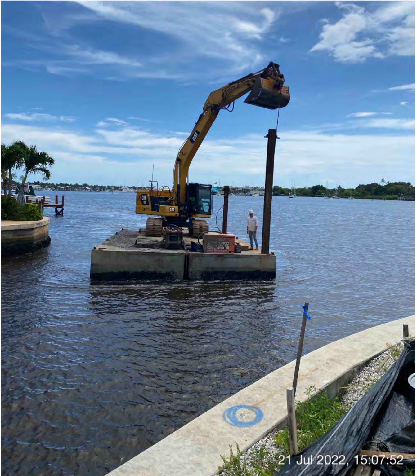
323 excavator lifting spud to allow push boat to transport barge from Canal BB-BB to Canal CC-CC
