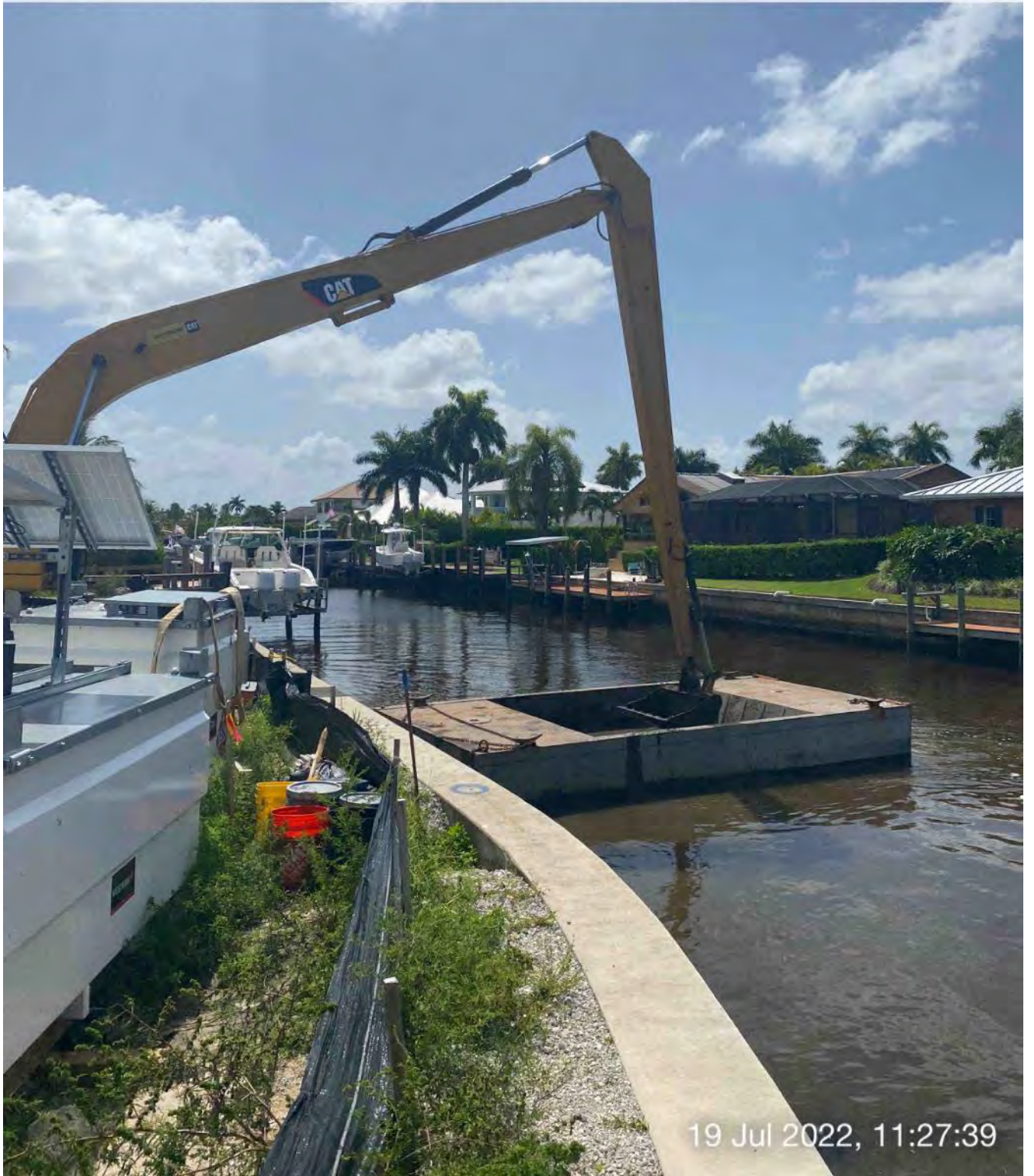
326 excavator transporting removed material from hopper to dewatering site at 1300 Curlew Avenue
