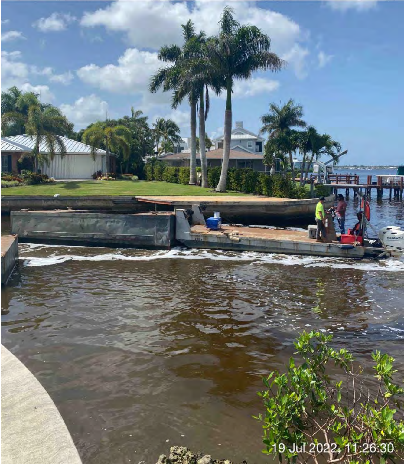
Push boat transporting empty hopper of material from Canal BB-BB to Canal CC-CC
