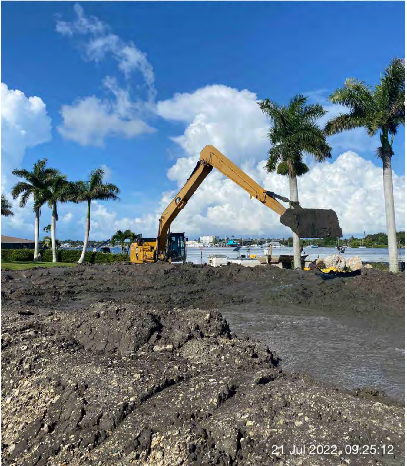
326 excavator transporting removed material from hopper to dewatering site at 1300 Curlew Avenue
