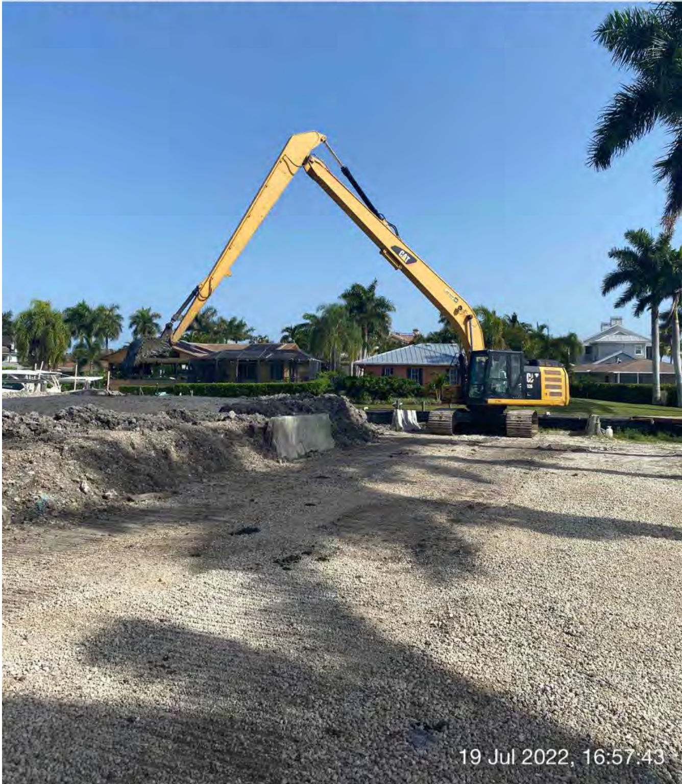
326 excavator transporting removed material from hopper to dewatering site at 1300 Curlew Avenue
