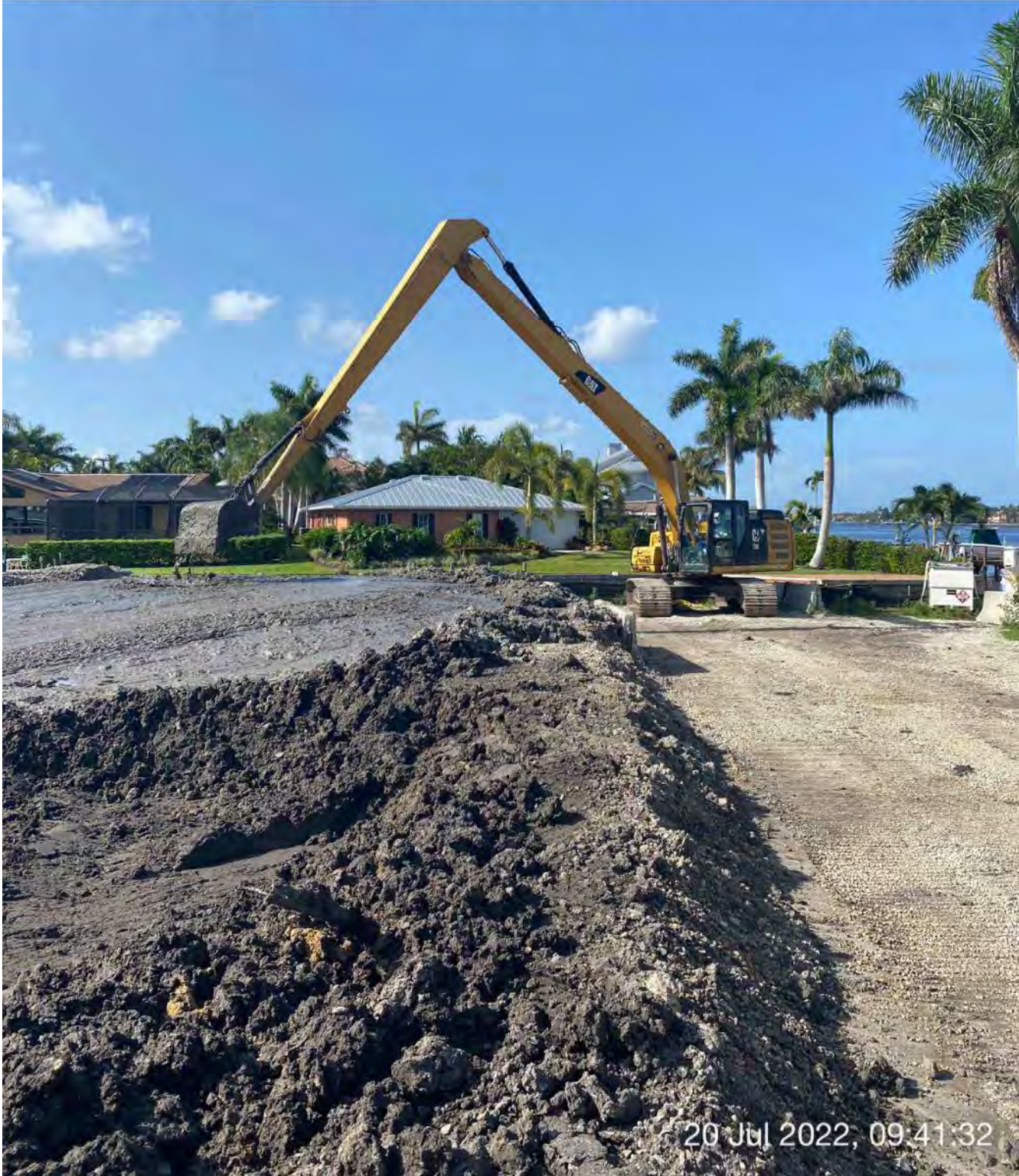
326 excavator transporting removed material from hopper to dewatering site at 1300 Curlew Avenue
