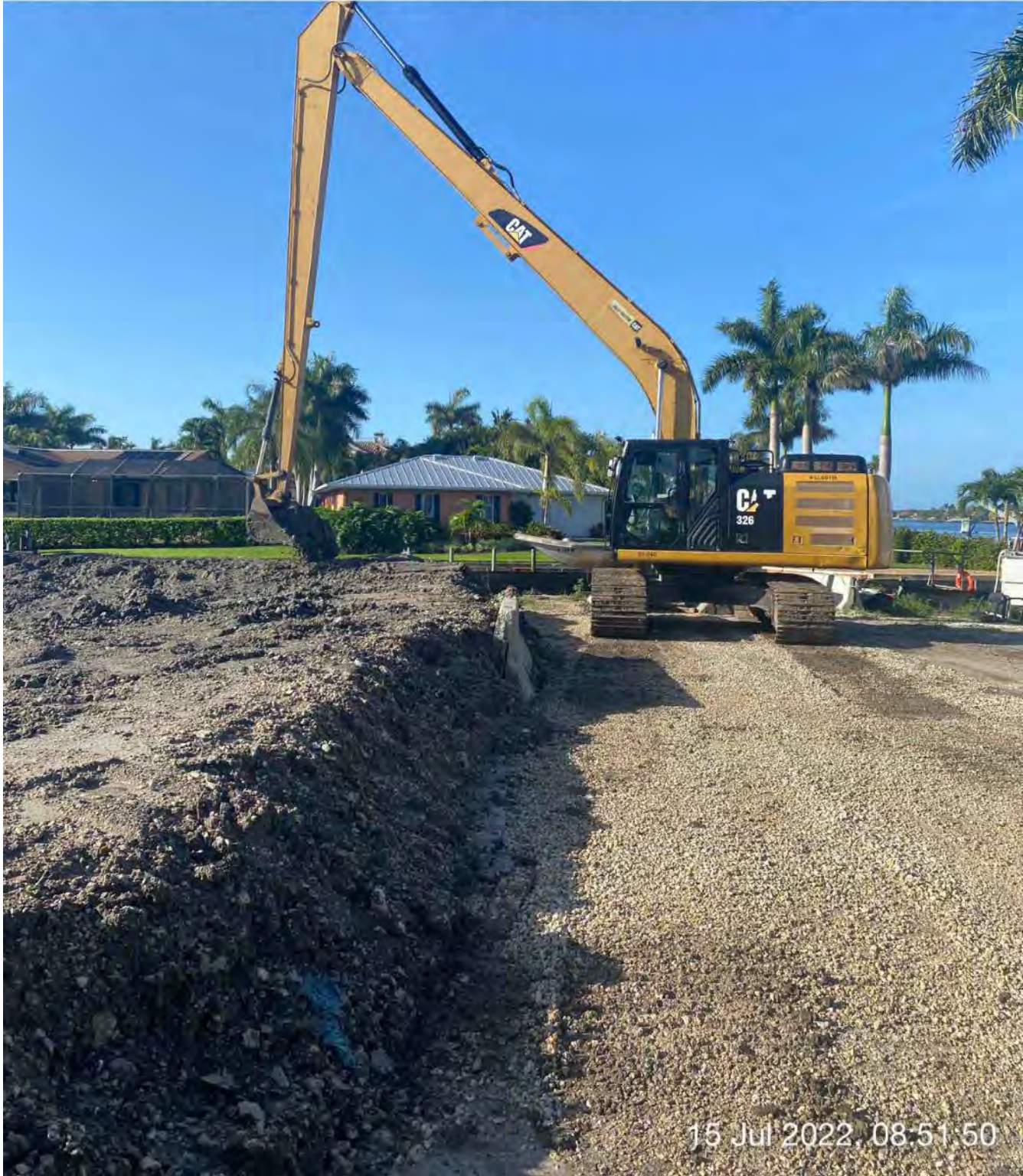
326 excavator transferring removed material from hopper to dewatering site at 1300 Curlew Avenue
