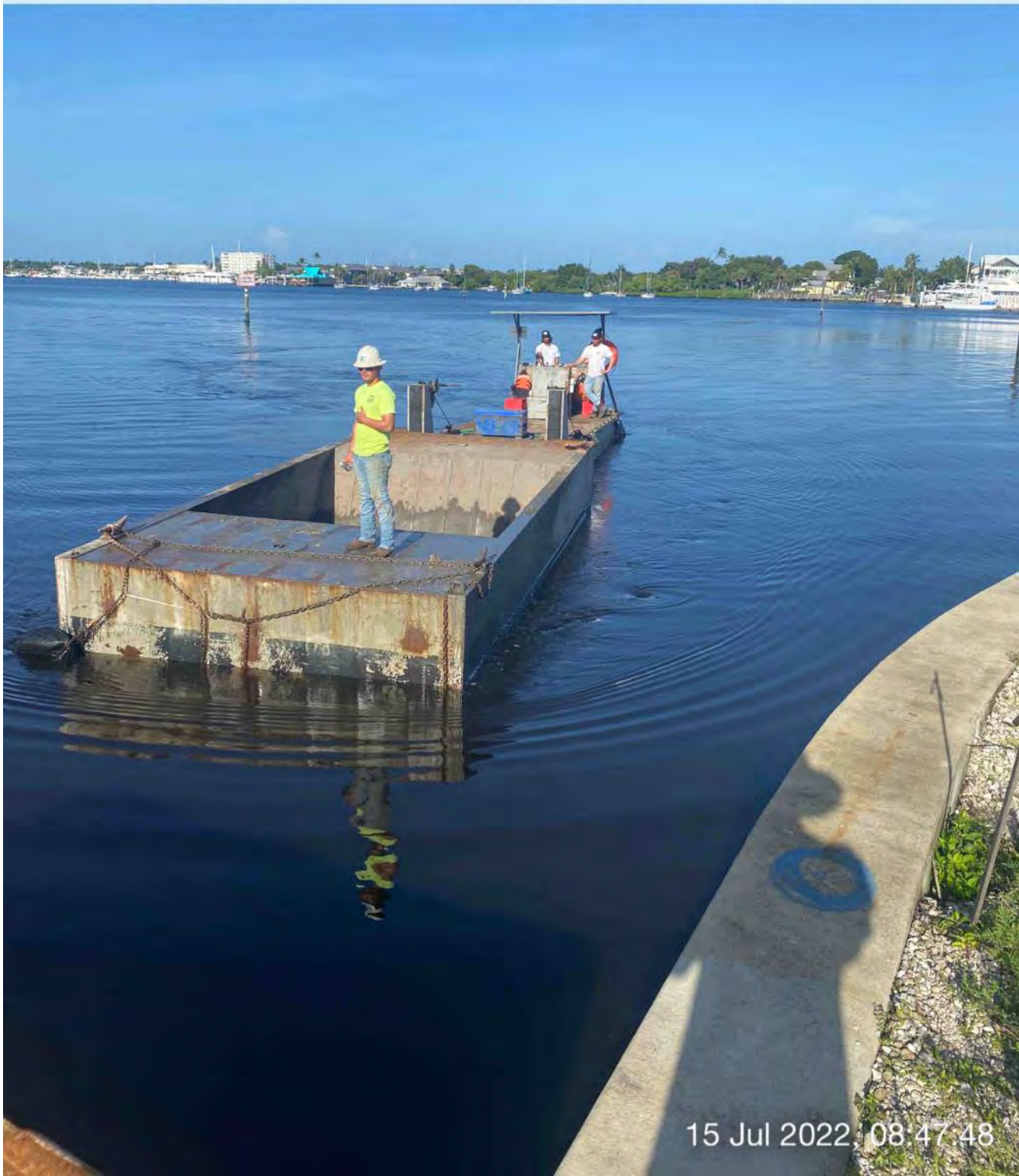
Push boat transporting full hopper of removed material from Canal X-X to Canal CC-CC
