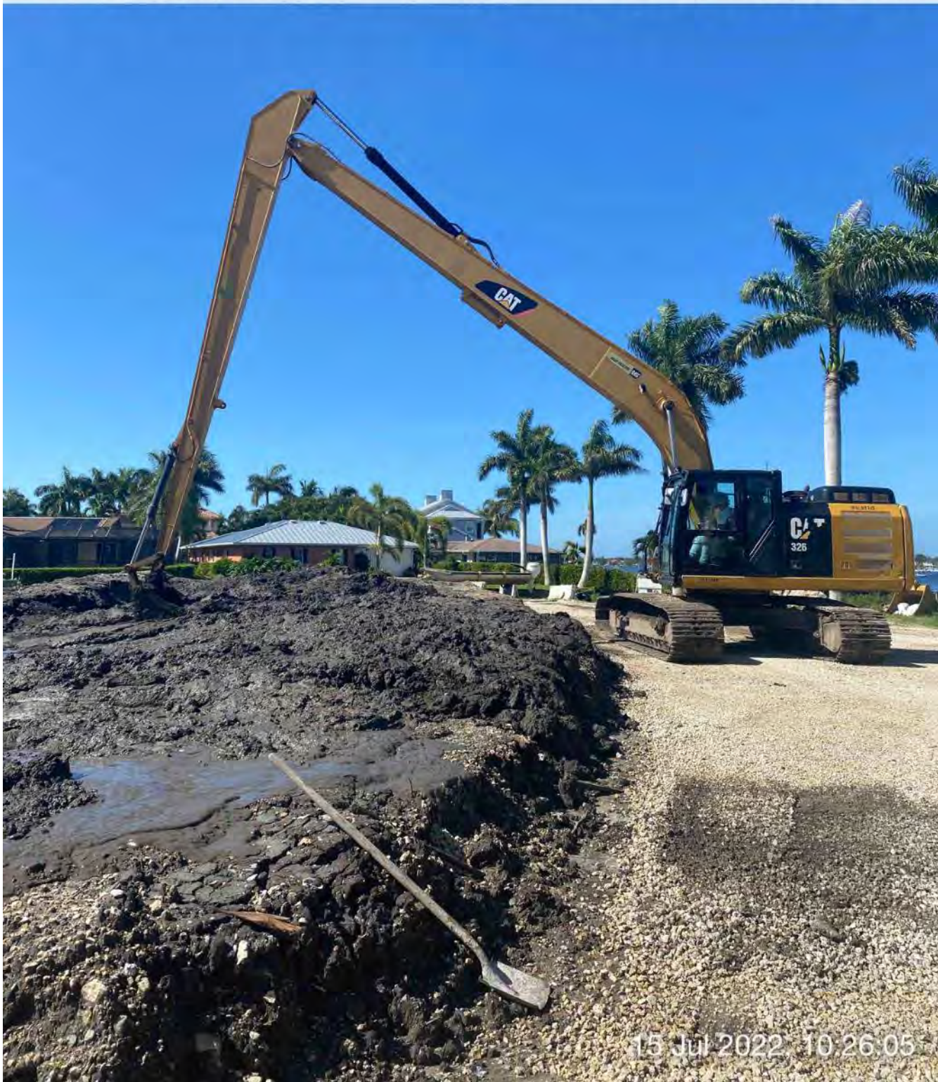
326 excavator transferring removed material from hopper to dewatering site at 1300 Curlew Avenue
