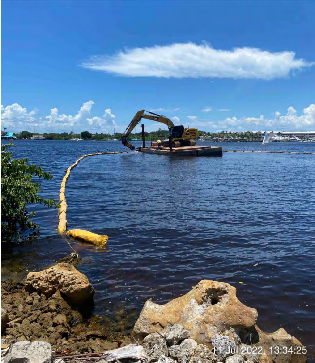
Contractor pumping water out of the bottom of the barge at station 0+00
