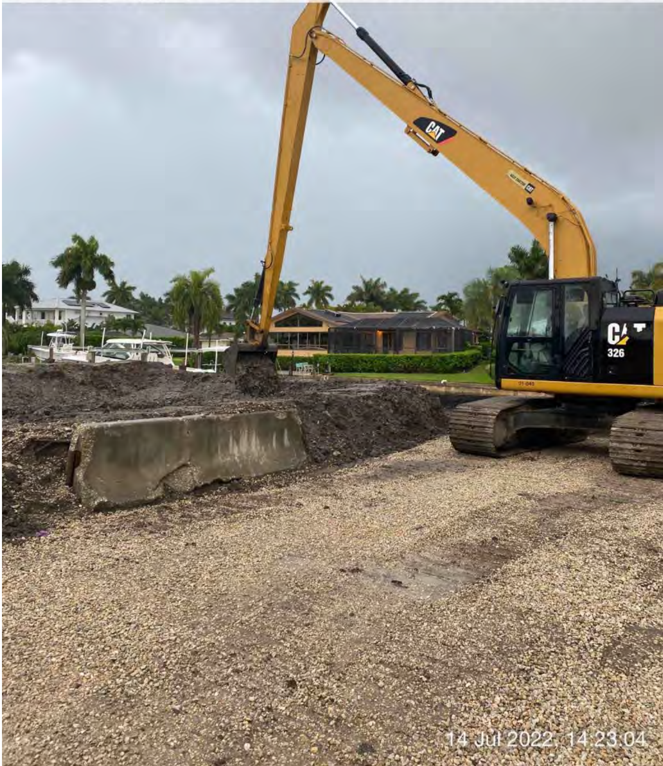
326 excavator transferring removed material from hopper to dewatering site at 1300 Curlew Avenue
