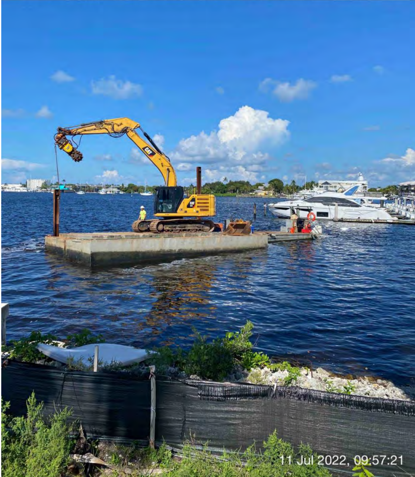
323 excavator lifting spud to allow push boat to transport barge from Canal CC-CC to Canal X-X
