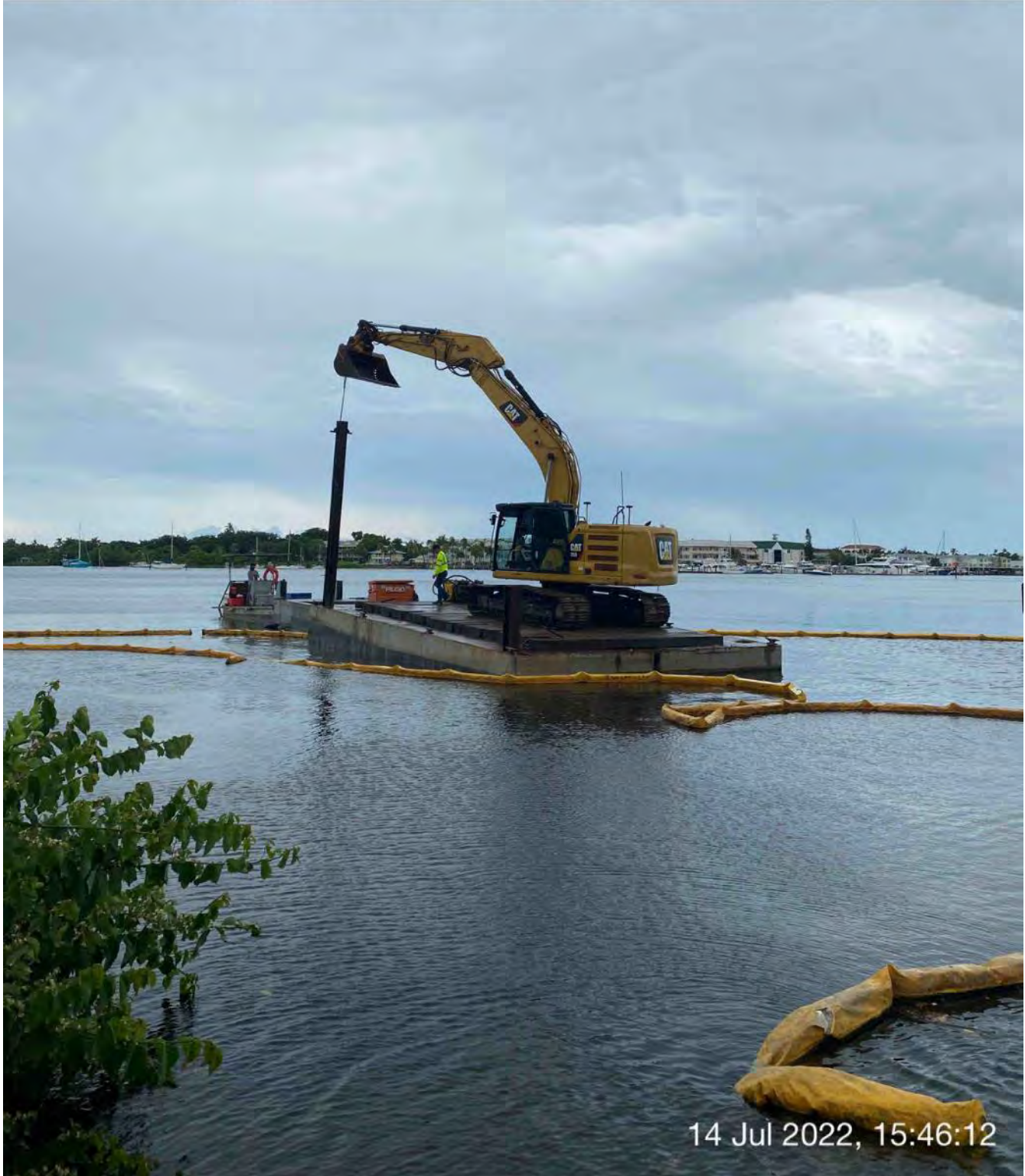
323 excavator lifting spud to allow push boat to mobilize barge at station 0+50
