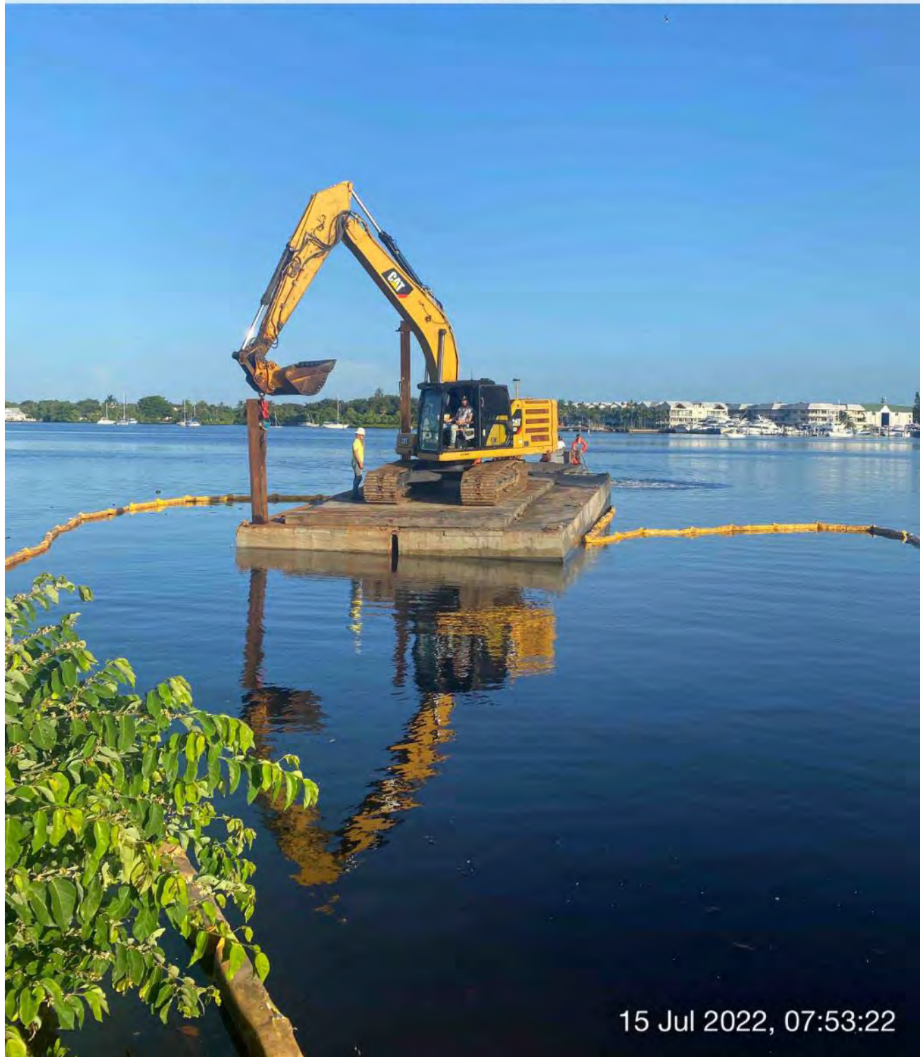
323 excavator lifting spud to allow push boat to mobilize barge at station 0+50
