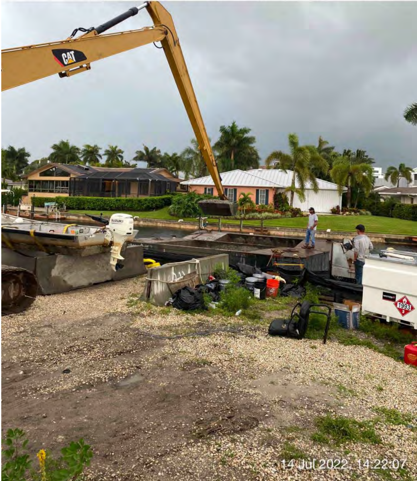
326 excavator transferring removed material from hopper to dewatering site at 1300 Curlew Avenue
