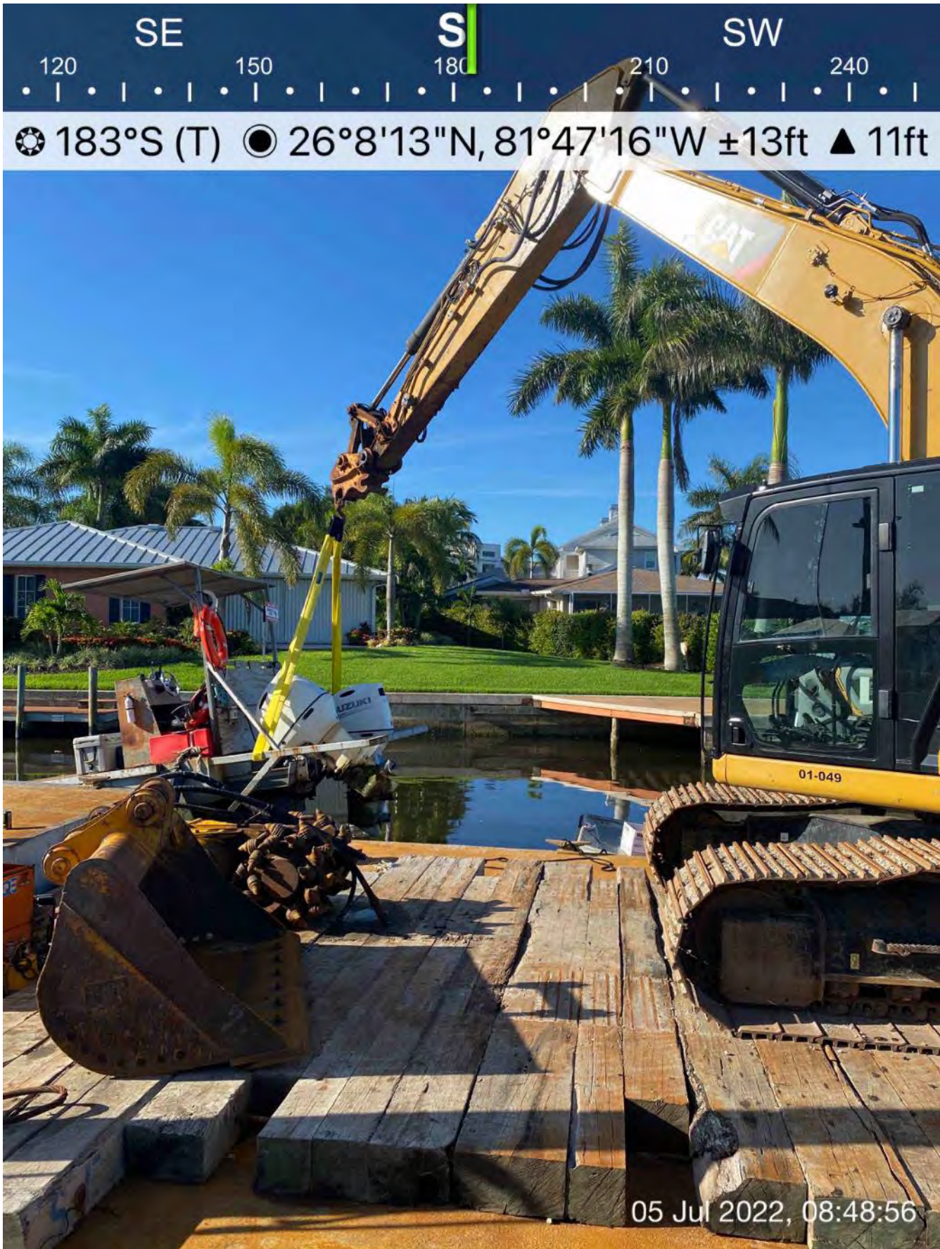
323 excavator lifting push boat to allow contractor to change oil on the lower section of the boat motors
