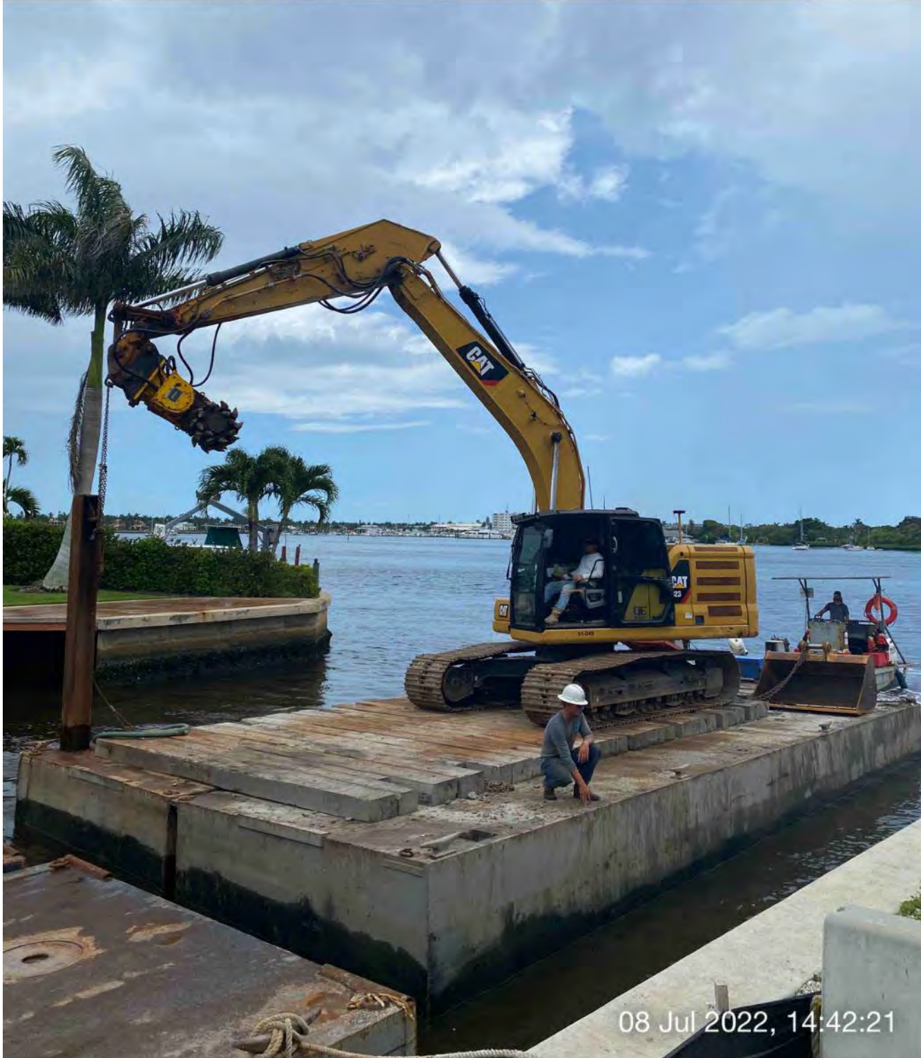
323 excavator lifting spud to allow push boat to transport barge from Canal X-X to Canal CC-CC
