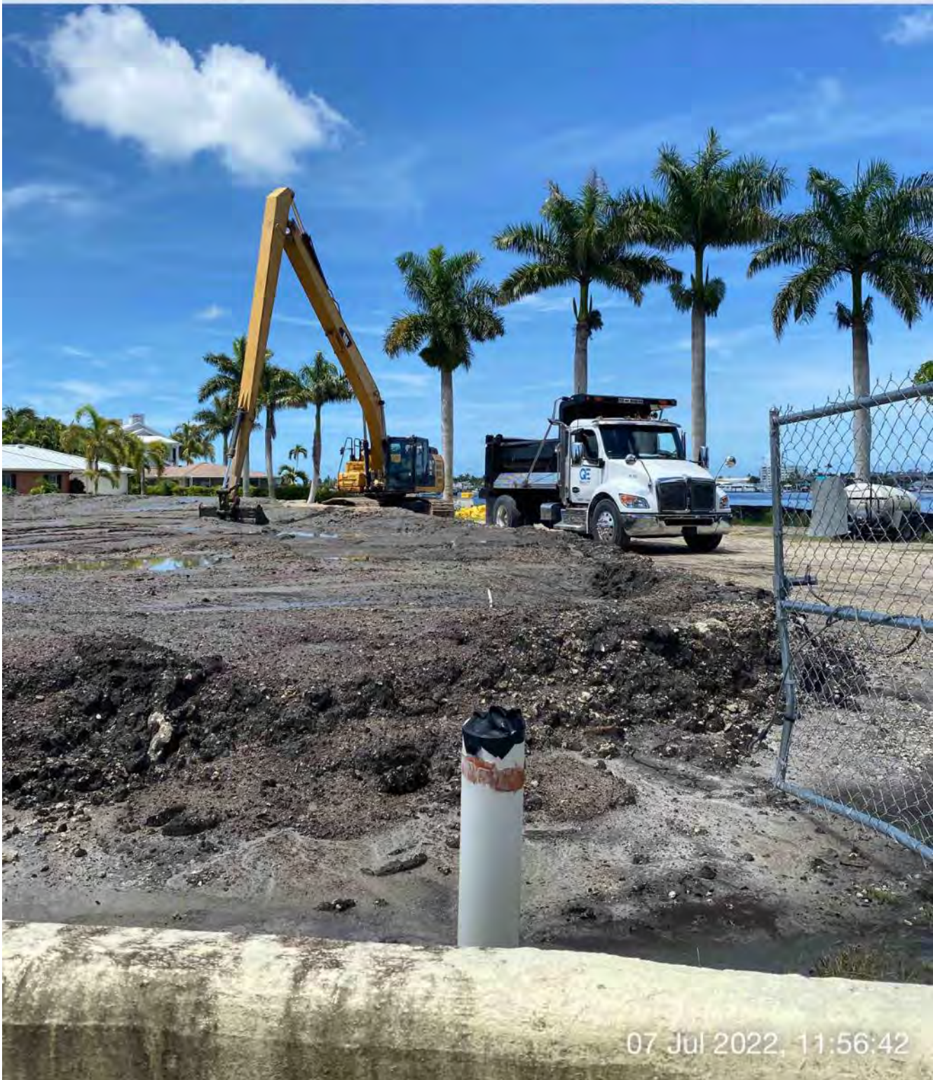
326 excavator transferring removed material from dewatering site to dump truck bed at 1300 Curlew Avenue
