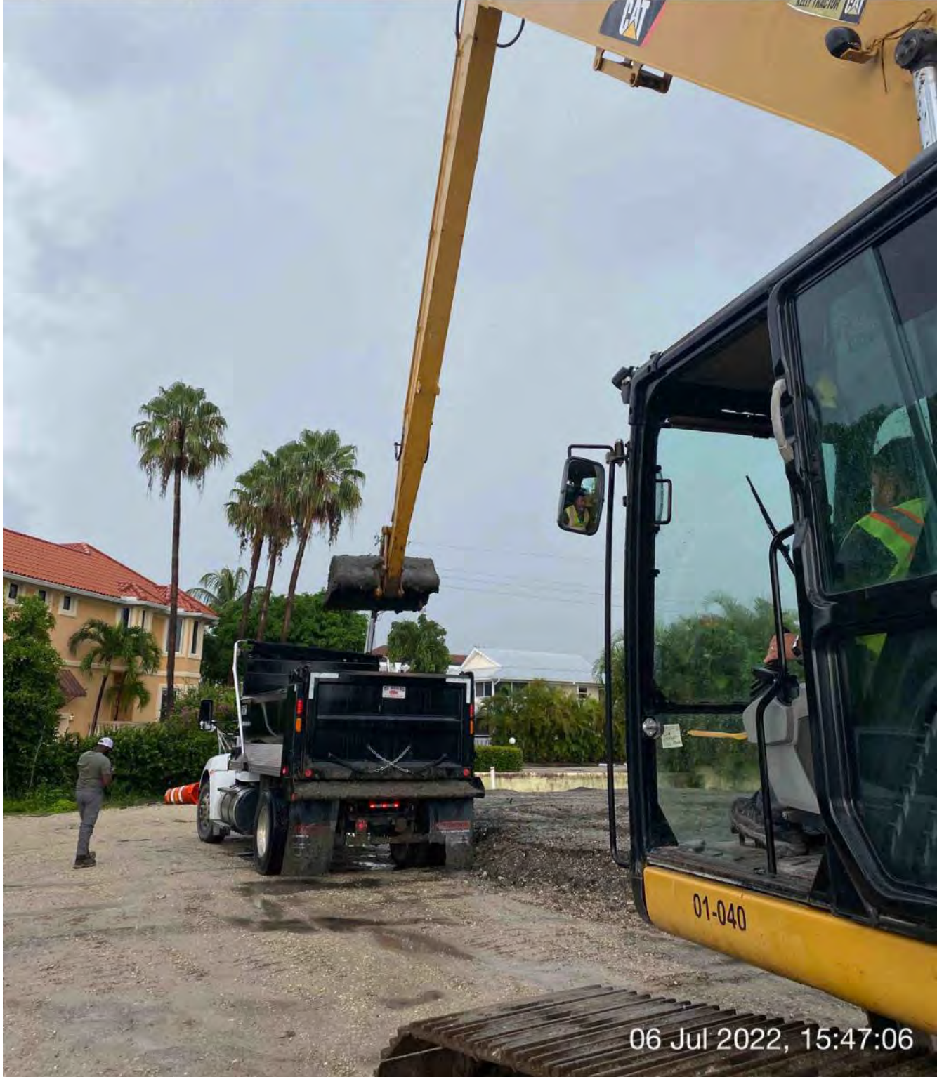
326 excavator transferring removed material from dewatering site to dump truck bed at 1300 Curlew Avenue
