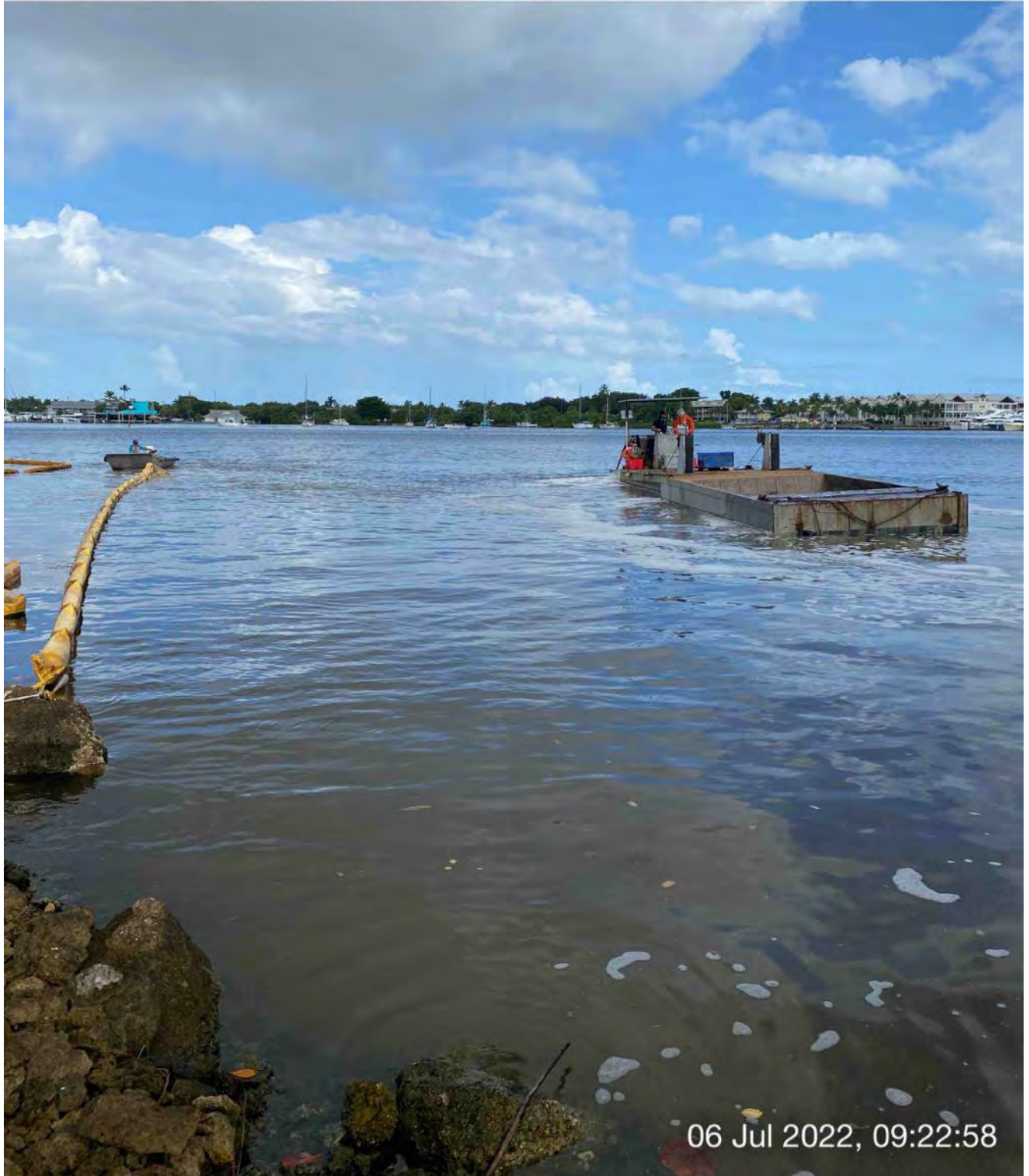
Support boat holding open turbidity curtain to allow push boat to transport full hopper of material to Canal CC-CC
