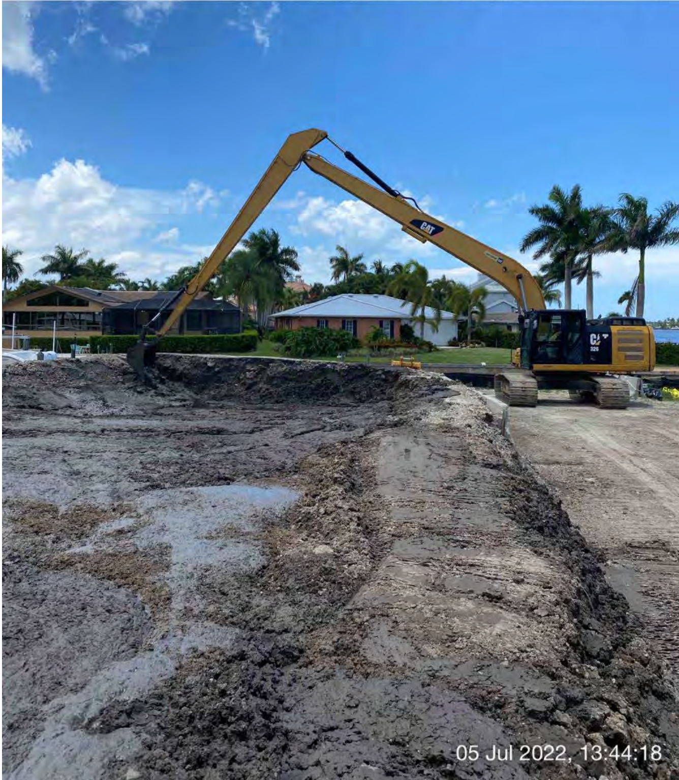
326 excavator transferring removed material from dewatering site to dump truck bed at 1300 Curlew Avenue
