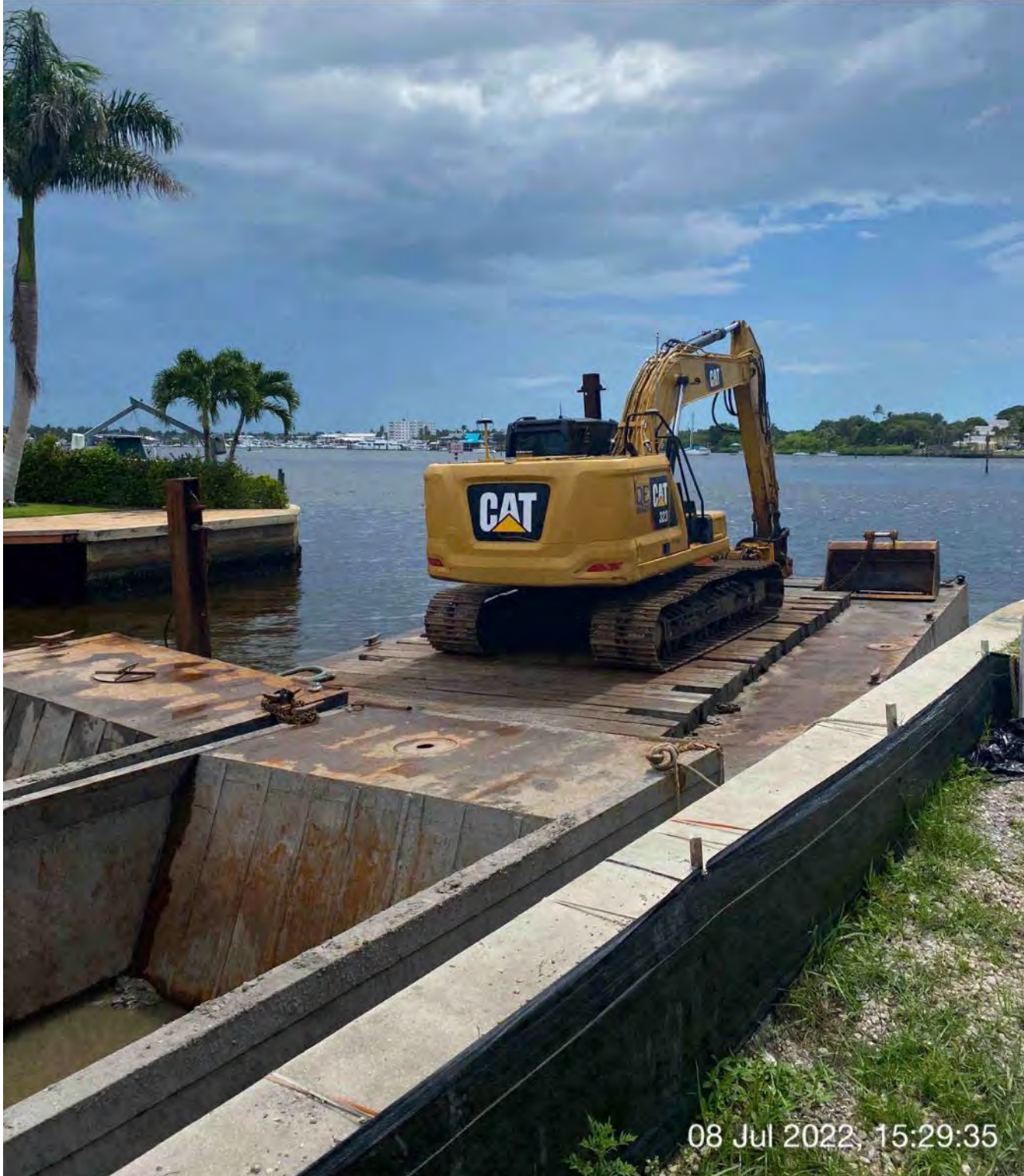
Hoppers, barge, and 323 excavator staged in Canal CC-CC between stations 1+00 and 2+00 for the weekend
