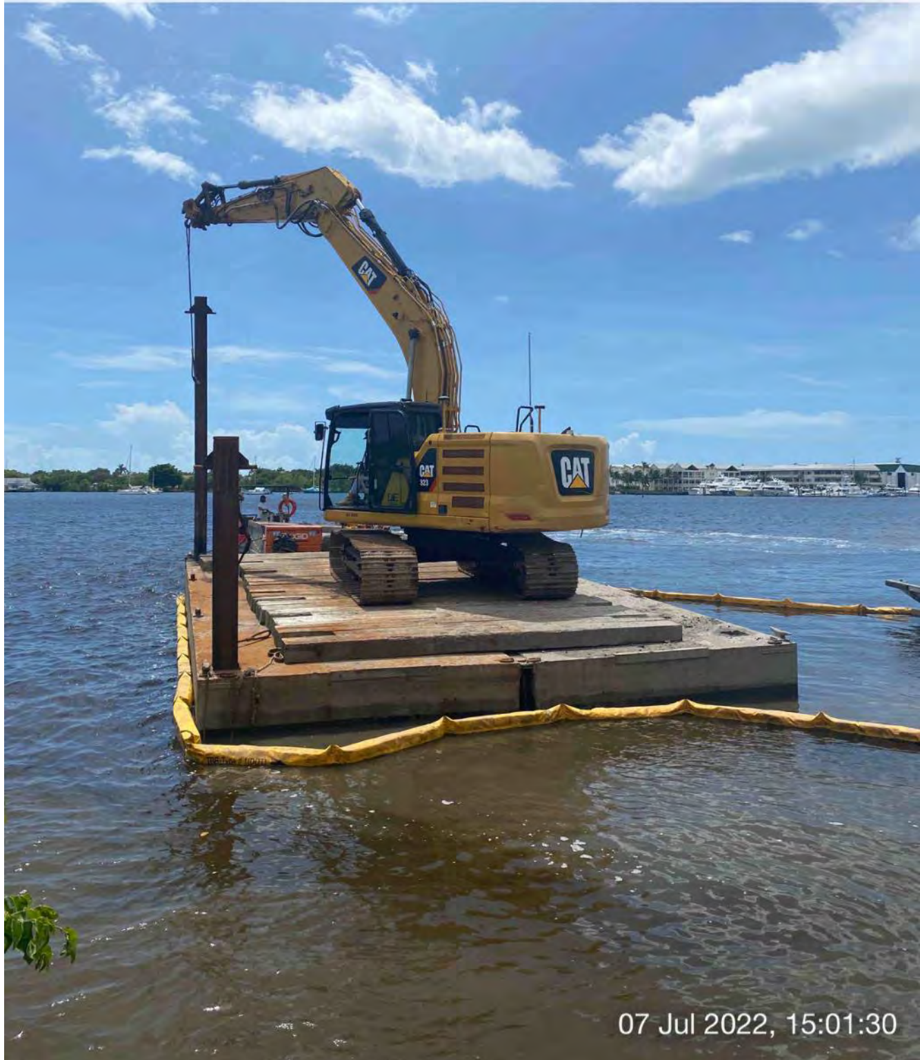
323 excavator lifting spud to allow push boat to mobilize barge outside of Canal X-X
