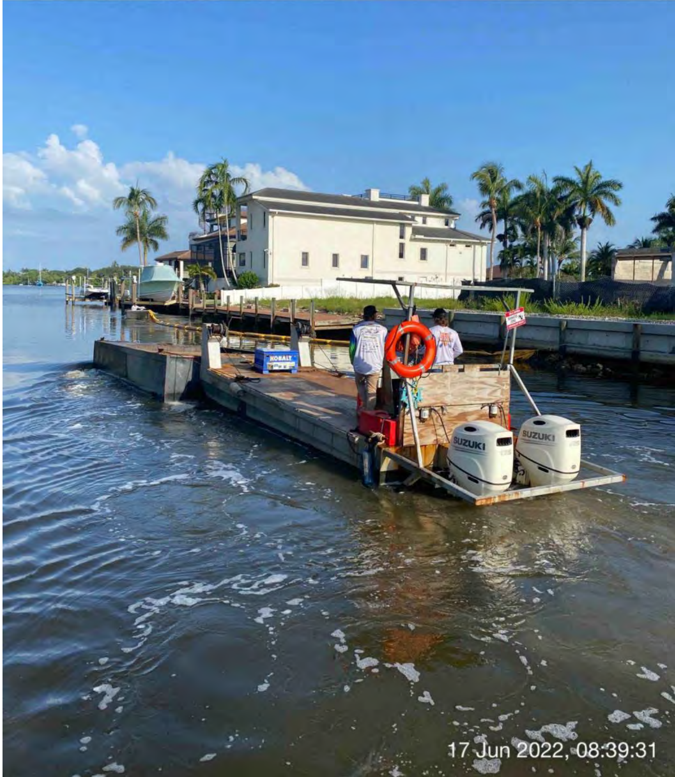
Support boat opening turbidity curtain to allow push boat to transport full hopper from Canal X-X to Canal CC-CC
