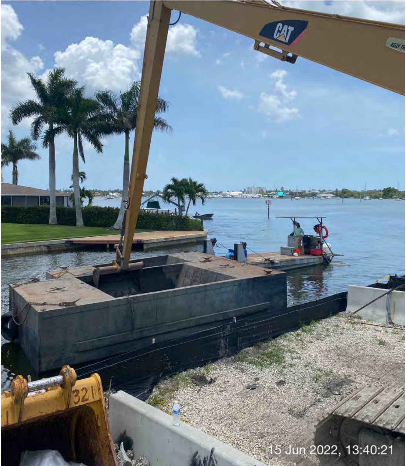
Push boat dropping off full hopper of material in Canal CC-CC at station 1+50
