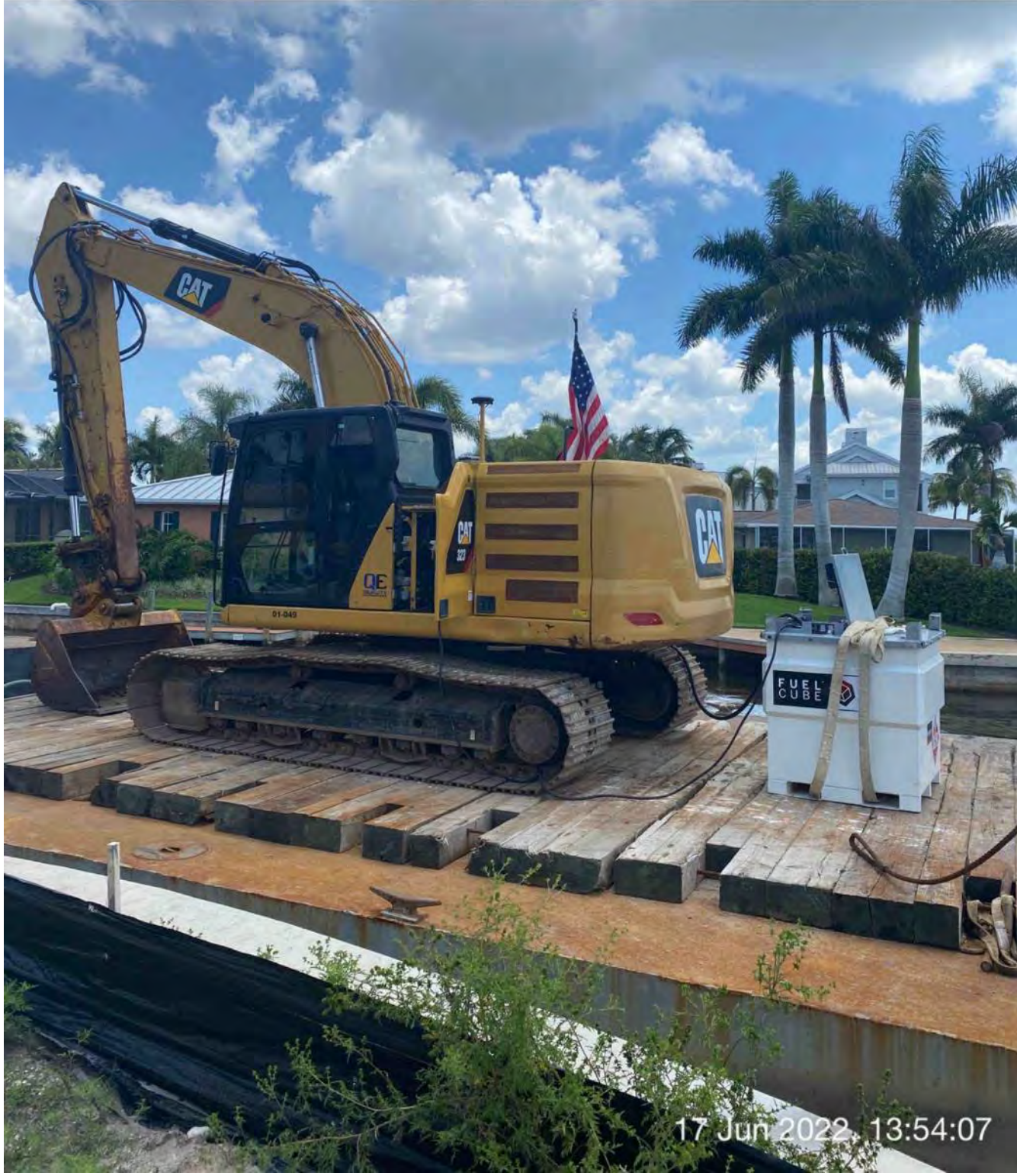
Small fuel cube being used to refuel 323 excavator on barge at station 1+25 in Canal CC-CC
