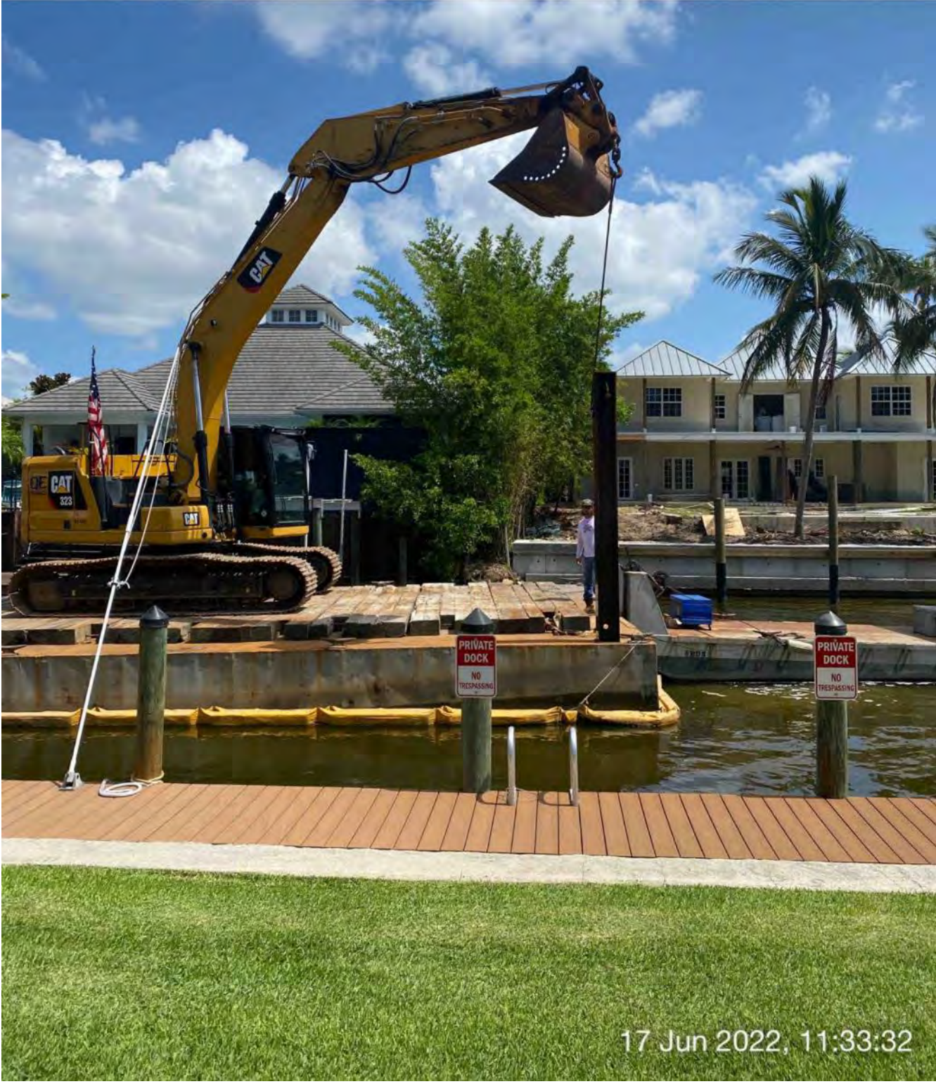
323 excavator lifting spud to allow push boat to mobilize barge at station 7+00
