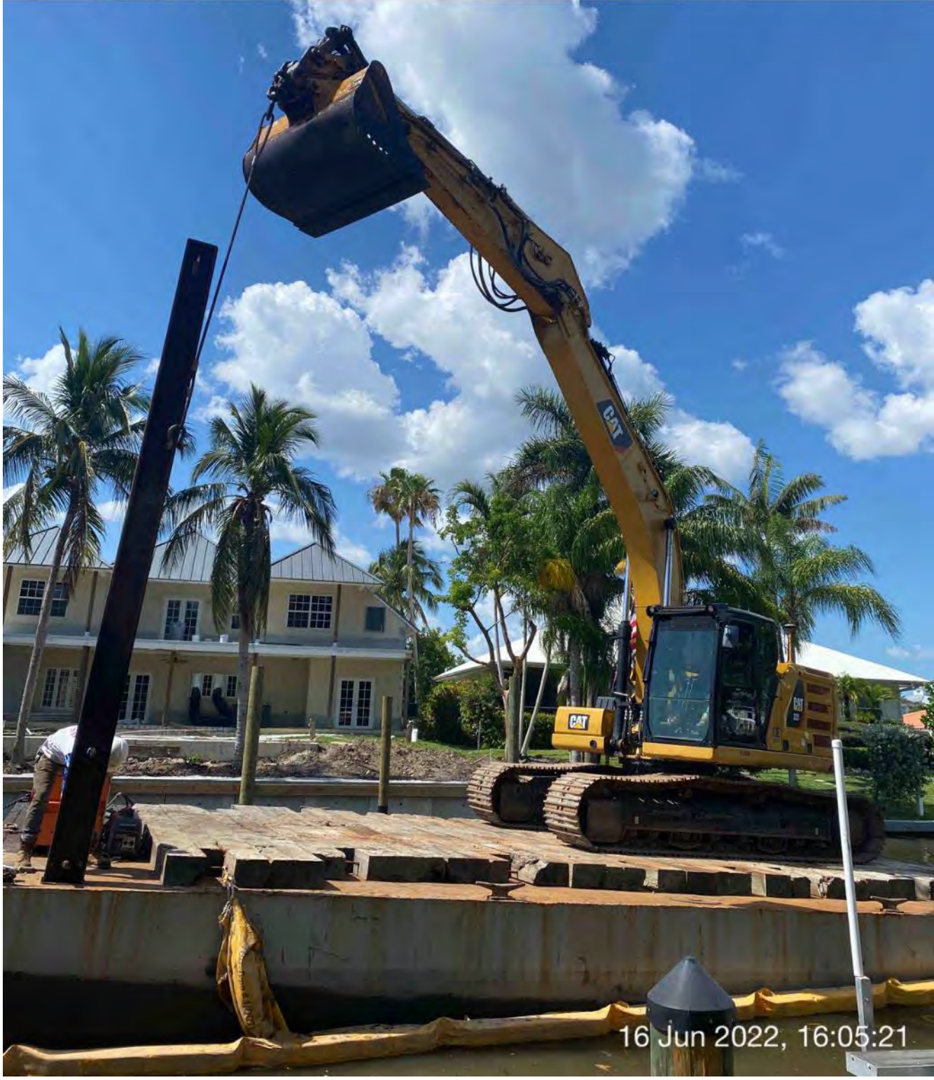
323 excavator lifting spud to allow push boat to mobilize barge at station 7+75
