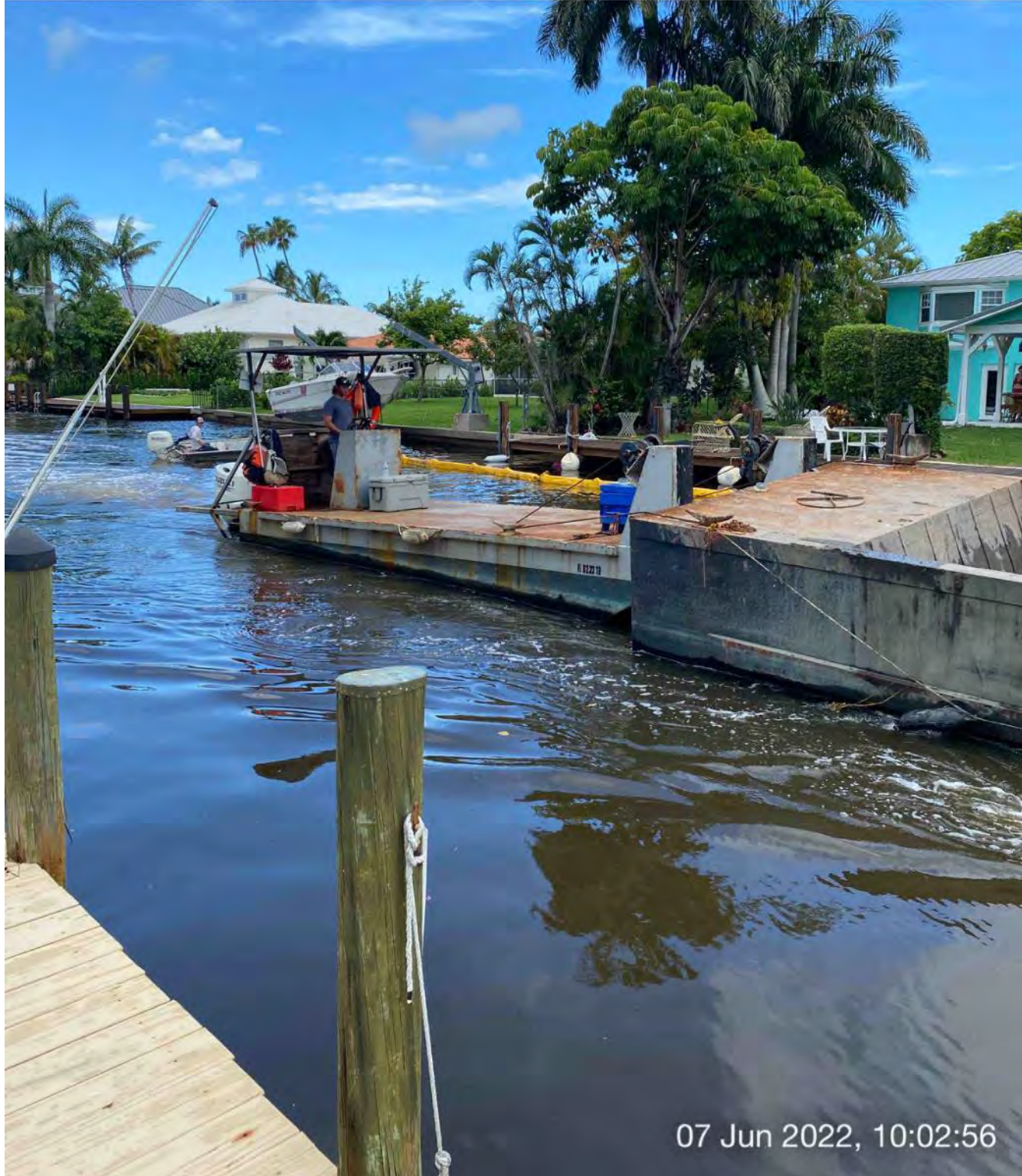
Support boat being used to open turbidity curtain to allow push boat to transport full hopper back to Canal CC-CC
