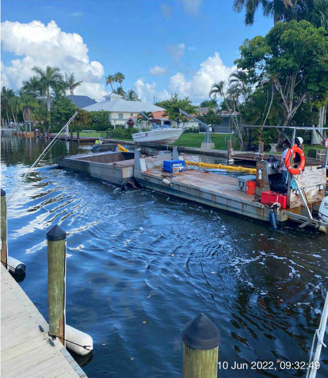
Support boat being used to open turbidity curtain to allow push boat to transport full hopper back to Canal CC-CC
