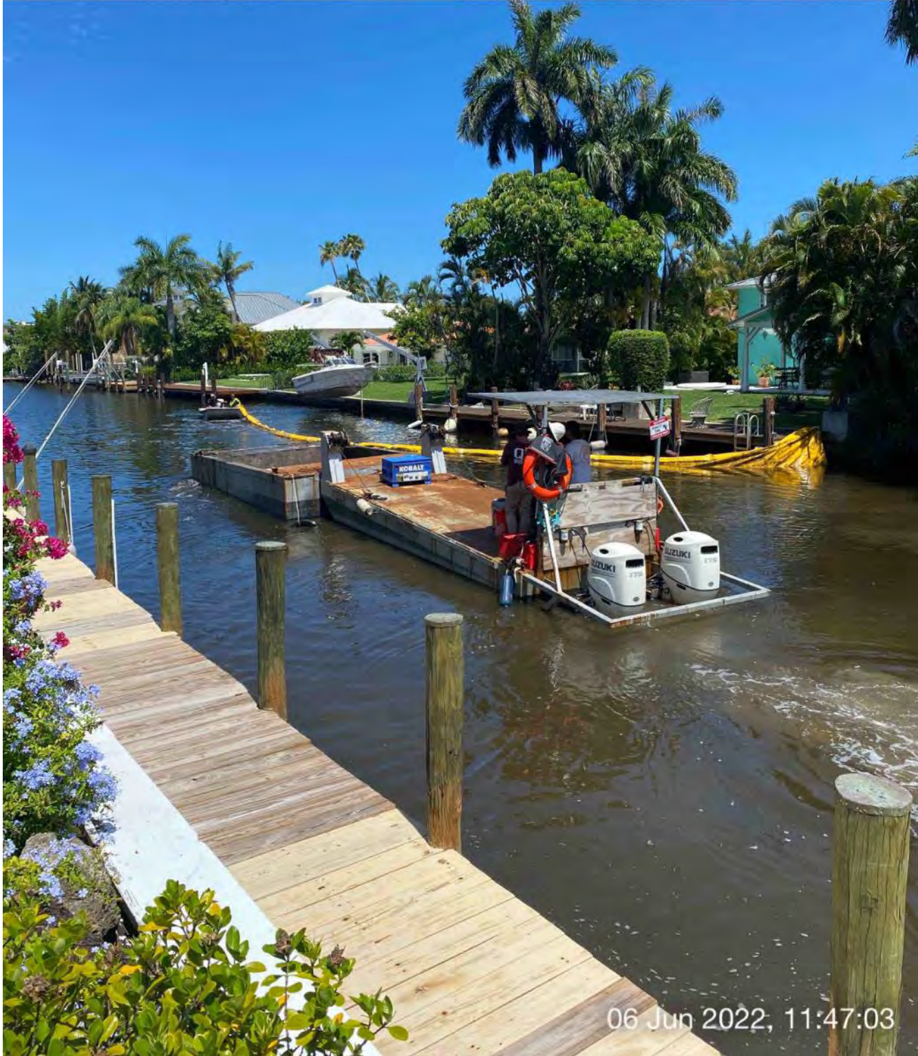
Support boat being used to open turbidity curtain to allow push boat to transport full hopper back to Canal CC-CC
