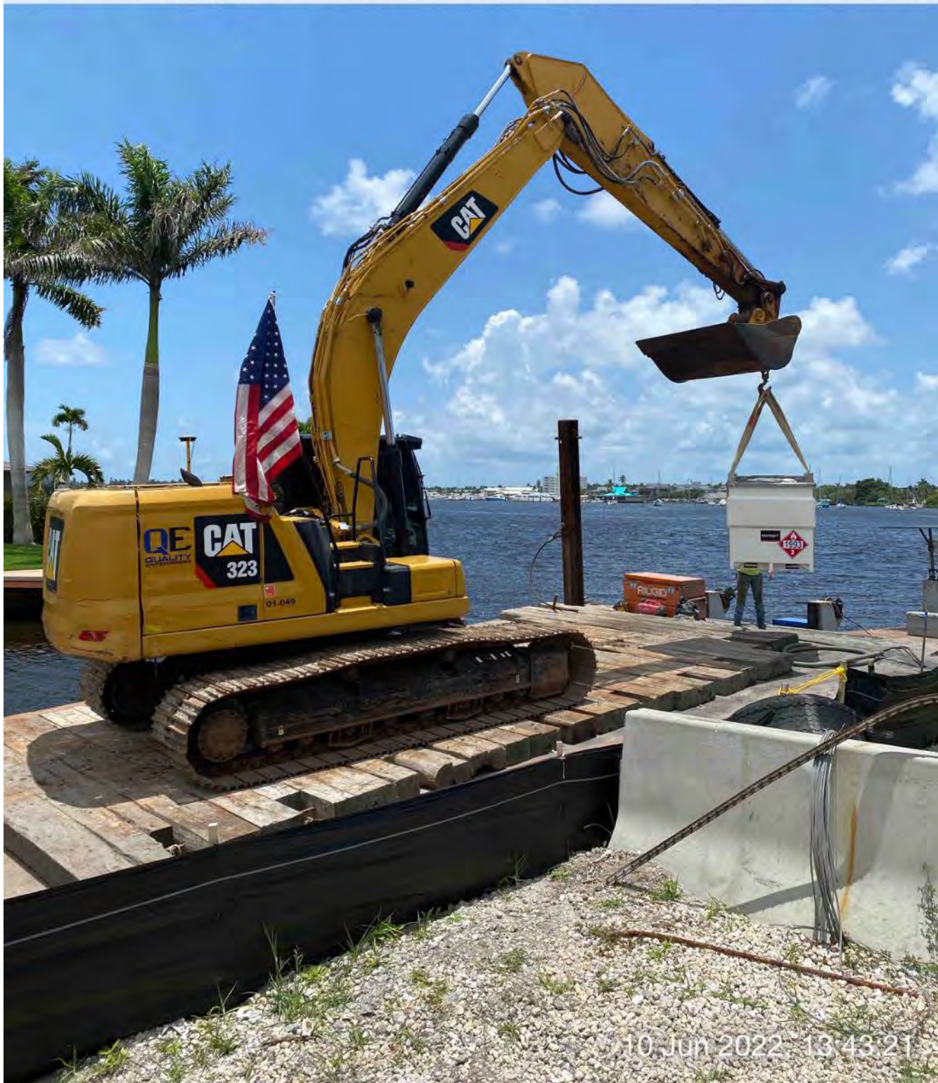
323 excavator transferring small fuel cube from southwest corner of 1300 Curlew Avenue to barge for refueling
