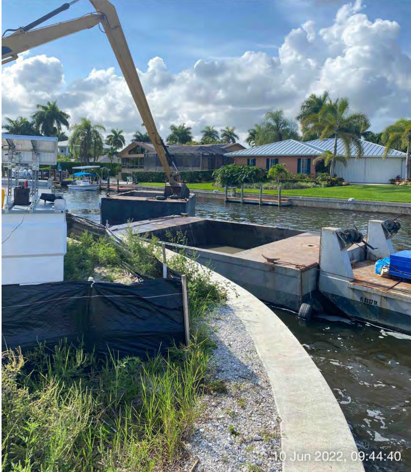
Push boat dropping off full hopper of material and picking up empty hopper of material in Canal CC-CC
