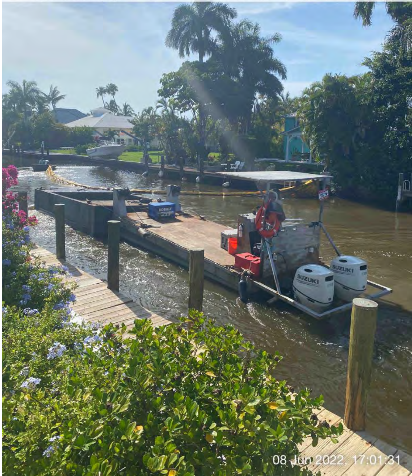
Support boat being used to open turbidity curtain to allow push boat to transport full hopper back to Canal CC-CC
