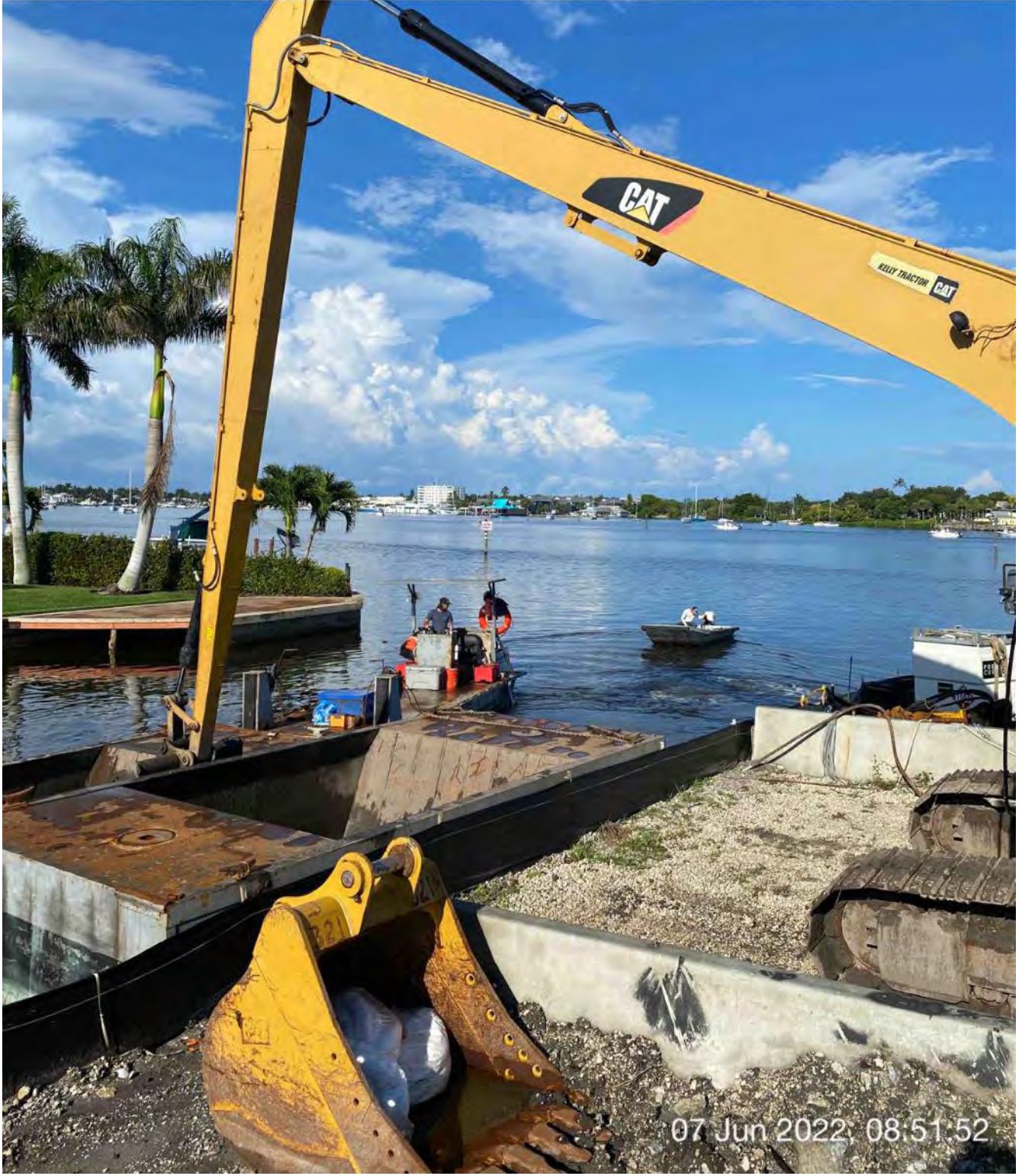
Push boat dropping off full hopper of material at Canal CC-CC station 1+50
