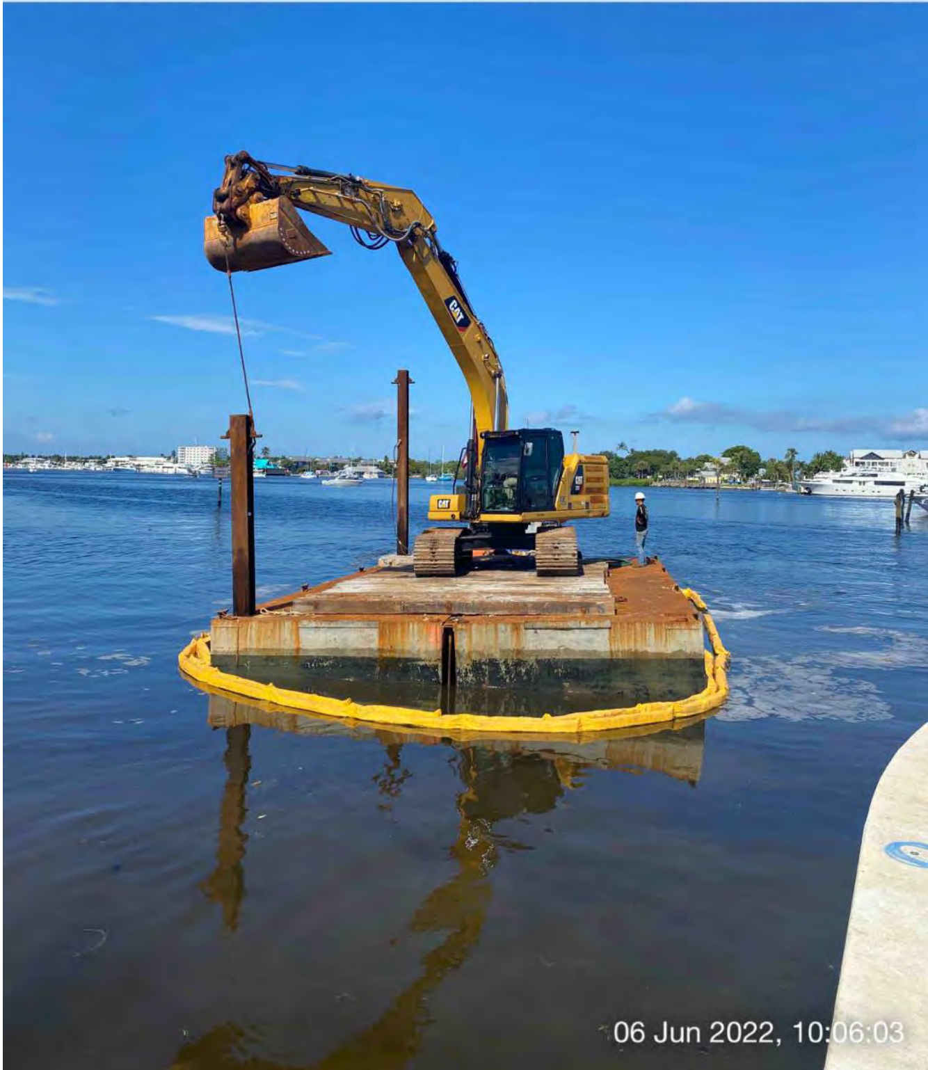
323 excavator lifting spud to allow push boat to mobilize barge from Canal CC-CC to Canal X-X
