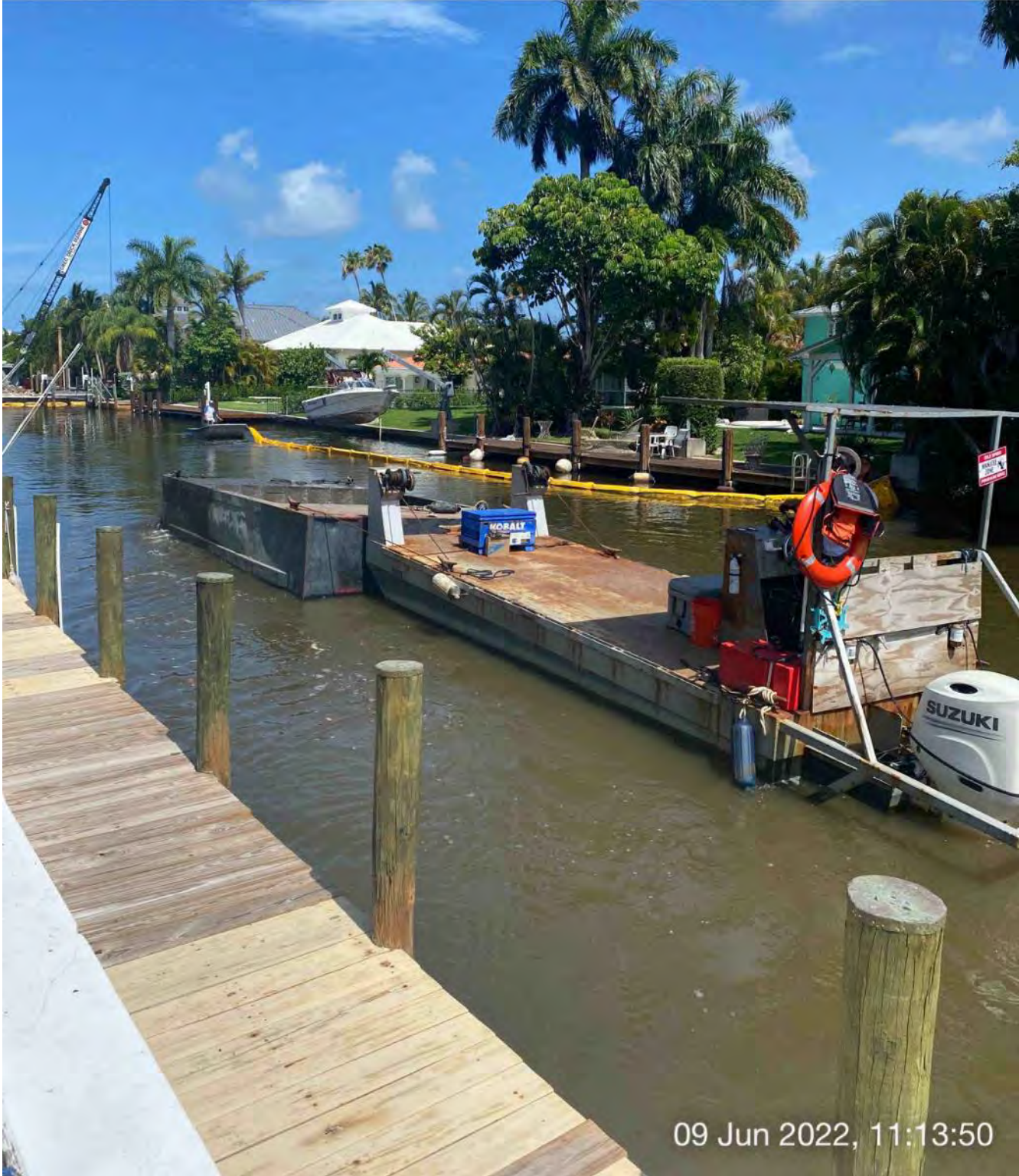
Support boat being used to open turbidity curtain to allow push boat to transport full hopper back to Canal CC-CC
