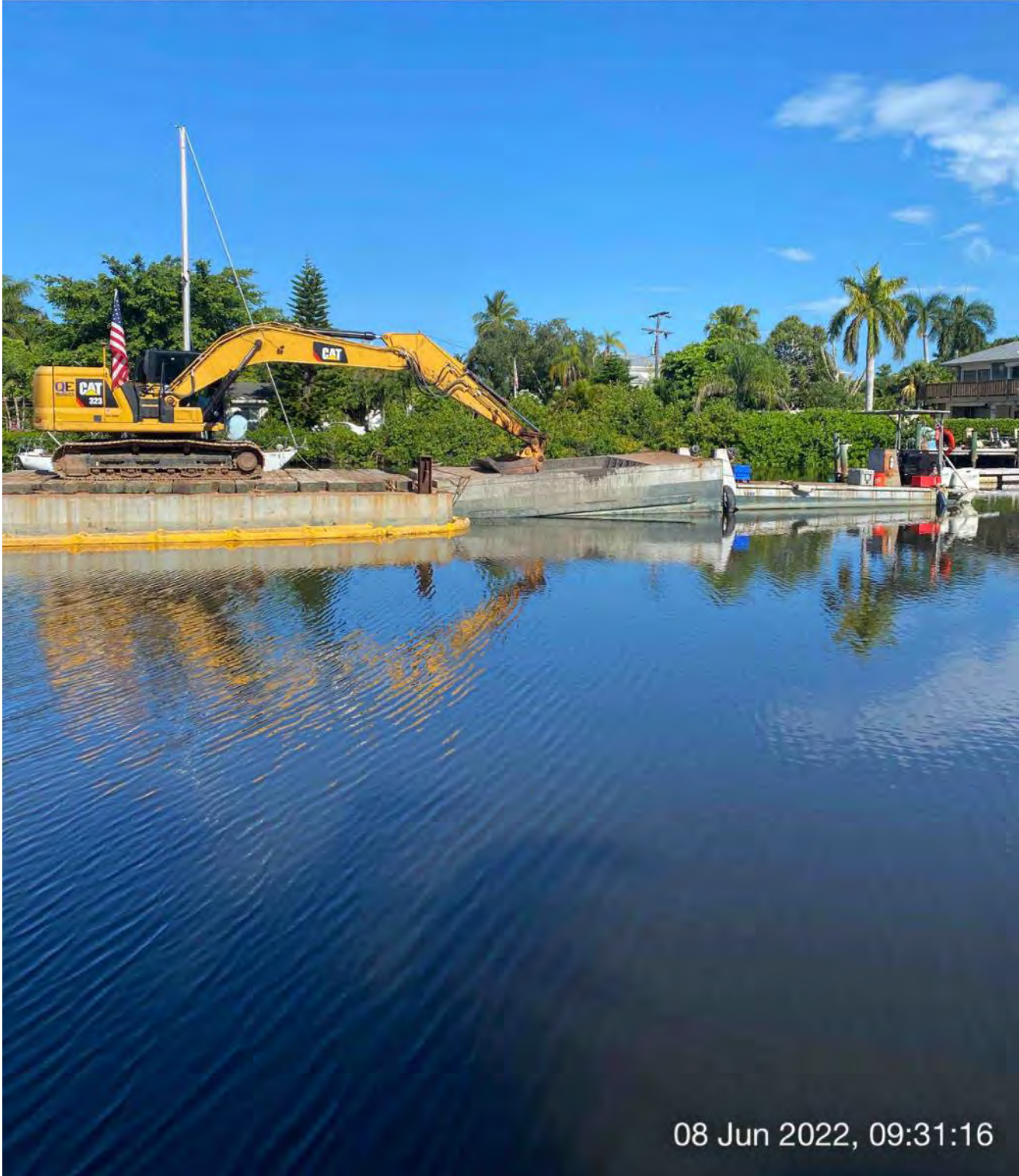
323 excavator, hopper, and push boat stationed in Canal X-X between stations 14+00 and 15+00
