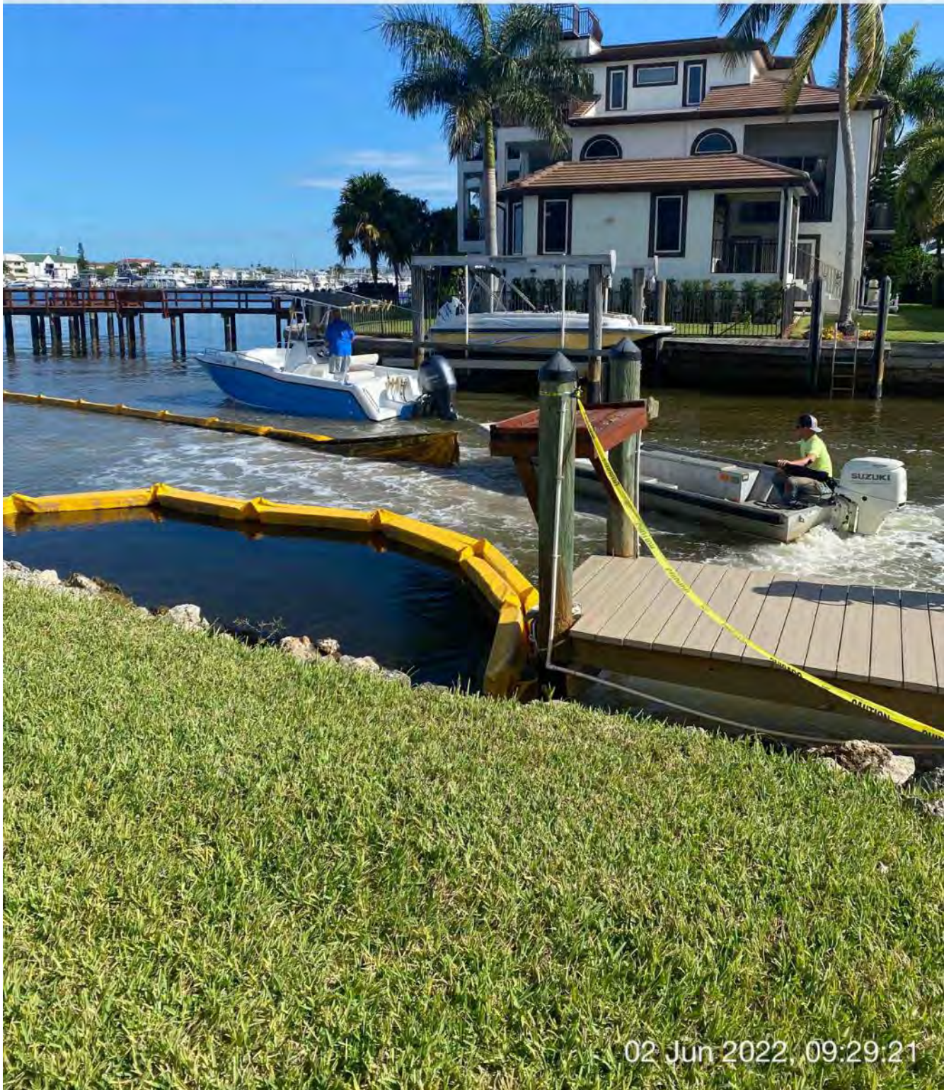
Contractor using support boat to open curtain to allow resident to exit the canal
