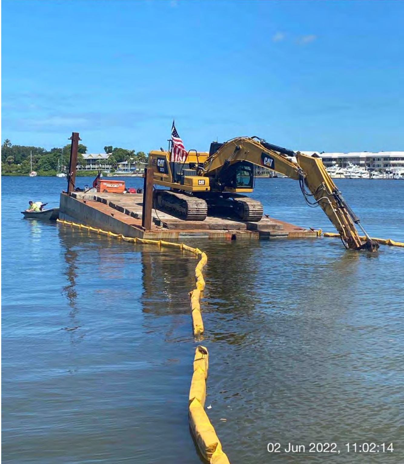
Contractor taking turbidity reading from support boat and 323 excavator grinding rock at station 0+25
