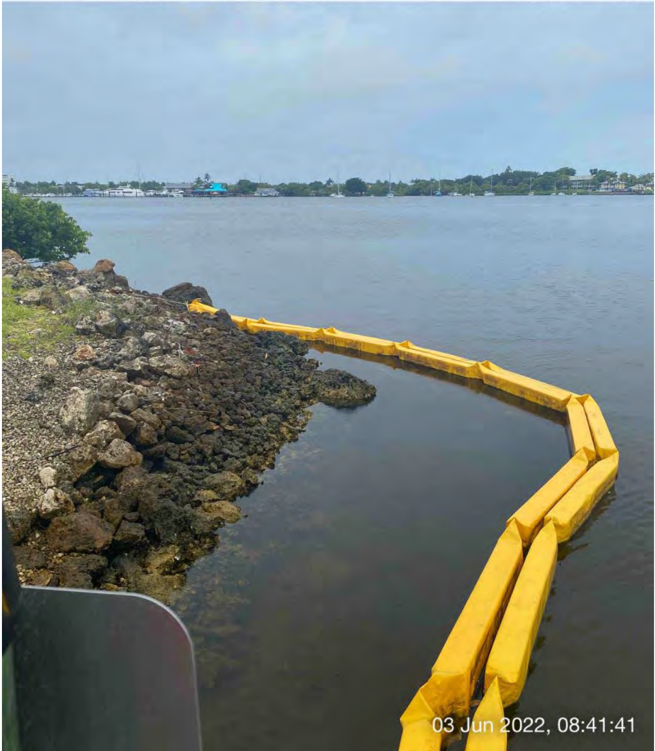
Turbidity curtain tied up to the southside of Canal X-X at station 1+00
