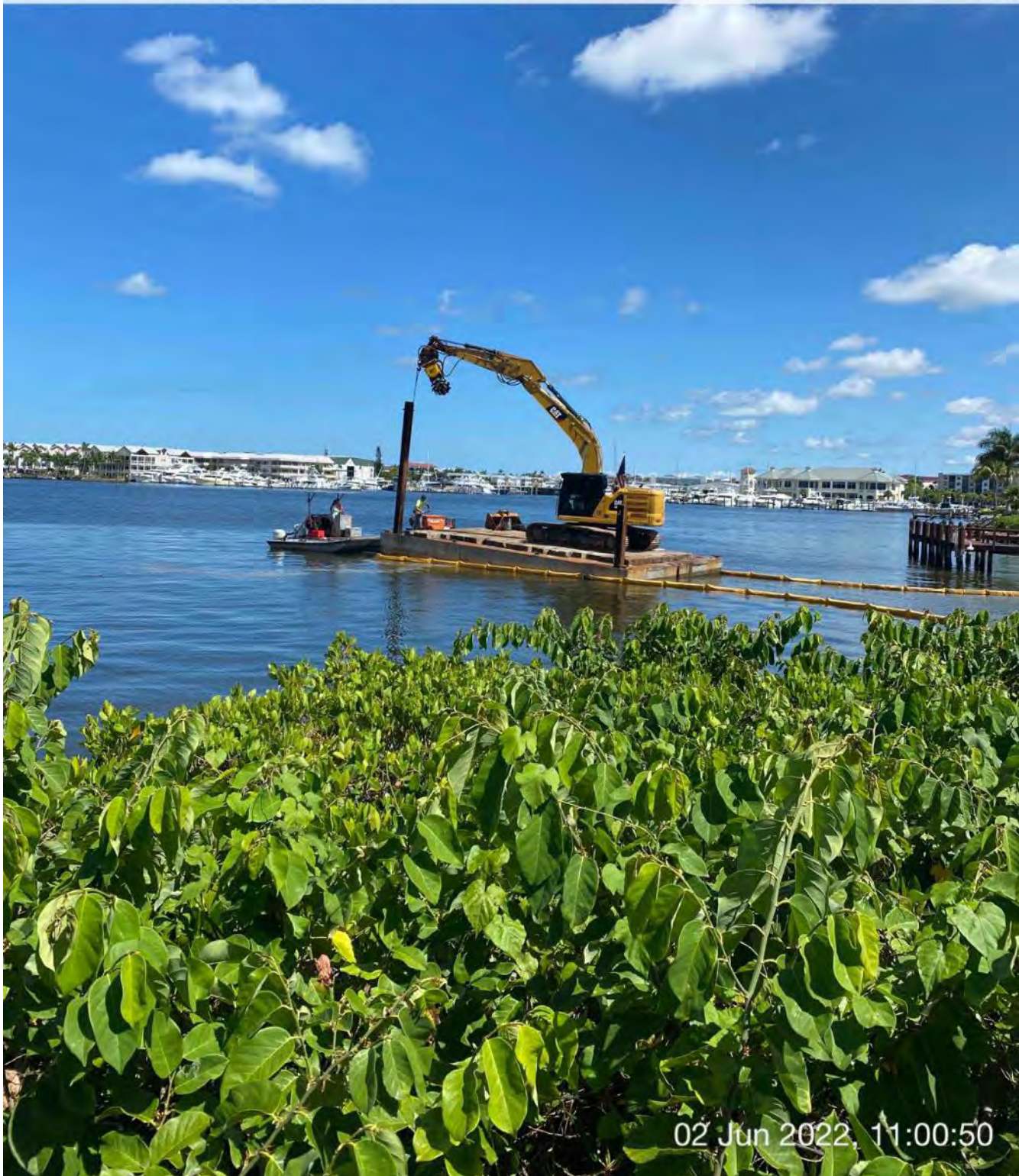
323 excavator lifting spud to allow push boat to mobilize barge at station 0+25
