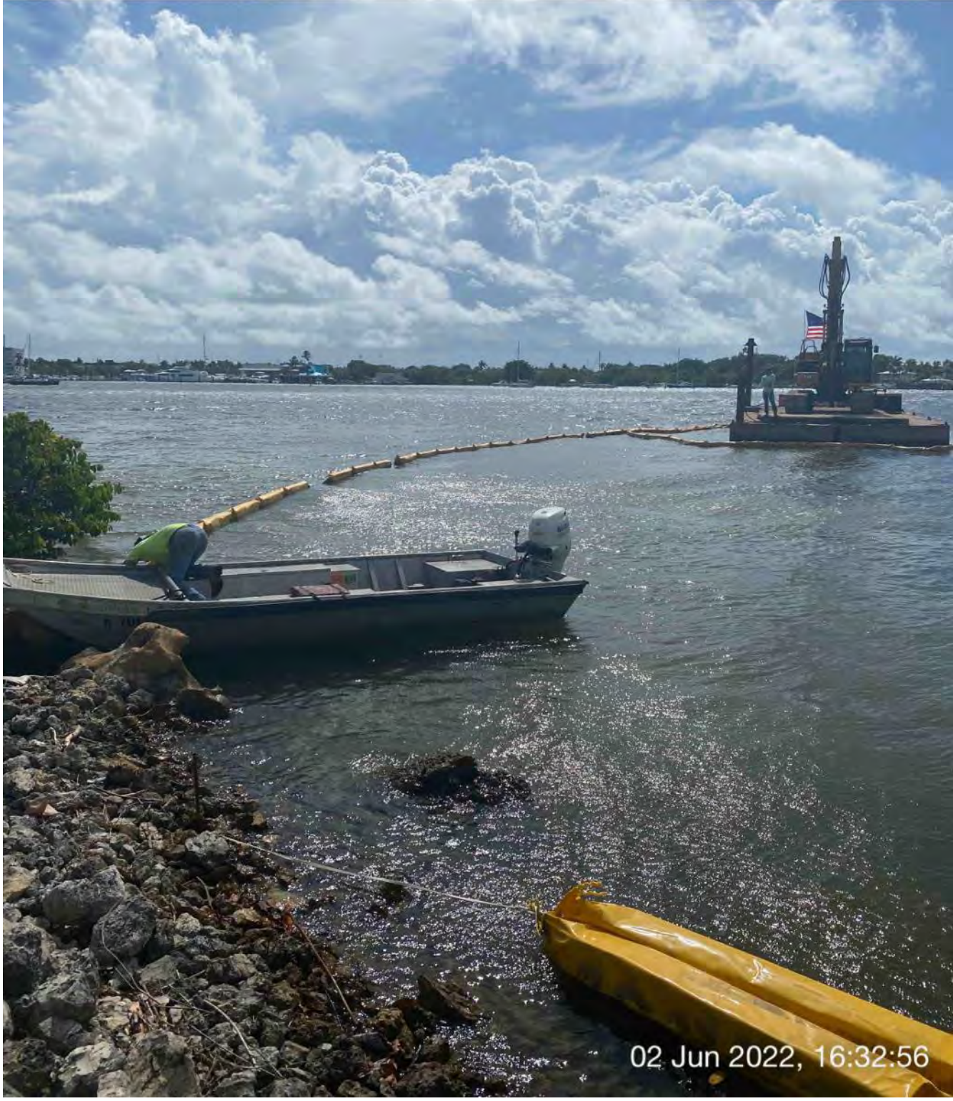
Contractor tying up turbidity curtain to the southside of Canal X-X at station 1+00
