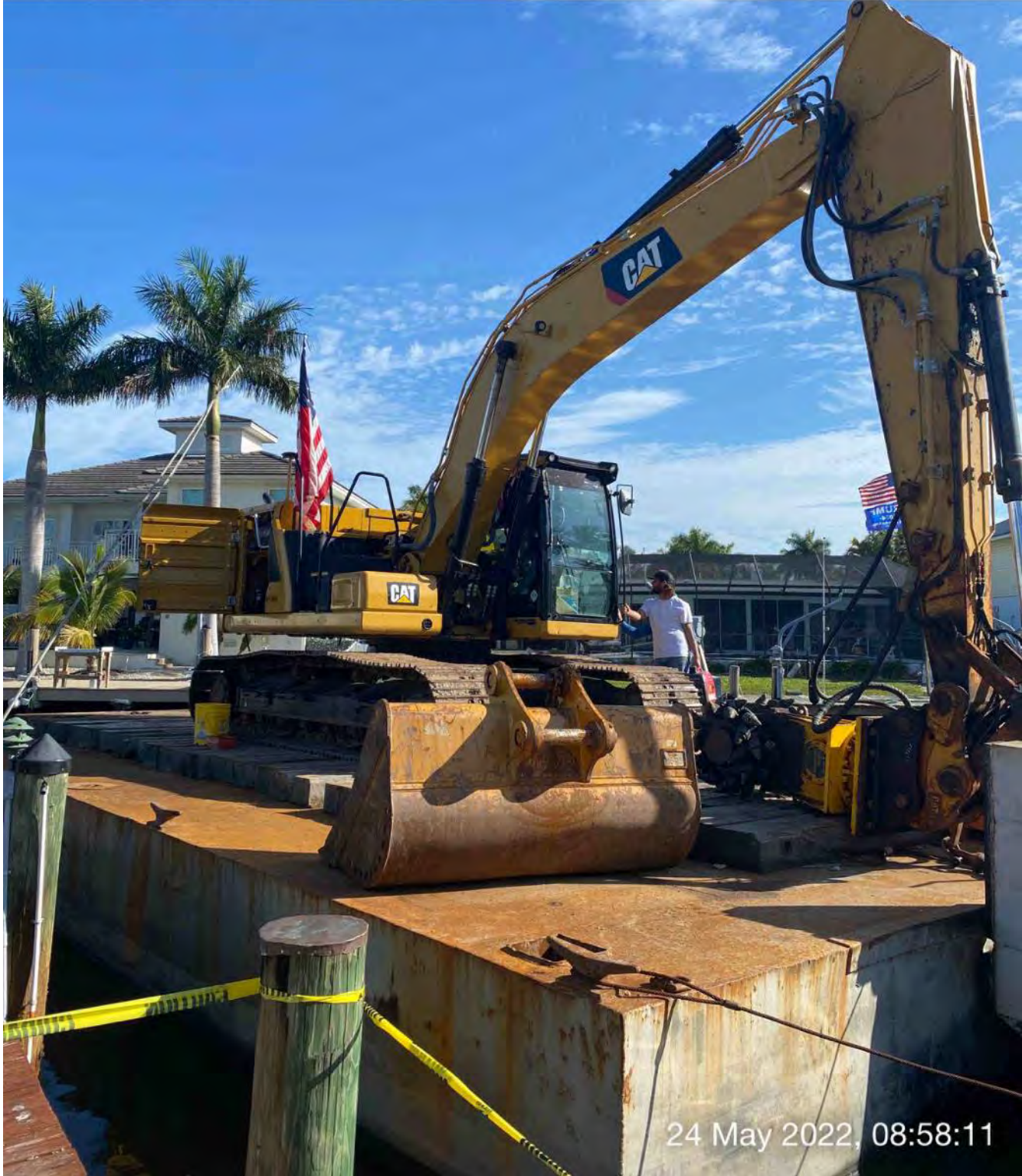
Barge and 323 excavator pushed up against the dock at between Canals X-X and Y-Y
