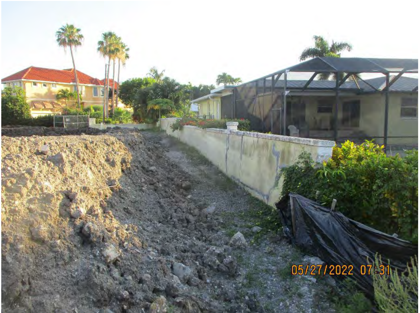
Dredged material removal and wall crack repair noted (1300/1350 Curlew Ave)
