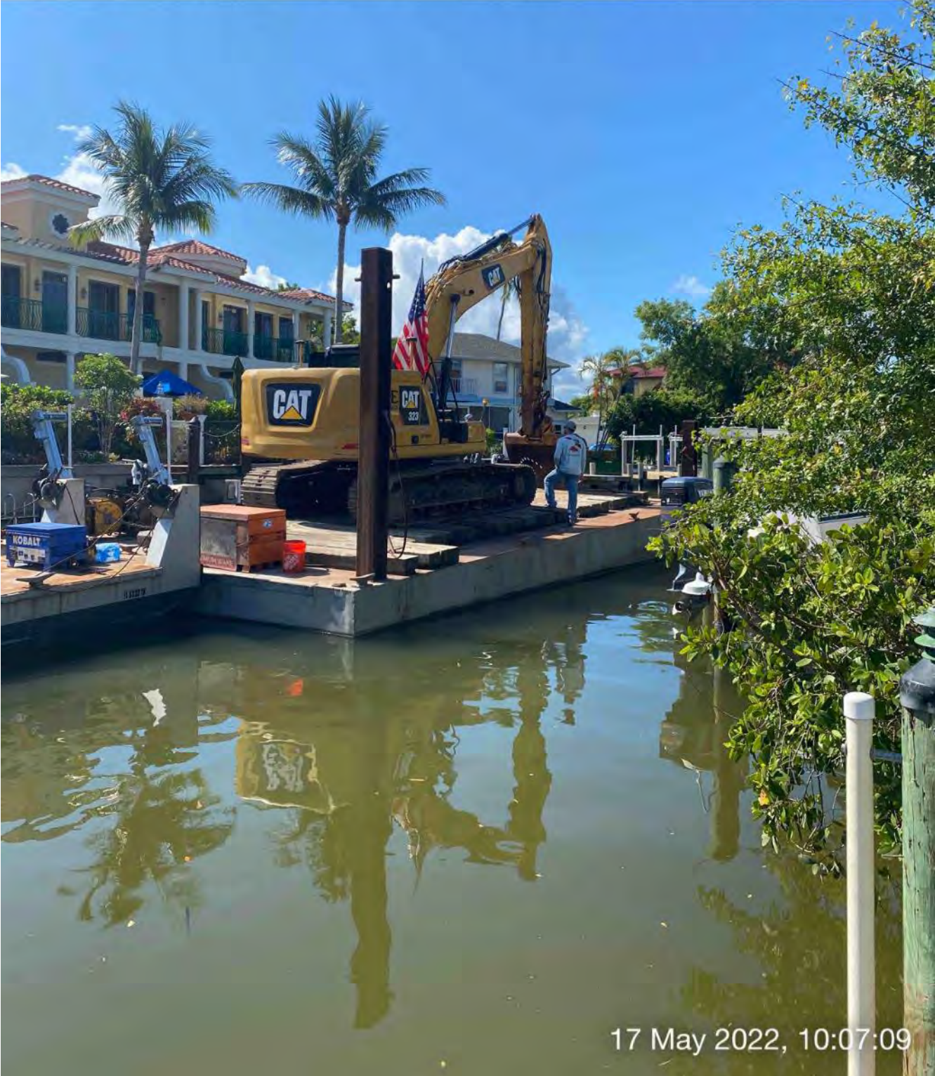
Technicians comparing the 323 excavator's bucket elevation to the Trimble GPS unit's elevation at station 3+50
