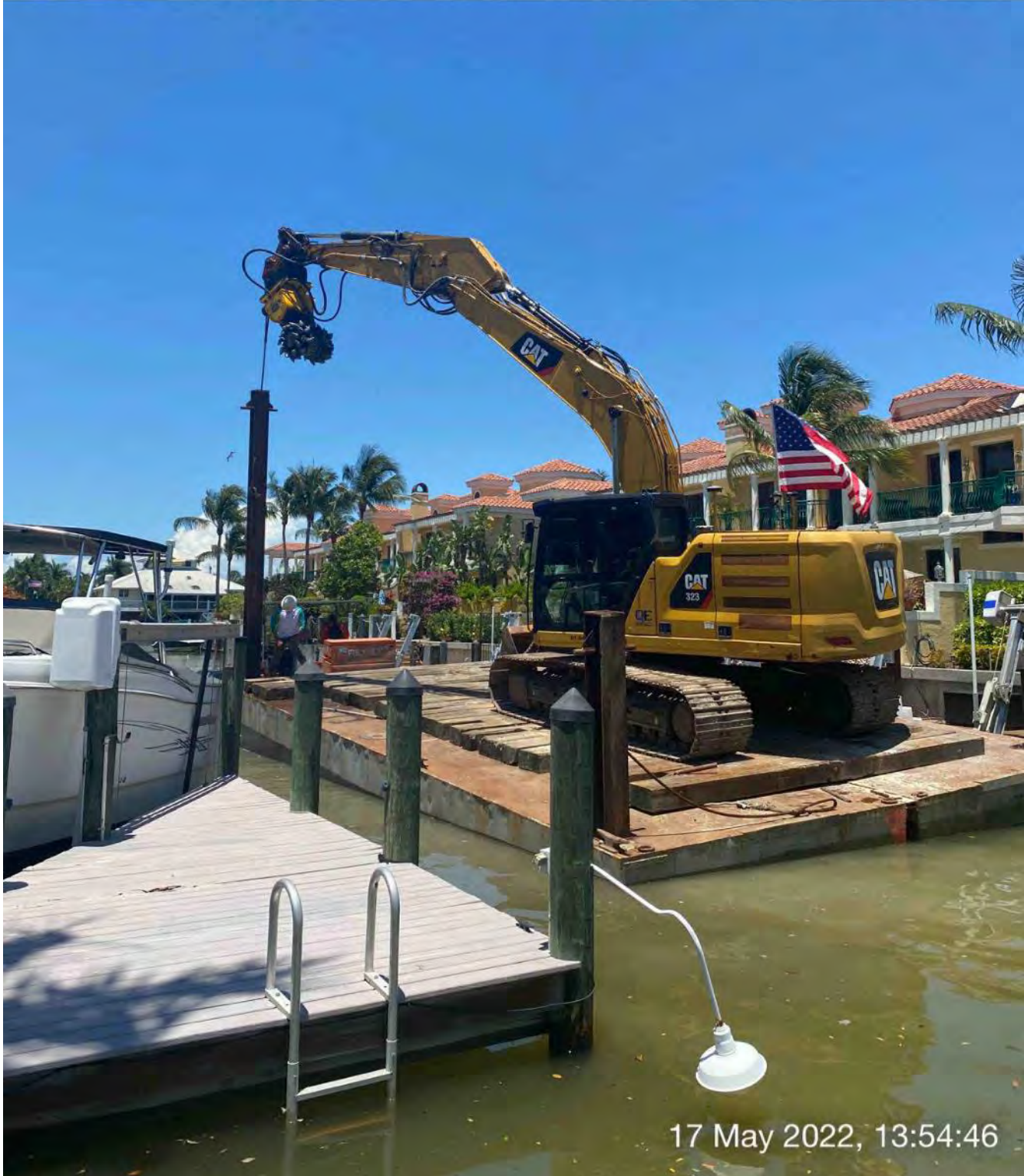
323 excavator lifting spud to allow push boat to mobilize barge at station 3+50
