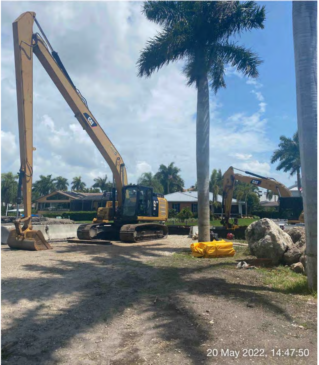
326 excavator on site at 1300 Curlew Avenue and 323 excavator on barge in Canal CC-CC at station 1+00
