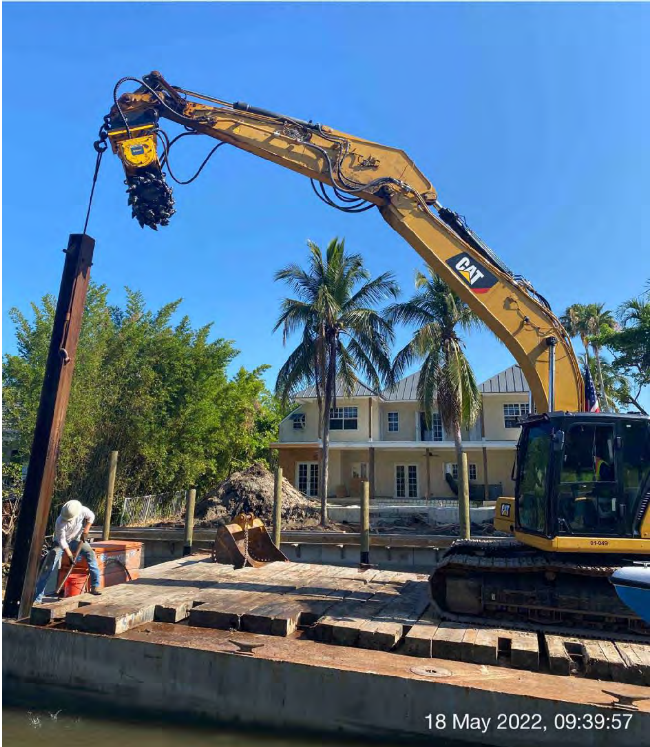
323 excavator lifting spud to allow push boat to mobilize barge at station 7+50
