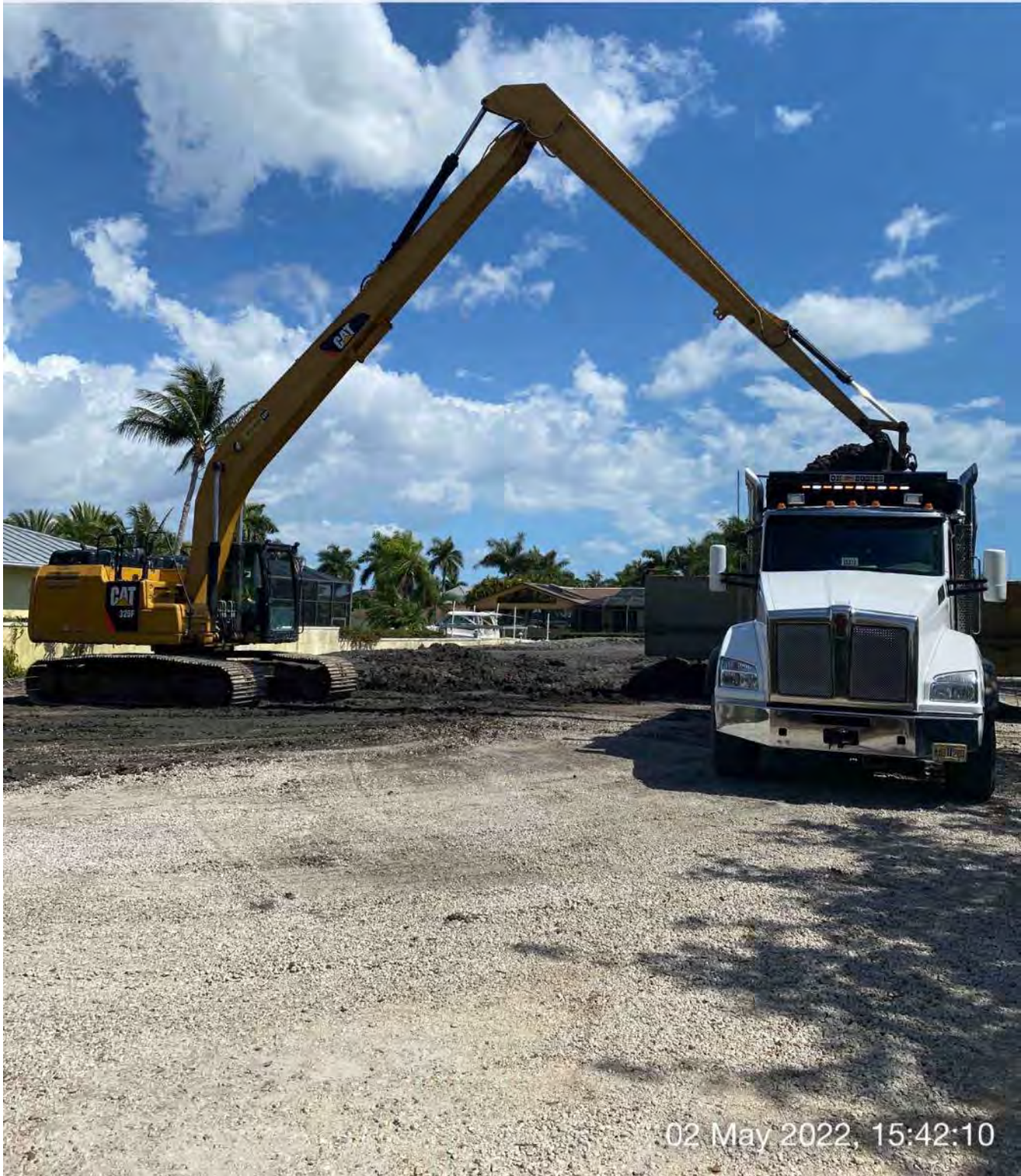
326 excavator transferring removed material from dewatering site to truck bed at 1300 Curlew Avenue
