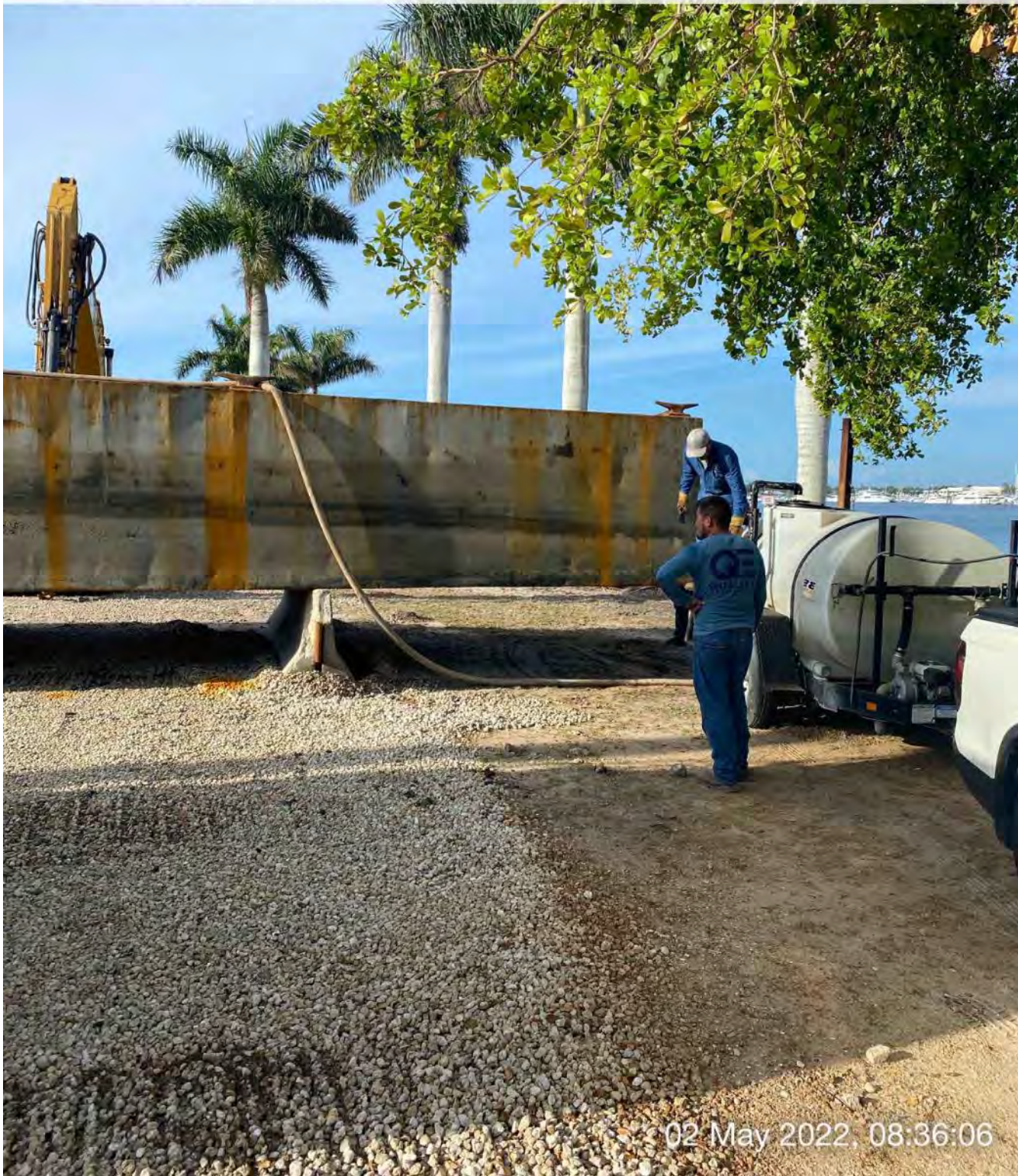
Using water tank to pump water into the barge to identify leak areas
