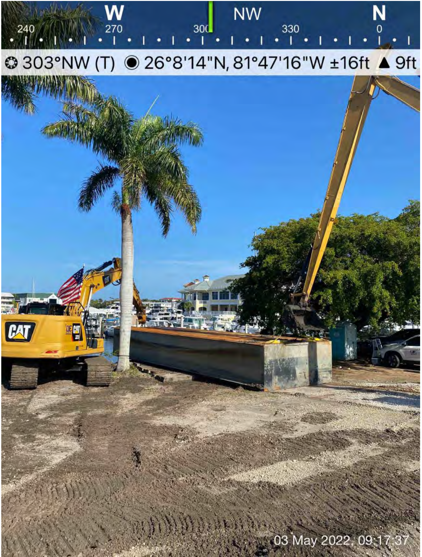
323 and 326 excavators moving barge section towards the west side of the property at 1300 Curlew Avenue
