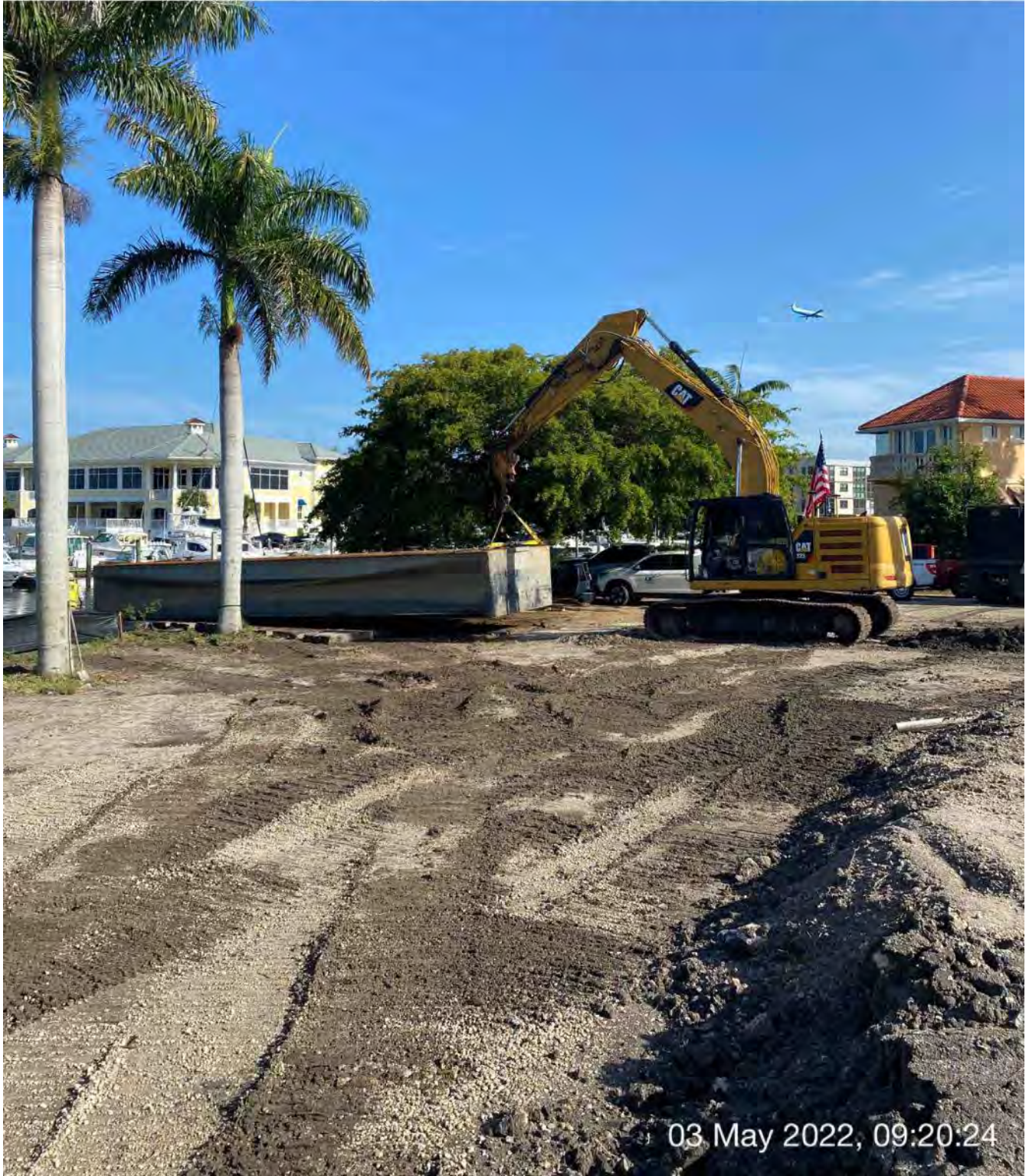
323 excavator lifting barge section at the west side of the property at 1300 Curlew Avenue
