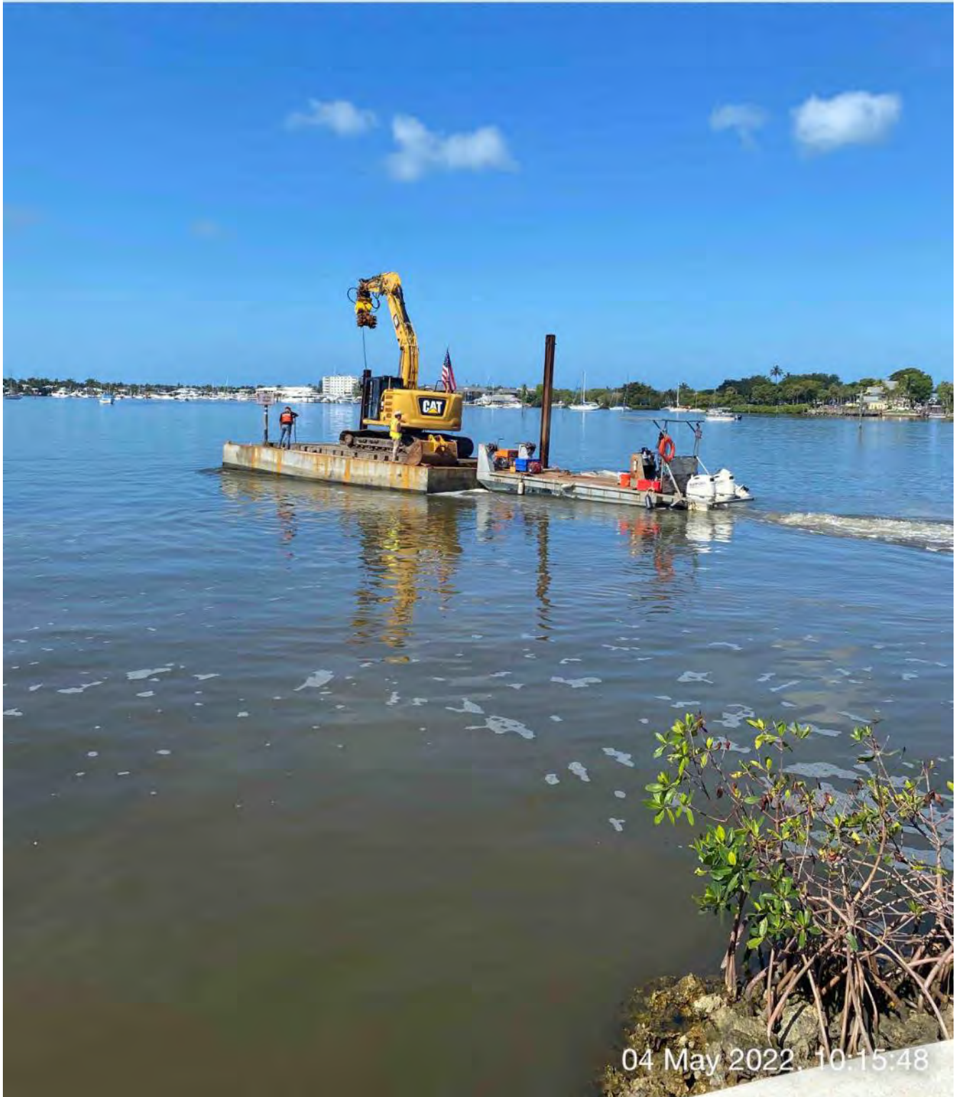
323 excavator lifting spud to allow push boat to transport barge from Canal CC-CC to Canal Y-Y
