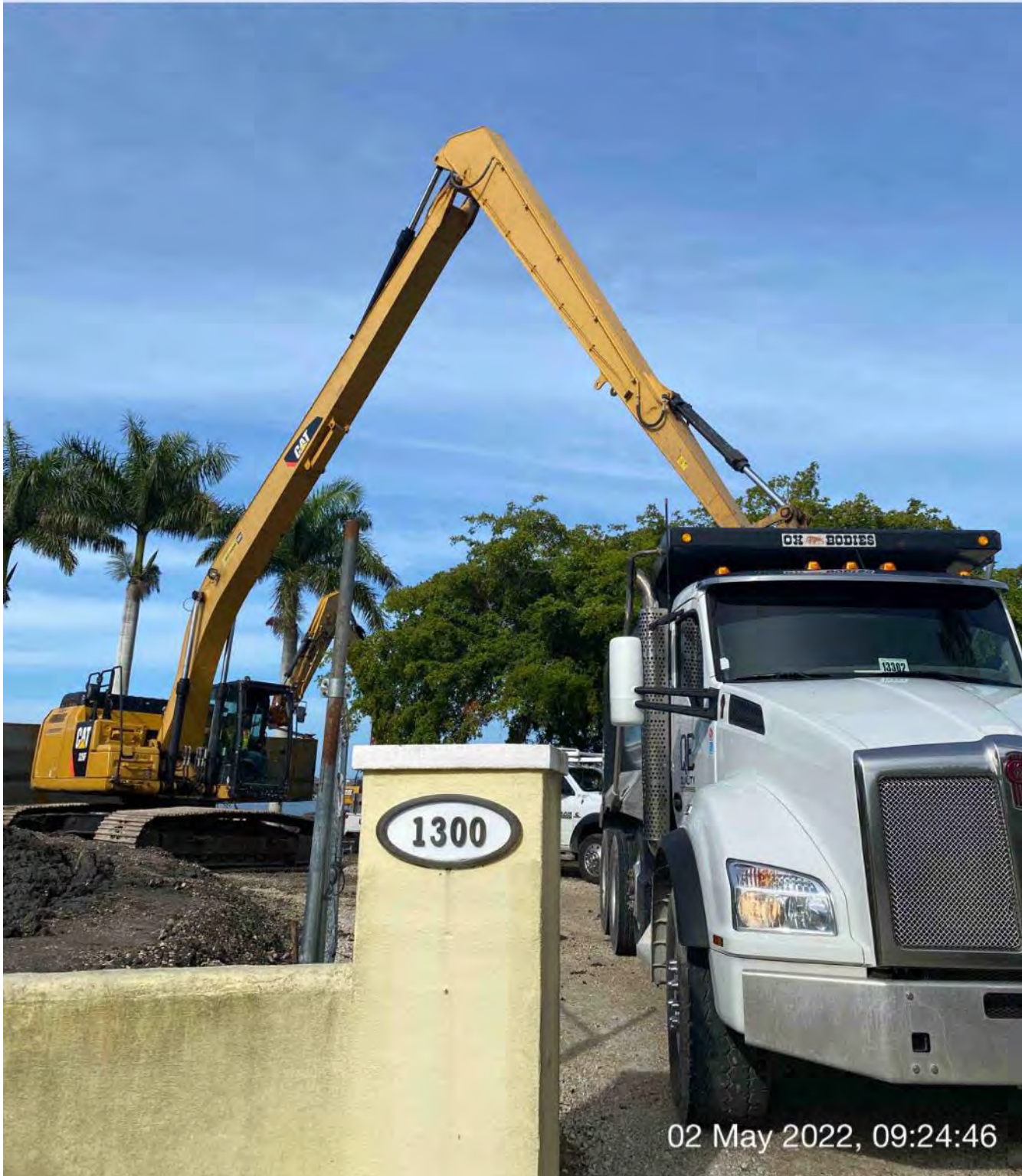
326 excavator transferring removed material from dewatering site to truck bed at 1300 Curlew Avenue
