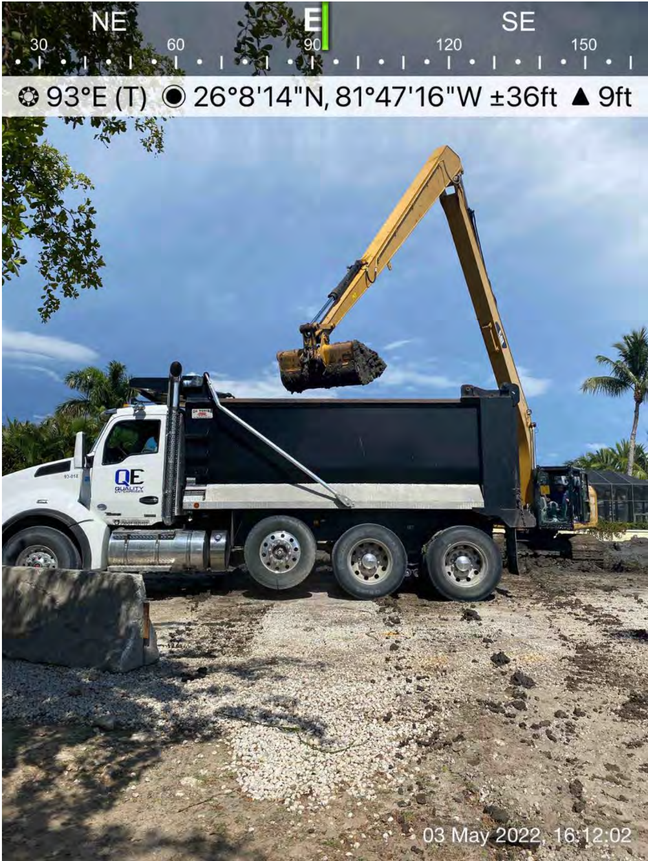
326 excavator transferring removed material from dewatering site to truck bed at 1300 Curlew Avenue
