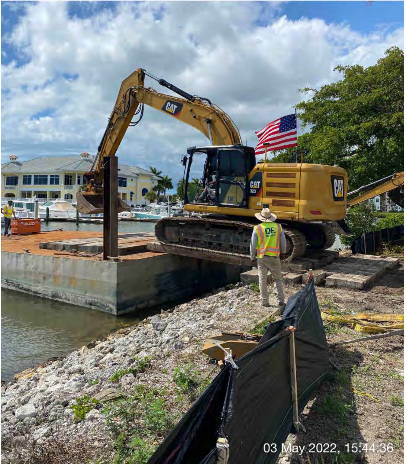
323 excavator traveling across crane tracks from west side of 1300 Curlew Avenue to barge
