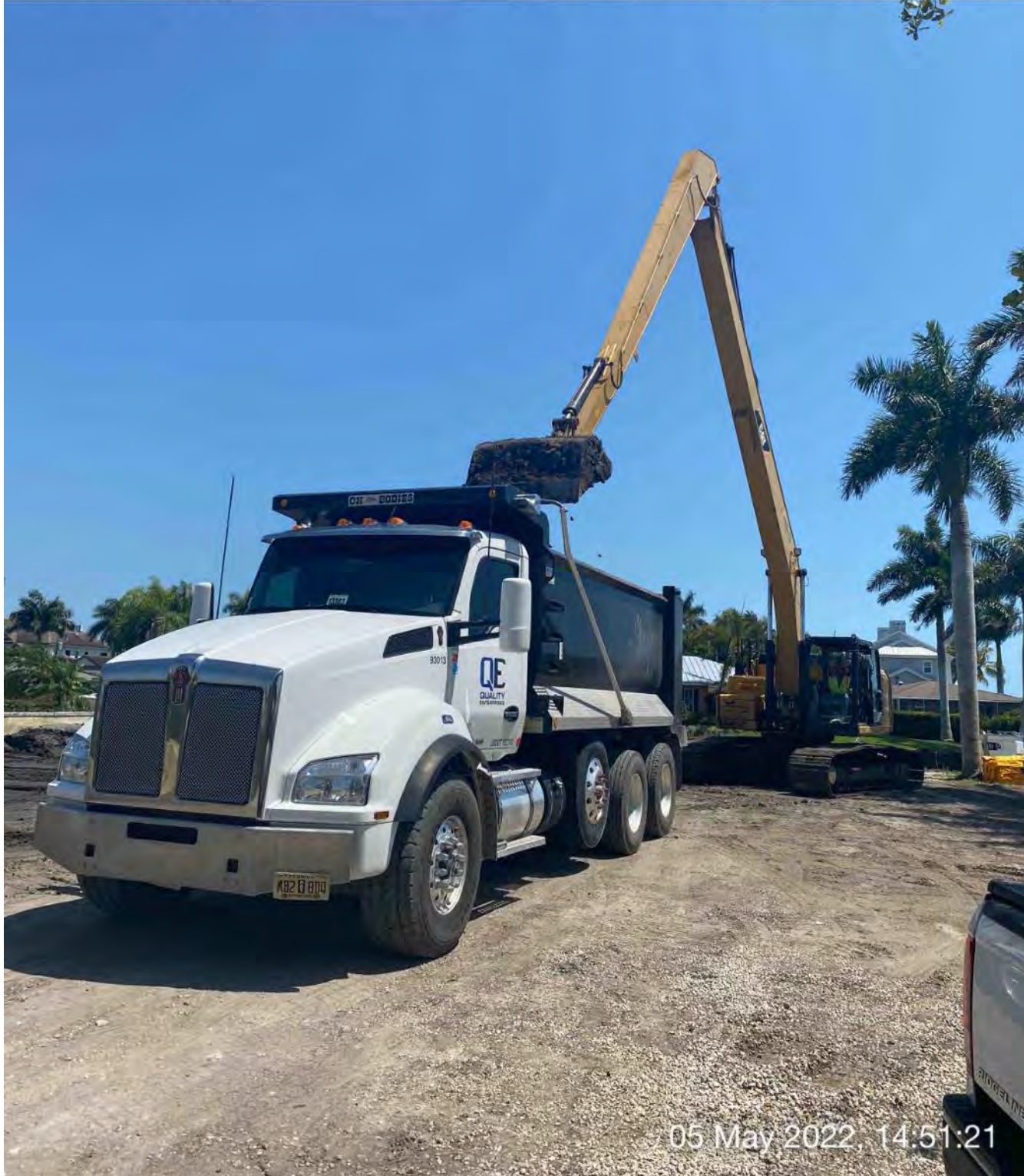
326 excavator transferring removed material from the dewatering site to dump truck bed at 1300 Curlew Avenue
