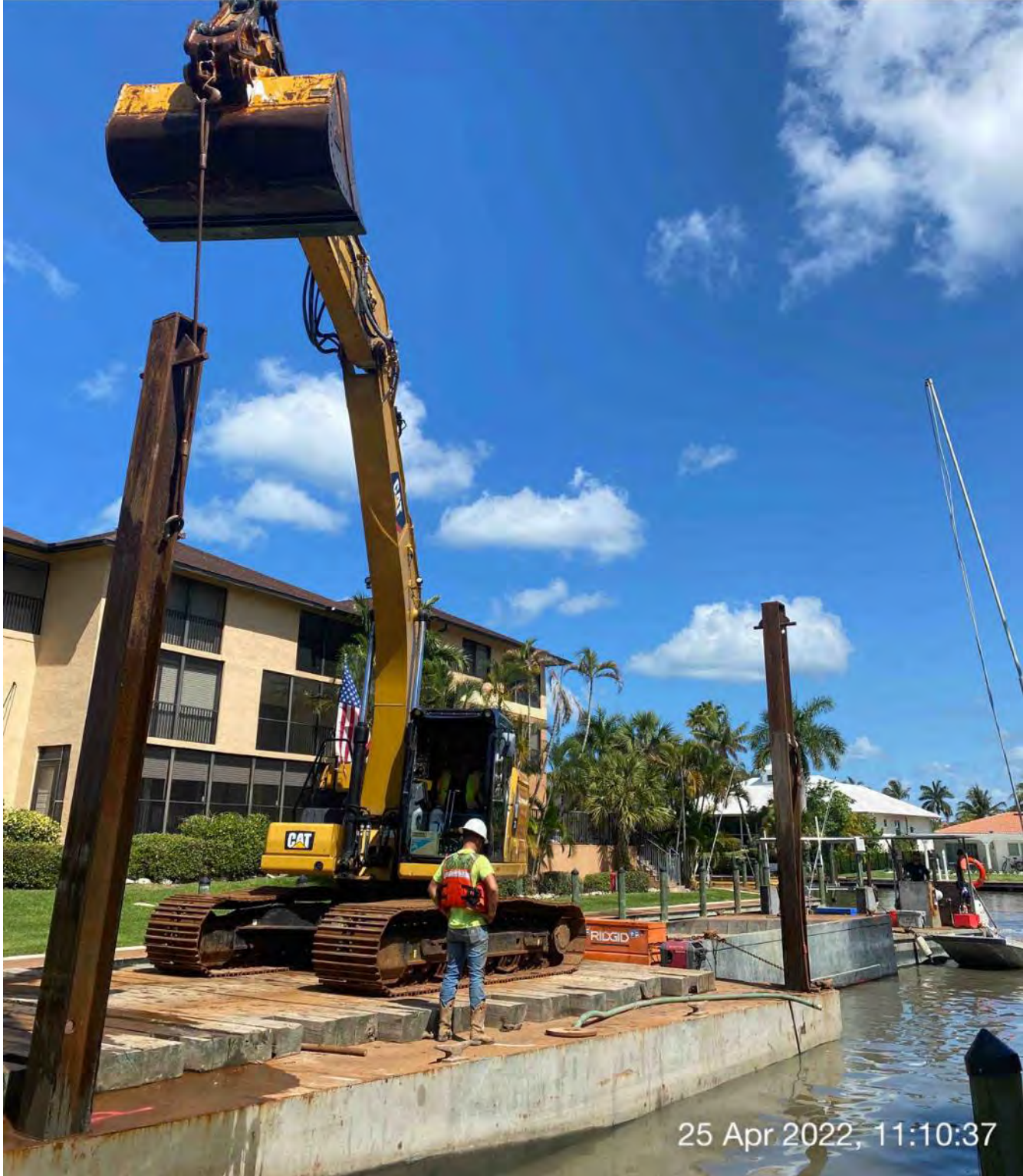
323 excavator lifting spud to allow push boat to mobilize barge at station 2+00
