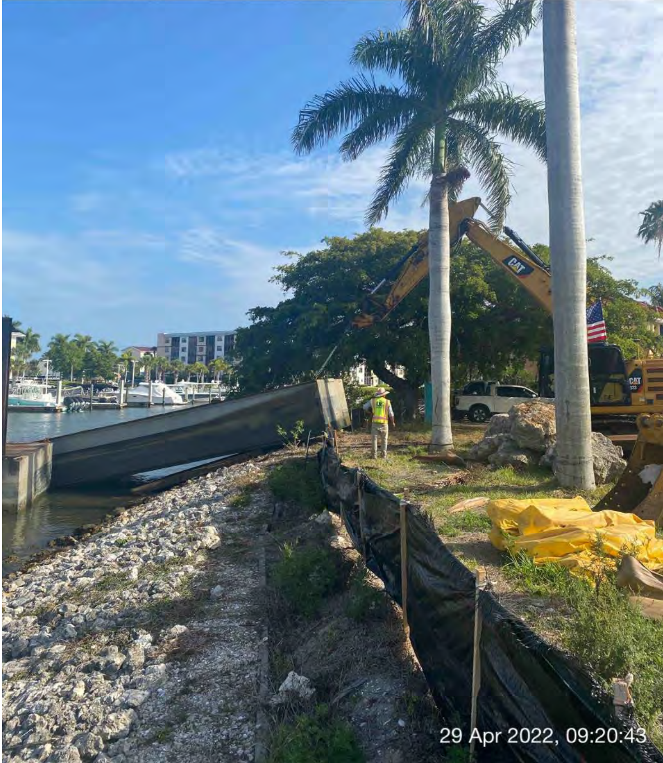
323 excavator lifting 1 section of the barge from the water to the property at 1300 Curlew Avenue
