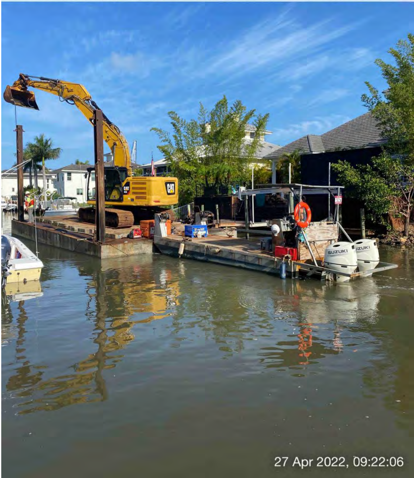
323 excavator lifting spud to allow push boat to mobilize barge at station 2+00 in Canal Z-Z
