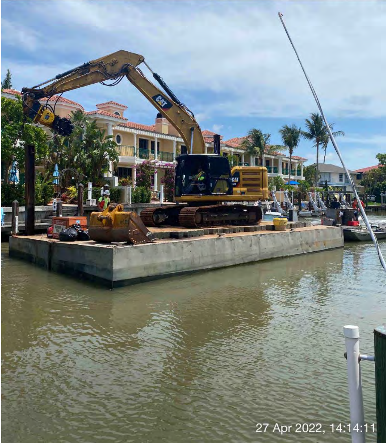
323 excavator lifting spud to allow push boat to mobilize barge at station 2+00 in Canal Y-Y
