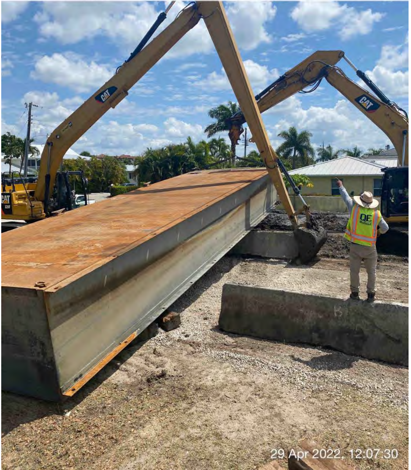
323 excavator lifting barge section so that 326 excavator can slide Jersey barrier underneath barge
