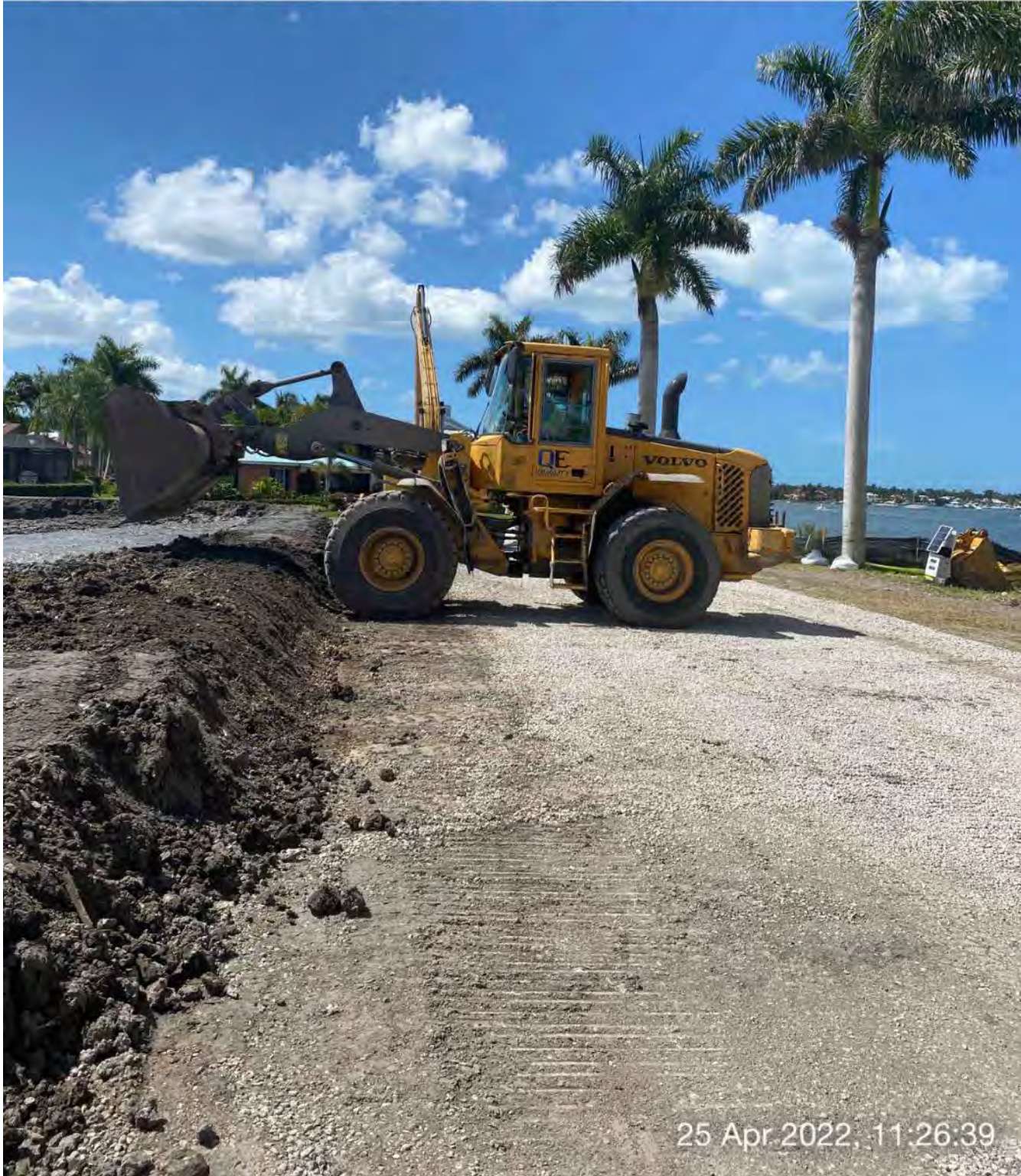
Front end loader redistributing removed material at the dewatering site at 1300 Curlew Avenue
