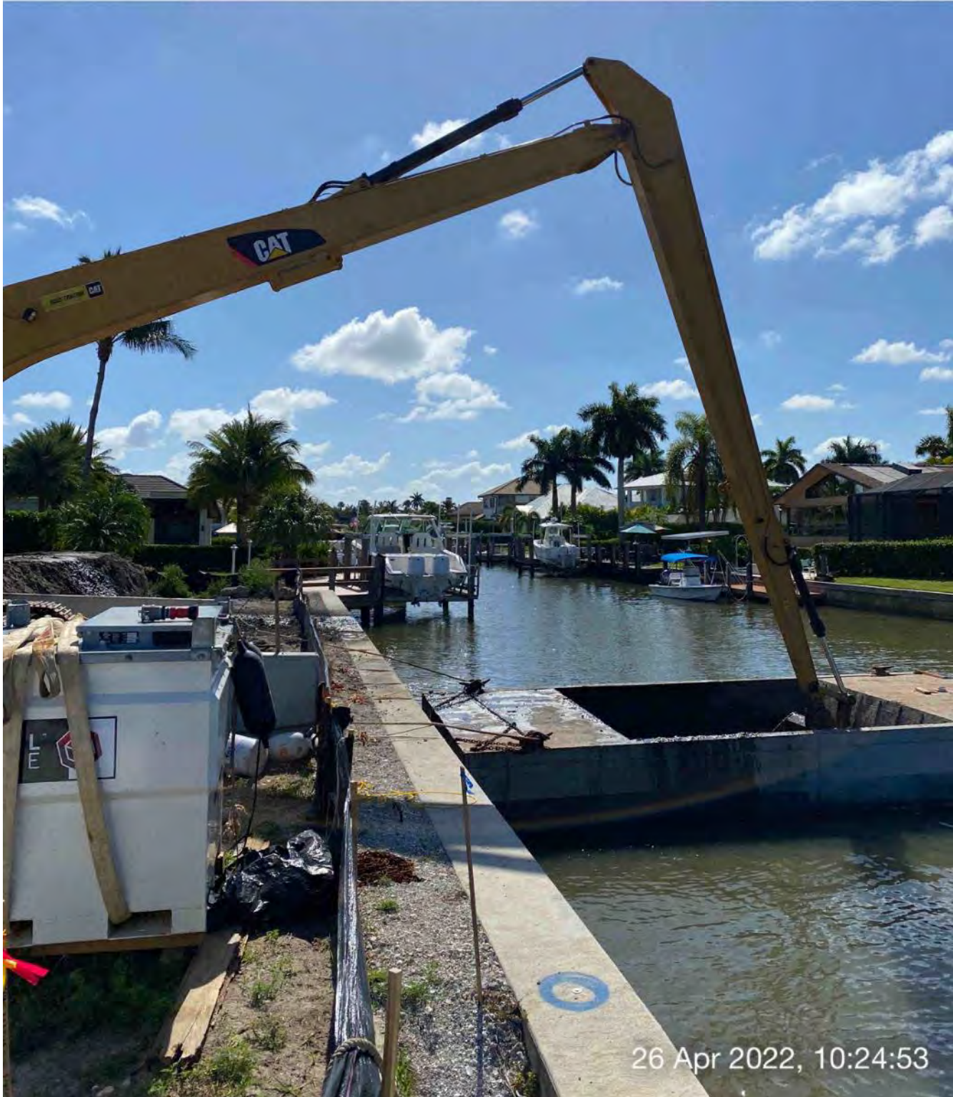
326 excavator transferring one hopper of removed material from hopper to dewatering site at 1300 Curlew Avenue
