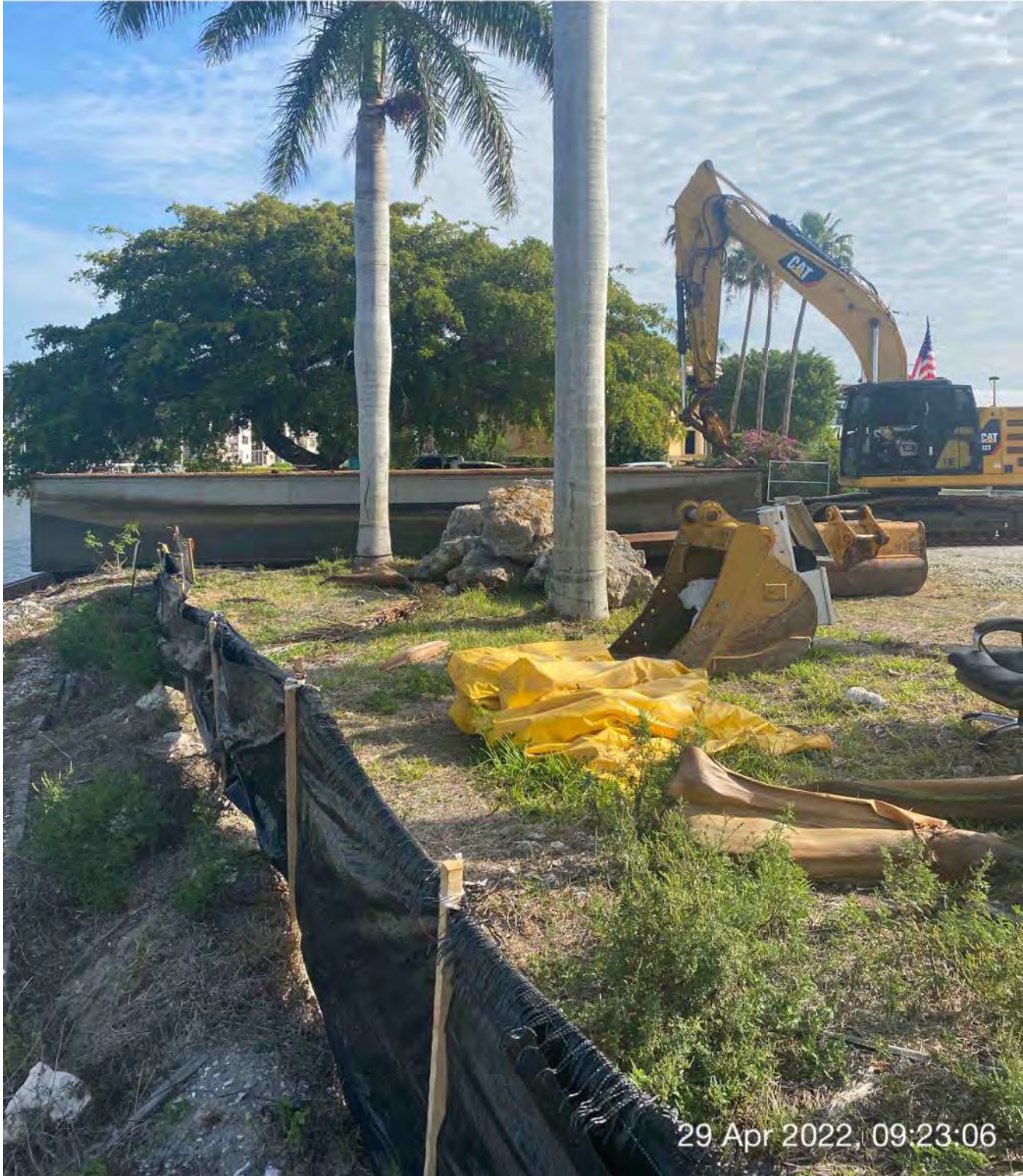
323 excavator lifting 1 section of the barge from the water to the property at 1300 Curlew Avenue
