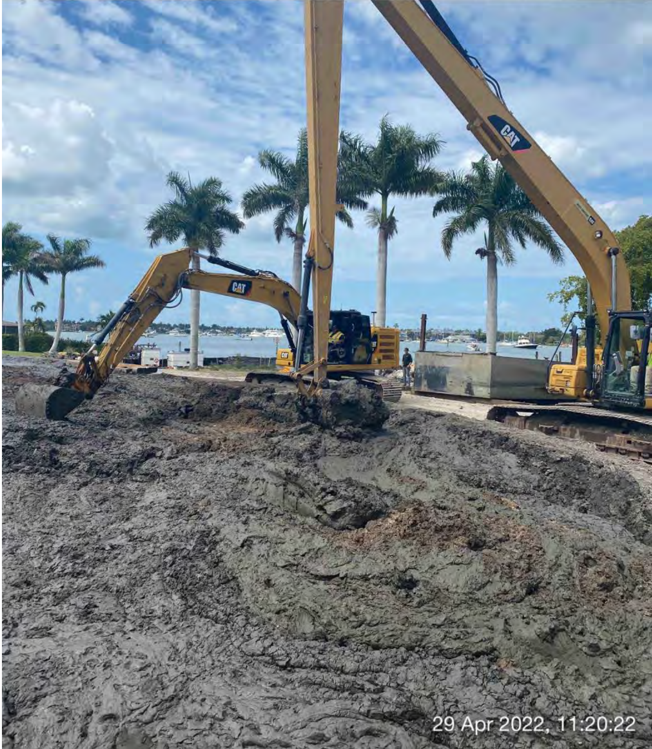
323 excavator and 326 excavator redistributing removed material at the dewatering site at 1300 Curlew Avenue
