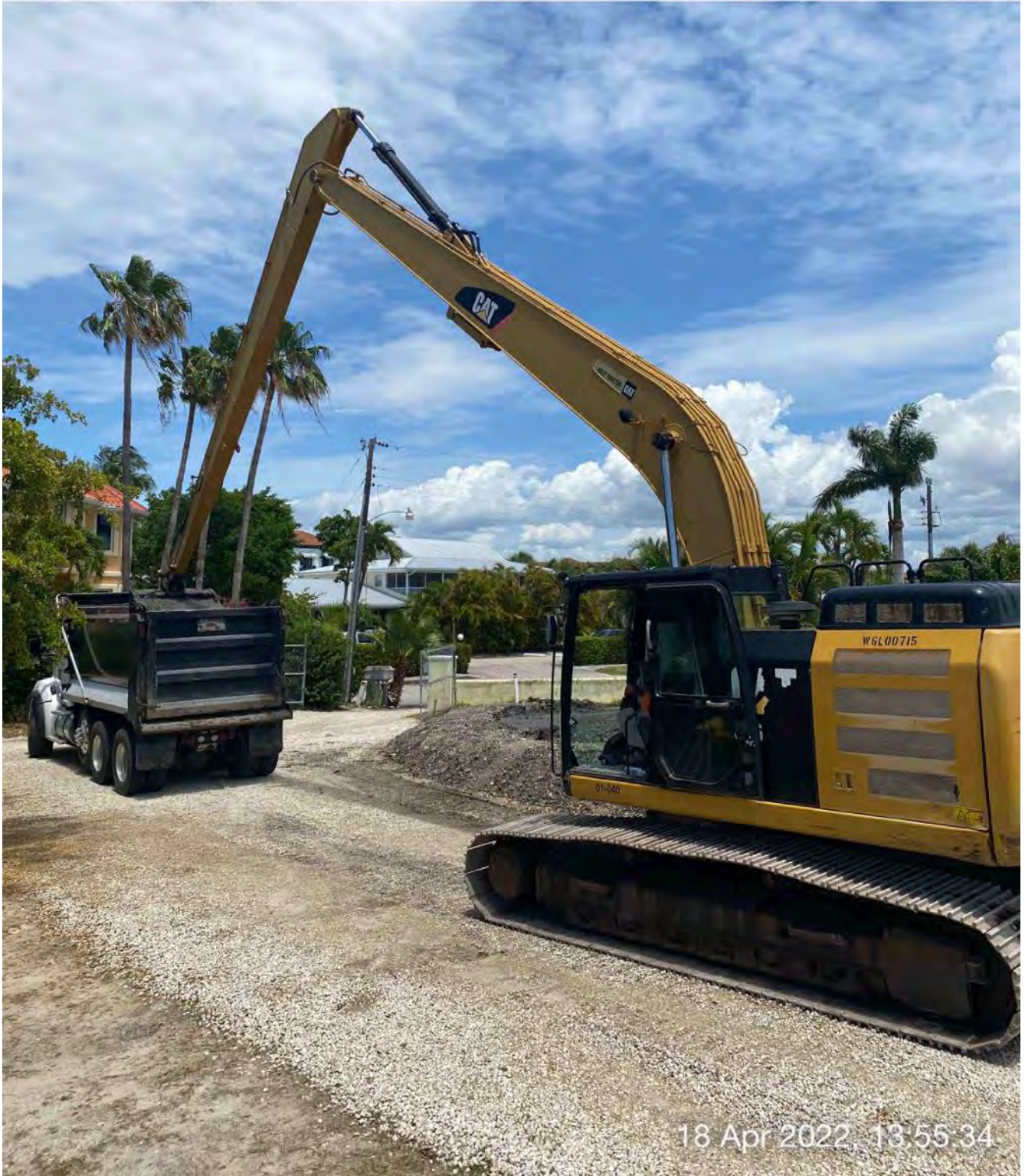
326 excavator transferring removed material from dewatering site to dump truck at 1300 Curlew Avenue
