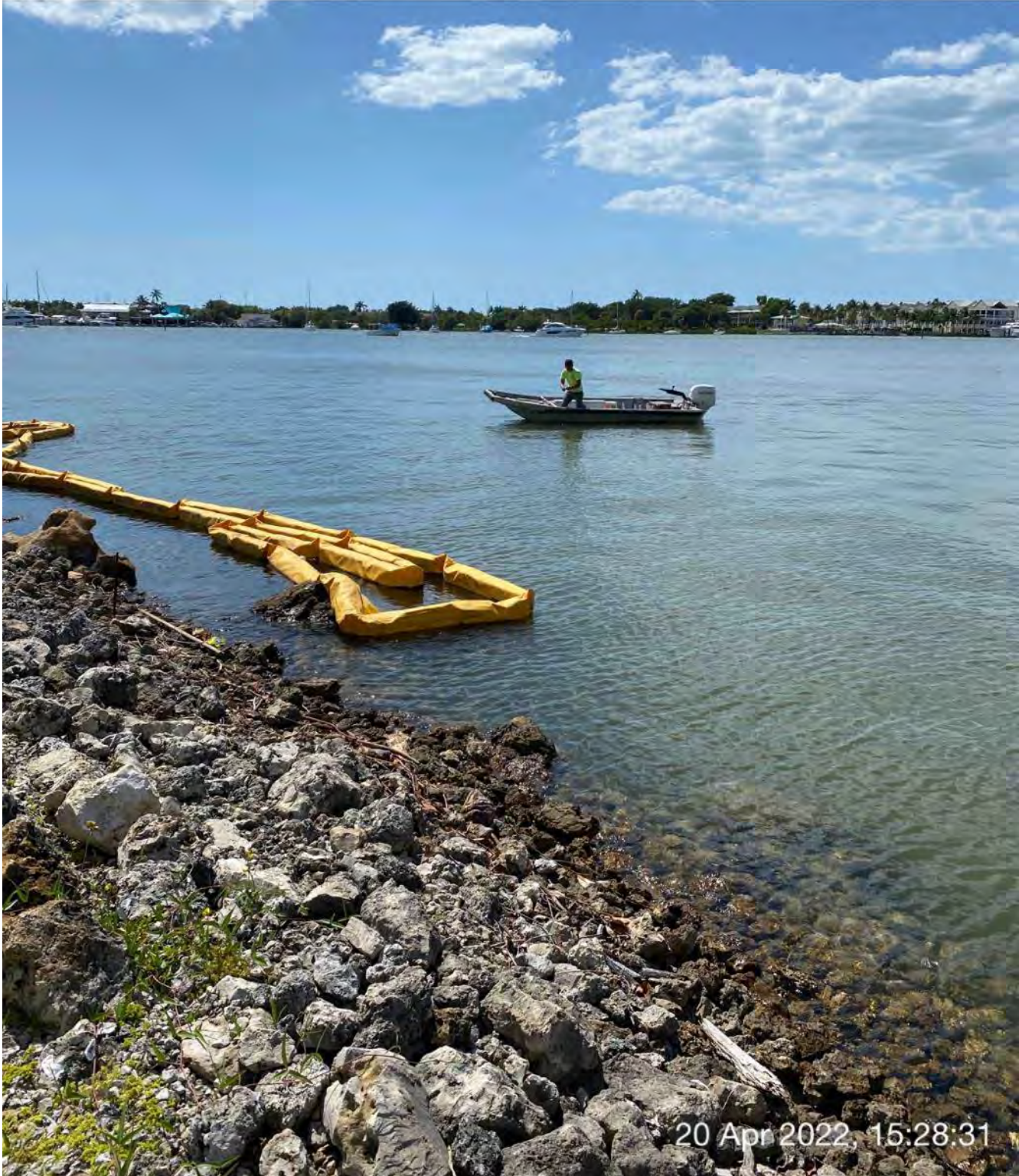
Contractor using support boat to take turbidity measurements at the mouth of Canal X-X
