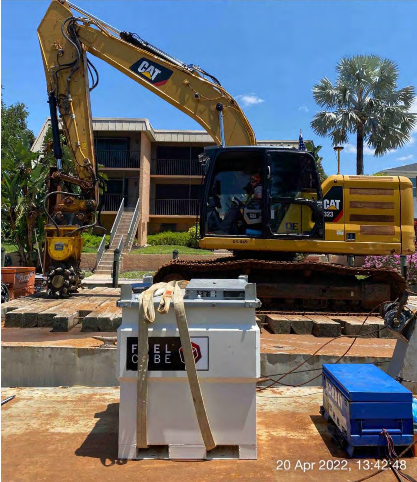
Kelly Tractor technician checking the exhaust signal on 323 excavator's computer at station 3+00
