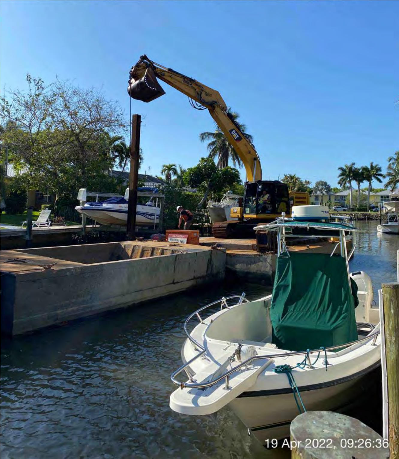
323 excavator lifting spud to allow push boat to mobilize barge in Canal AA-AA at station 1+50
