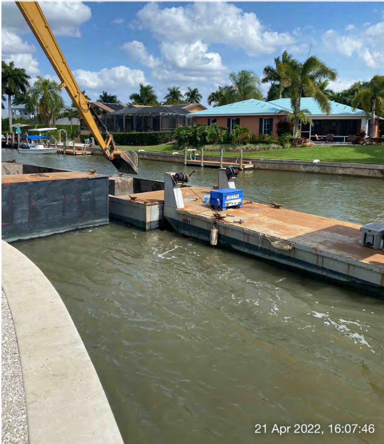
Push boat dropping off a full hopper of material in Canal CC-CC at station 1+50
