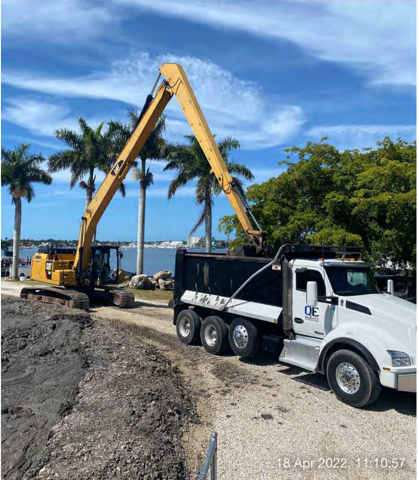
326 excavator transferring removed material from dewatering site to dump truck at 1300 Curlew Avenue
