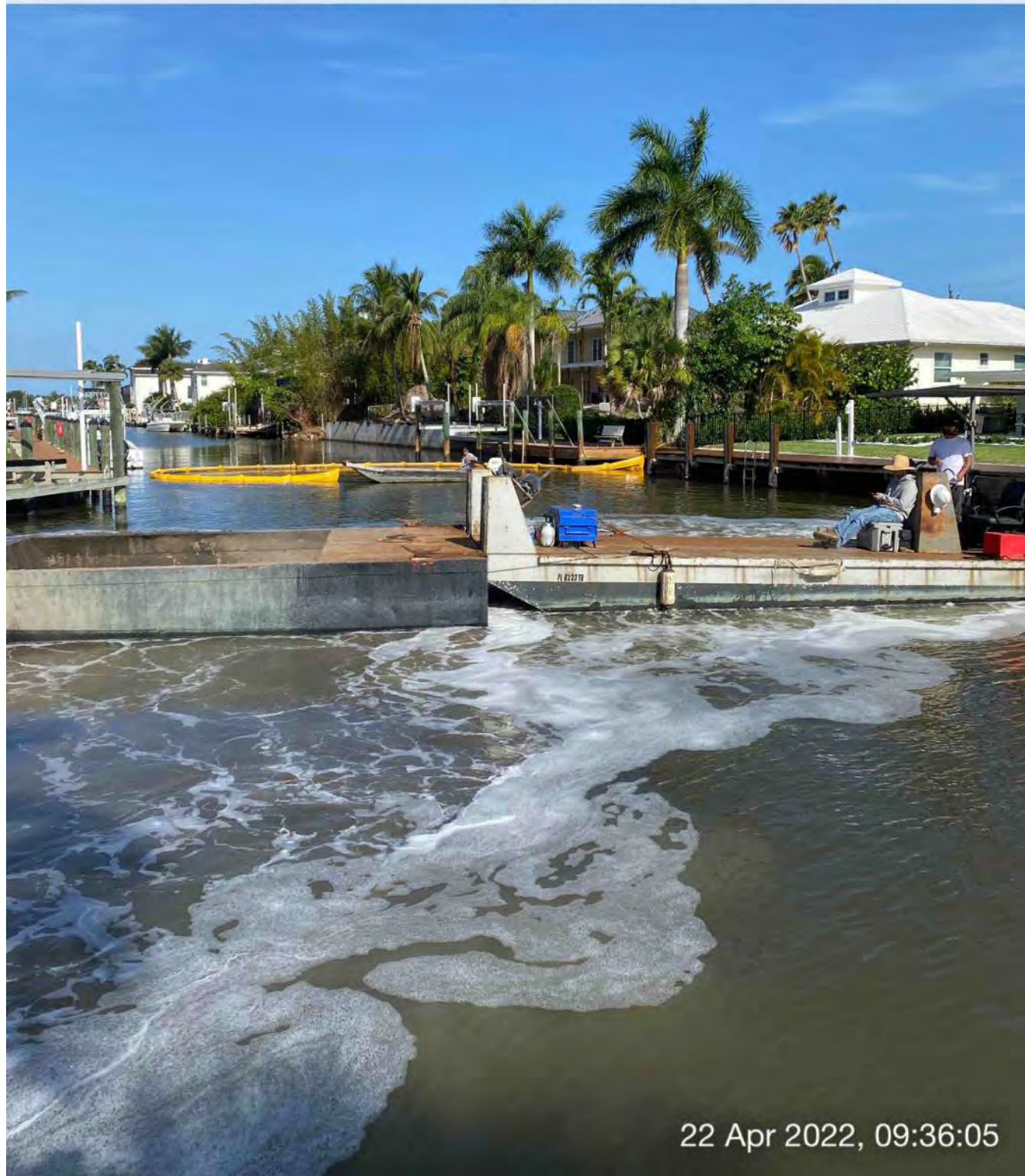
Support boat opening turbidity curtain to allow push boat to transport hopper out of Canal X-X
