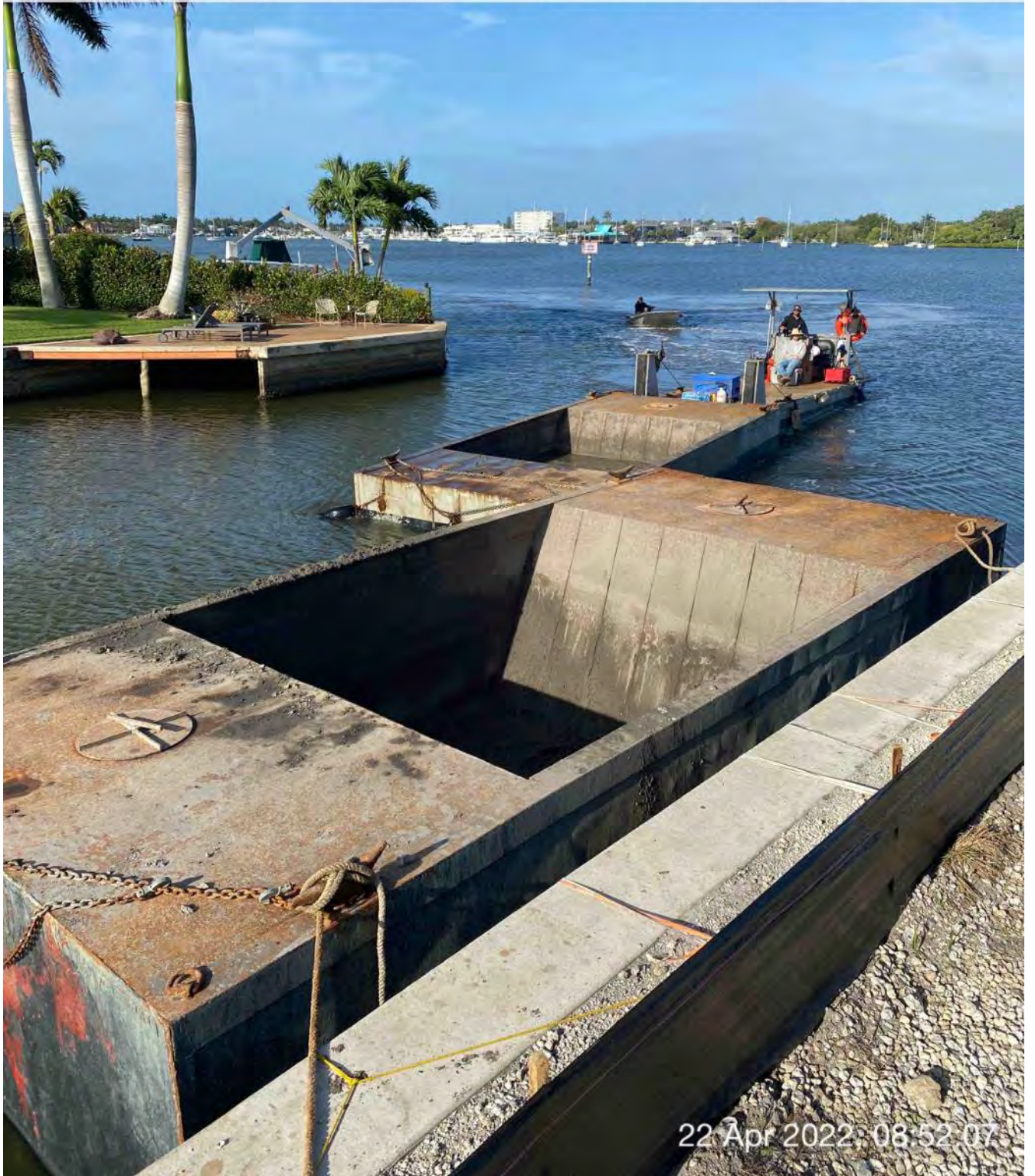
Push boat transporting full hopper of material from Canal Z-Z to Canal CC-CC
