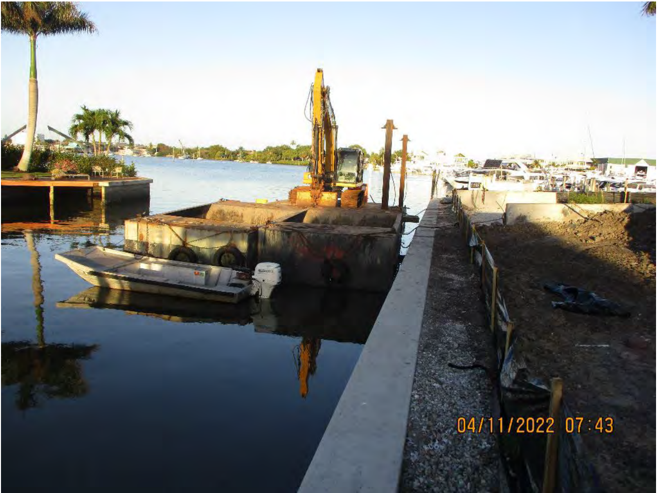
323 excavator, barge, 2 hoppers, and support boat staged in Canal CC-CC at station 1+00 to 1+75
