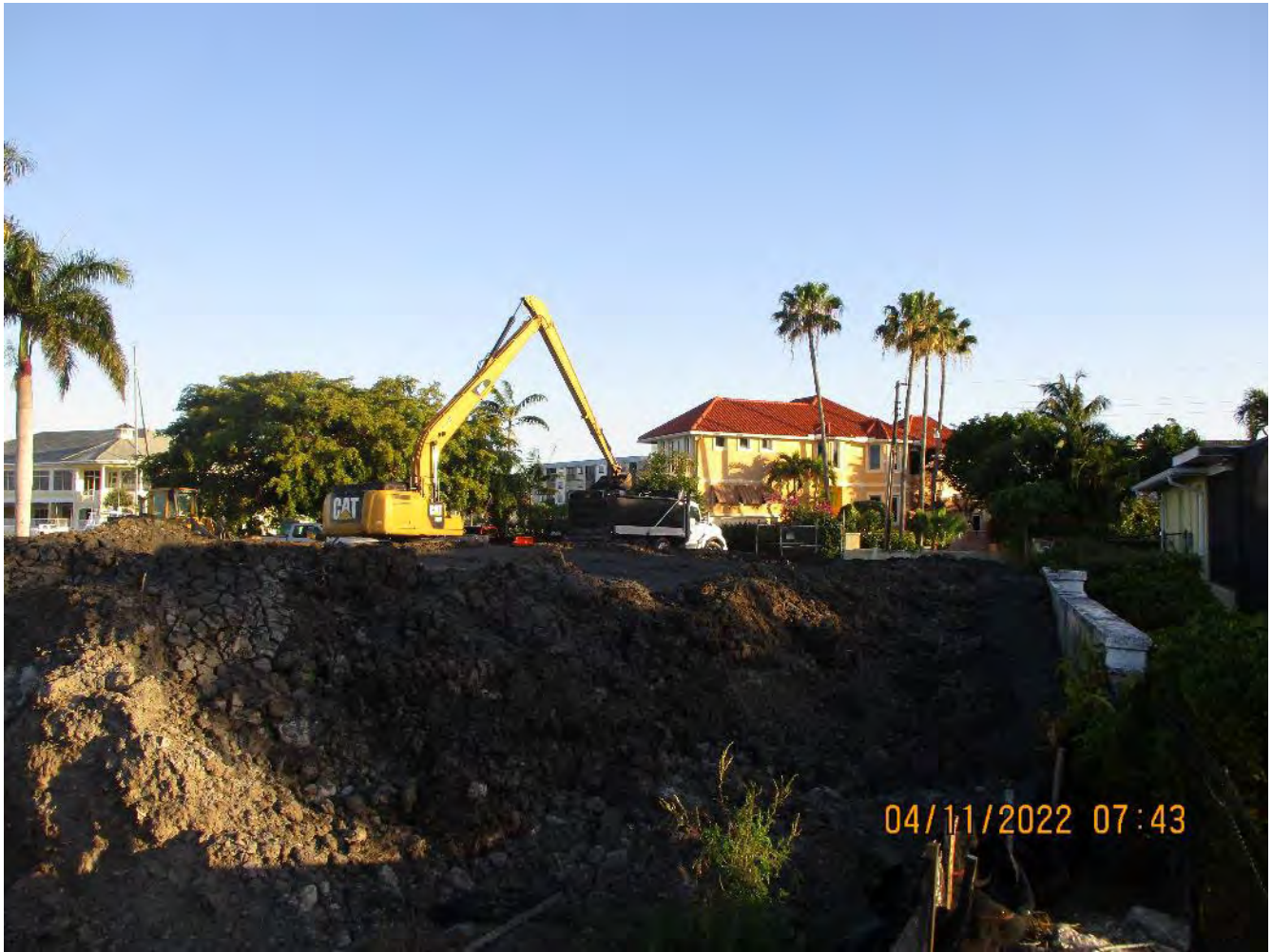
326 excavator transferring removed material from dewatering site to dump truck at 1300 Curlew Avenue
