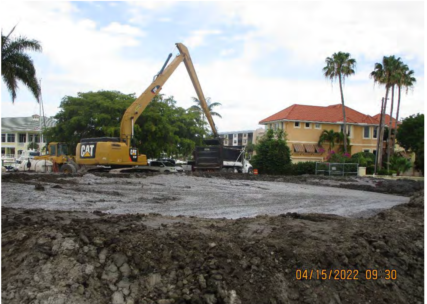
326 excavator transferring removed material from hopper to dewatering site at 1300 Curlew Avenue
