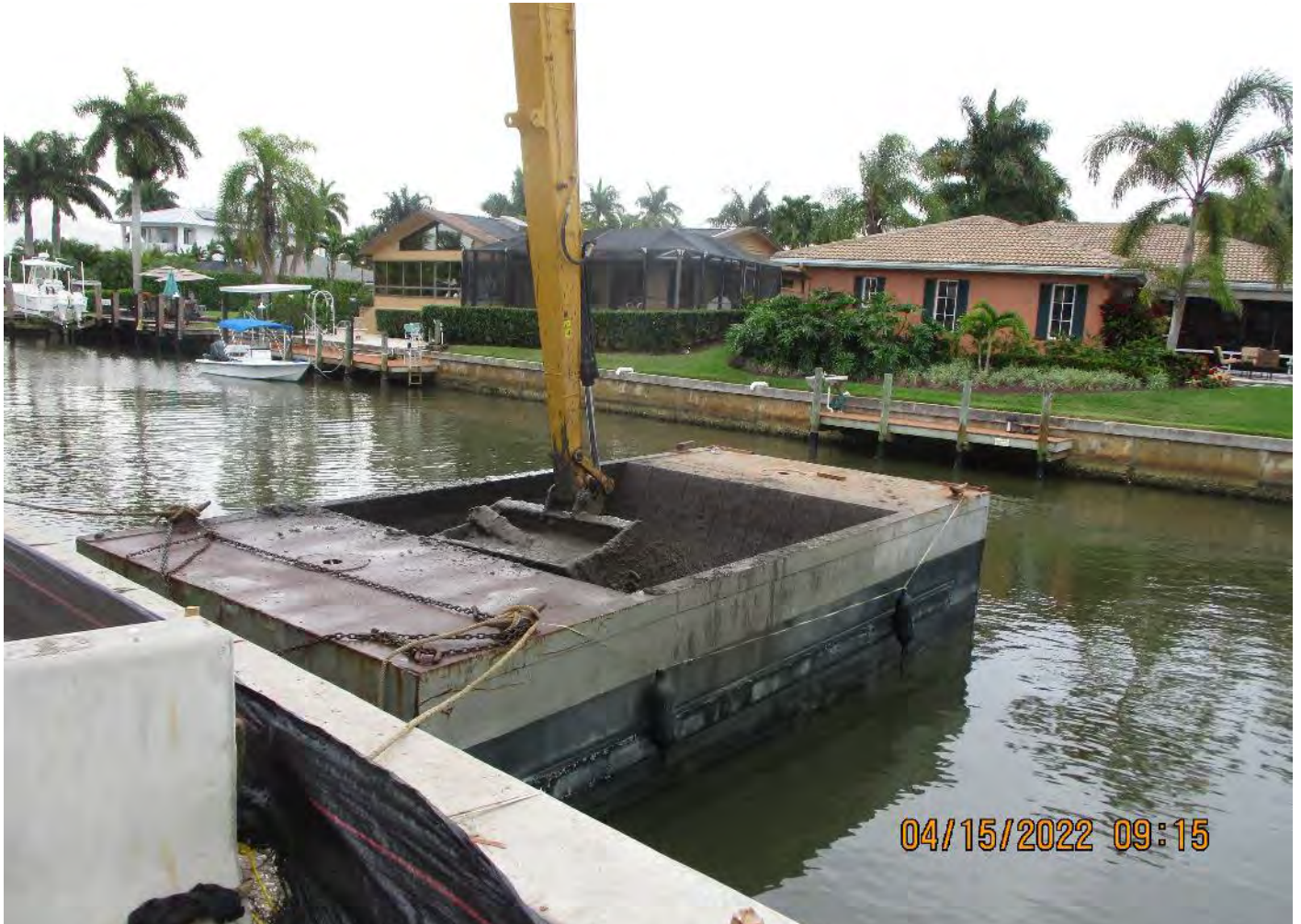
326 excavator transferring removed material from hopper to dewatering site at 1300 Curlew Avenue
