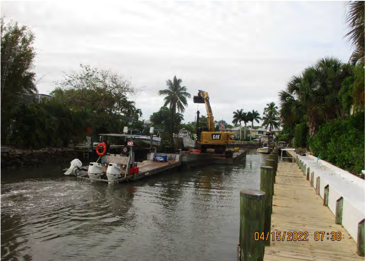
323 excavator lifting spud to allow push boat to mobilize barge and hopper in Canal AA-AA
