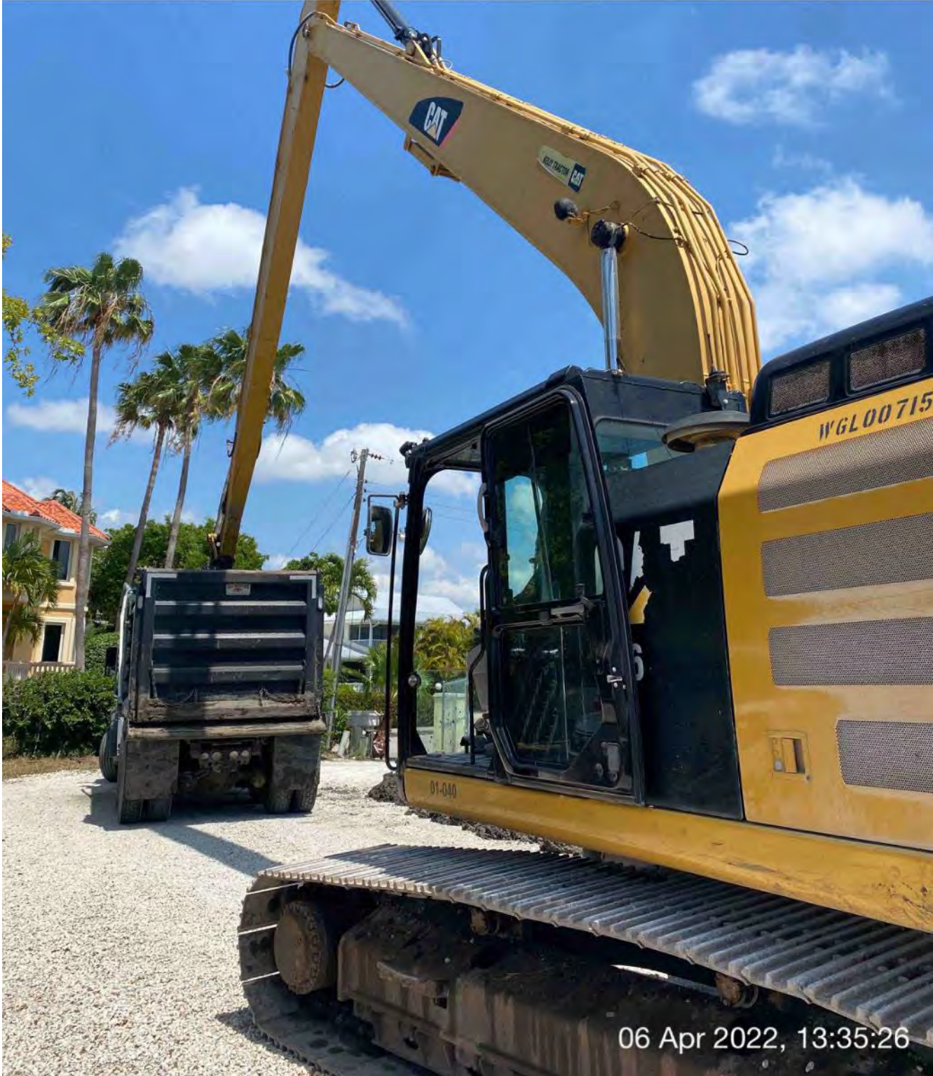
326 excavator transferring removed material from dewatering site at 1300 Curlew Avenue to dump truck
