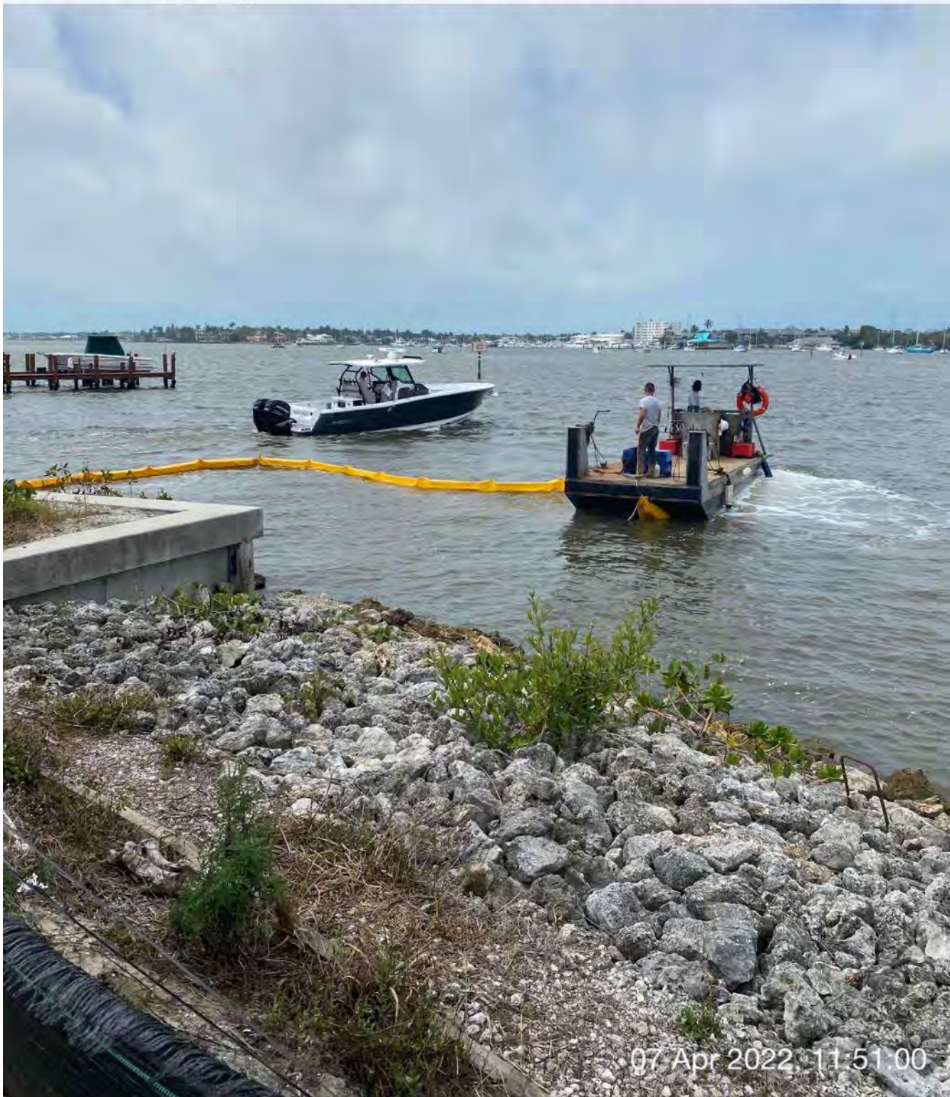
Push boat opening turbidity curtain to allow resident to exit Canal CC-CC
