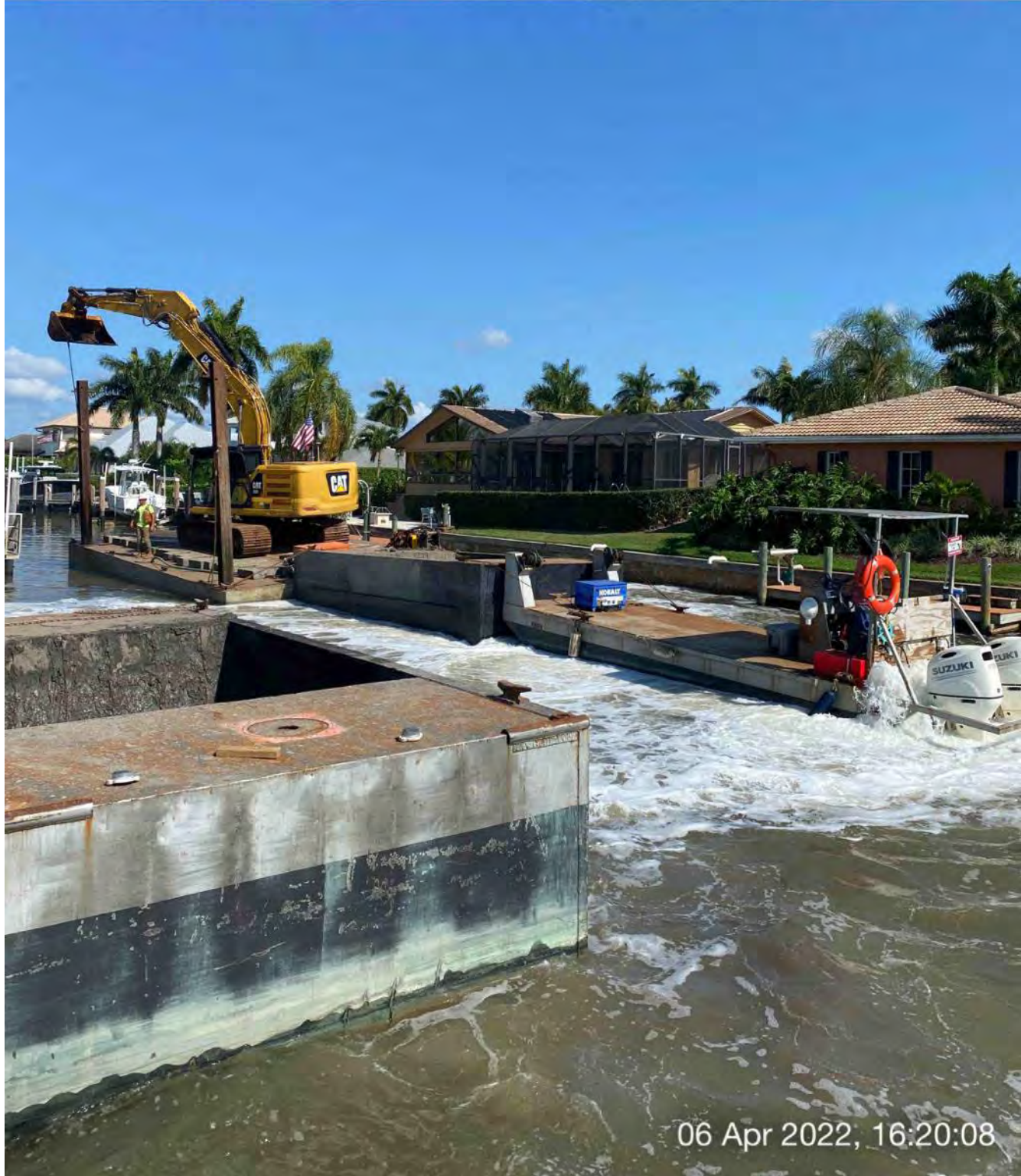
323 excavator lifting spud to allow push boat to mobilize barge and hopper at station 2+00
