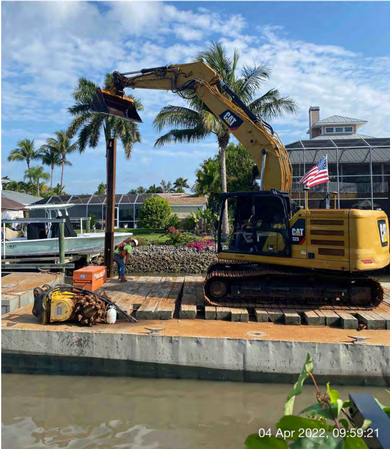
323 excavator lifting spud to allow push boat to mobilize barge at station 9+00
