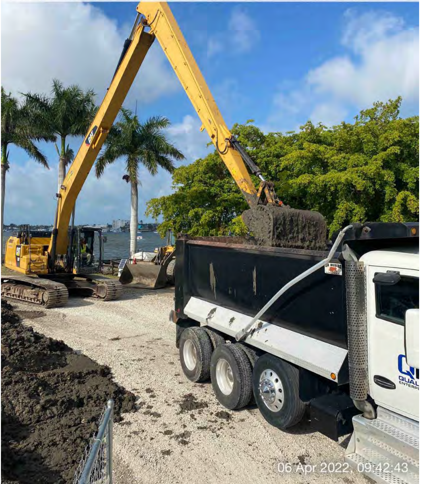
326 excavator transferring removed material from dewatering site at 1300 Curlew Avenue to dump truck
