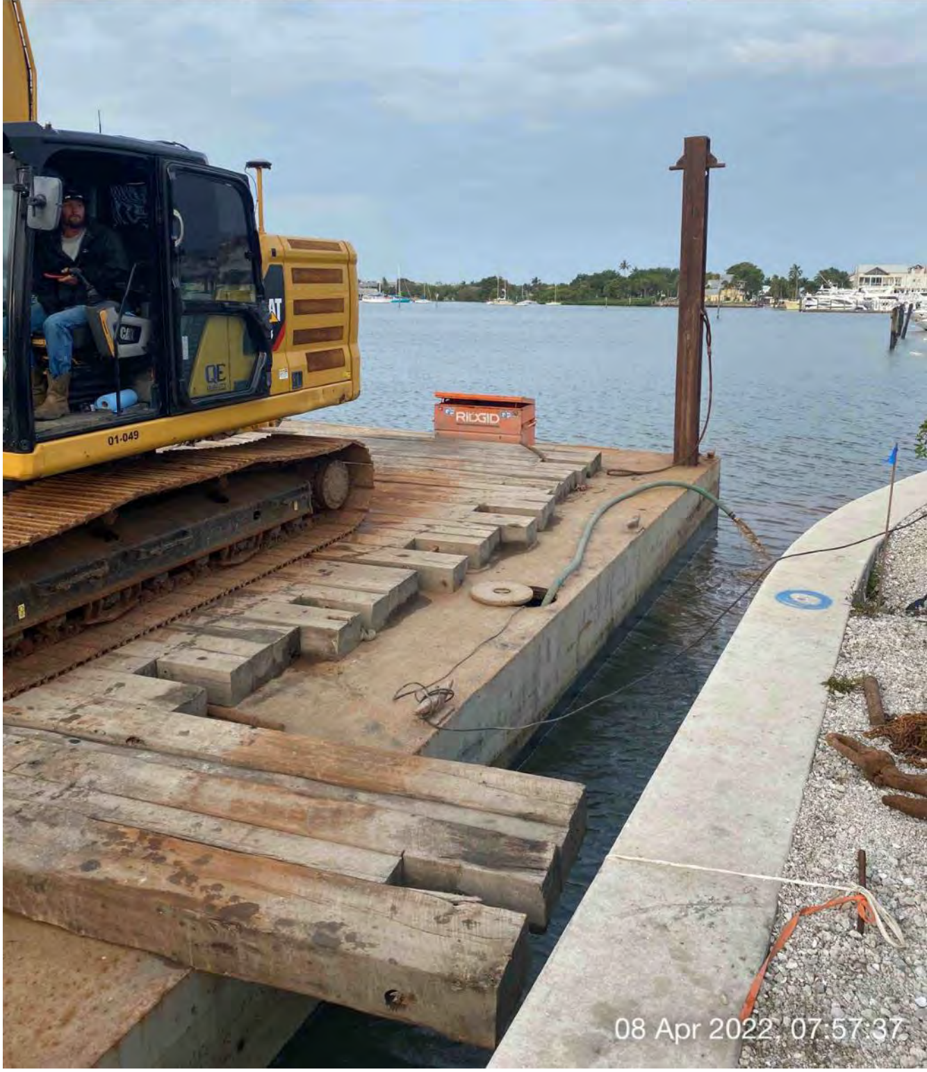
Pumping water out of the bottom of the barge stated at station 1+00
