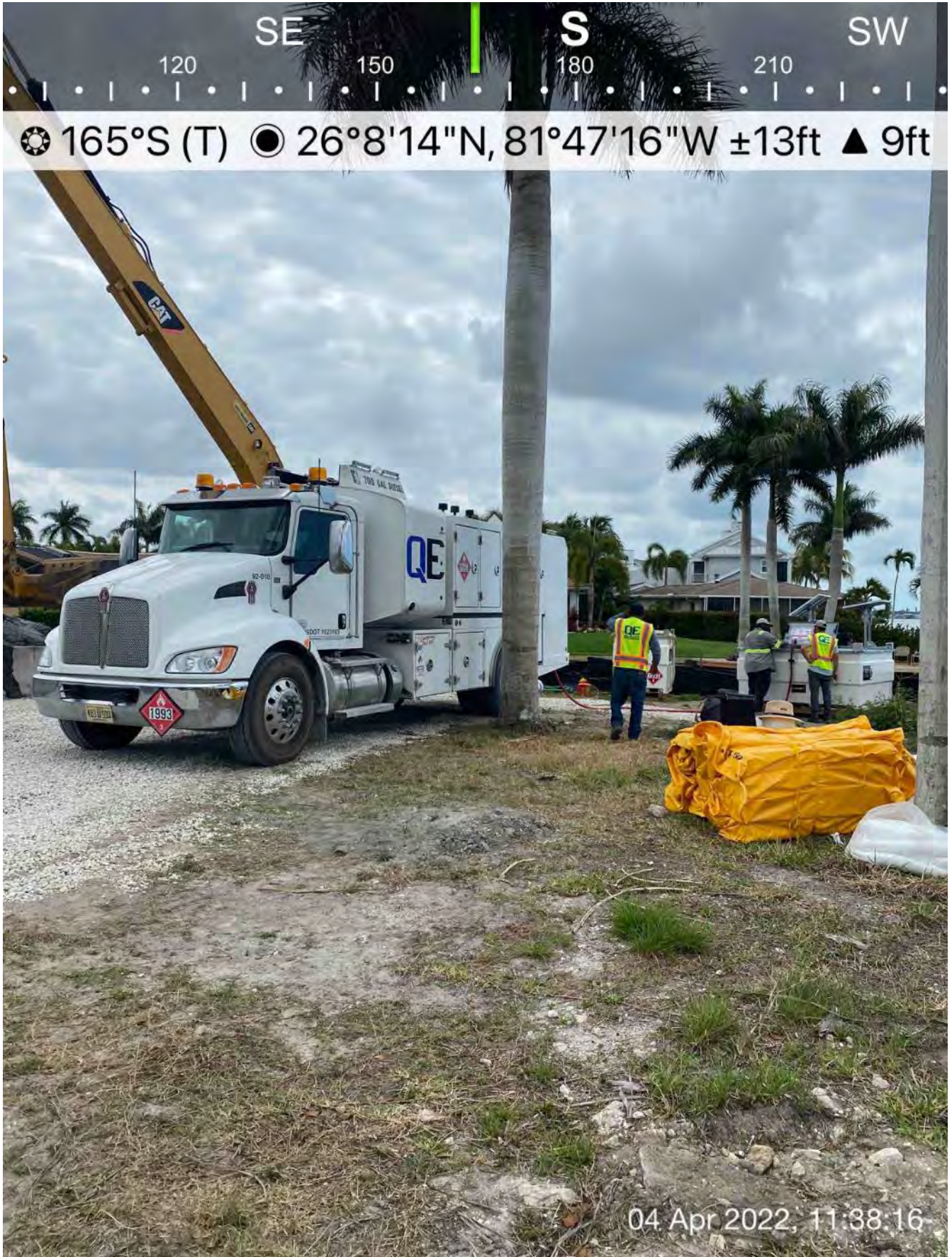
Mechanic truck refilling the fuel cubes at 1300 Curlew Avenue
