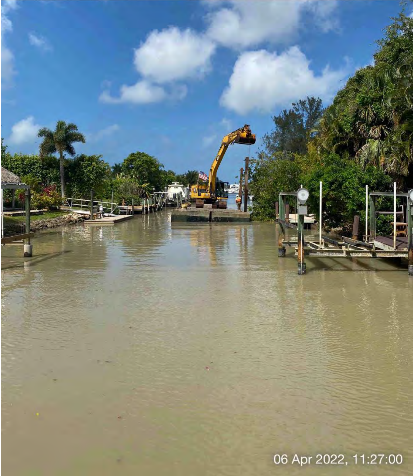
323 excavator lifting spud to allow push boat to mobilize barge at station 13+00
