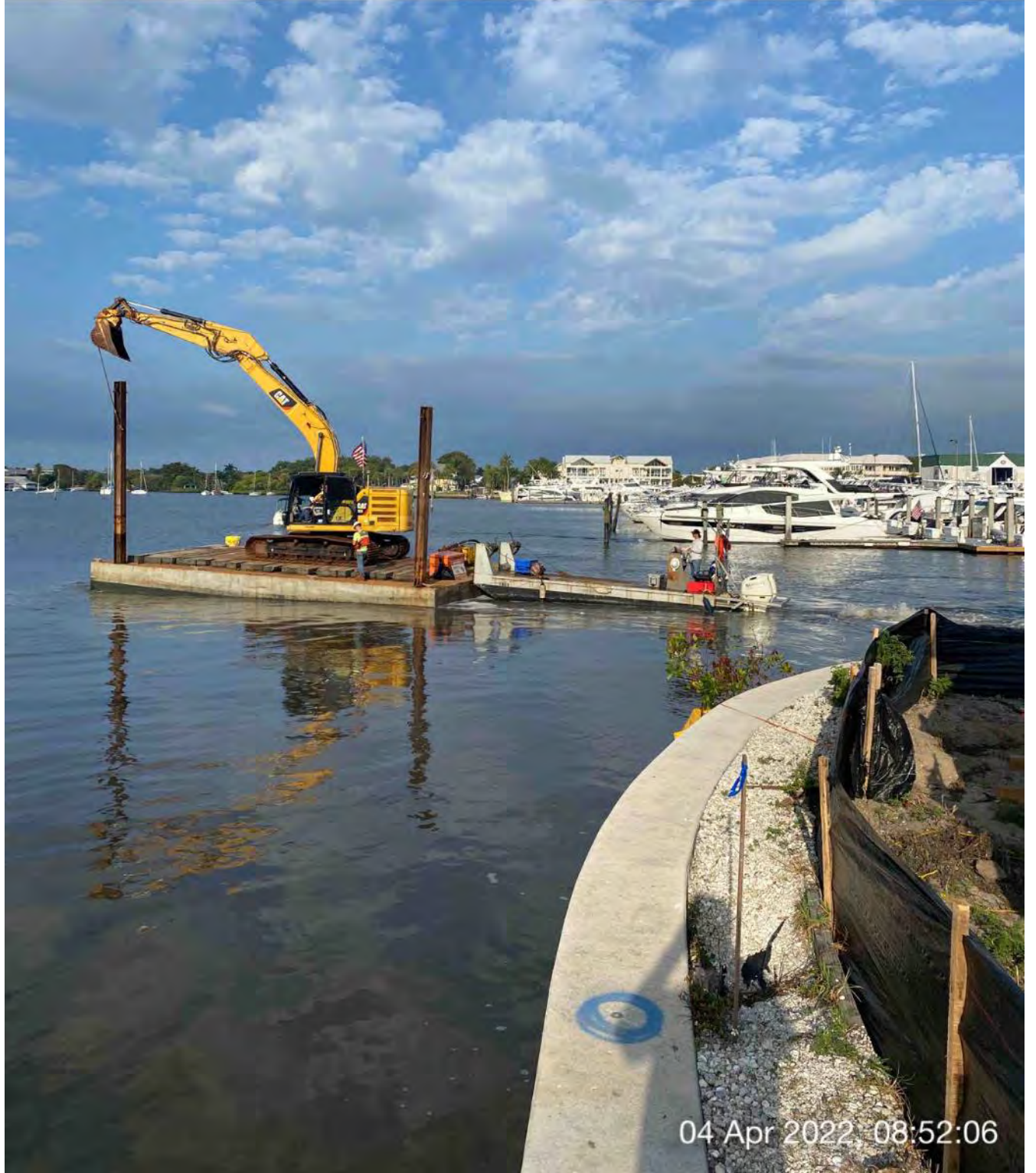
Push boat transporting barge and 323 excavator from Canal CC-CC to Canal BB-BB
