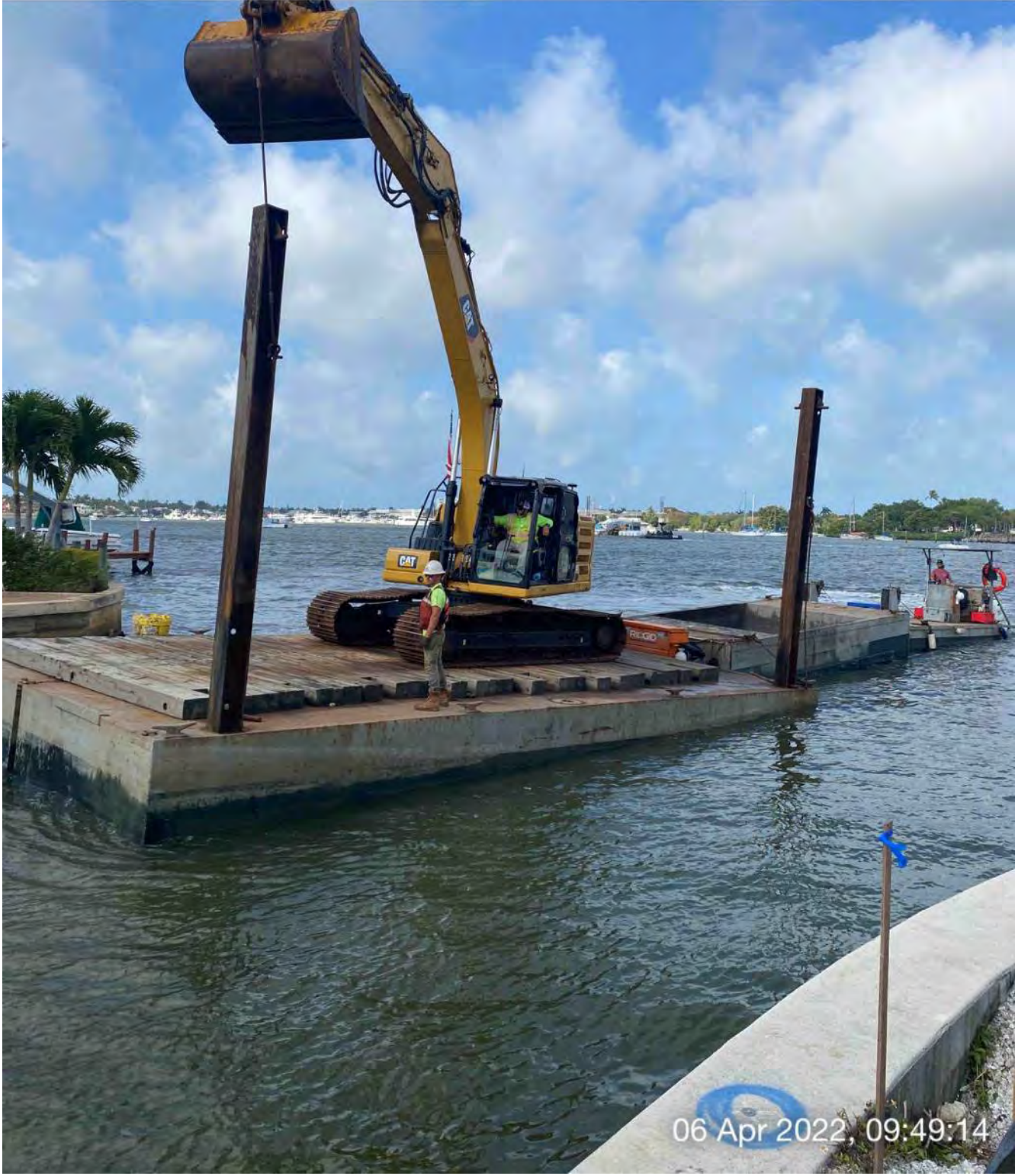
323 excavator lifting spud to allow push boat to mobilize barge at the mouth of Canal CC-CC
