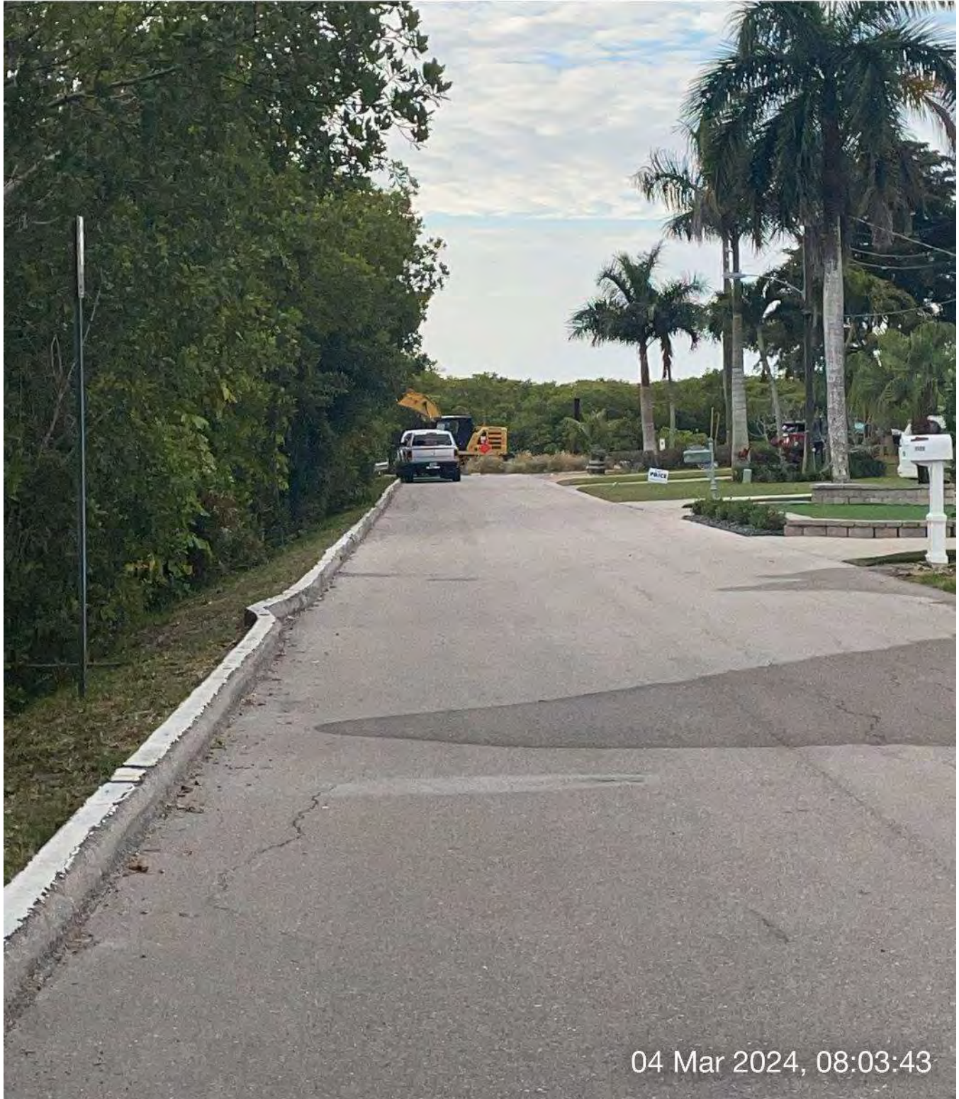
Contractor waiting on mechanic to arrive.
