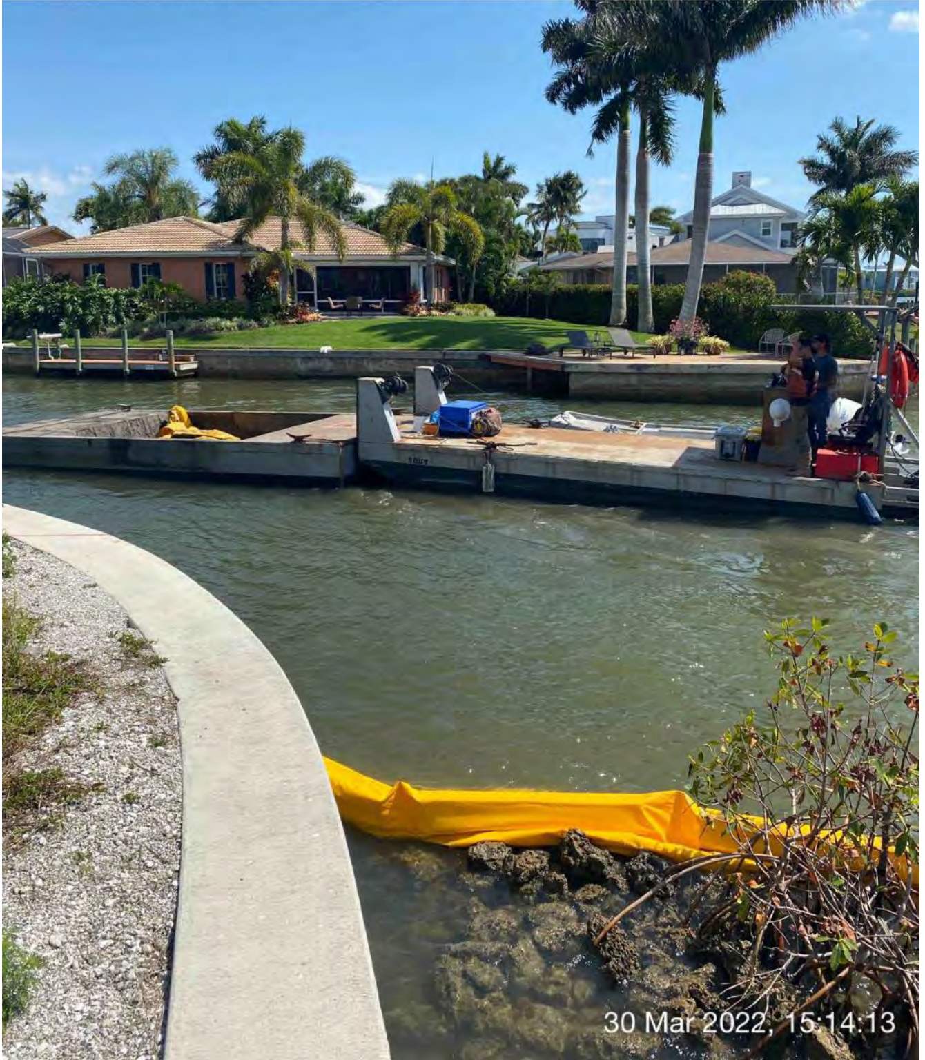
Push boat dropping off full hopper of removed material and taking empty hopper back to barge in Canal BB-BB
