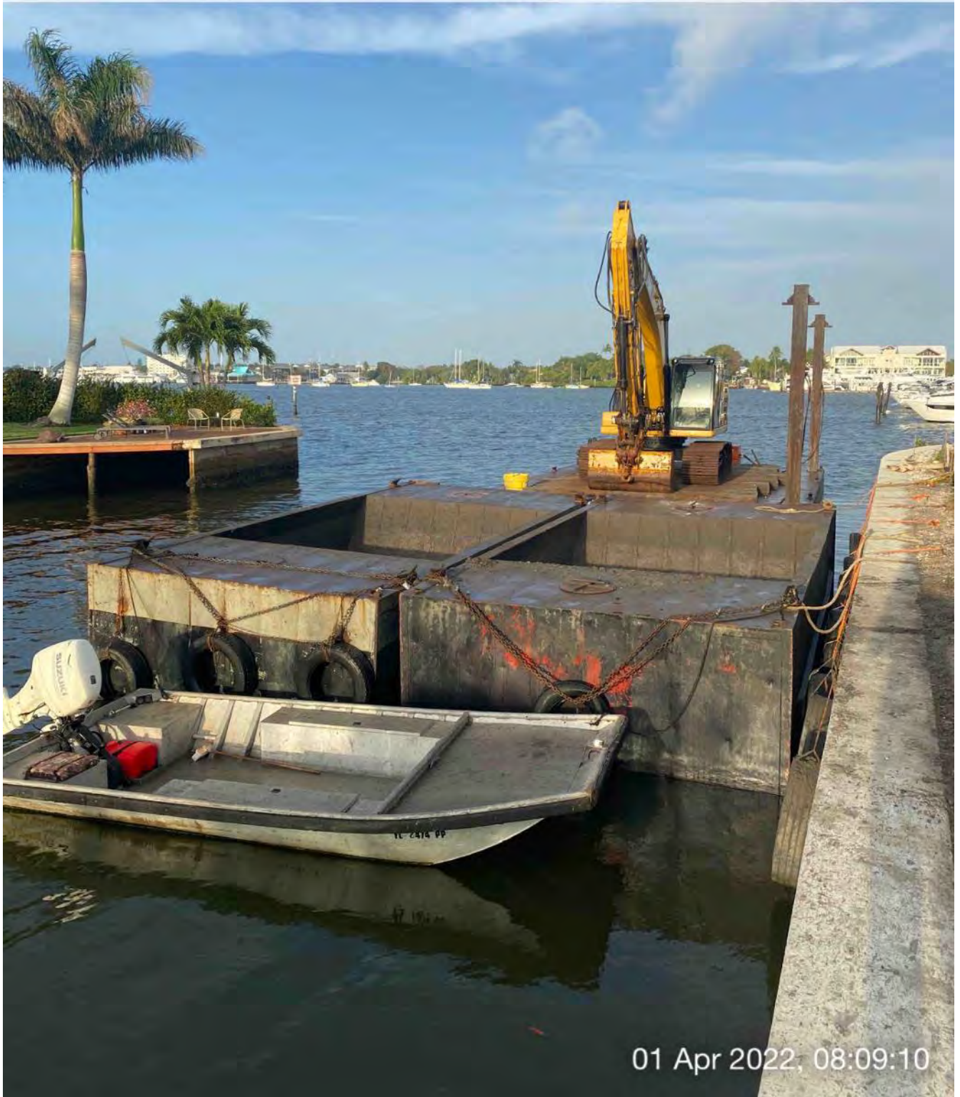
Support boat, 2 hoppers, barge, and 323 excavator stationed in Canal CC-CC between stations 1+00 and 2+00
