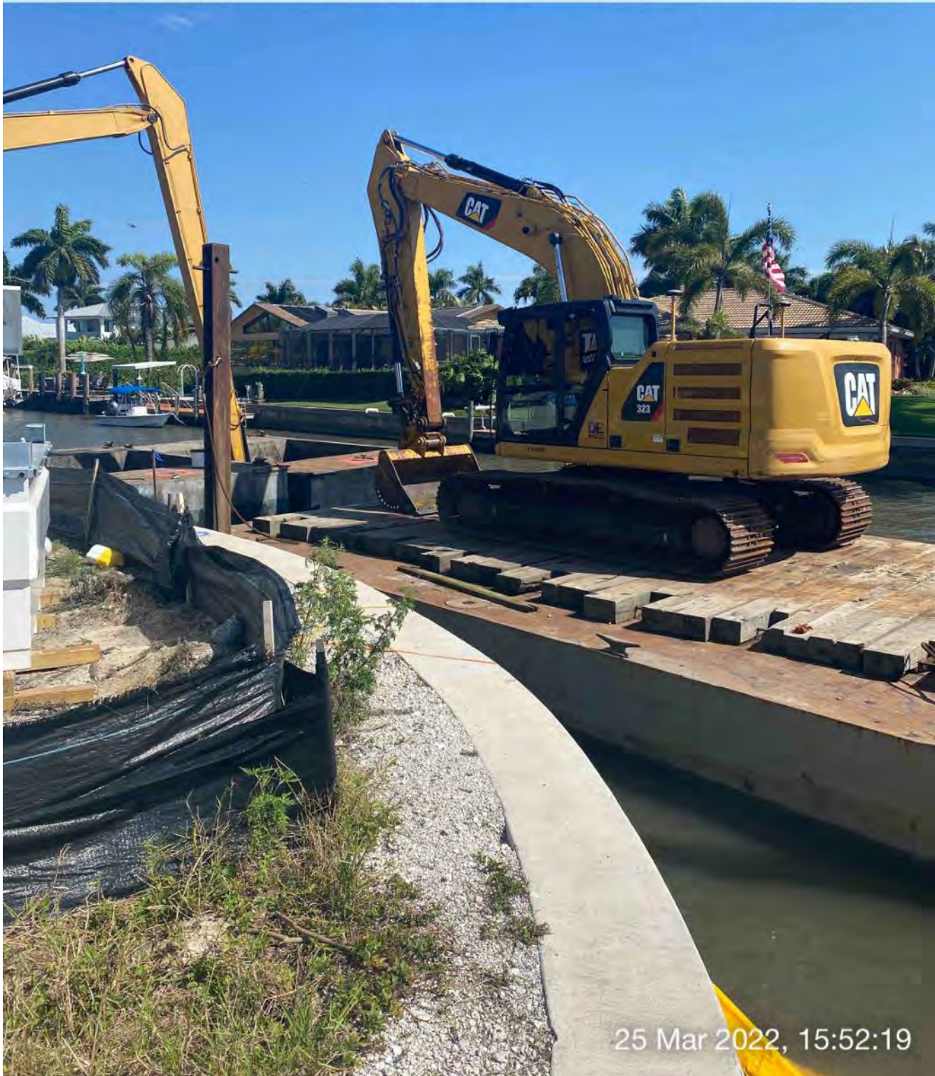
323 excavator, barge, and two hoppers tied up in Canal CC-CC at station 1+00
