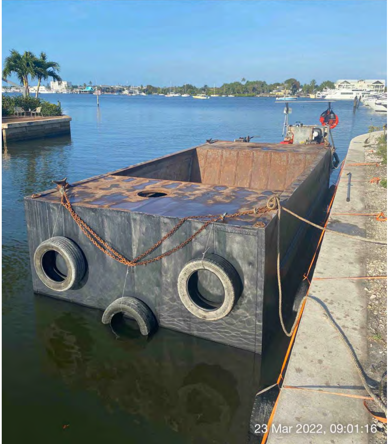
New hopper with tires attached tied to barrier elements at station 1+50 in Canal CC-CC
