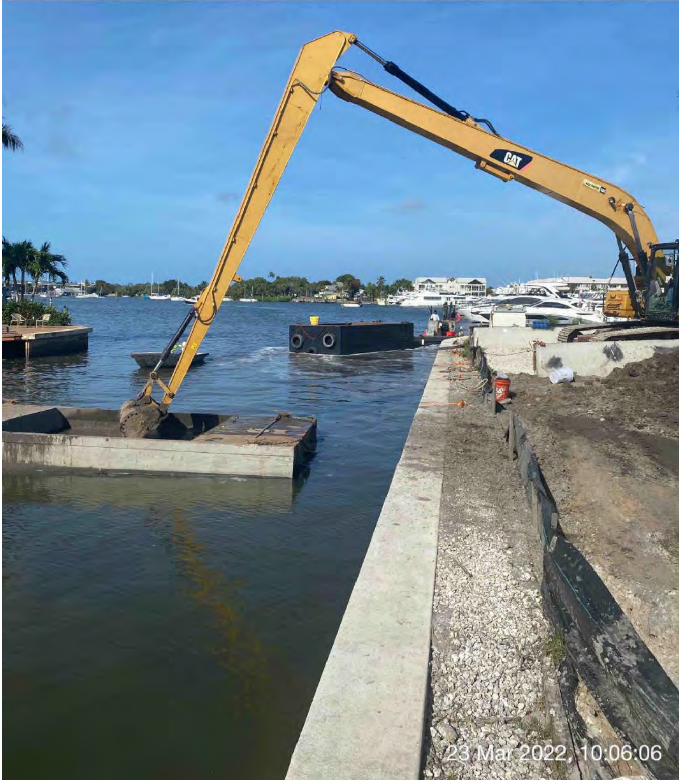
326 excavator holding old hopper in place while push boat transports new hopper to Barge in Canal BB-BB
