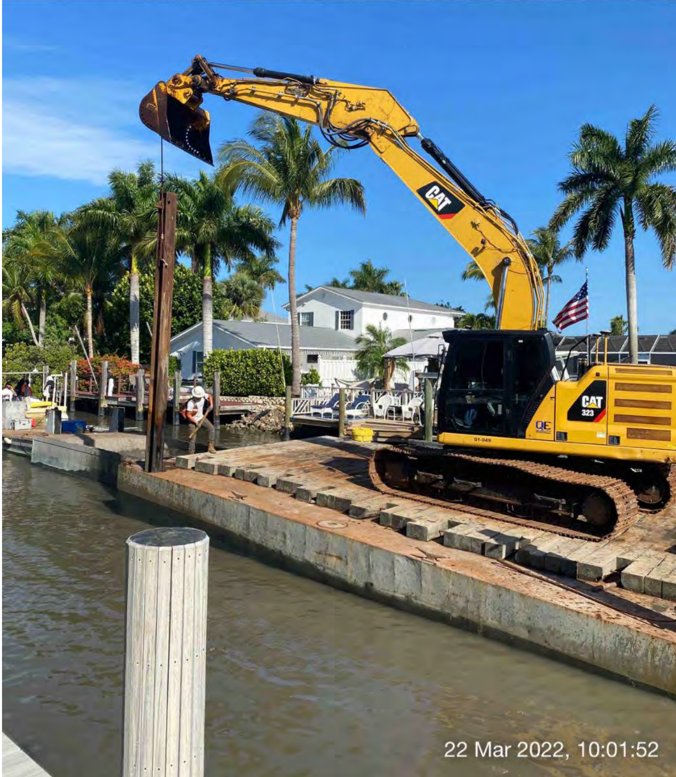
323 excavator lifting spud to allow push boat to mobilize barge at station 9+50 in Canal CC-CC
