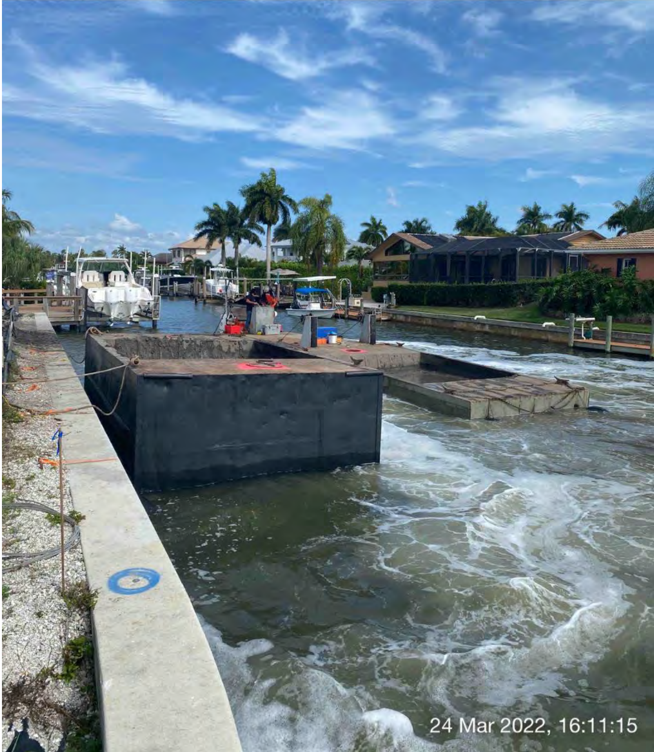
Push boat transporting full hopper back to Canal CC-CC station 1+50 and picking up empty hopper
