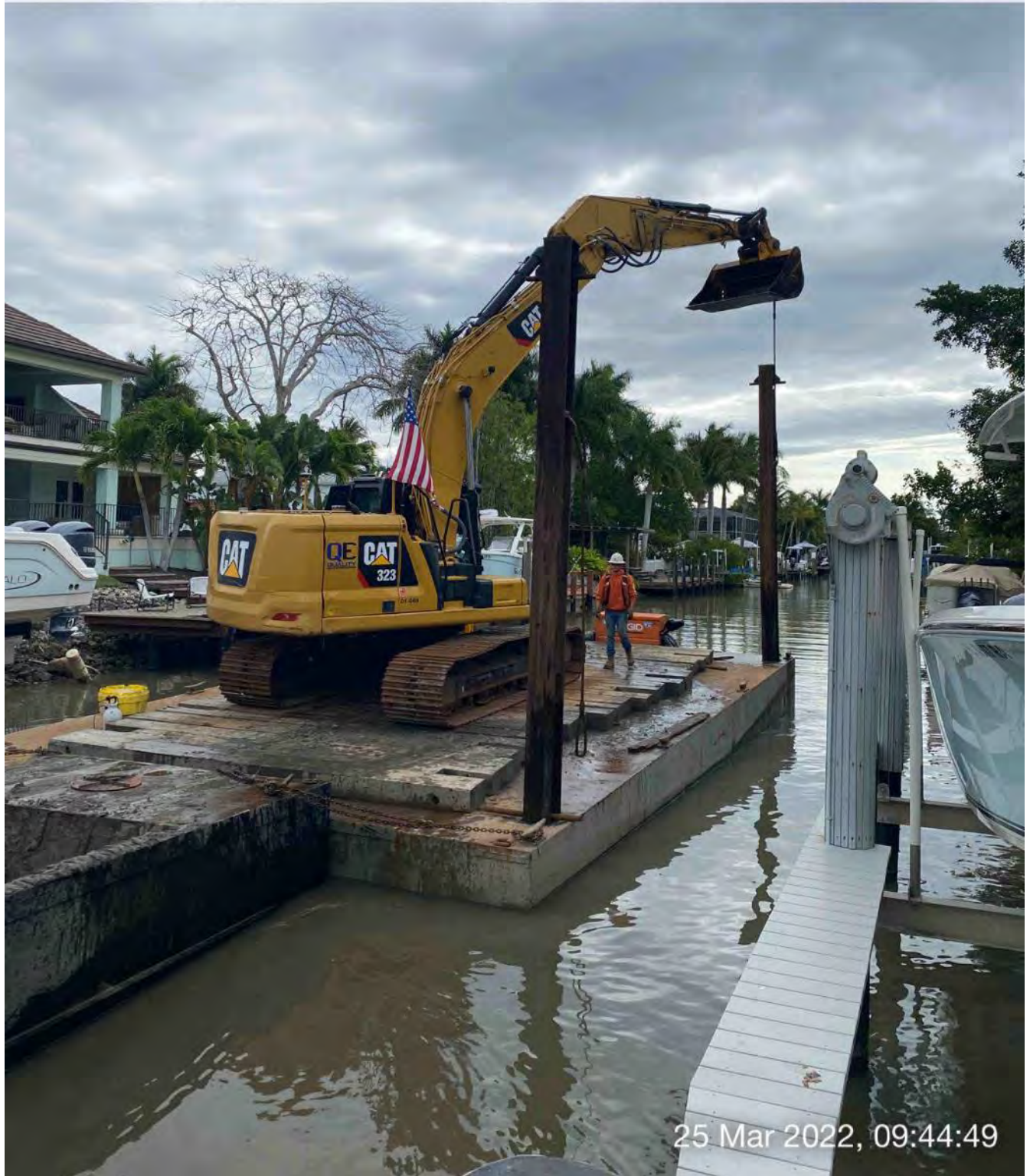
323 excavator lifting spud to allow push boat to mobilize barge at station 5+50 in Canal CC-CC
