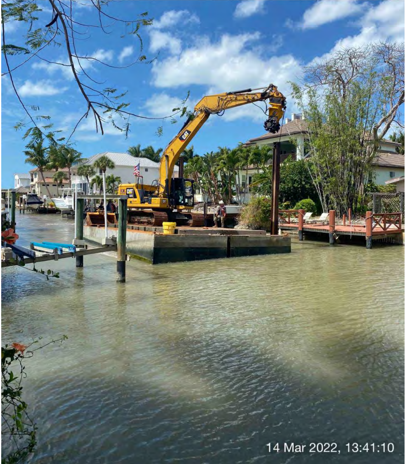
323 excavator lifting spud to allow push boat to mobilize barge at station 6+00
