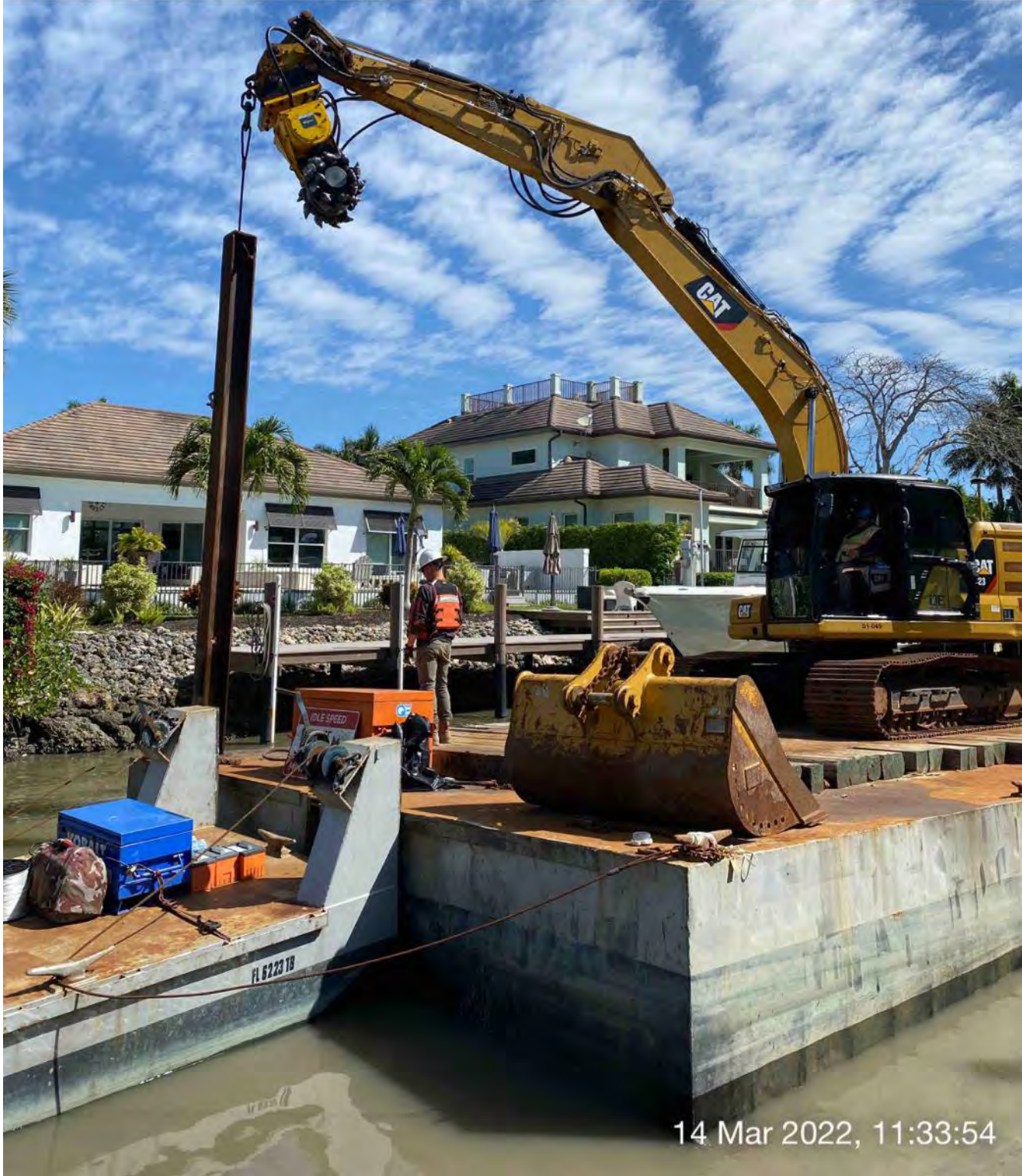
323 excavator lifting spud to allow push boat to mobilize barge at station 4+50
