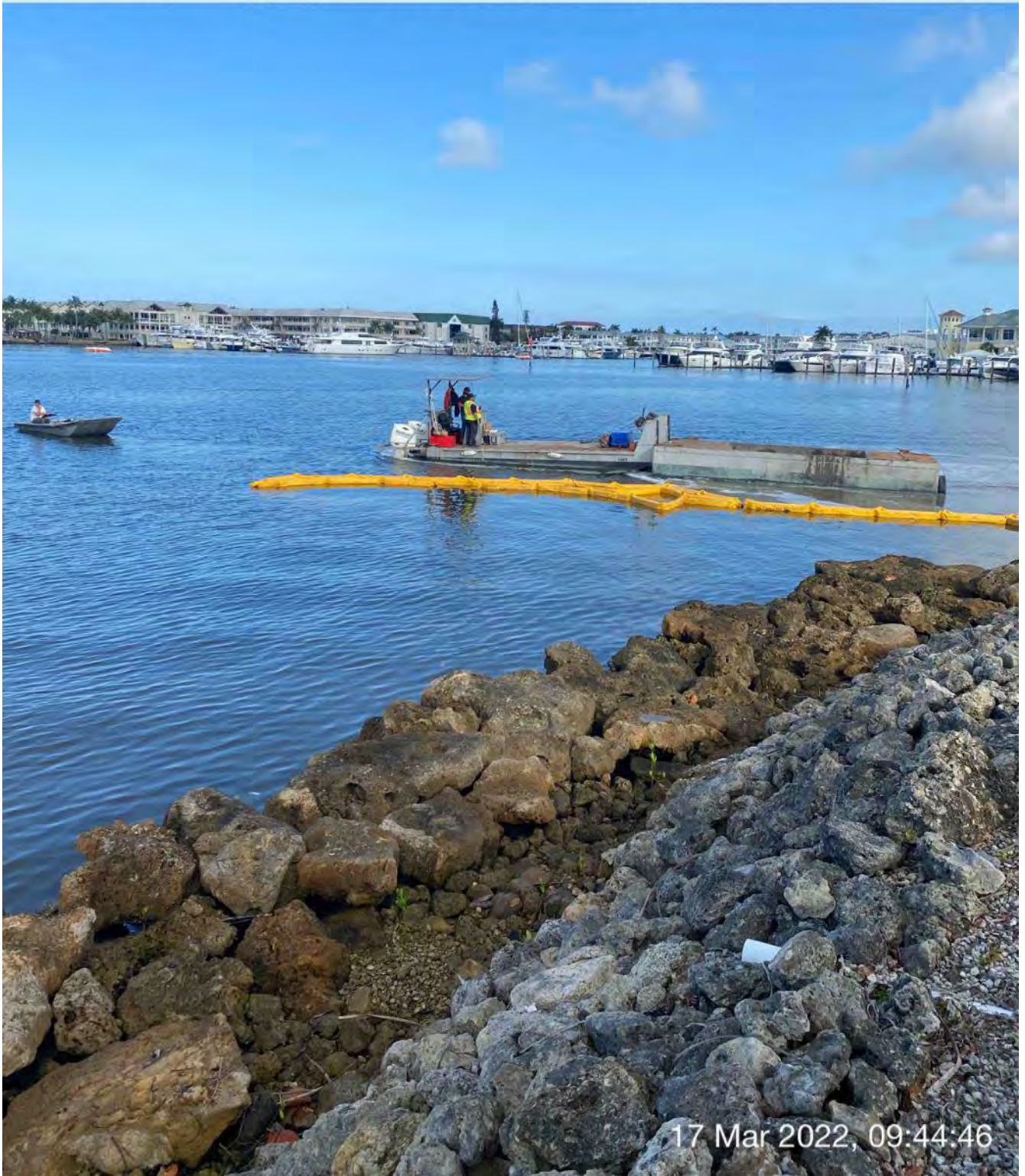
Support boat opening turbidity curtain to allow push boat to exit Canal BB-BB with hopper
