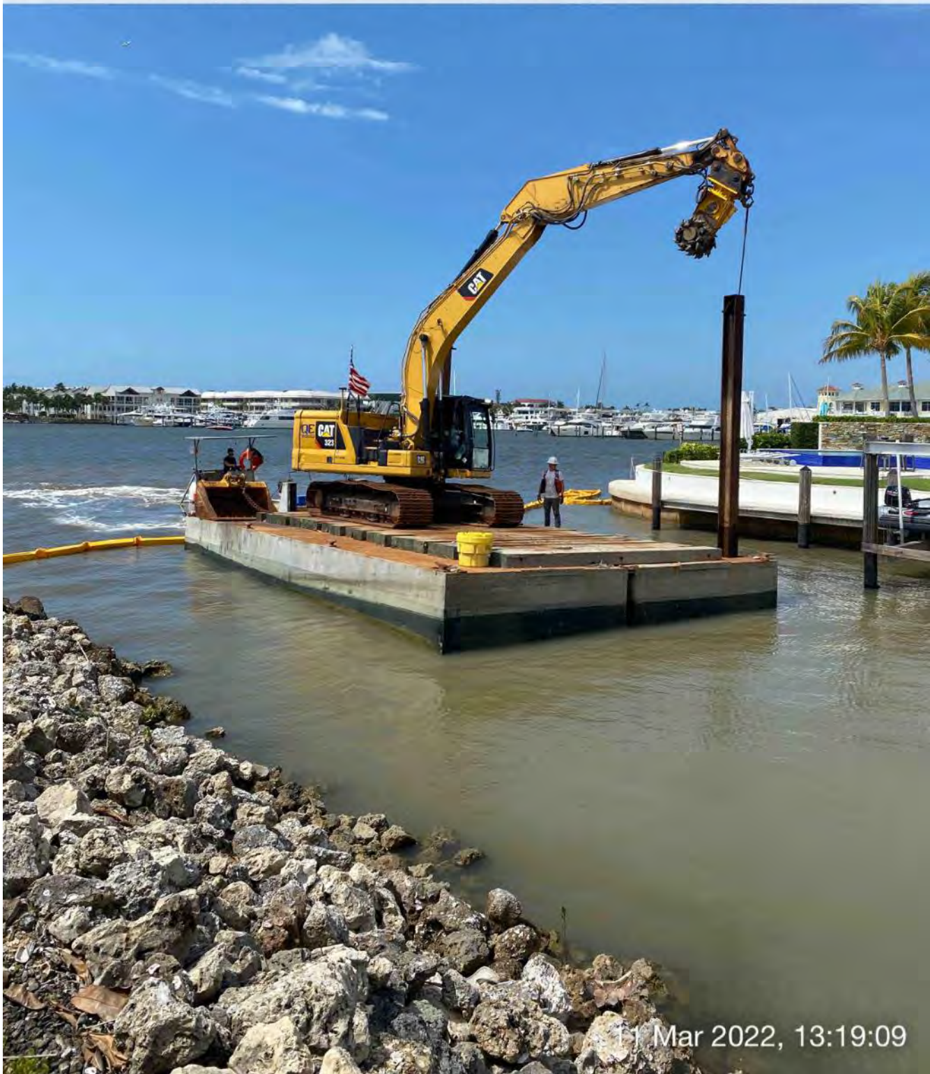
323 excavator lifting spud to allow push boat to mobilize barge at station 1+25
