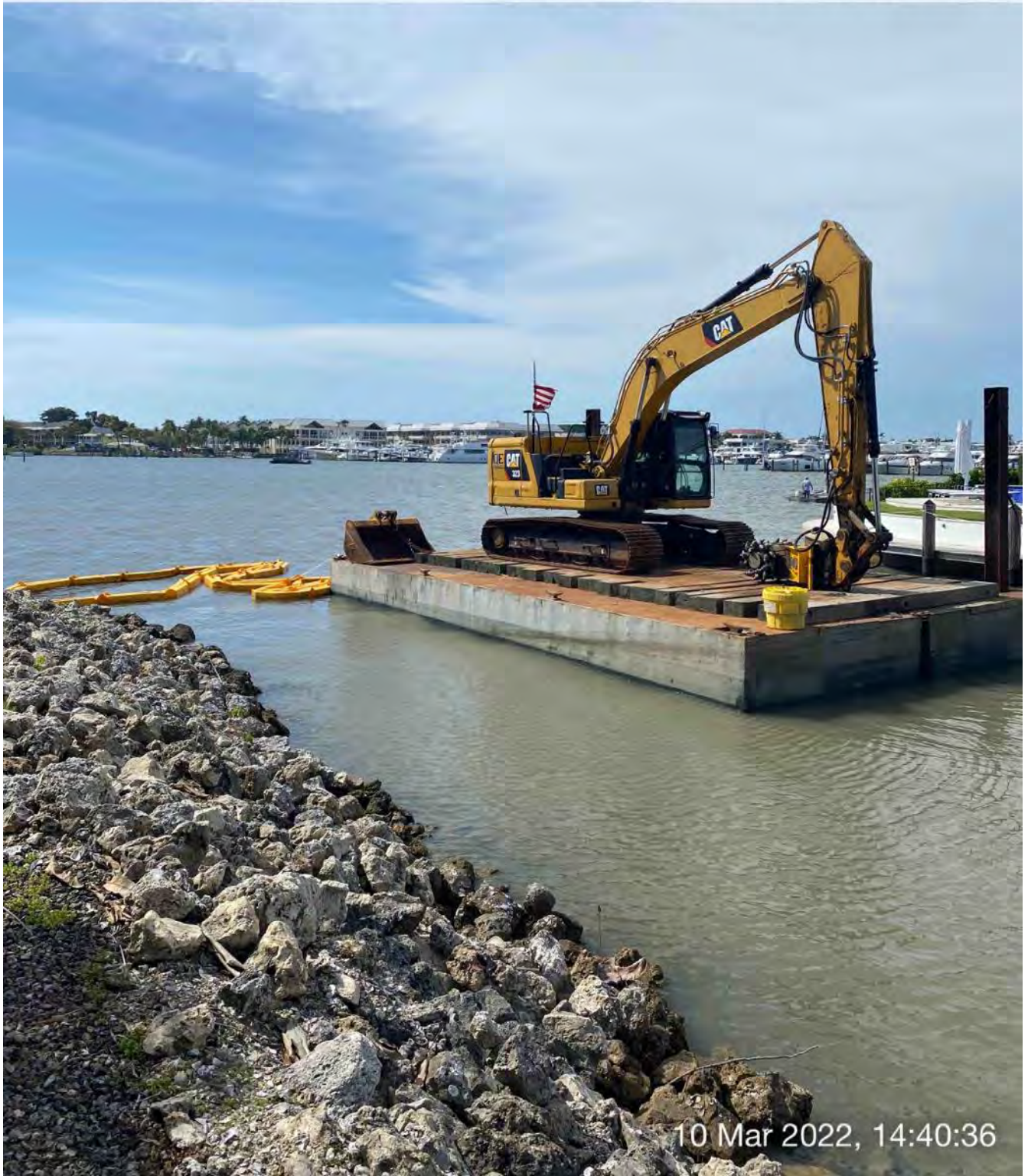
323 excavator on barge at station 1+50 with turbidity curtain tied back to south side of barge
