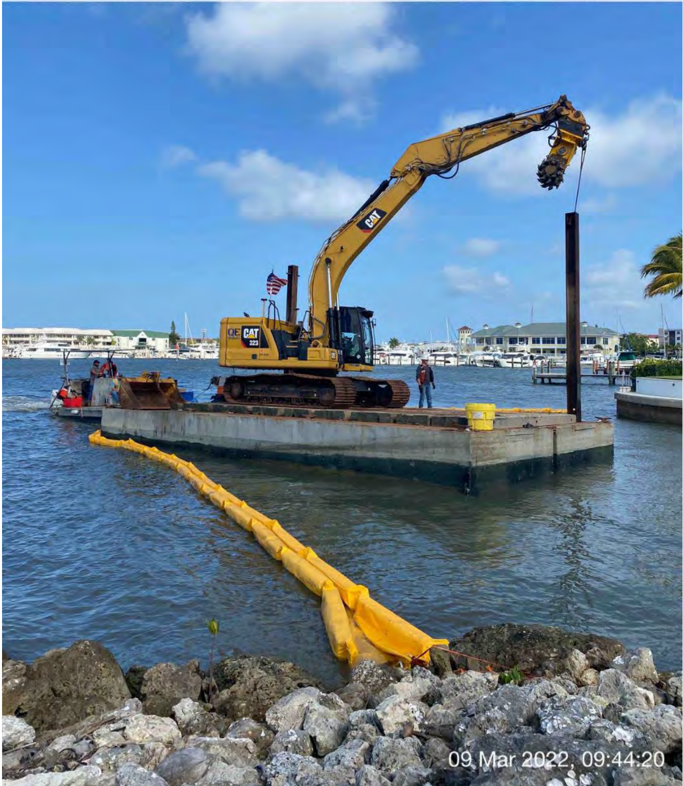
323 excavator lifting spud to allow push boat to mobilize barge at station 1+00
