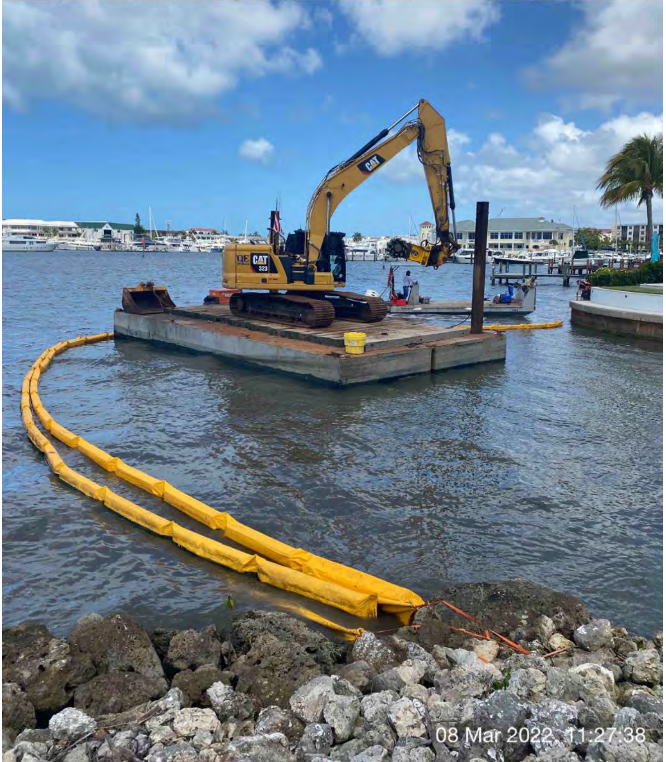
323 excavator with Epiroc grinder on barge at station 1+00. Push boat being used to install turbidity curtain.
