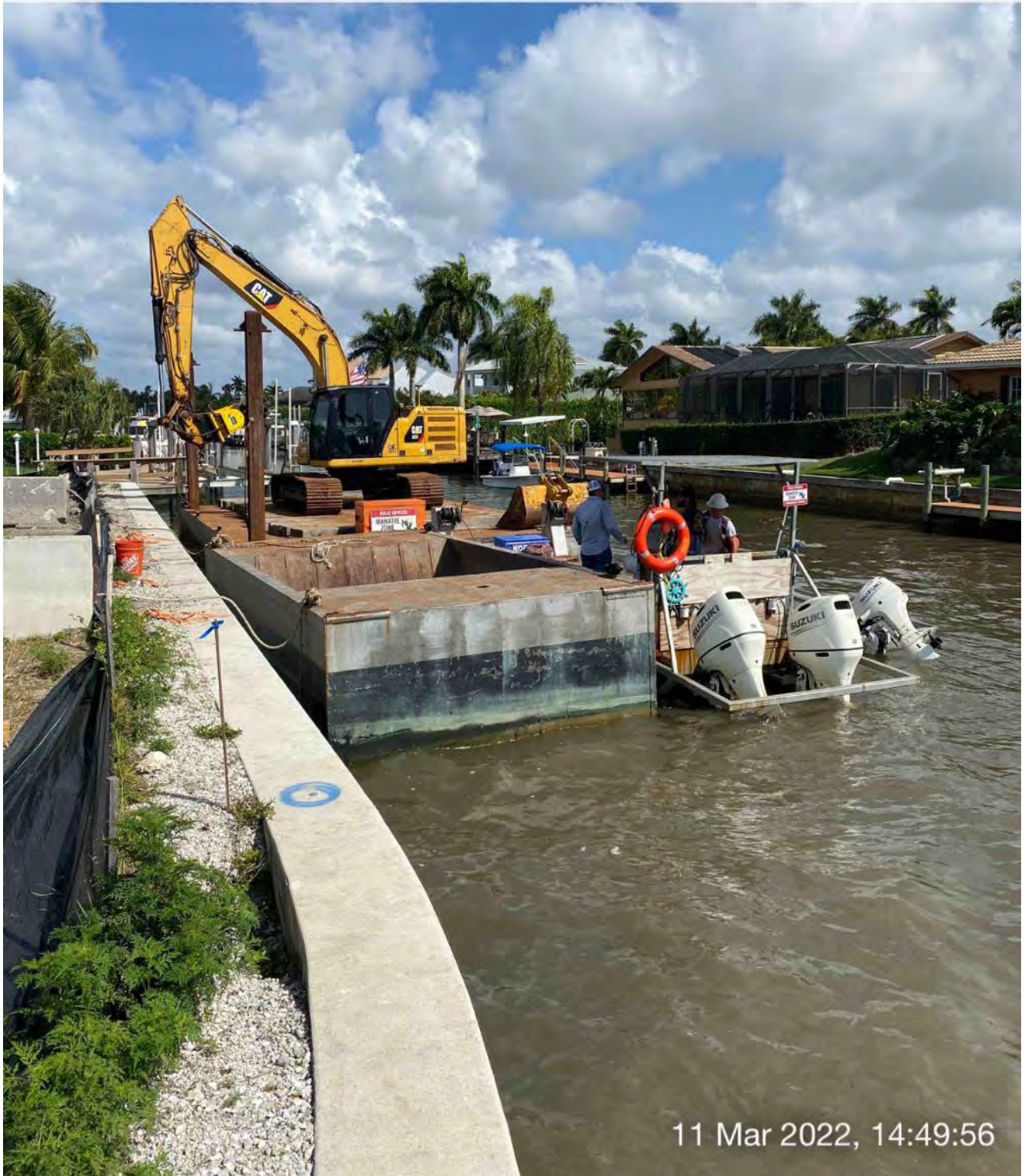
323 excavator on barge, push boat, support boat, and hopper staged in Canal CC-CC at station 1+50
