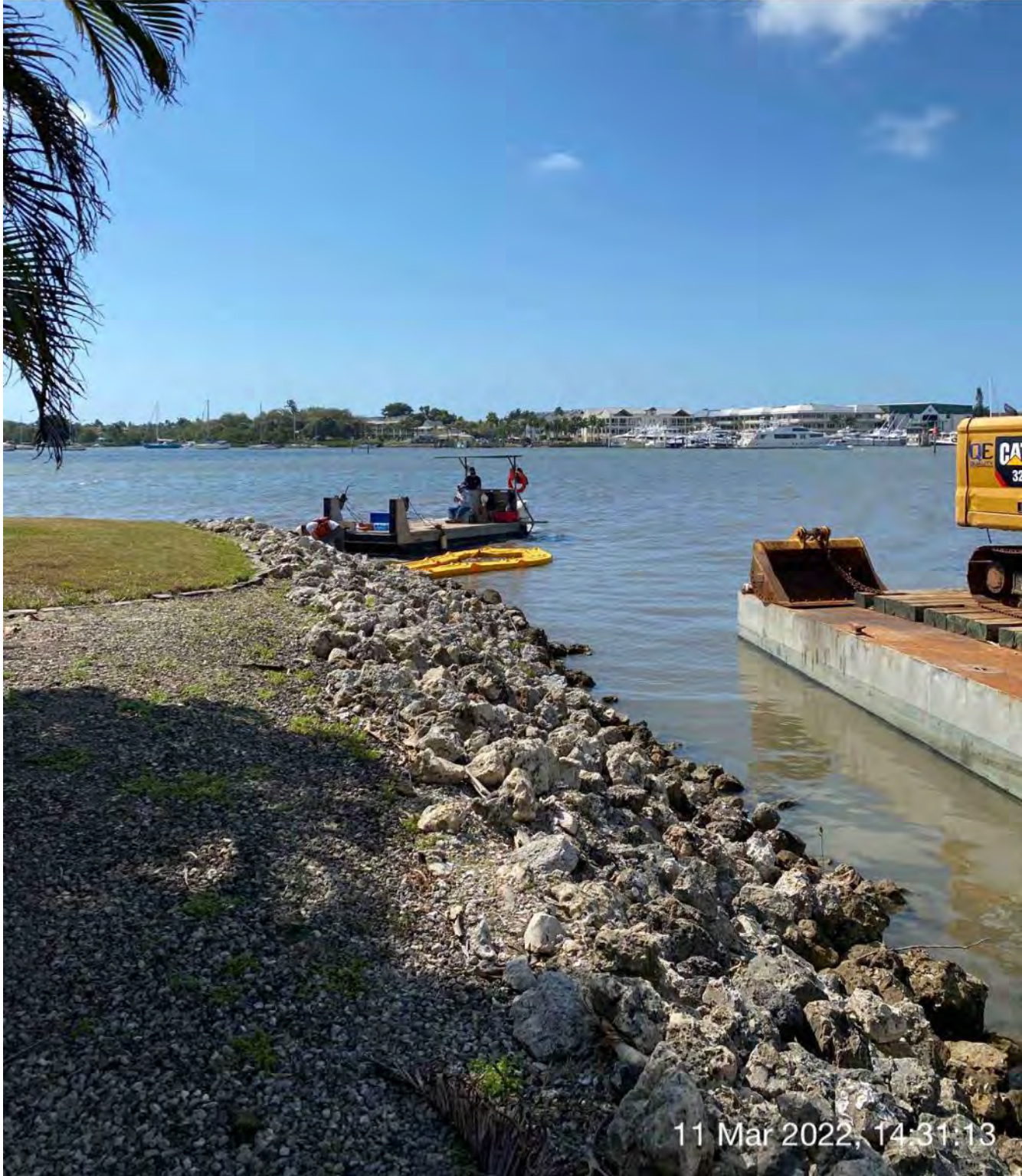
Contractor using push boat to tie turbidity curtain up to rocks on south side of canal at station 1+00
