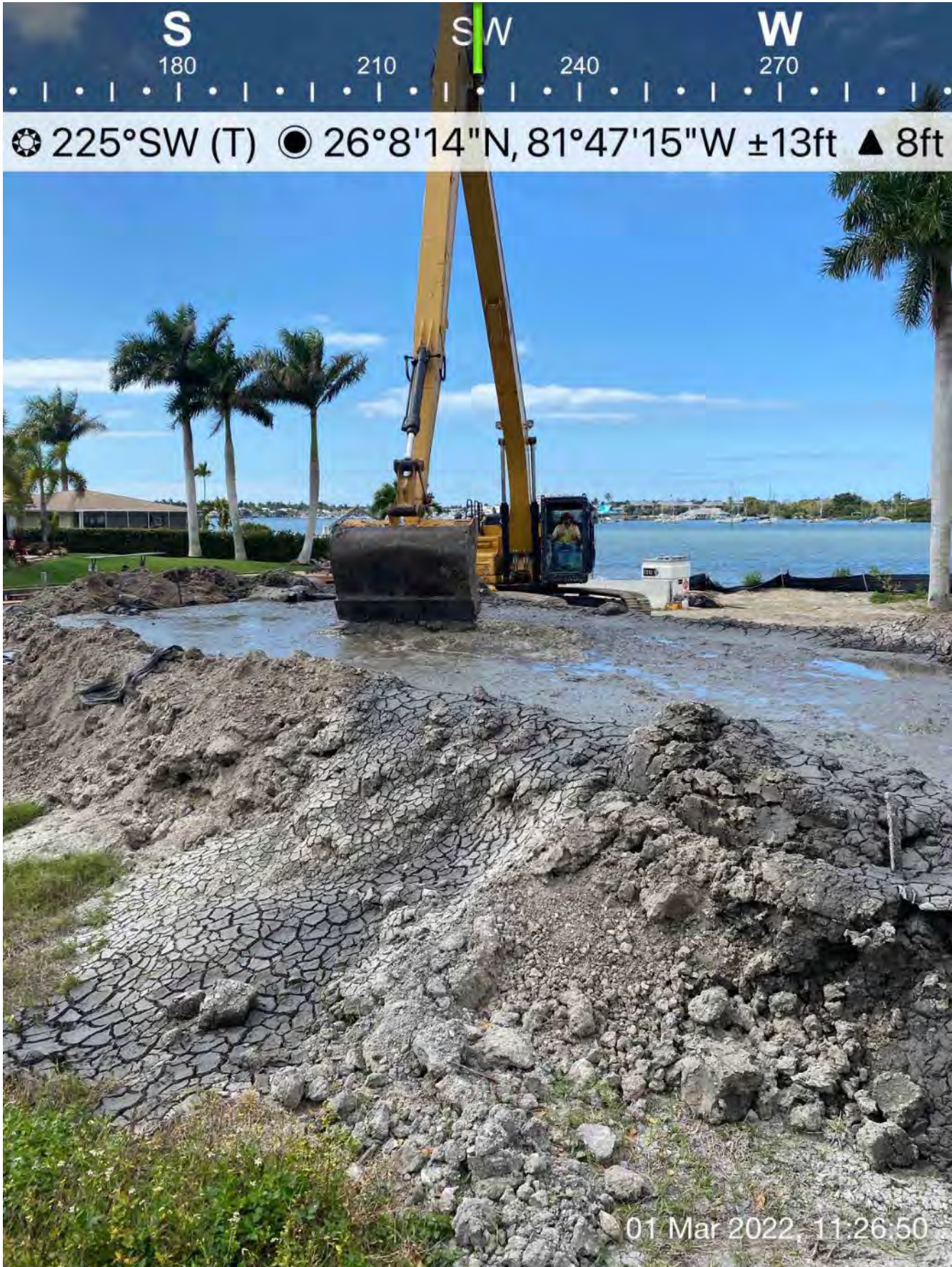
326 excavator transferring removed material from hopper to dewatering site at 1300 Curlew Avenue
