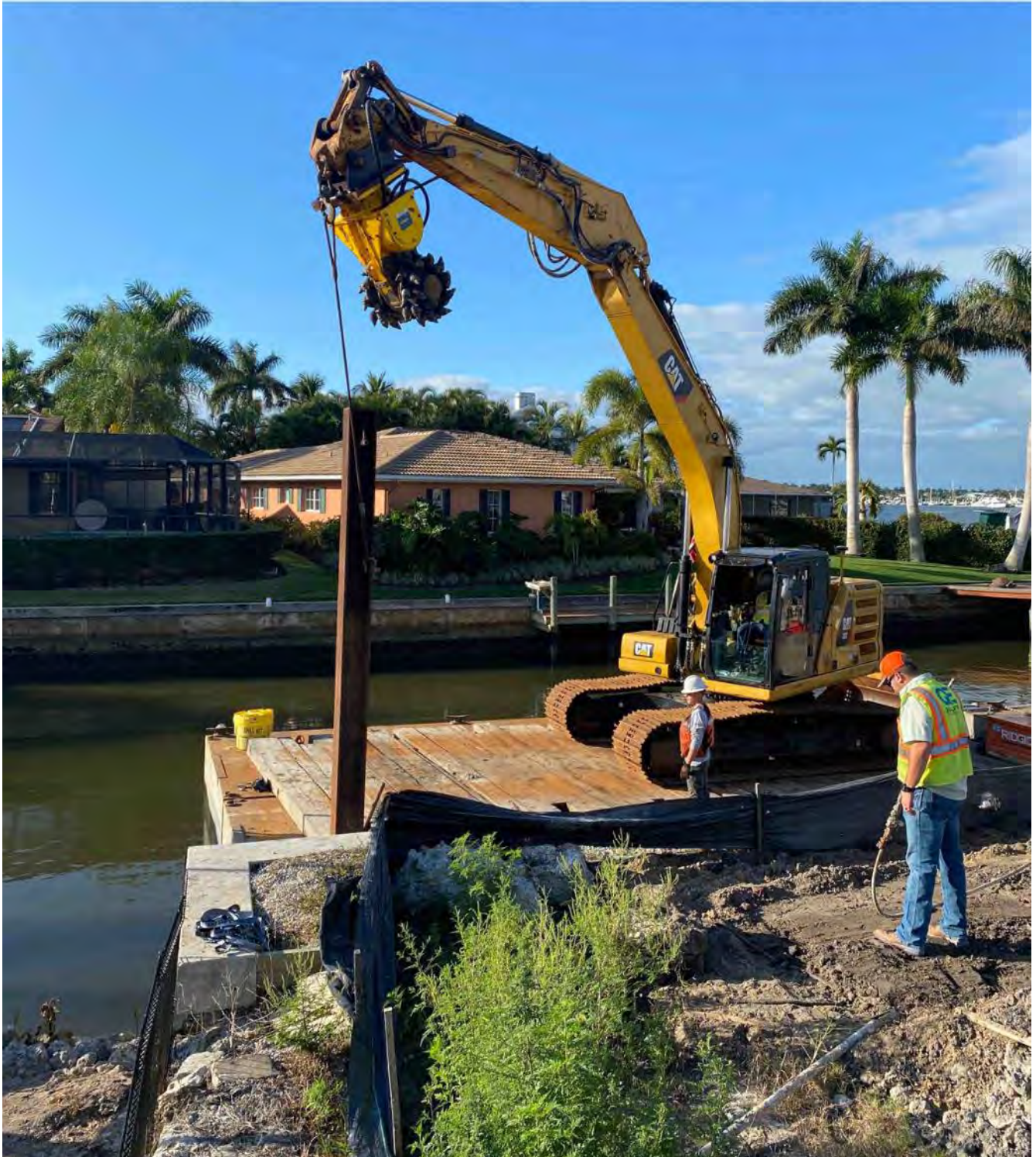
323 excavator lifting spud to allow push boat to mobilize barge at station 2+00
