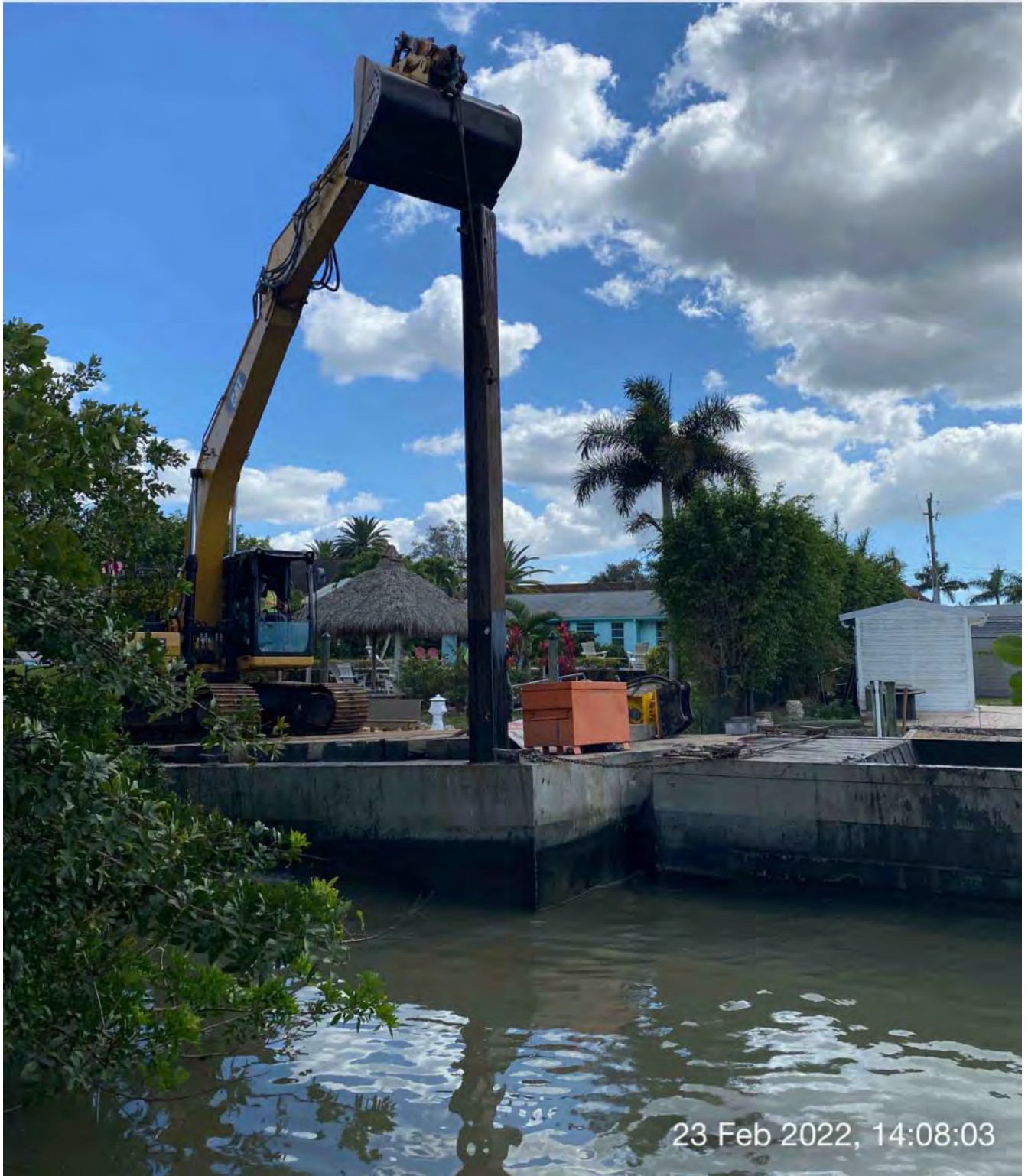
323 excavator lifting spud to allow push boat to mobilize barge at station 13+50
