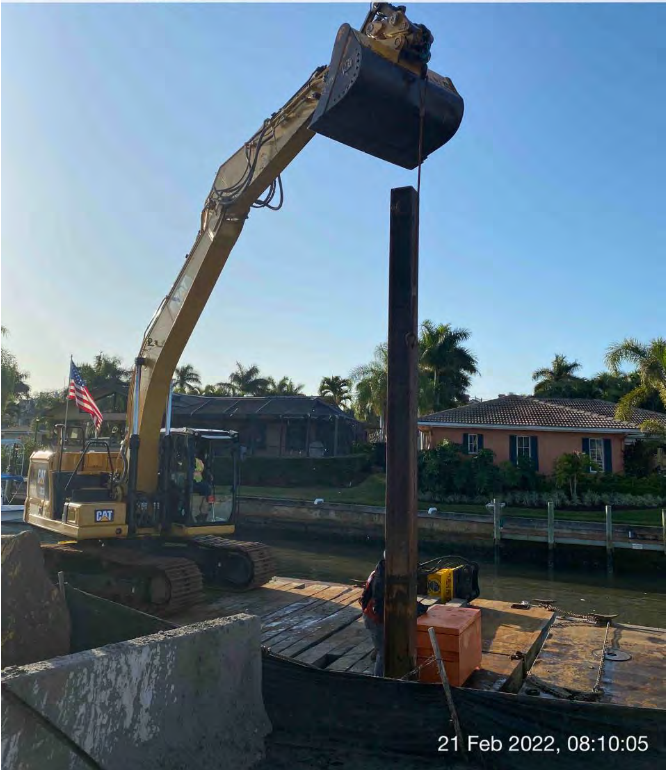
323 excavator lifting spud to allow push boat to mobilize barge at station 1+50
