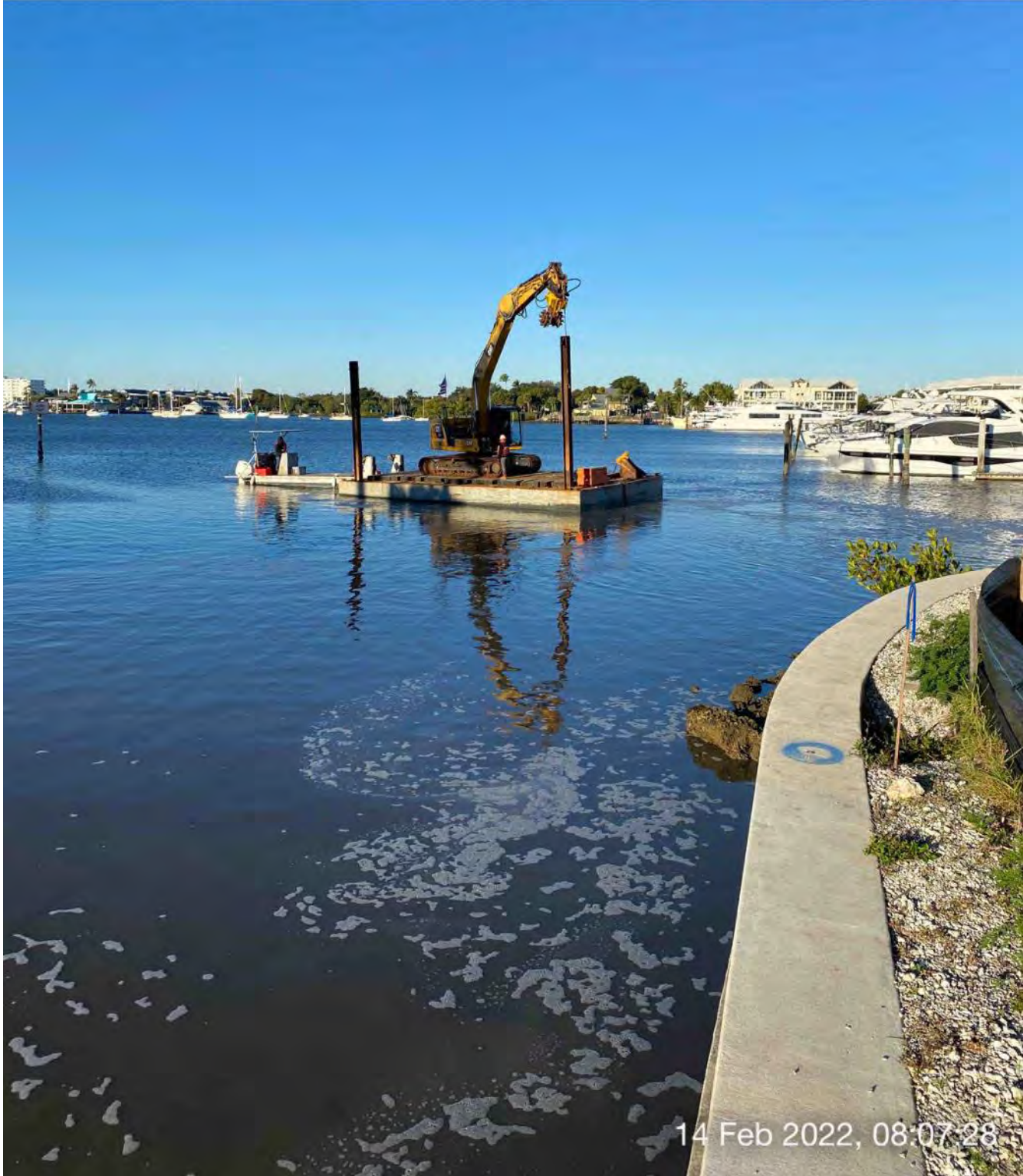
Push boat transporting barge and 323 excavator from Canal CC-CC to Canal BB-BB
