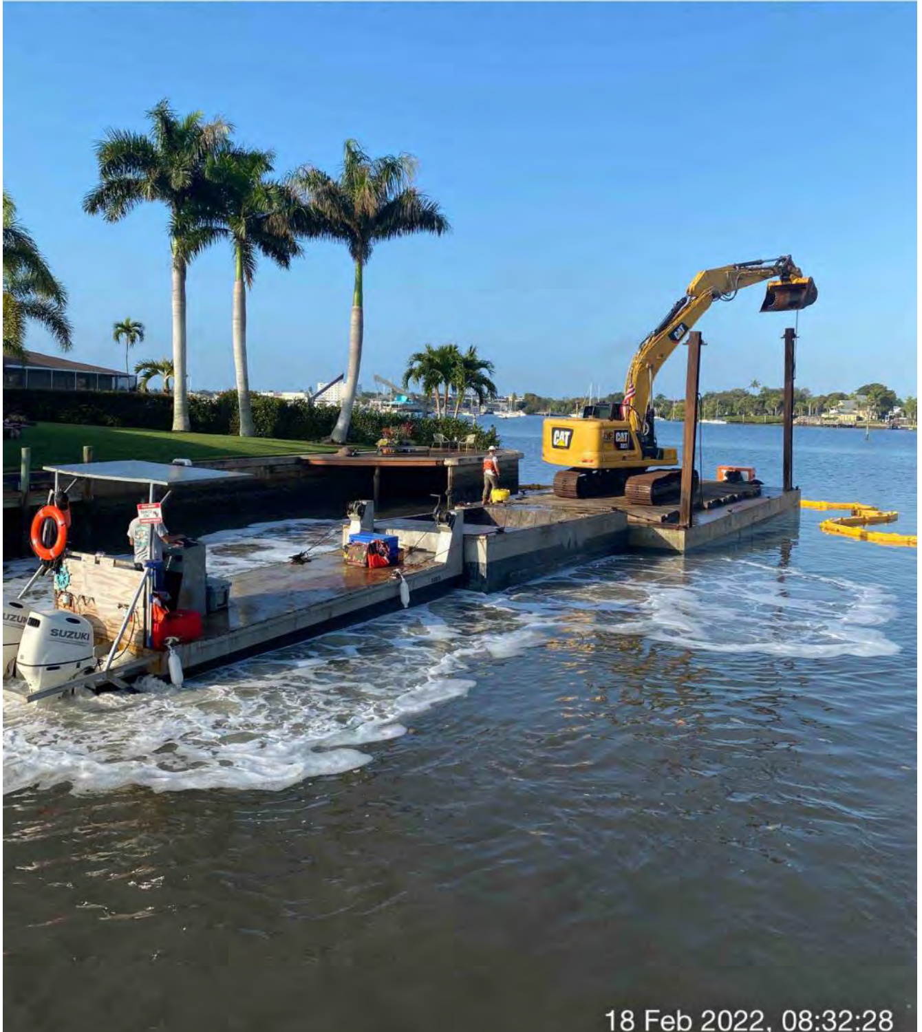
323 excavator lifting spud to allow push boat to mobilize barge at station 1+00
