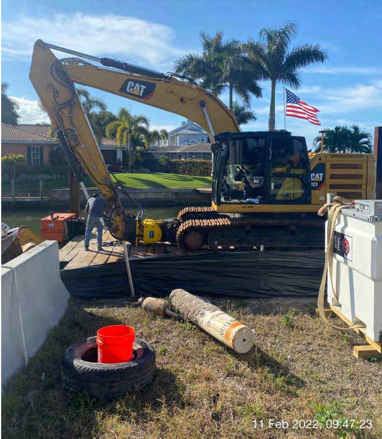
Mechanic inspecting the grease lines on 323 excavator
