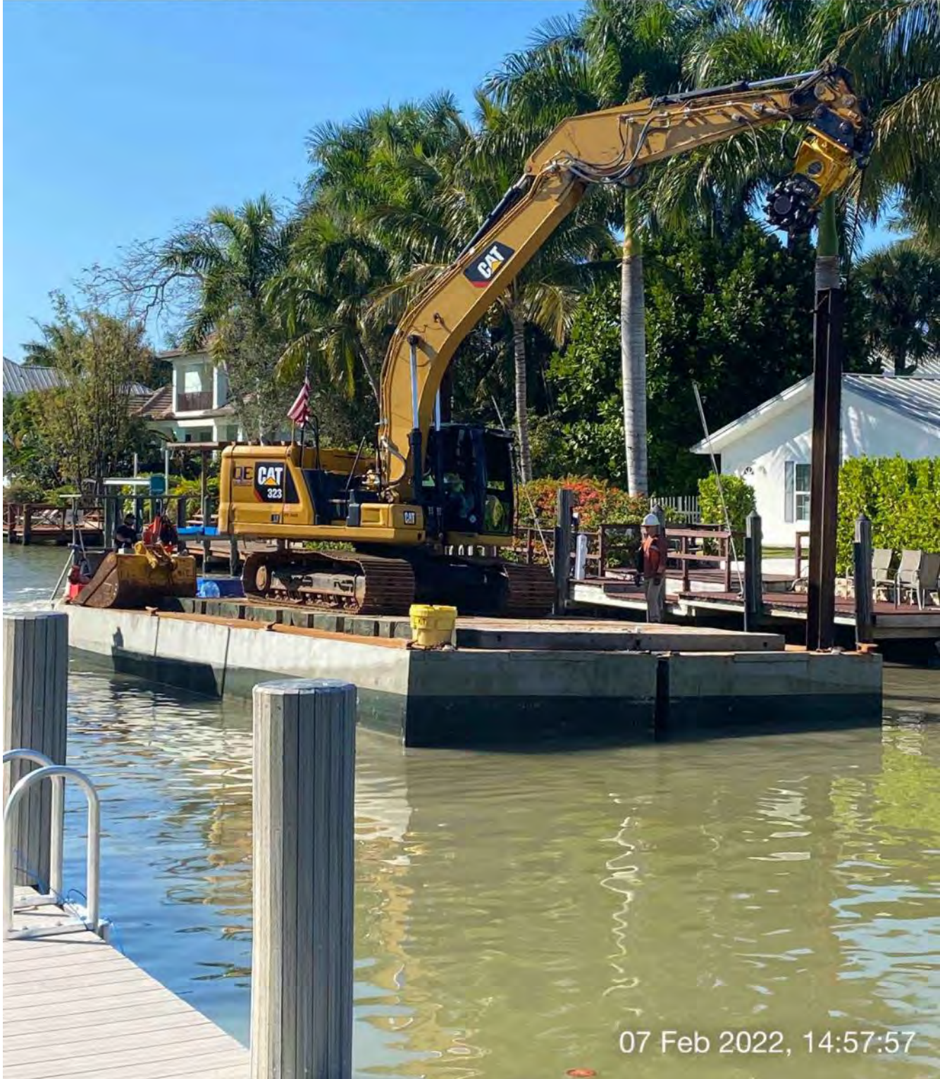
323 excavator lifting spud to allow push boat to mobilize barge at station 8+50
