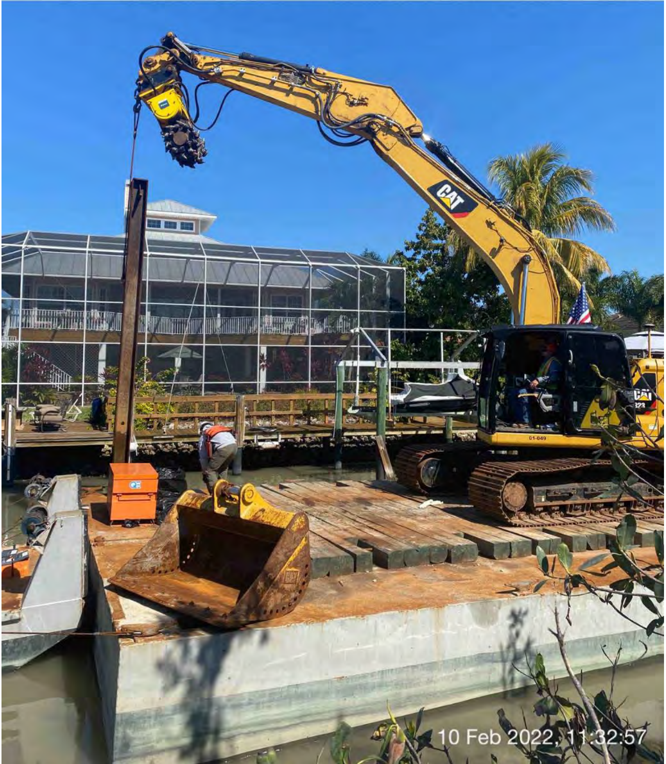
323 excavator lifting spud to allow push boat to mobilize barge at station 9+50
