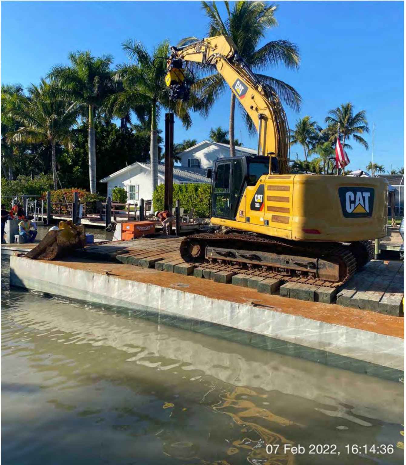
323 excavator lifting spud to allow push boat to mobilize barge at station 8+75
