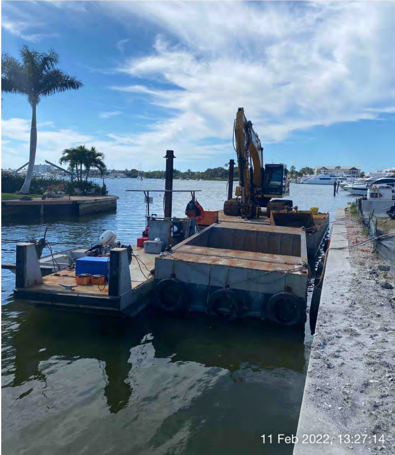
Hopper, push boat, support boat, barge, and 323 excavator staged in Canal CC-CC at station 1+50
