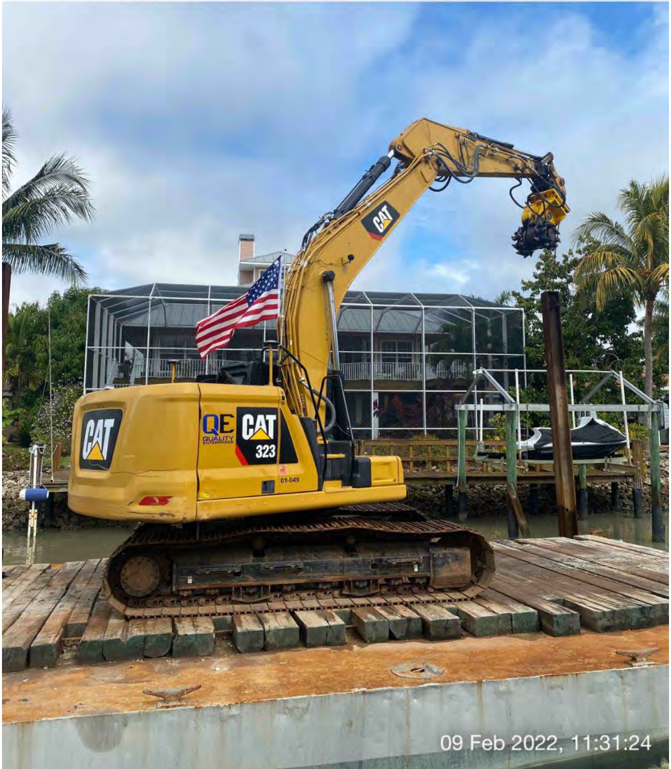
323 excavator lifting spud to allow push boat to mobilize barge at station 9+25
