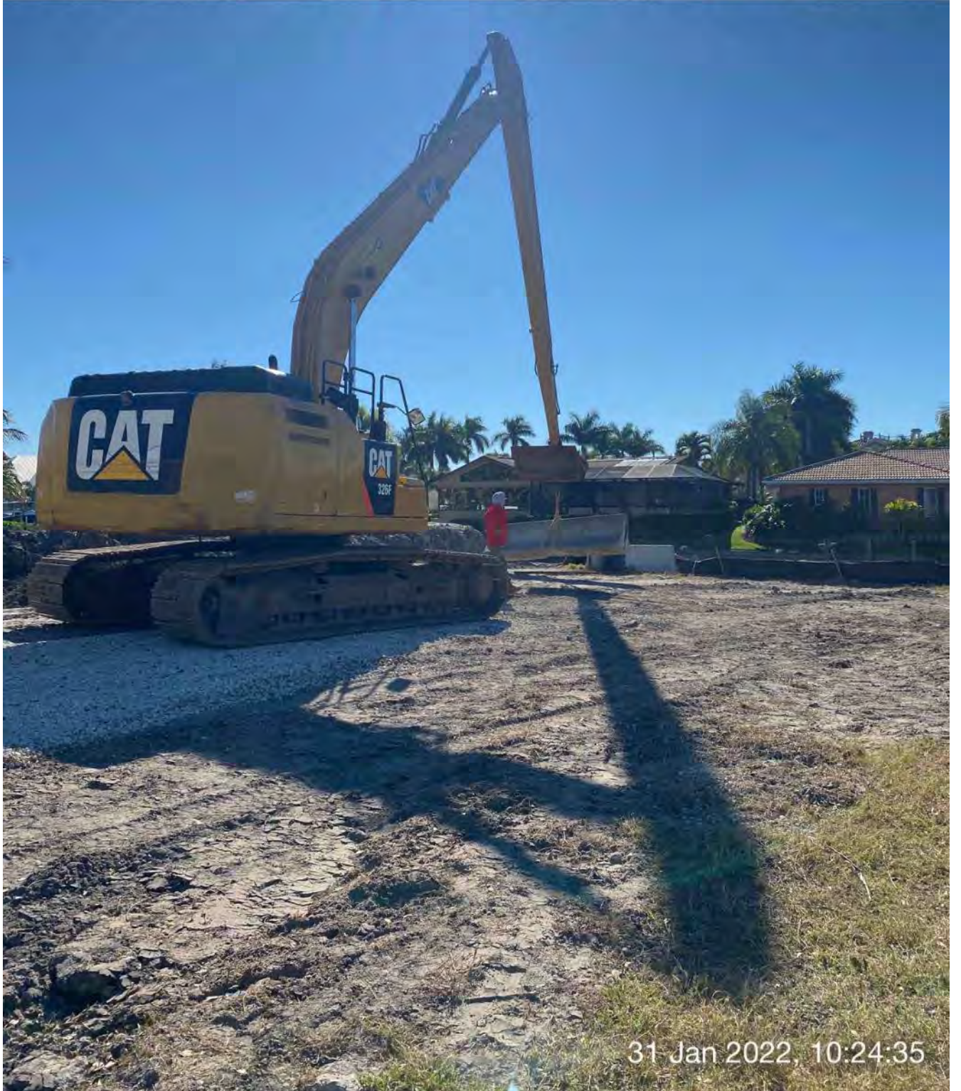
326 excavator transporting barrier elements from east side of 1300 Curlew Avenue to south side
