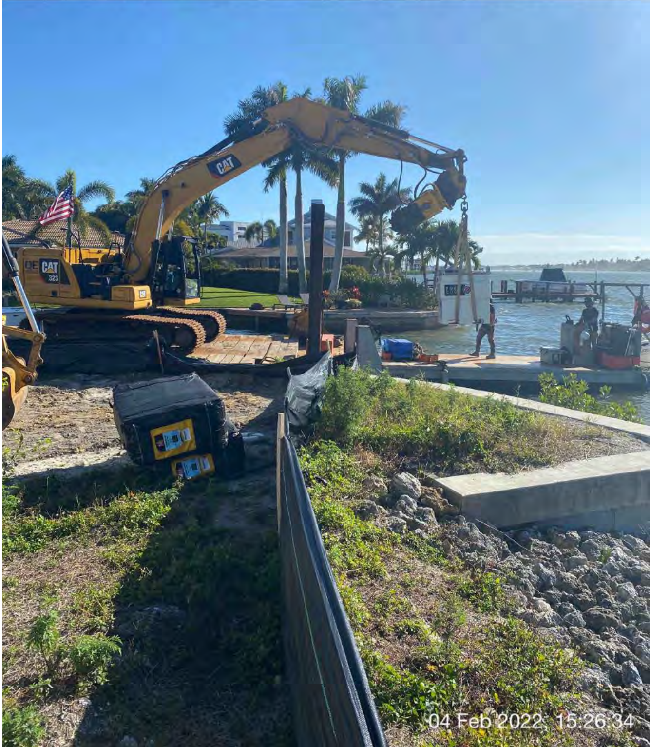
323 excavator transporting small fuel cube from push boat to southwest corner of 1300 Curlew Avenue
