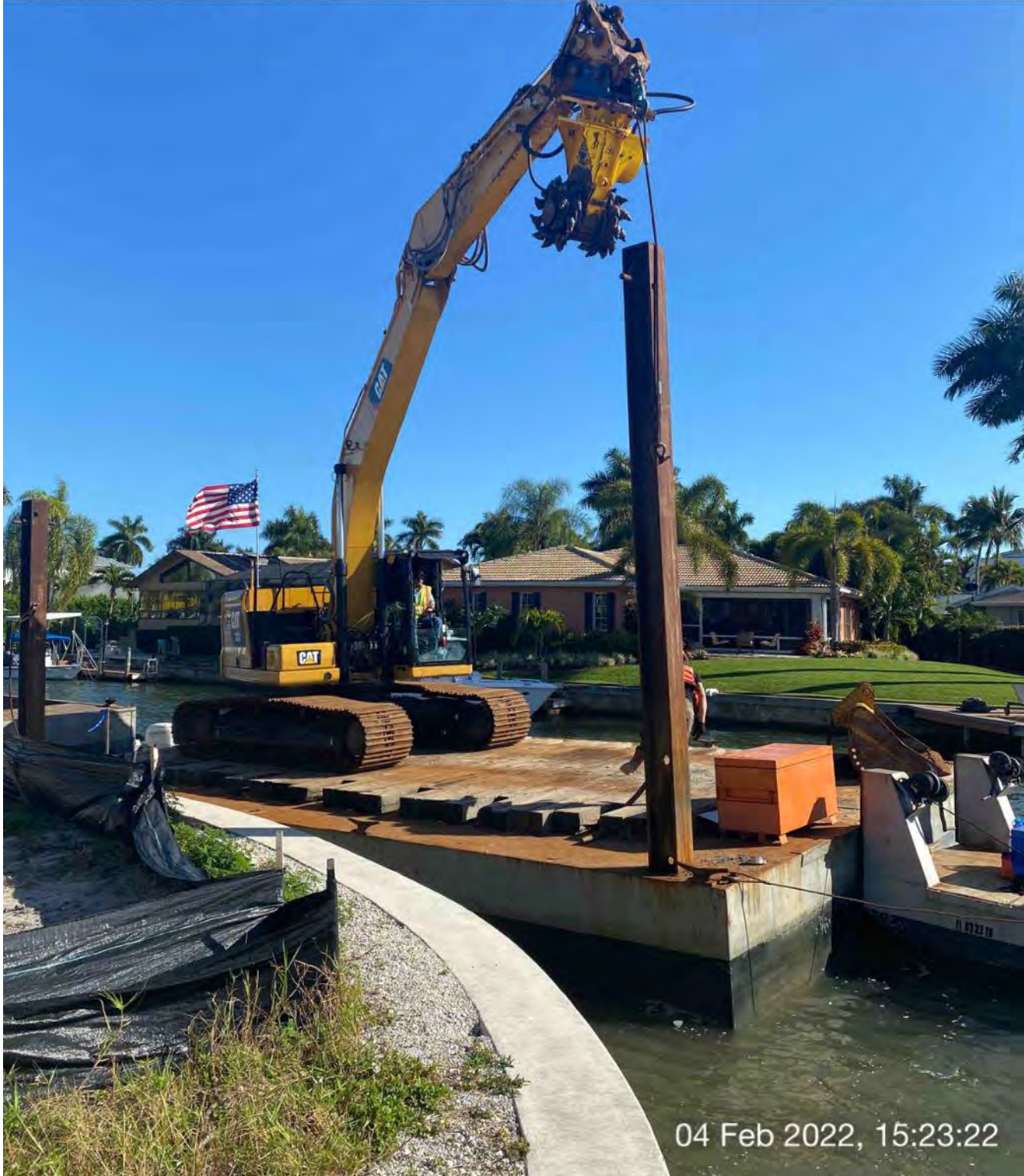
323 excavator lifting spud to allow push boat to mobilize barge at station 1+00 in Canal CC-CC
