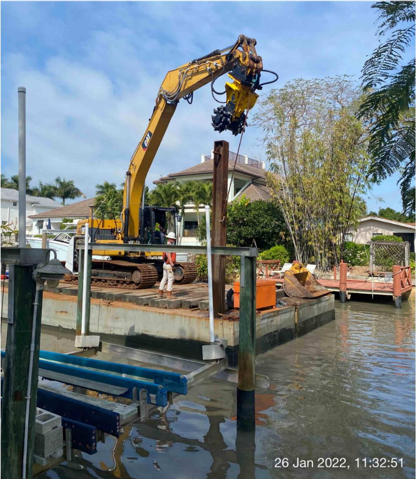
323 excavator lifting spud to allow push boat to move barge at station 6+00
