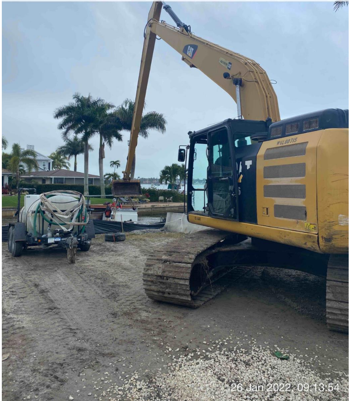
326 excavator transporting small fuel cube from southwest corner of 1300 Curlew Avenue to push boat
