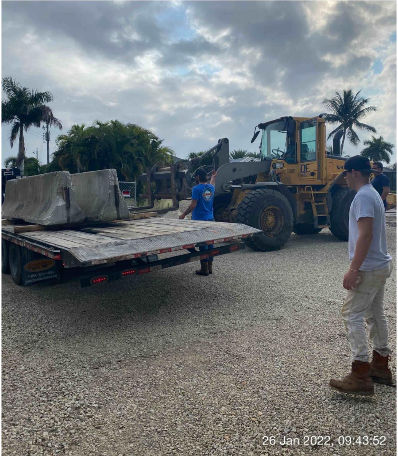
Front end loader transporting barrier walls from truck bed to site at 1300 Curlew Avenue
