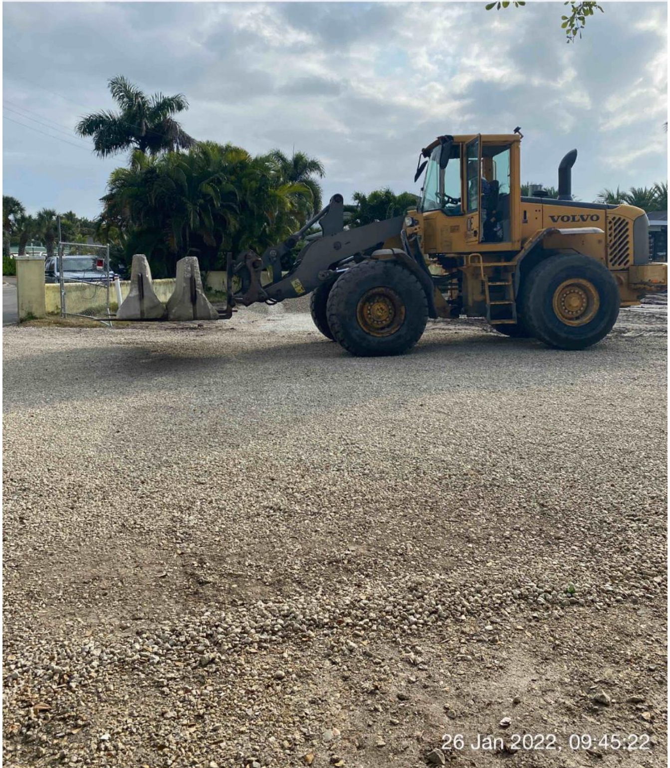
Front end loader transporting barrier walls from truck bed to site at 1300 Curlew Avenue
