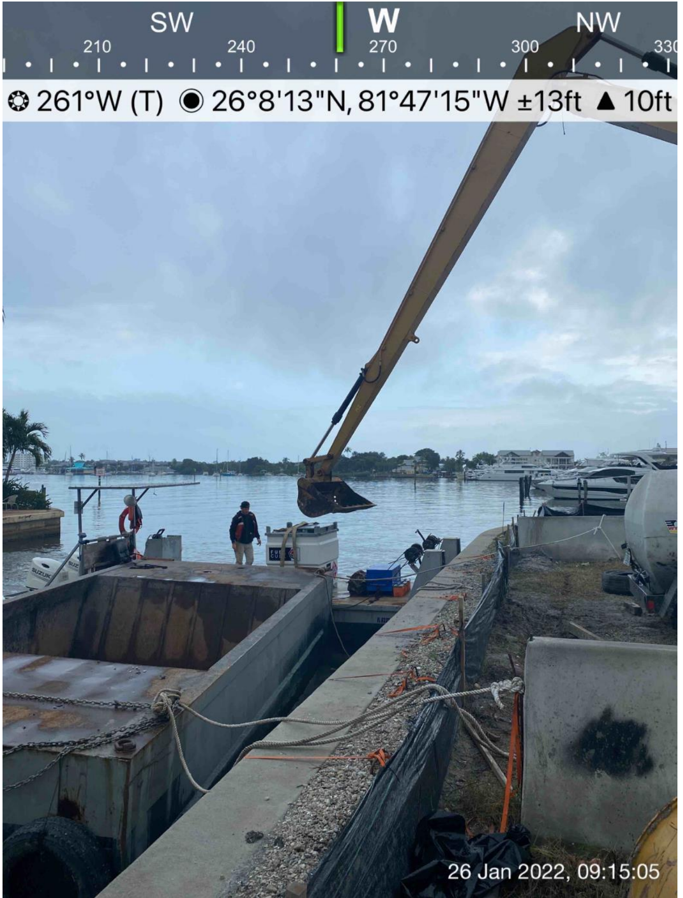
326 excavator transporting small fuel cube from southwest corner of 1300 Curlew Avenue to push boat
