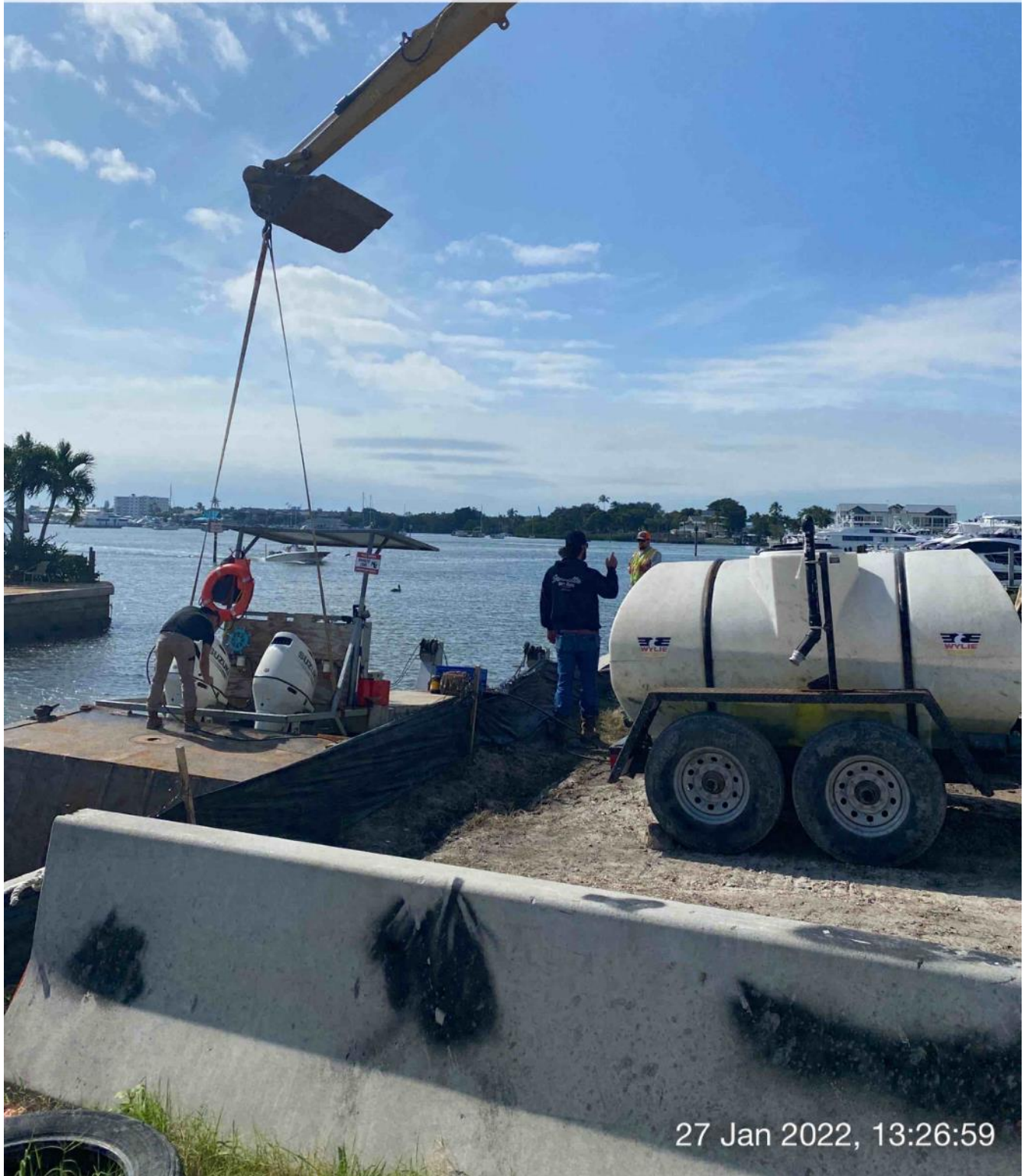
326 excavator lifting push boat to allow for contractor to pressure wash the engines
