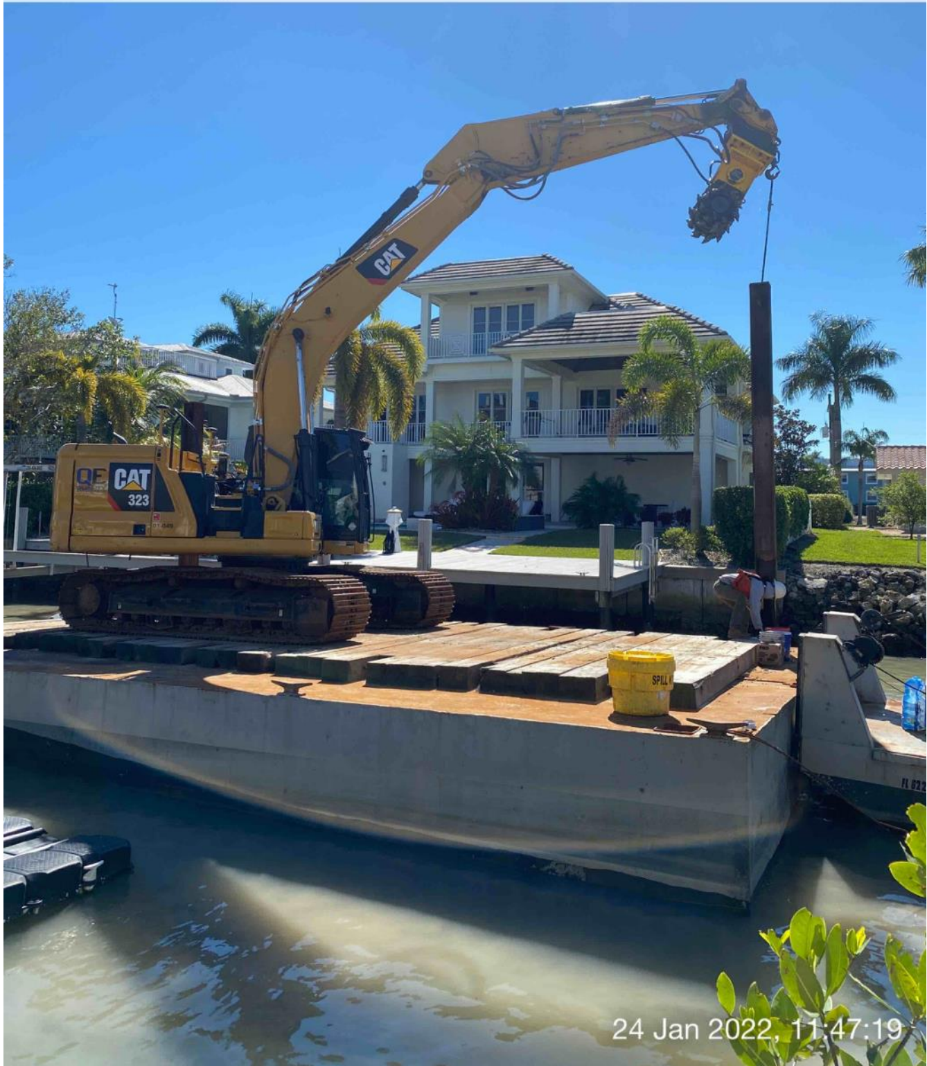
323 excavator lifting spud to allow push boat to move barge at station 4+75
