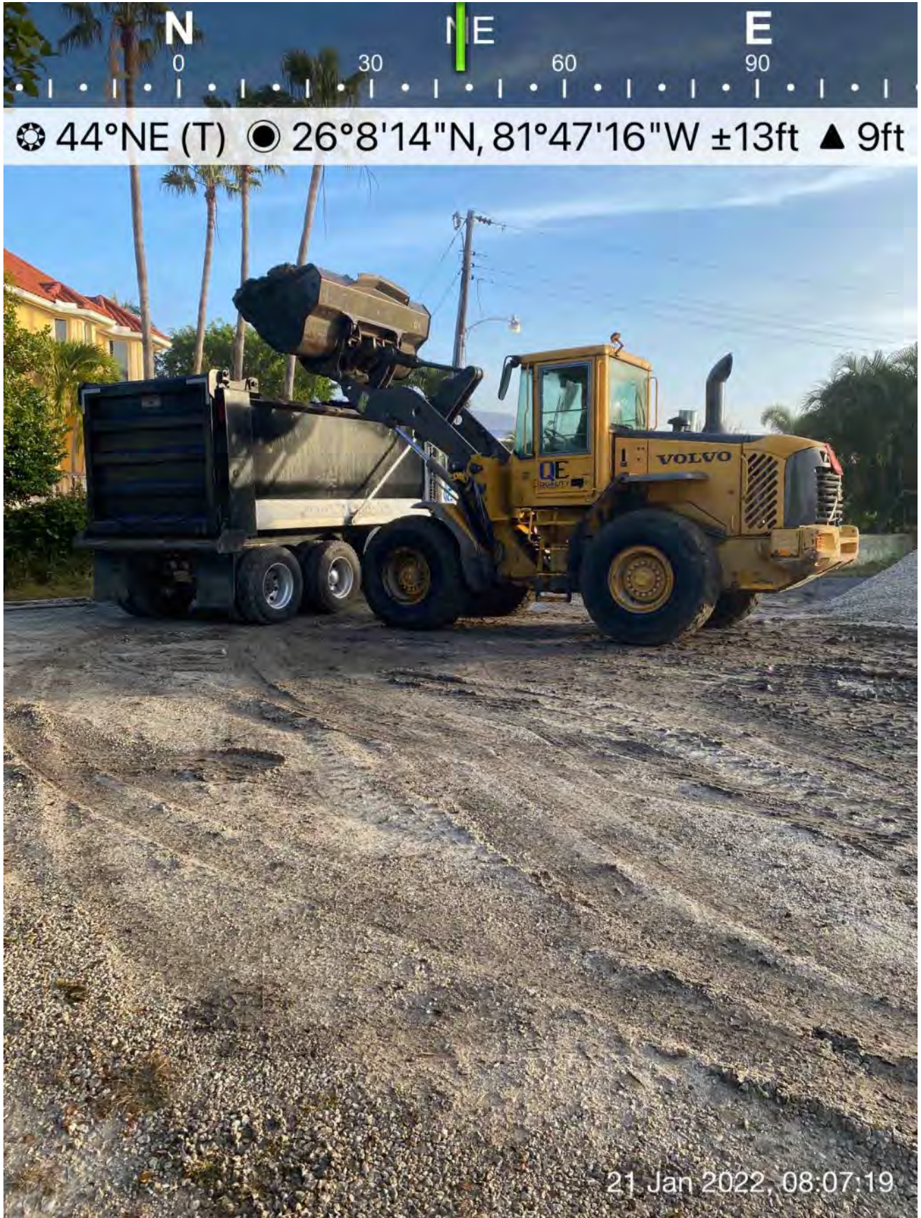
Front end loader transferring material from dewatering site to dump truck at 1300 Curlew Avenue
