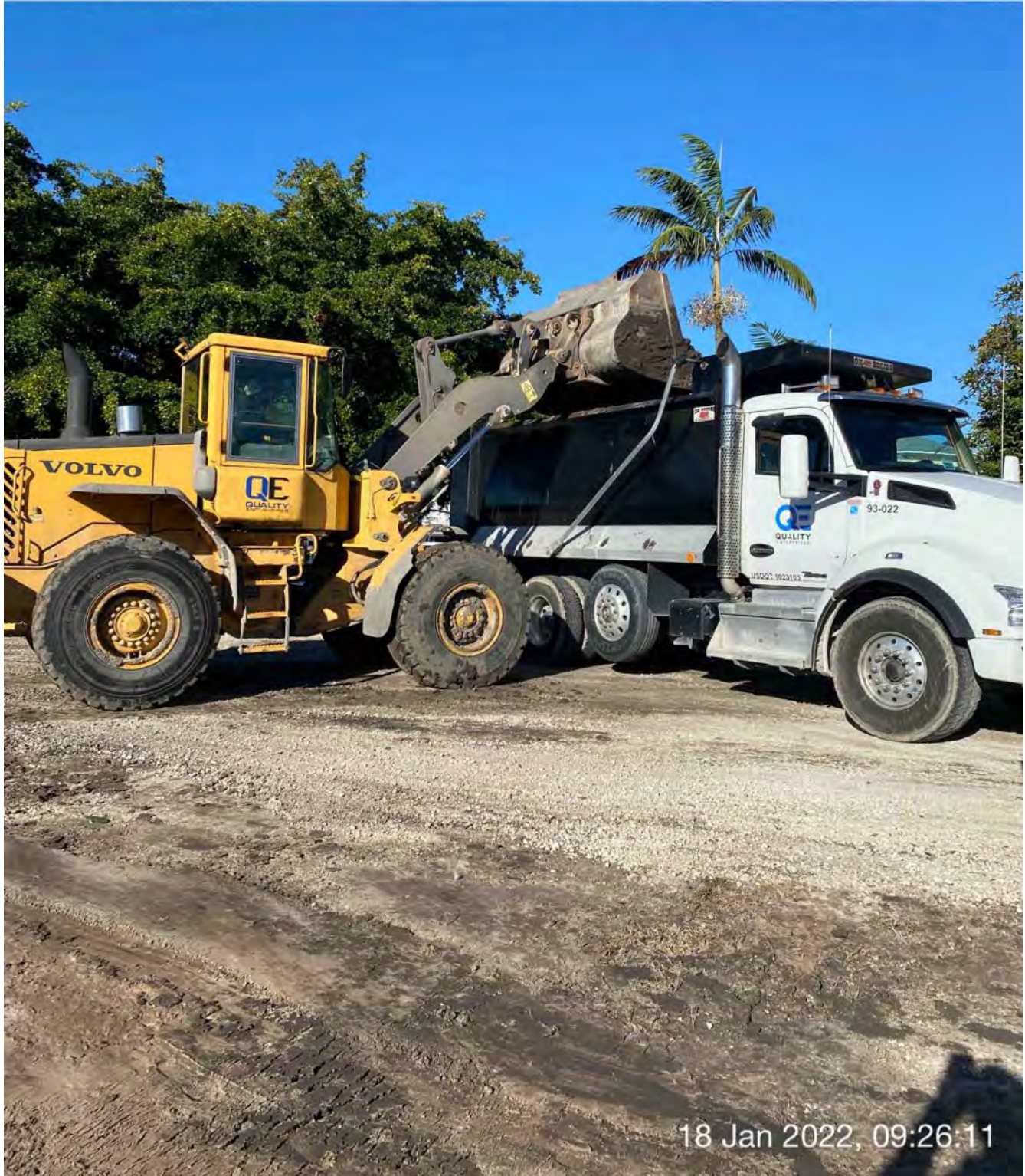
Front end loader transferring material from dewatering site to dump truck at 1300 Curlew Avenue
