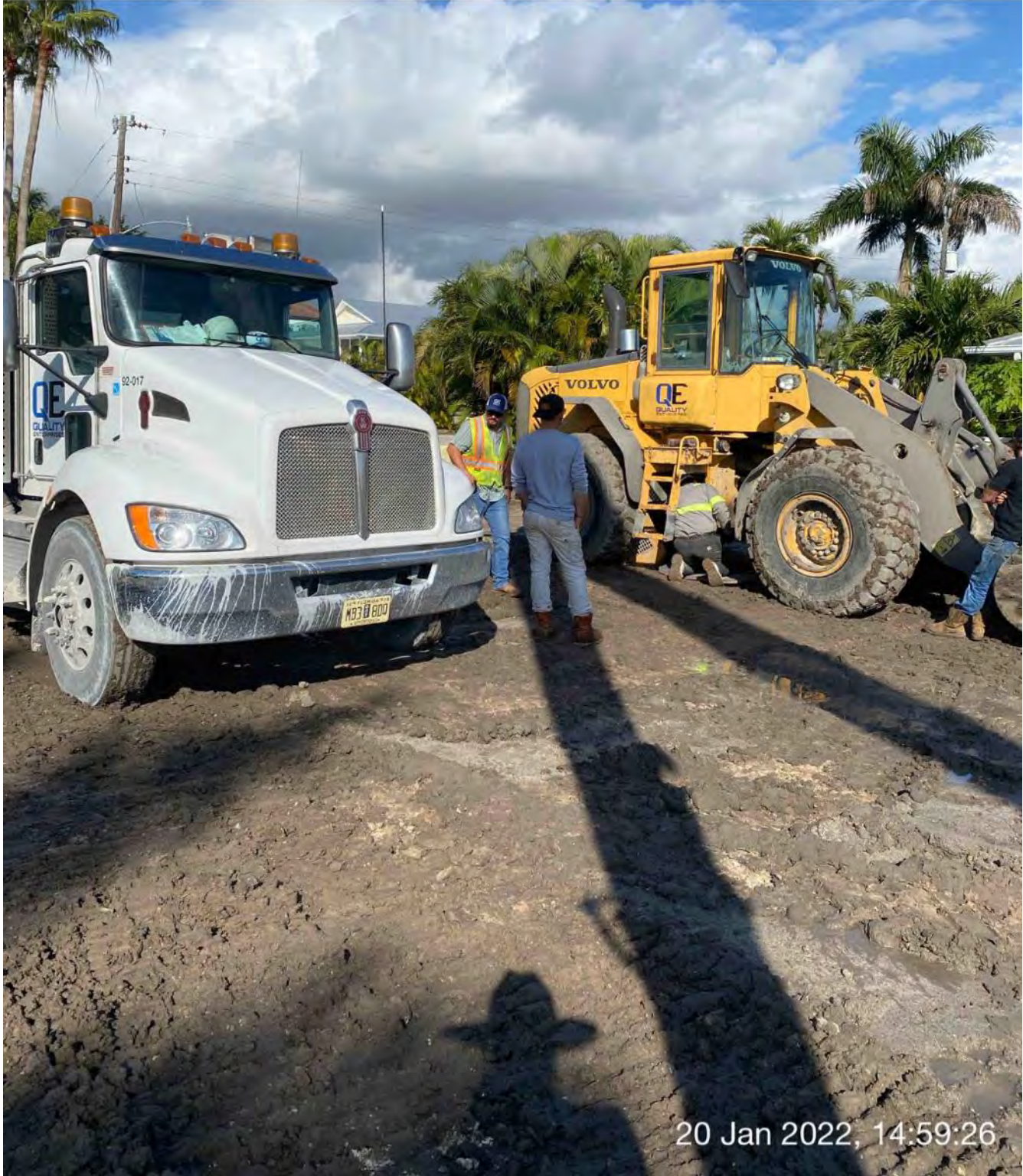
Contractor inspecting and fixing hydraulic hose on front end loader on site at 1300 Curlew Avenue
