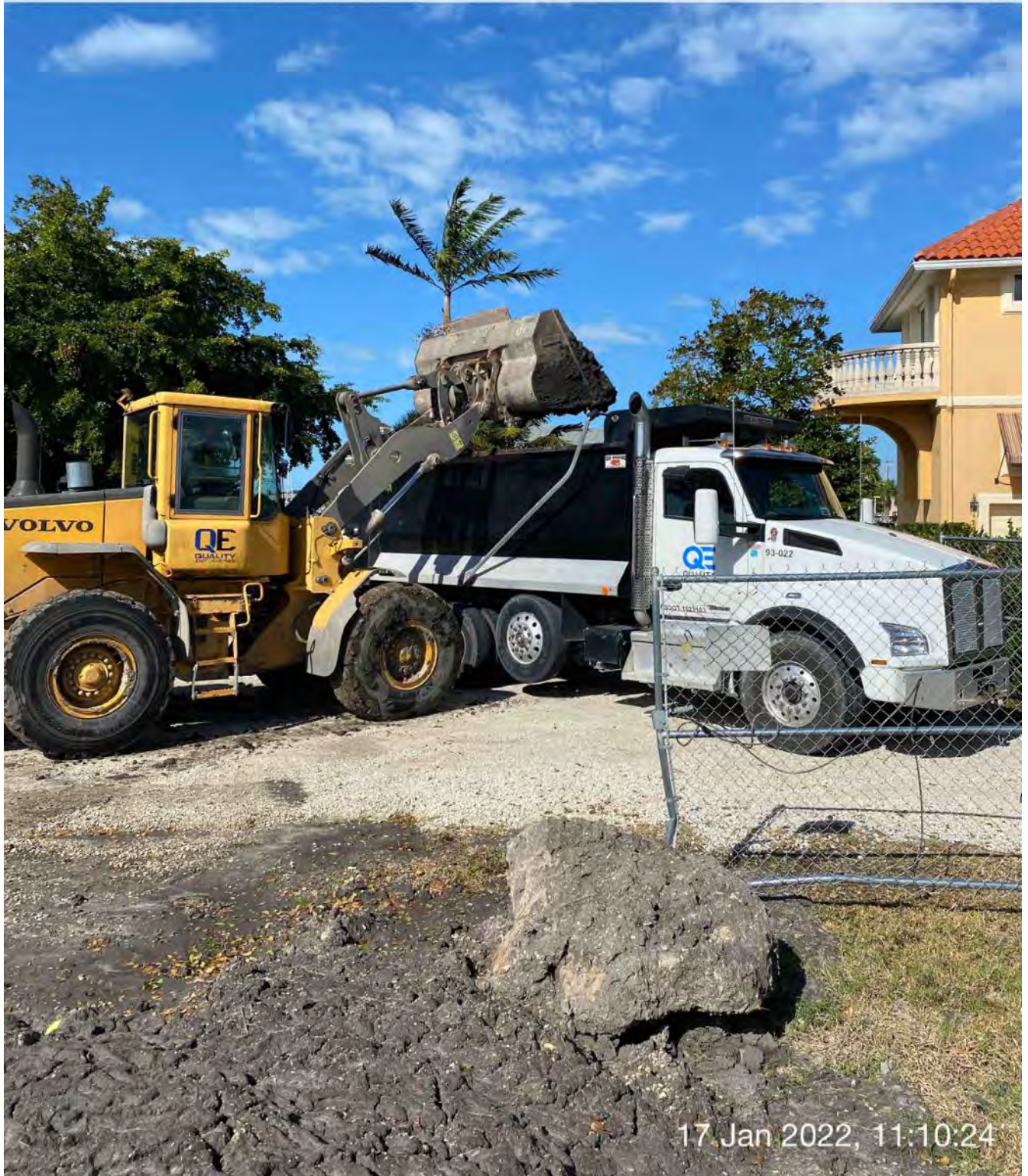
Front end loader transferring material from dewatering site to dump truck at 1300 Curlew Avenue
