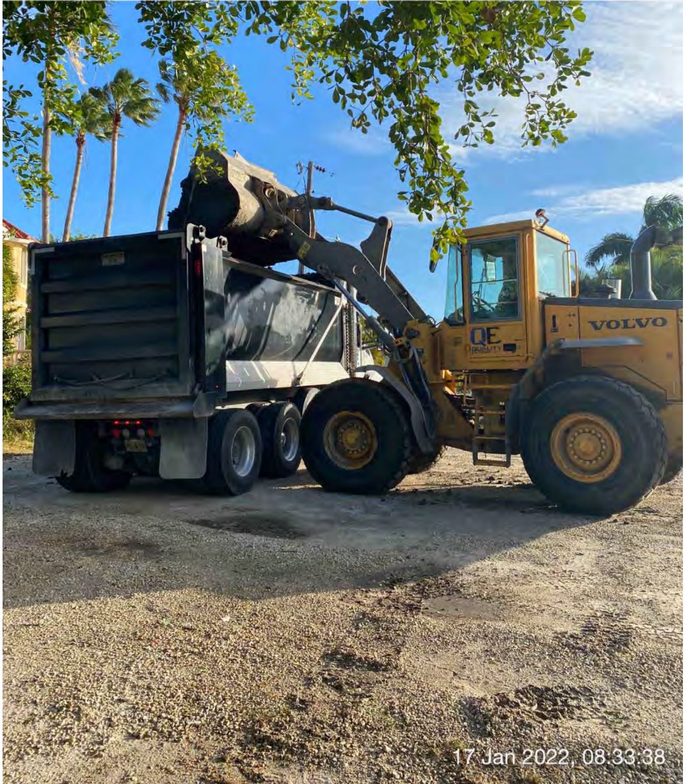
Front end loader transferring material from dewatering site to dump truck at 1300 Curlew Avenue
