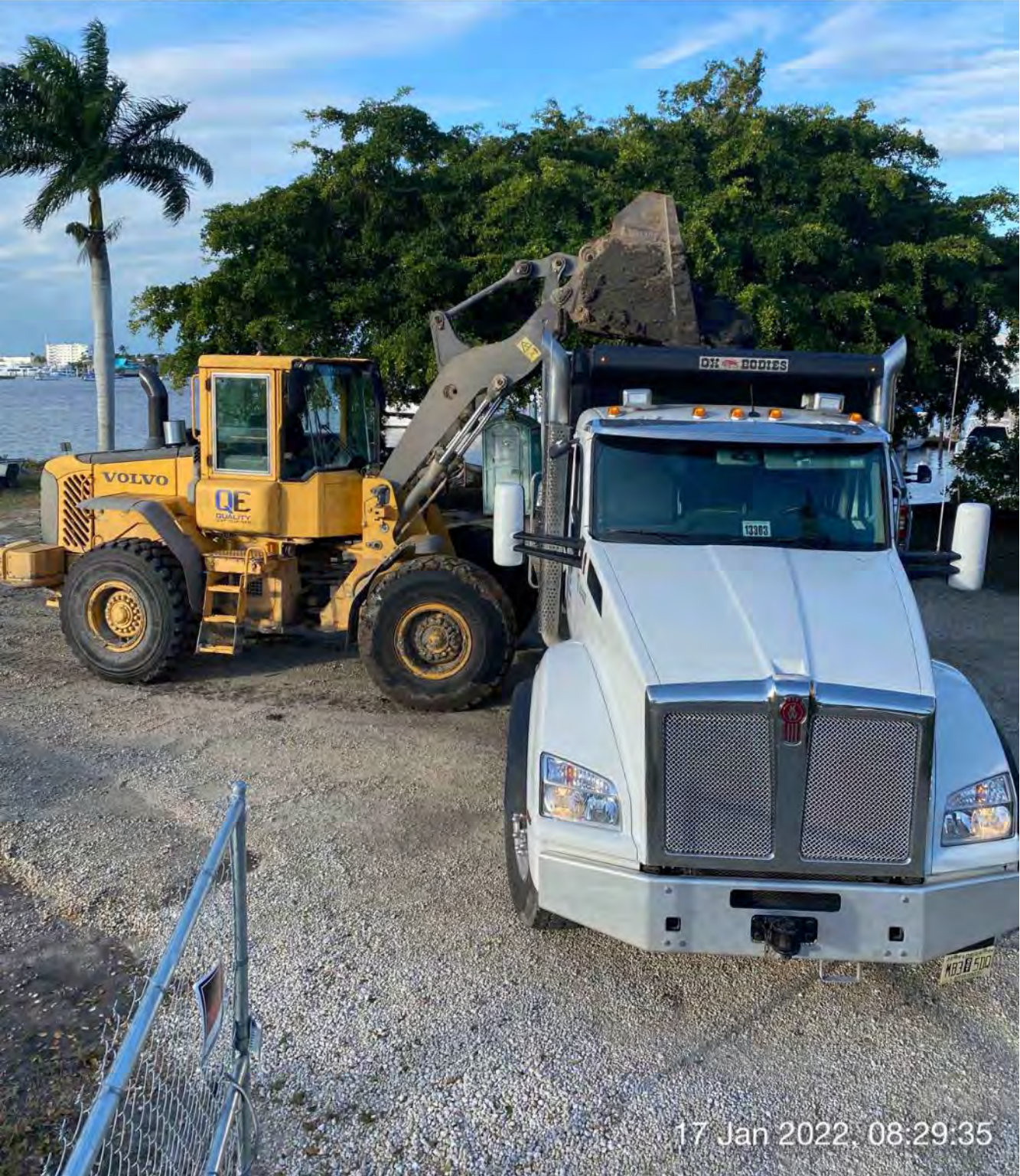
Front end loader transferring material from dewatering site to dump truck at 1300 Curlew Avenue
