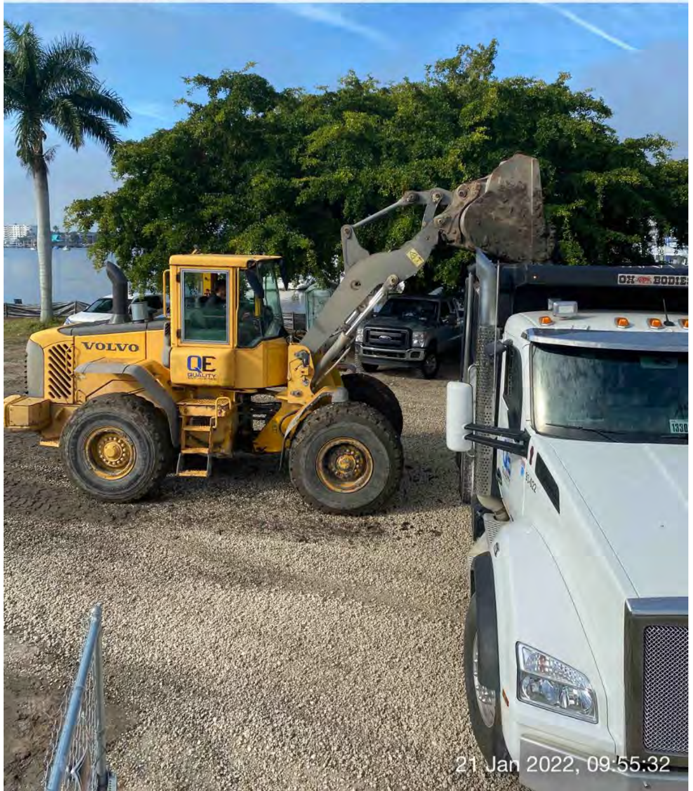
Front end loader transferring material from dewatering site to dump truck at 1300 Curlew Avenue
