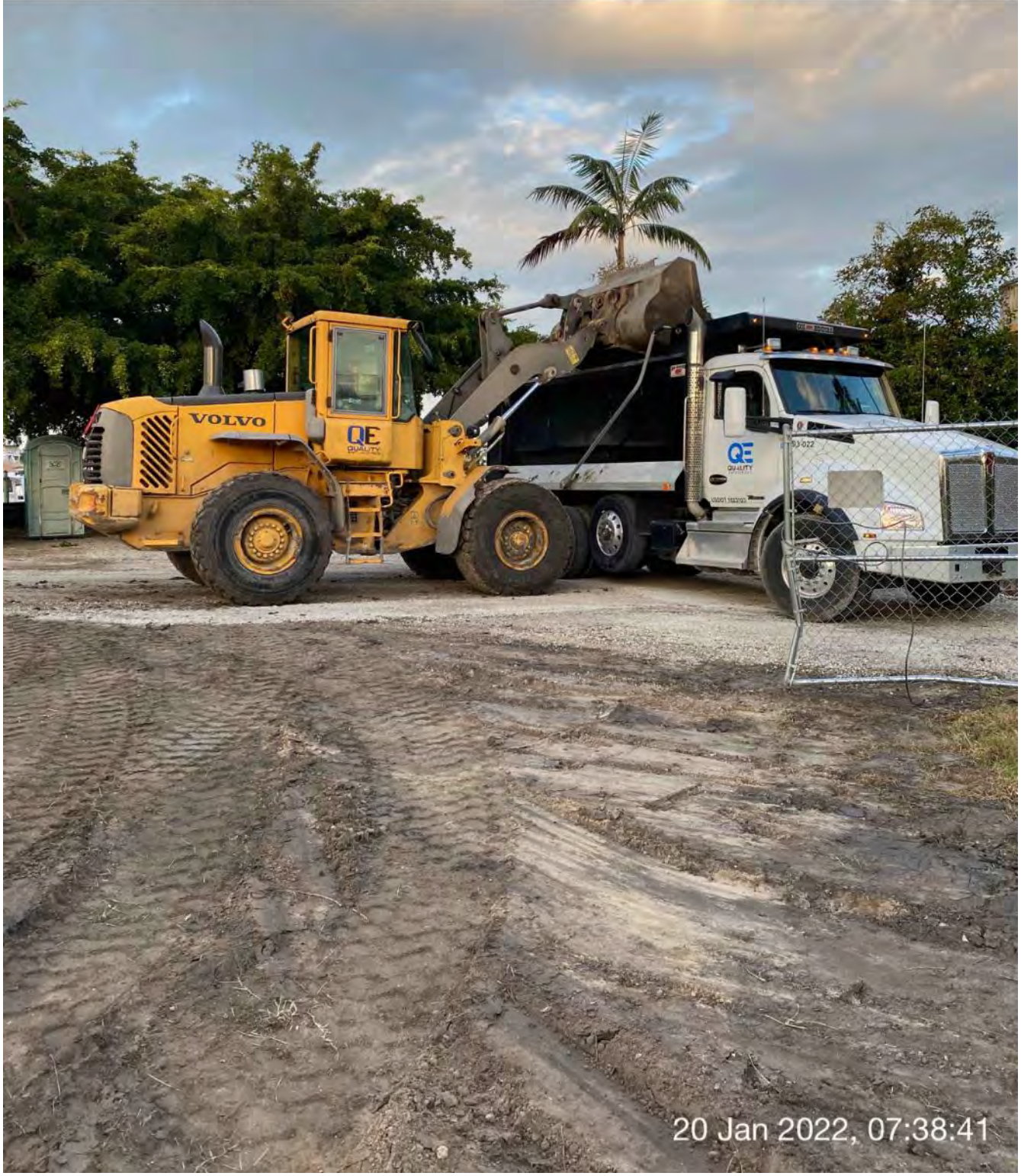
Front end loader transferring material from dewatering site to dump truck at 1300 Curlew Avenue
