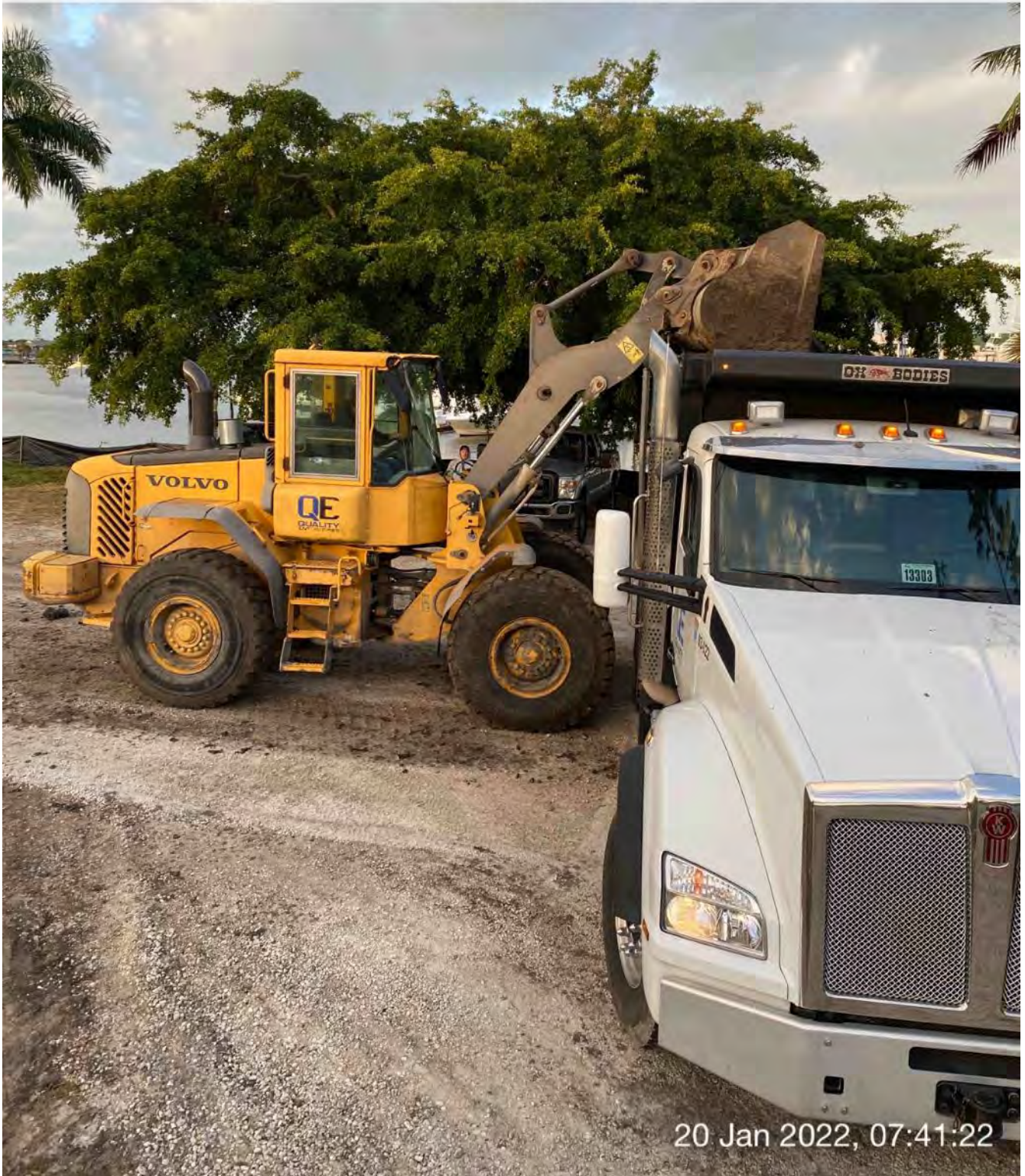
Front end loader transferring material from dewatering site to dump truck at 1300 Curlew Avenue
