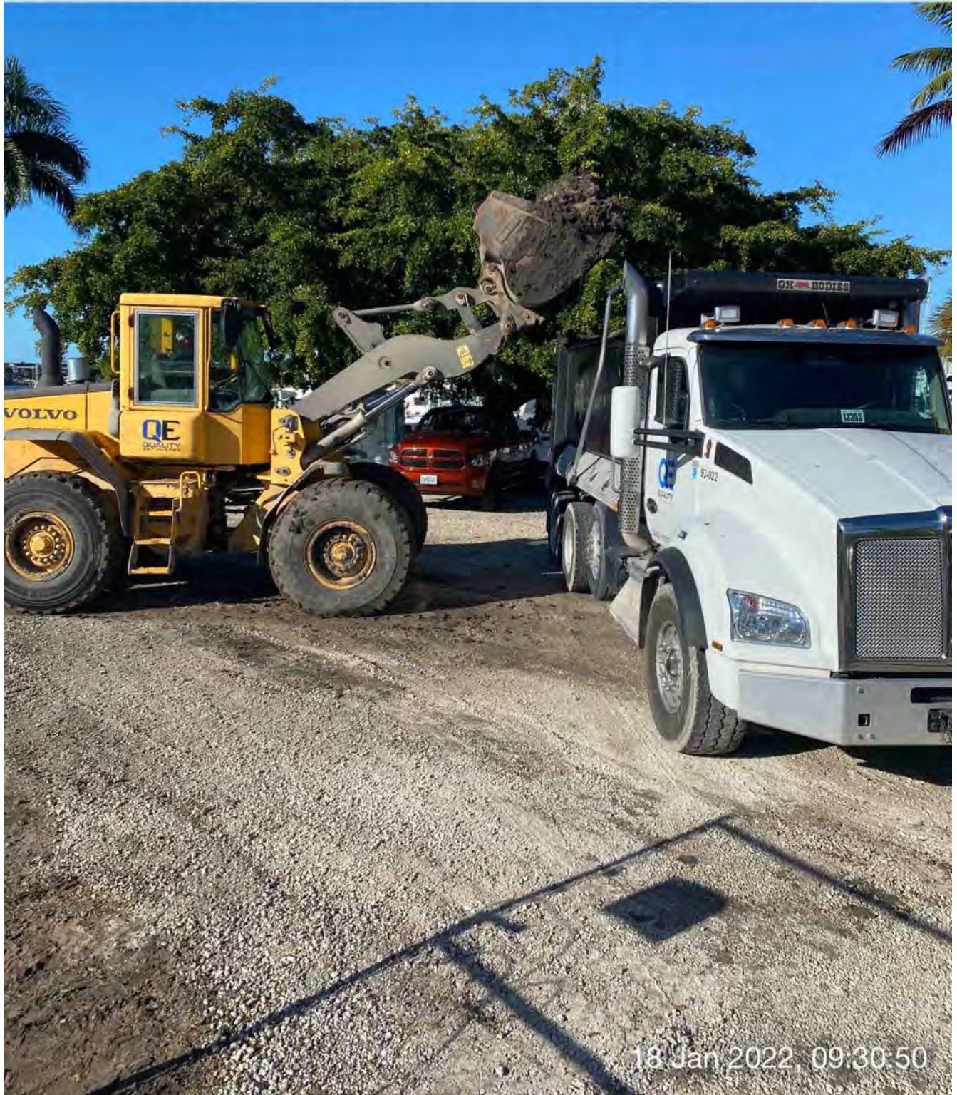
Front end loader transferring material from dewatering site to dump truck at 1300 Curlew Avenue
