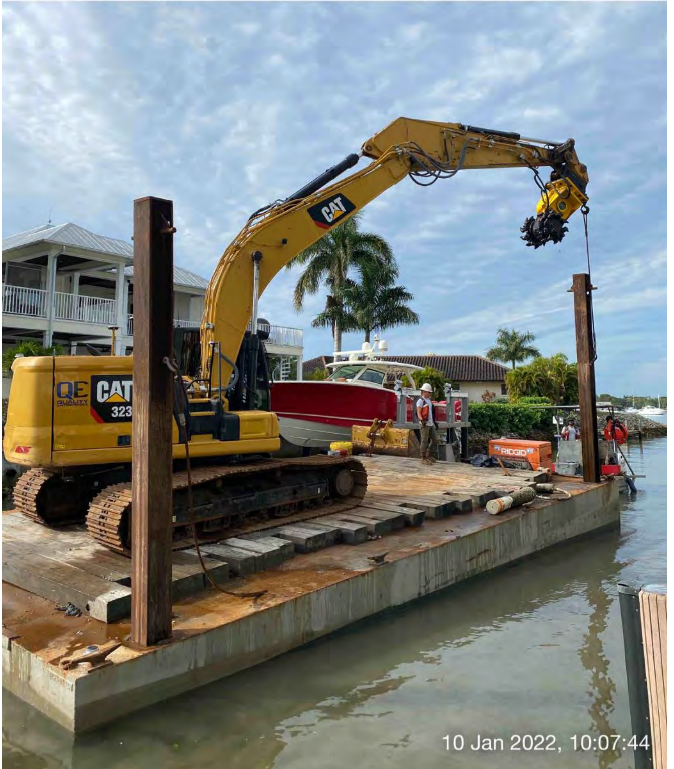
323 excavator lifting spud to allow push boat to move barge at station 3+50
