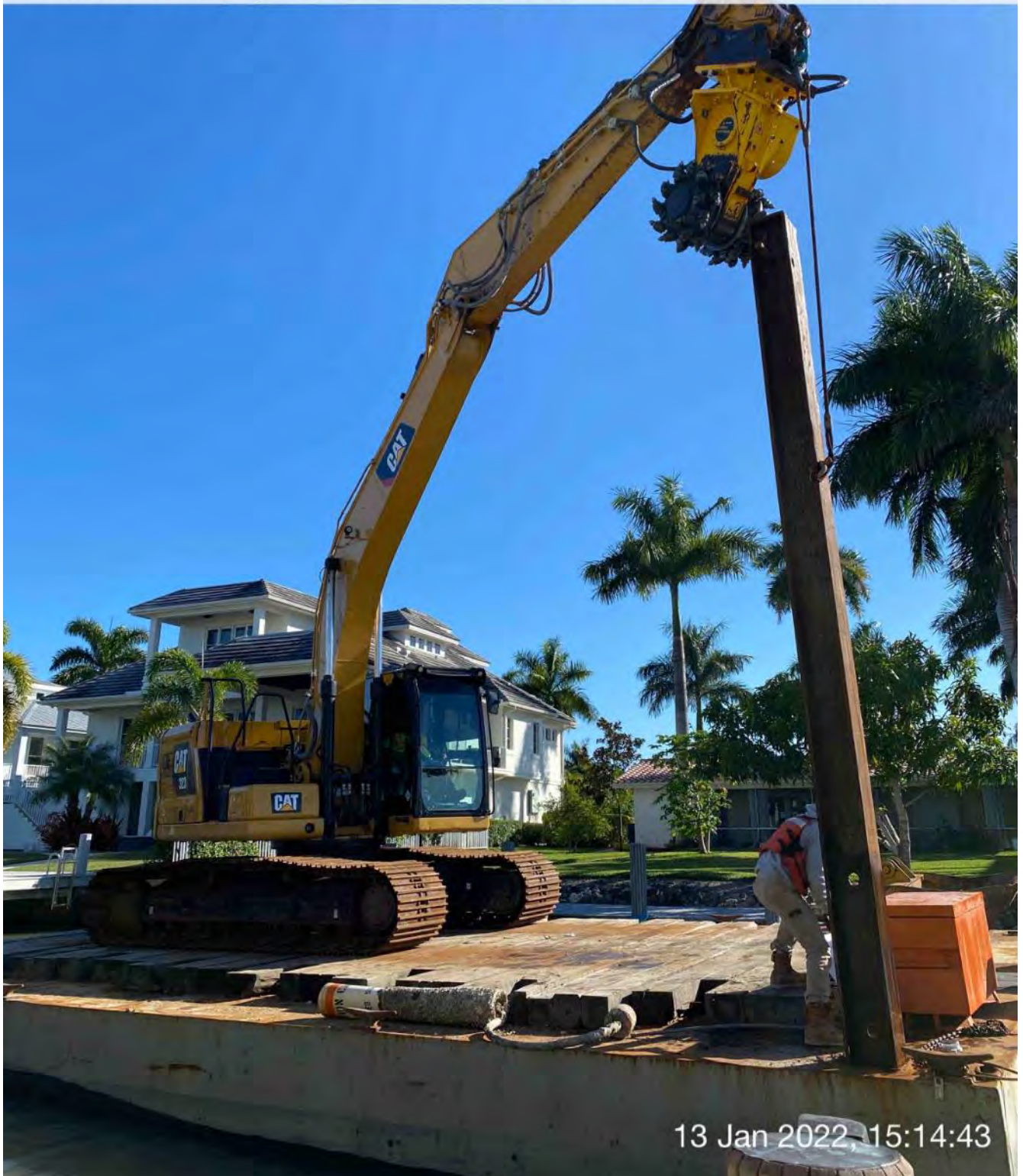
323 excavator lifting spud to allow push boat to move barge at station 4+25
