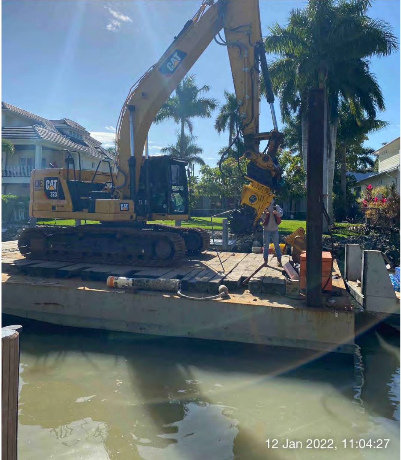
Cleaning the Epiroc grinder and removing an entangled piece of plastic
