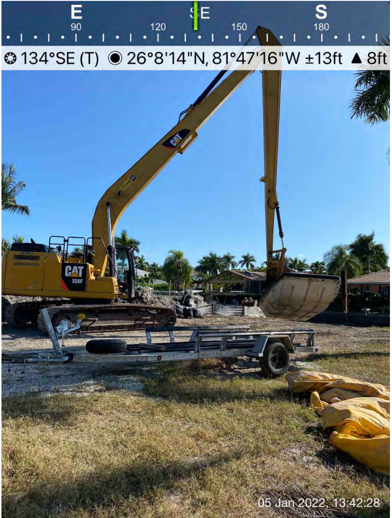
326 excavator lifting support boat and transporting it into the water in Canal CC-CC
