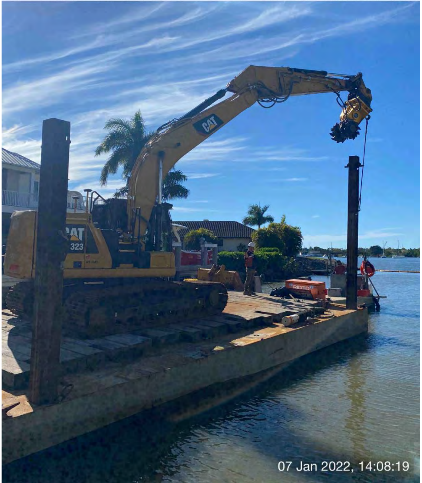
323 excavator lifting spud to allow push boat to move barge at station 3+50 in Canal BB-BB
