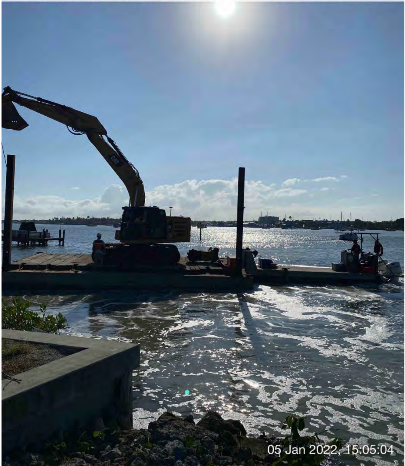
323 excavator lifting spud to allow push boat to move barge from Canal CC-CC to Canal BB-BB
