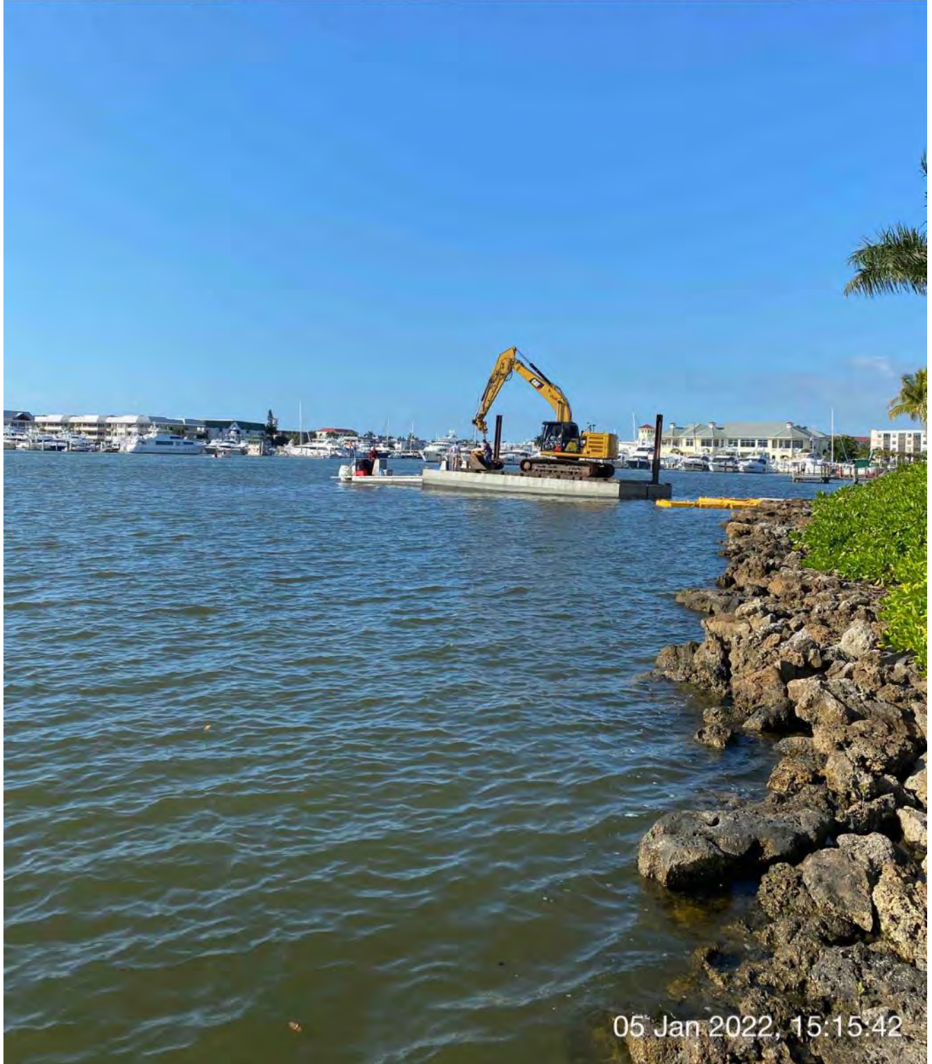
323 excavator, barge, push boat, and turbidity curtain at station 0+00 in Canal BB-BB
