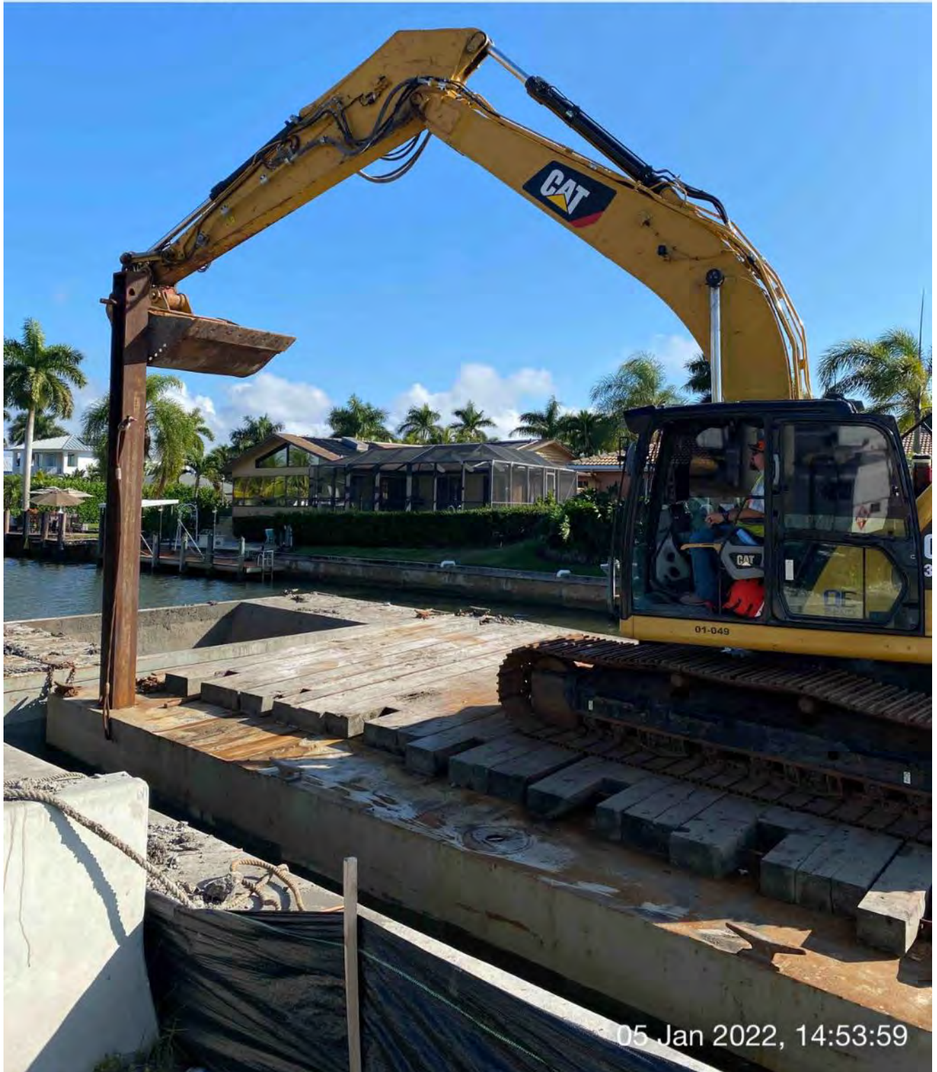
323 excavator lifting spud to allow push boat to move barge at station 1+50 in Canal CC-CC
