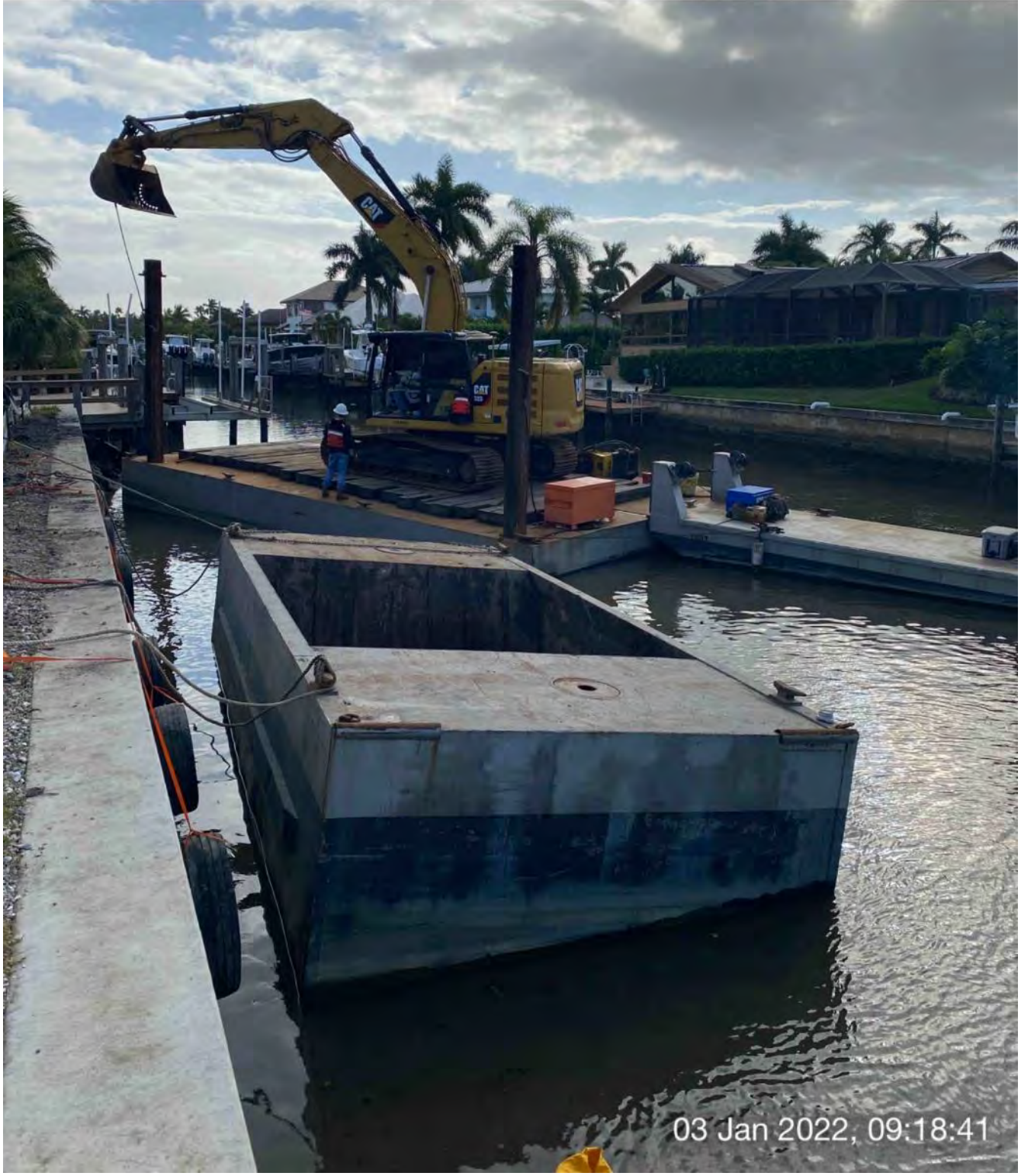
323 excavator lifting spud to allow push boat to move barge at station 2+00
