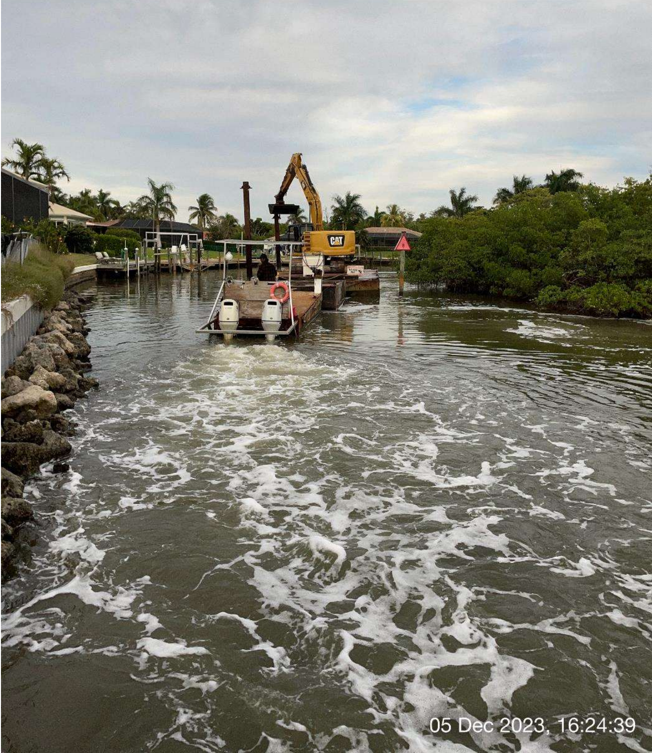
Push boat moving equipment to station 4+00 in Canal Main B1 to be staged for the night.
