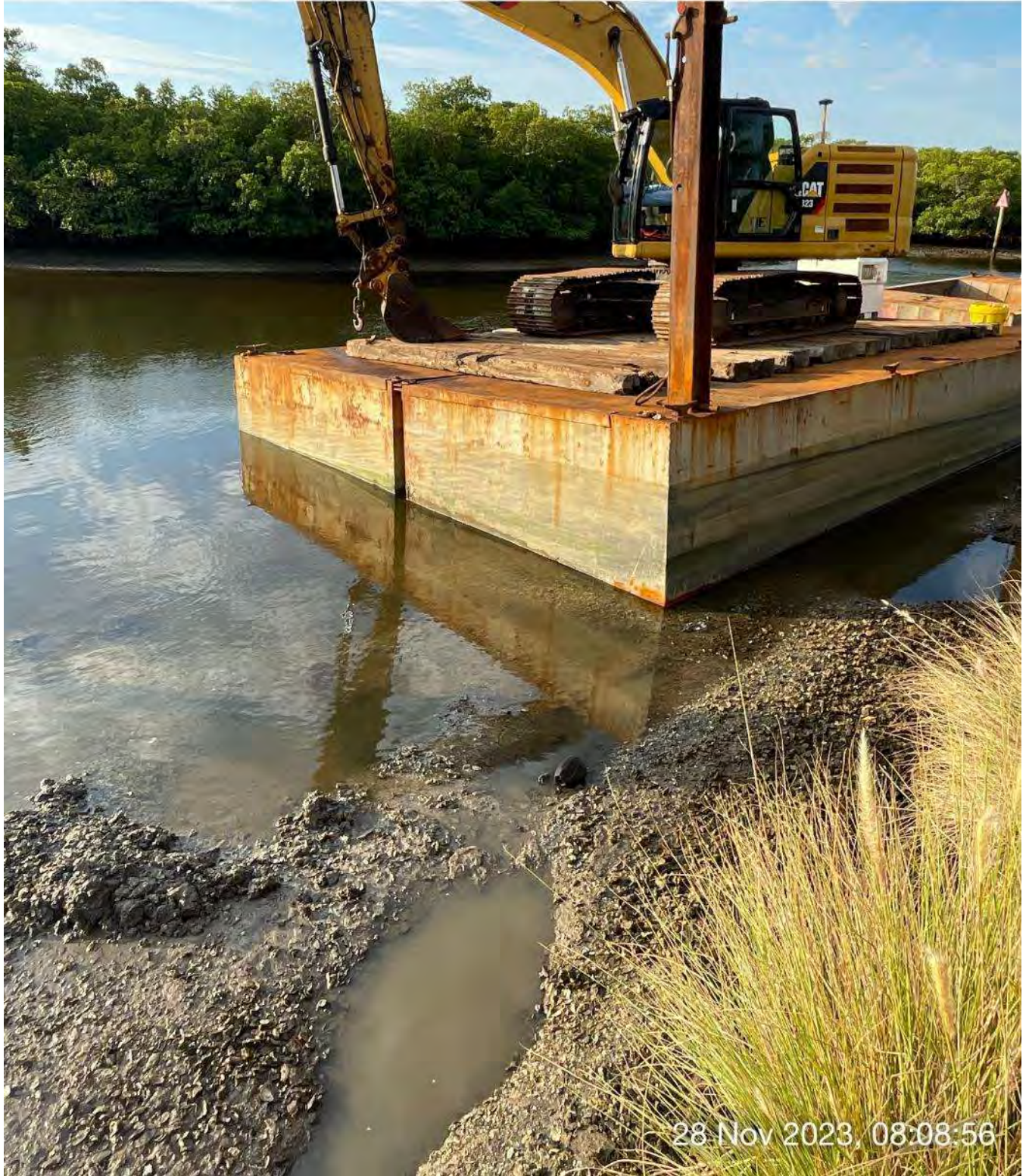
Barge sitting on canal bottom at station 4+00 in Canal Main B1.
