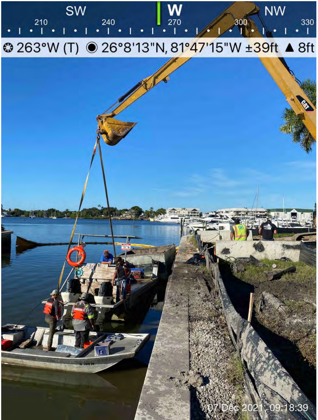
326 excavator lifting push boat to allow technician to change the oil on the motors from the support boat
