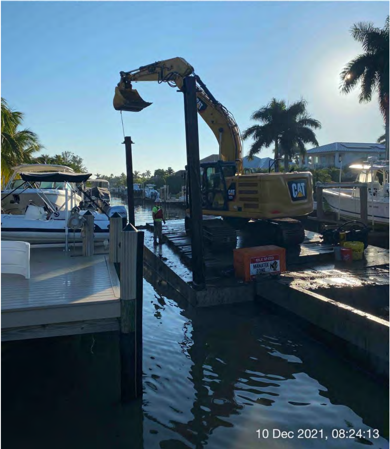
323 excavator lifting spud to allow push boat to move barge from station 4+00 to 3+50
