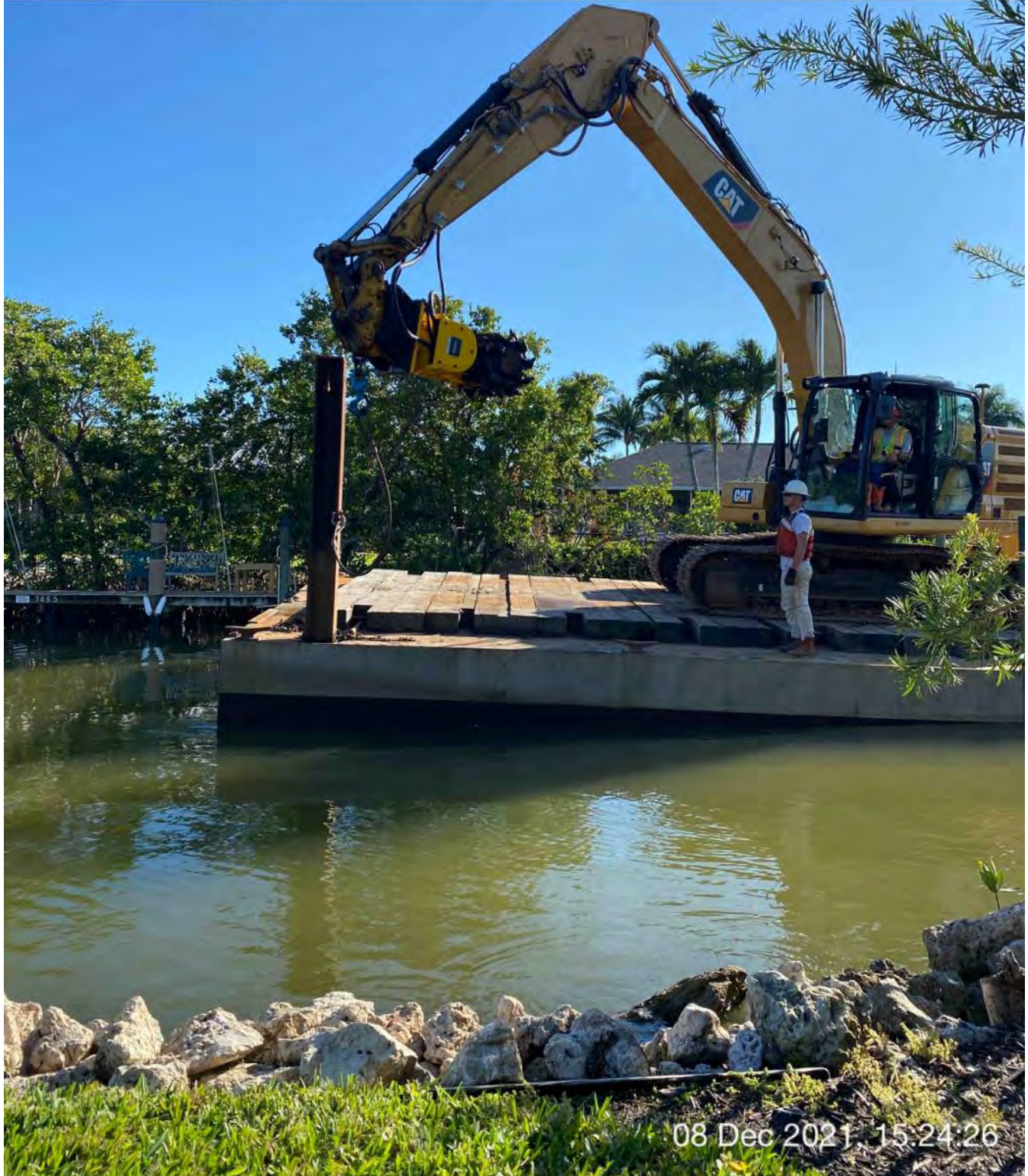
323 excavator lifting spud to allow push boat to move barge from station 8+50 to 9+00
