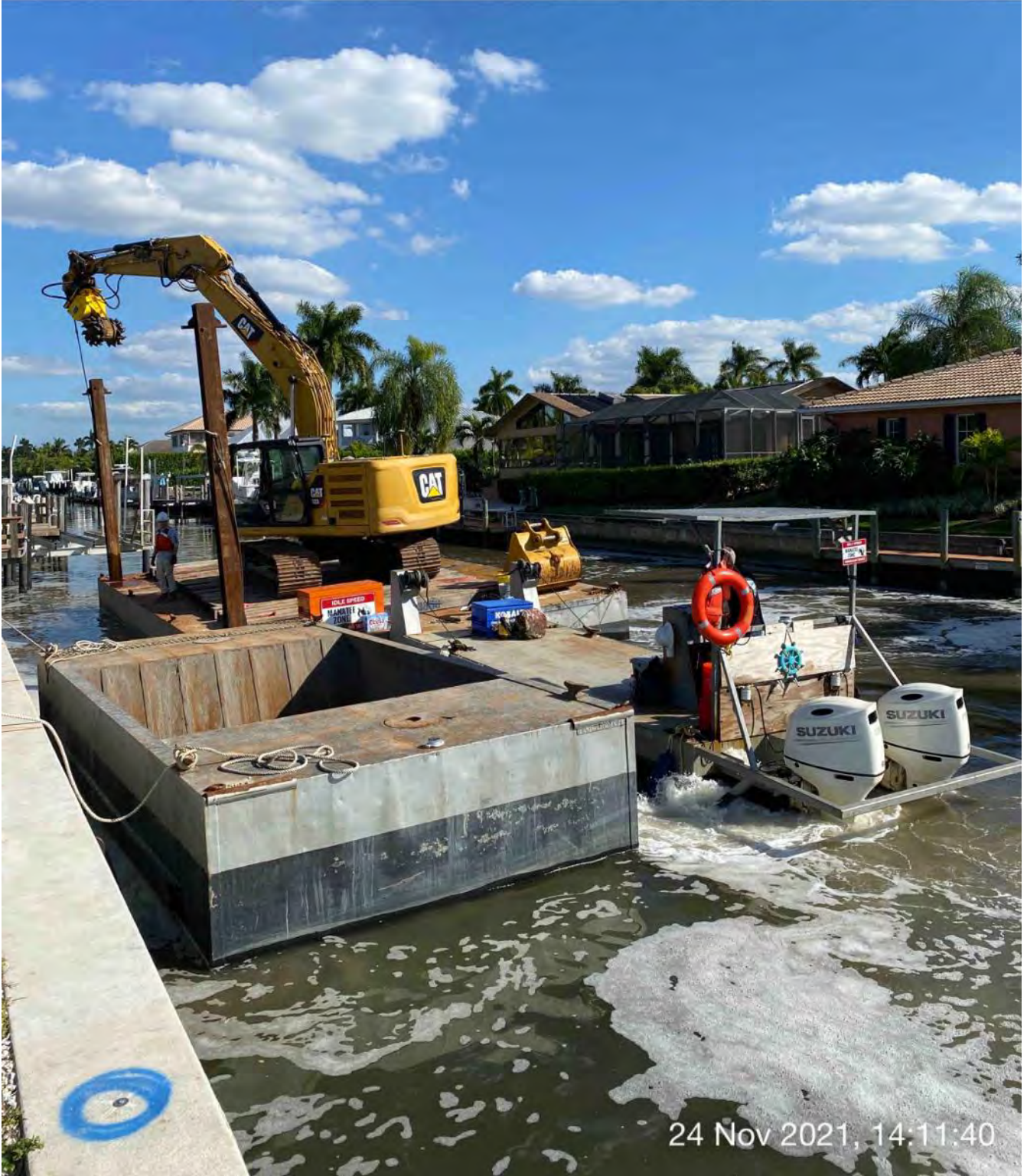
323 excavator lifting spud to allow push boat to move barge to station 2+00
