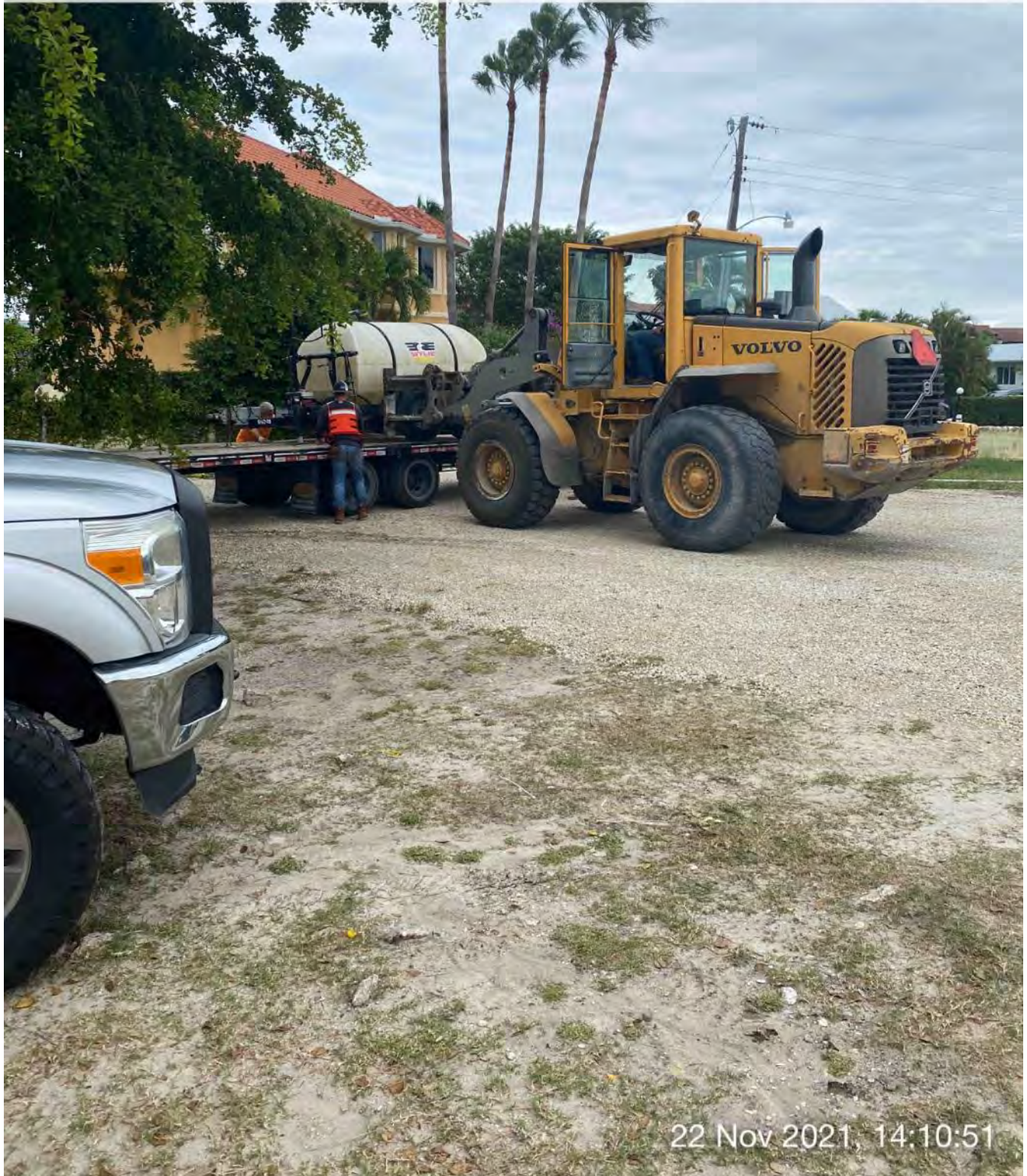
Front end loader moving water tank from transport truck to east side of 1300 Curlew Avenue
