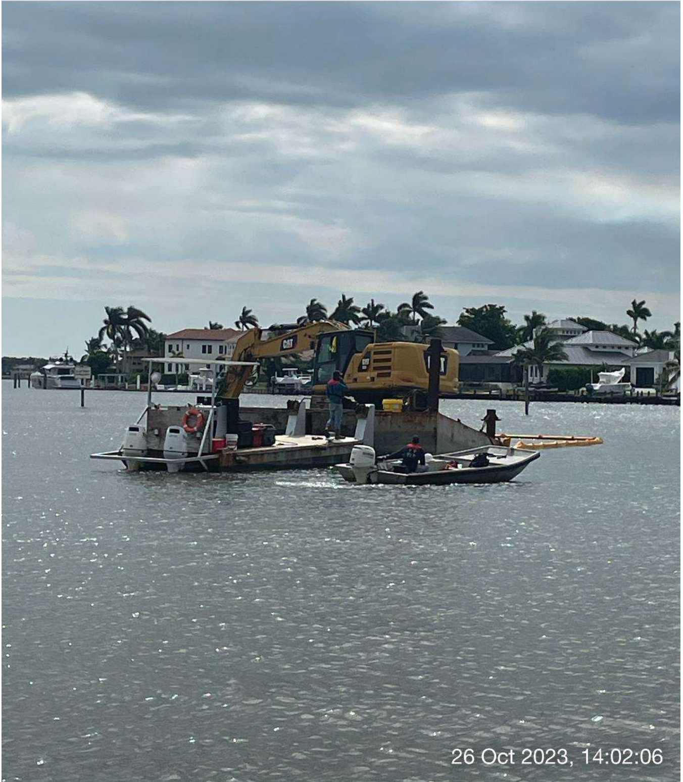
323 excavator digging for missing cutter drum at station 1+00 in Canal Main B.
