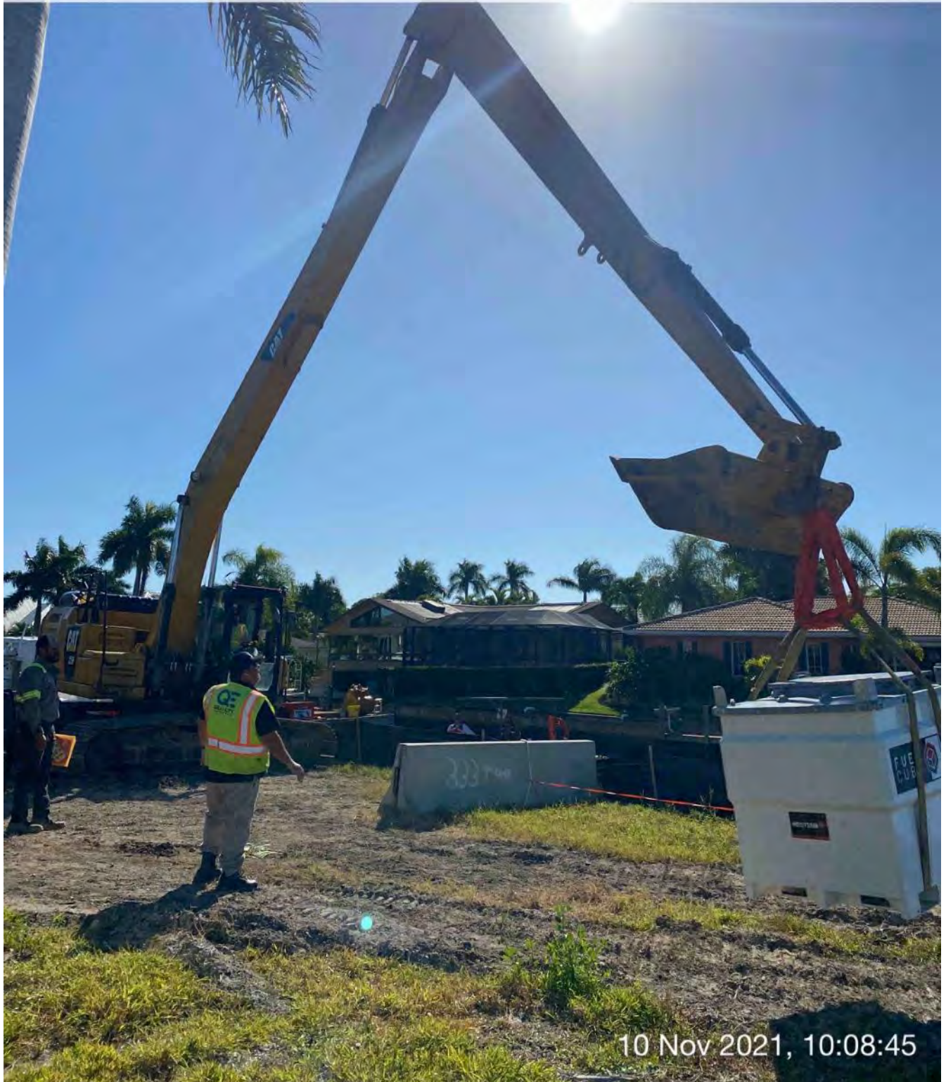
326 excavator transporting small fuel cell from south side of empty lot at 1300 Curlew Avenue to push boat
