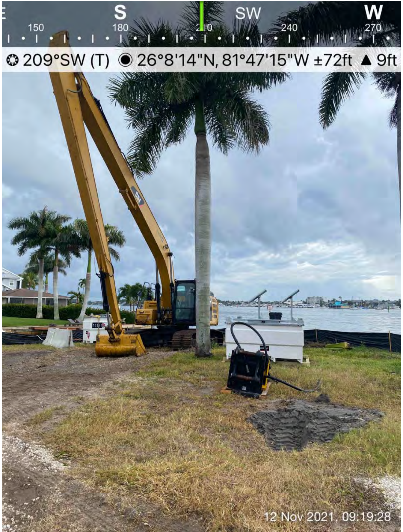
326 excavator, Epiroc grinder, and two fuel cubes staged in the southwest corner of the lot at 1300 Curlew Avenue
