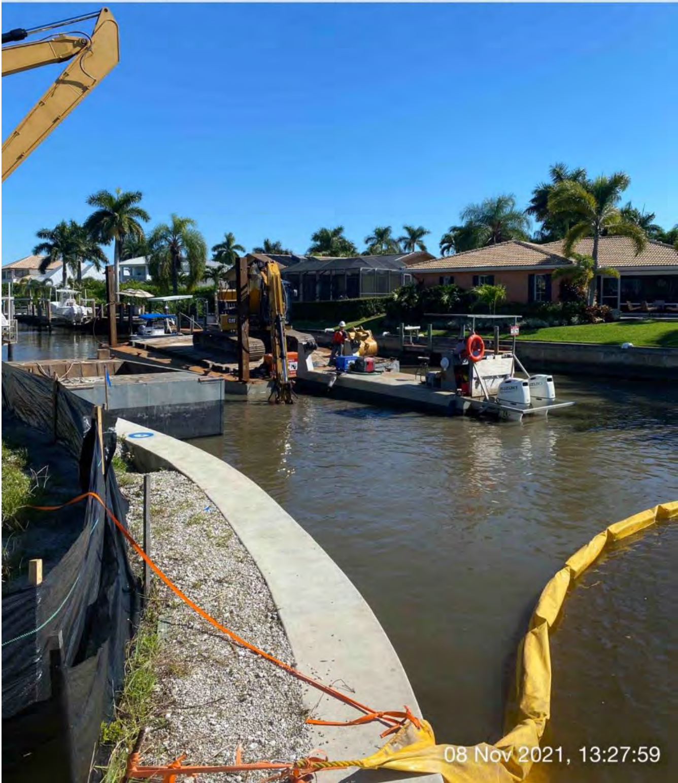
Turbidity curtain across the mouth of Canal CC-CC. 323 excavator grinding rock at station 2+00
