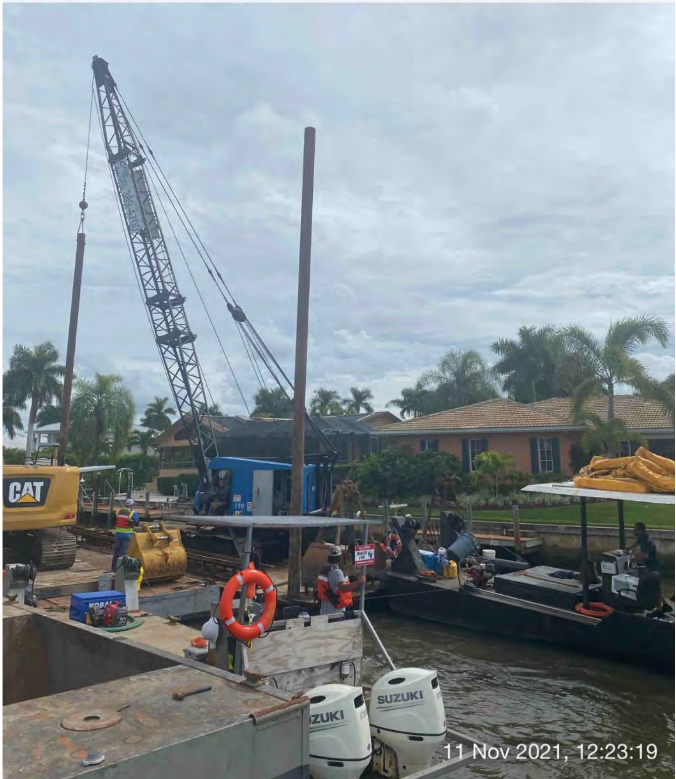
Another contractor's barge, crane, and push boat moving west down canal CC-CC
