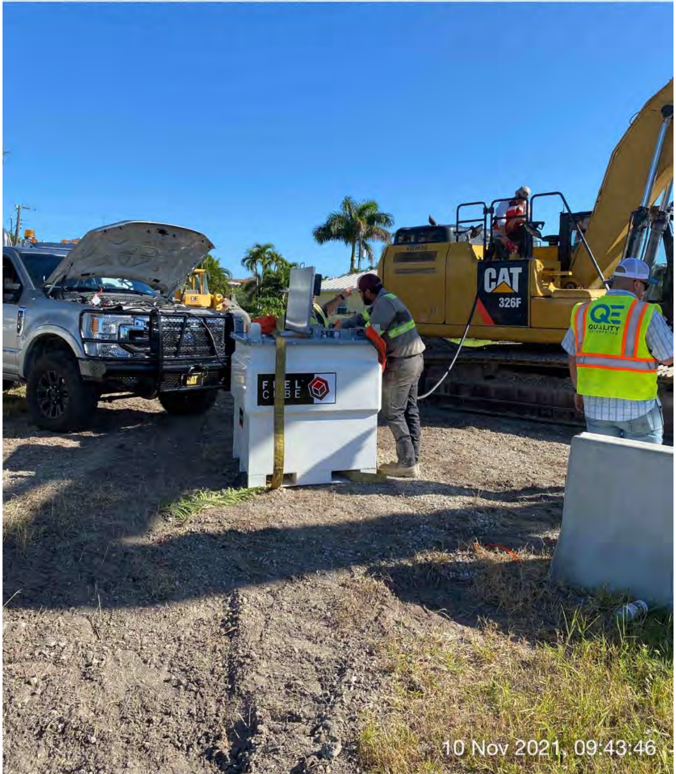
Technician connecting jumper cables from car battery to fuel cell battery. Assistant filling up 326 excavator with fuel.
