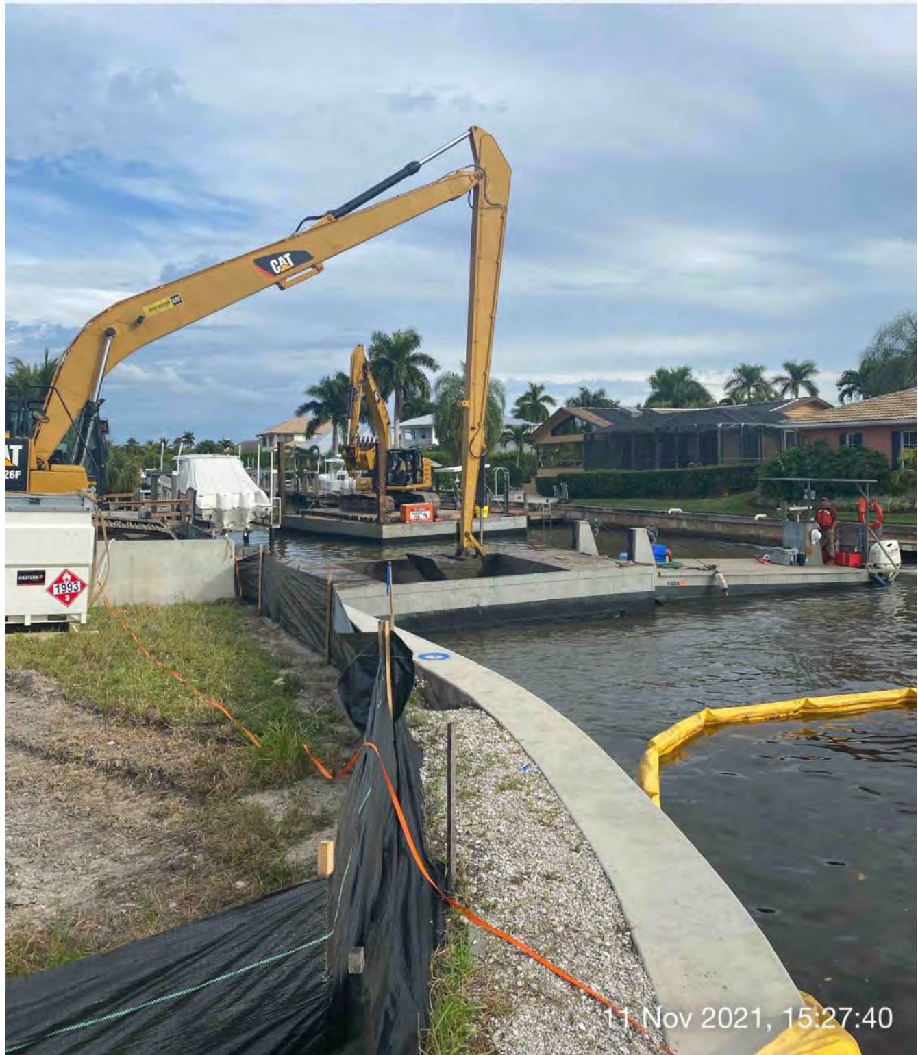
326 excavator transporting rock and sediment from the hopper to the dewatering site at 1300 Curlew Avenue
