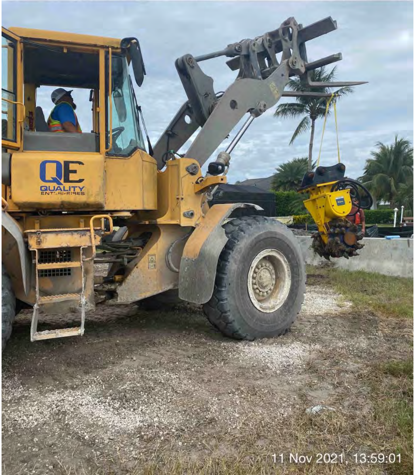
Front end loader transporting Epiroc grinder to the empty lot at 1300 Curlew Avenue
