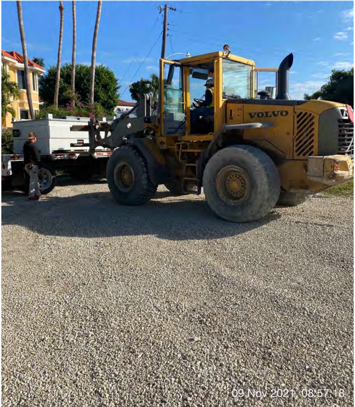
Front end loader moving large fuel cube from transport truck to empty lot at 1300 Curlew Avenue
