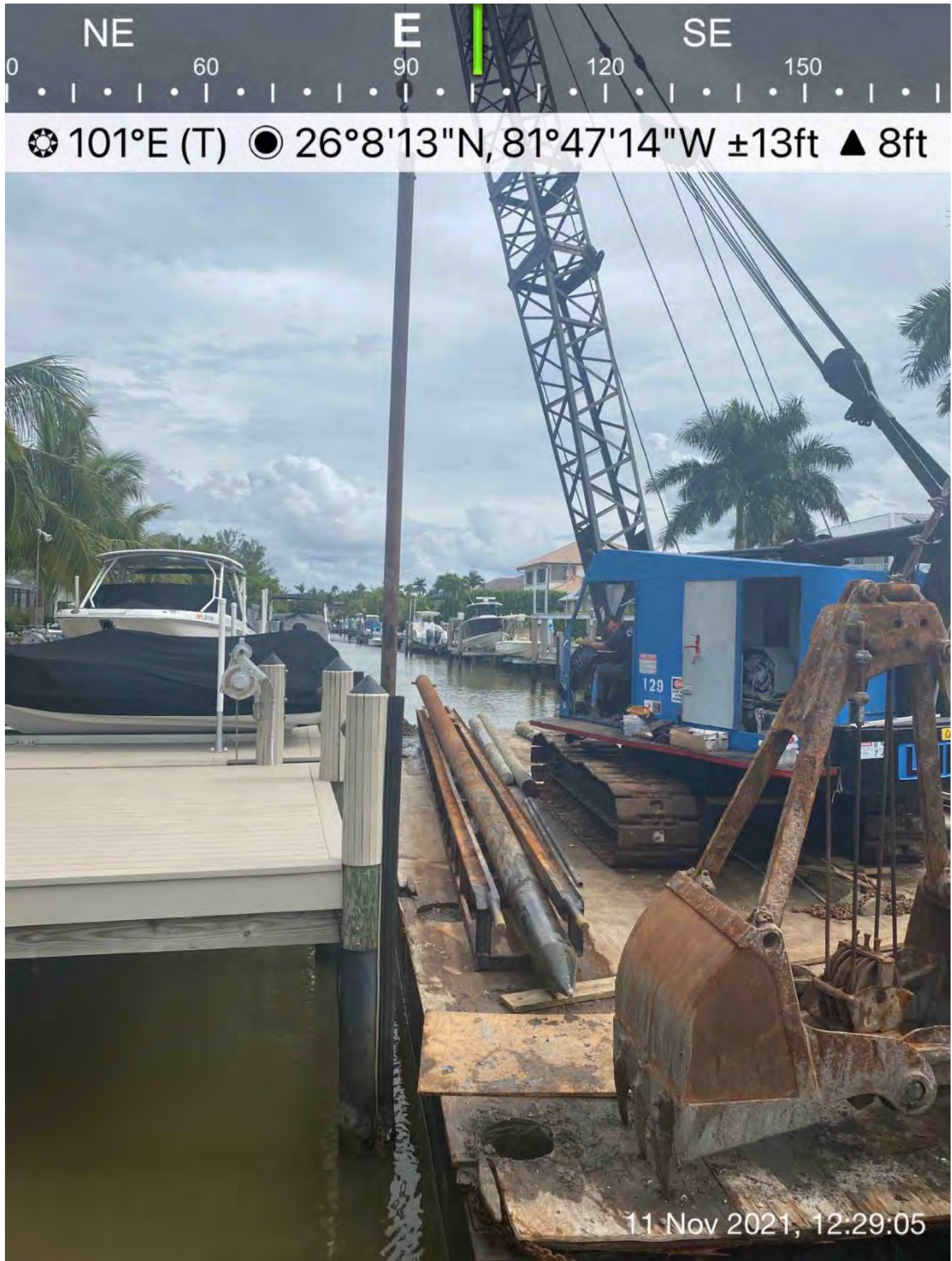
Another contractor's barge, crane, and push boat near a dock at station 4+00
