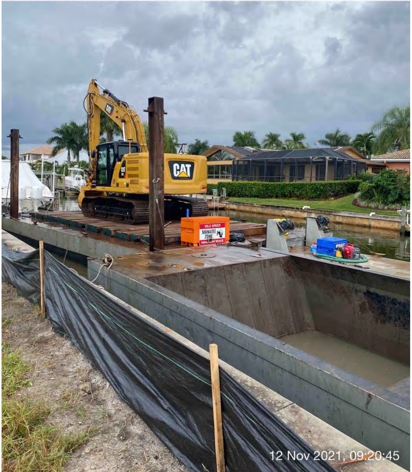
Barge, 323 excavator, push boat, and hopper staged in Canal CC-CC between stations 1+50 and 2+00
