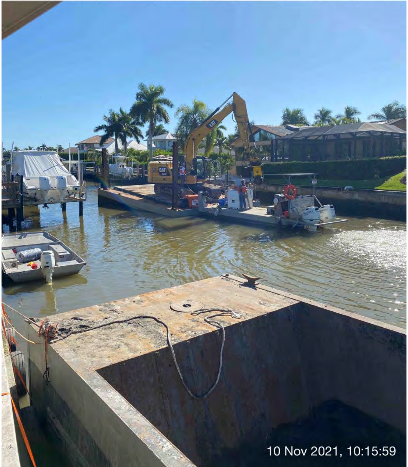
Push boat moving barge and hopper tied to barrier walls on the North side of Canal CC-CC near station 1+50
