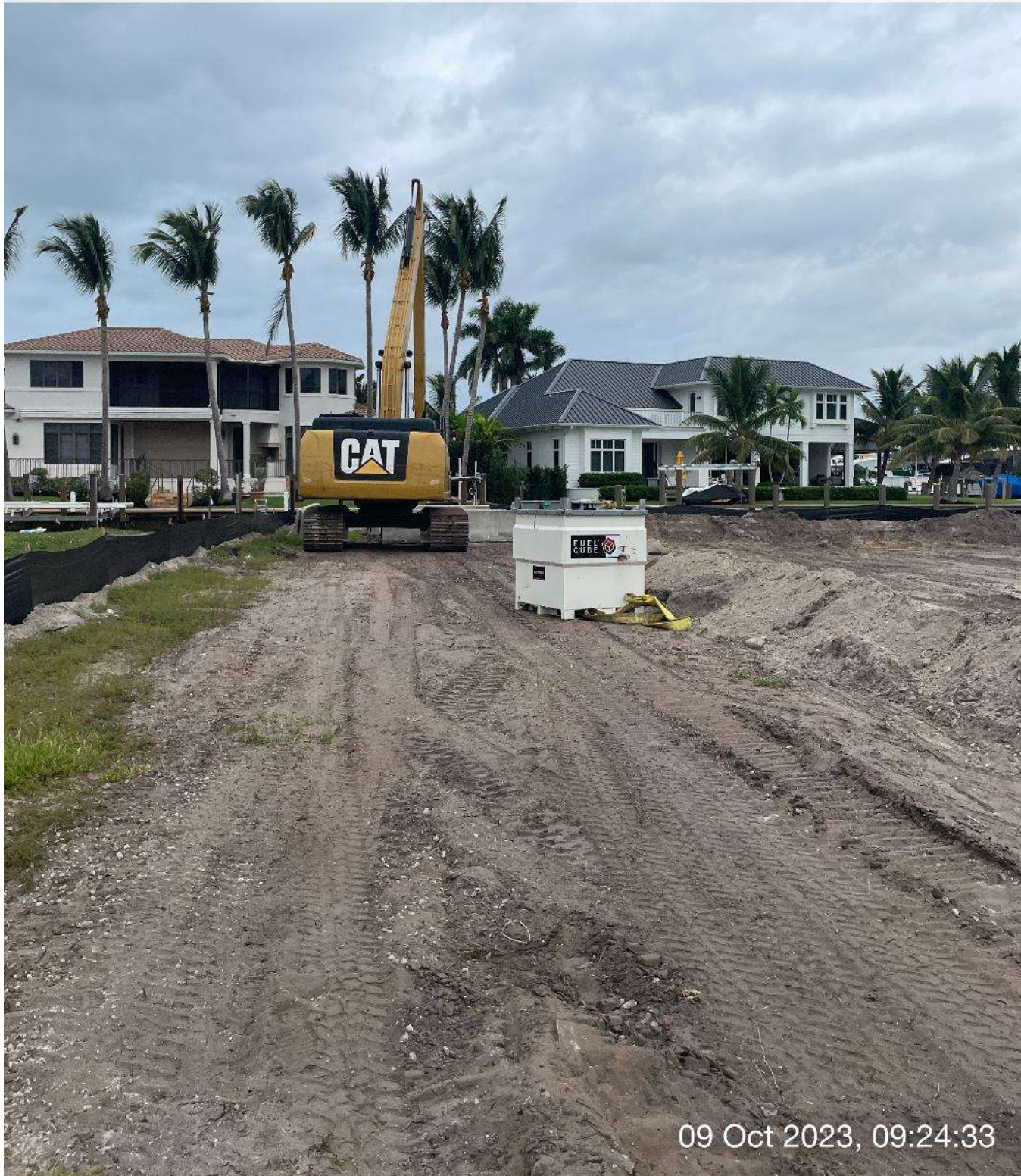
Fuel cube at staging area at 1387 Marlin Drive.
