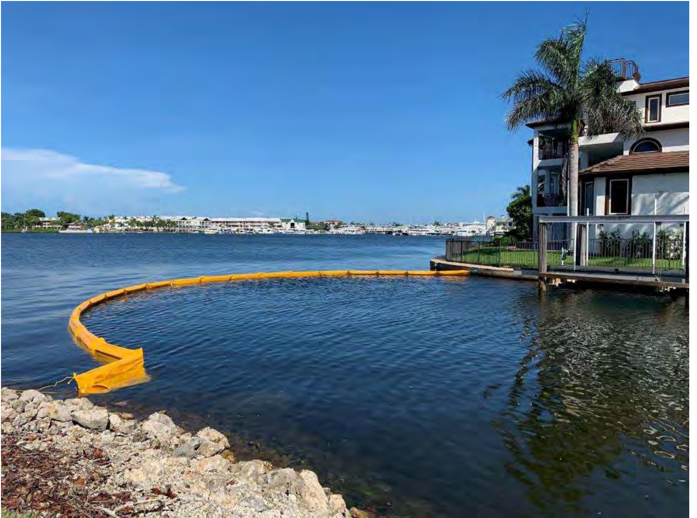
Turbidity curtain closed at mouth of Canal X-X (station 1+00) after dredge equipment entered the Canal.
