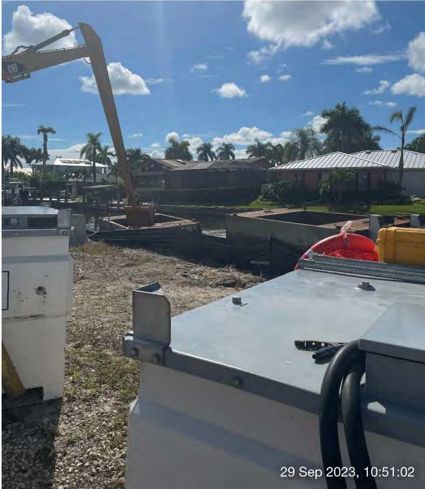
Returning hopper filled with material to the staging area and taking empty hopper back to Canal X-X.
