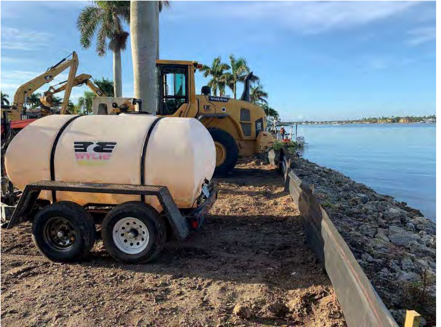
Water tank on trailer at staging area. Silt Fence in place along perimeter of staging area.
