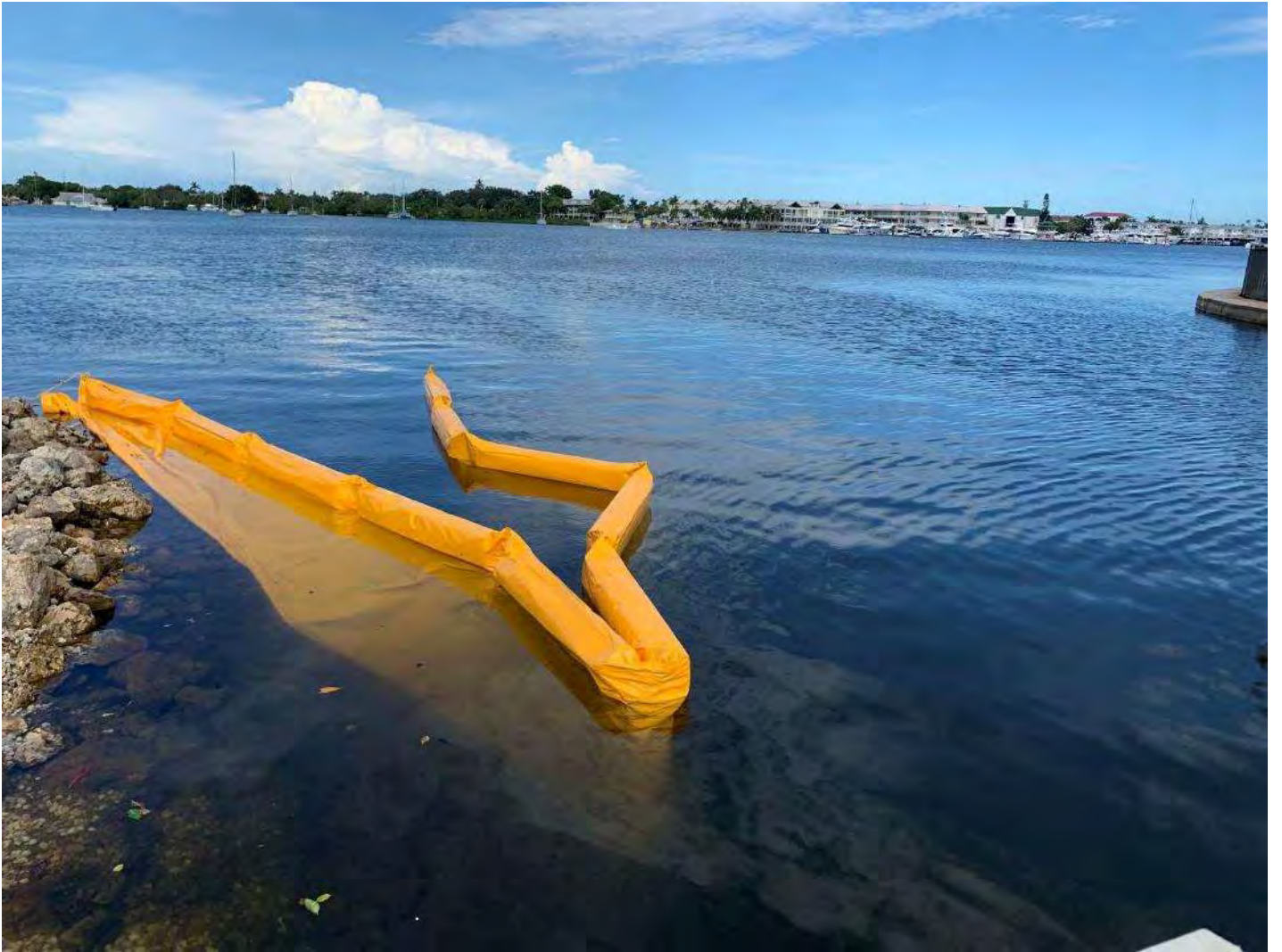
Turbidity curtain open to allow barge, hopper, and push boat into Canal X-X.
