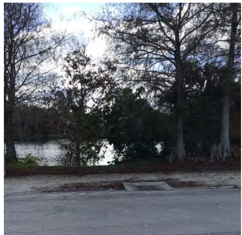
6. Lake 19: Curbside Inlet capturing runoff from 15 th Ave N. 24" reinforced concrete pipe discharging into Lake 19.
