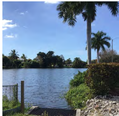
12. Lake 19: Stormwater grate outfall with weir with 2 - 30" reinforced concrete pipe discharging from Lake 19.
