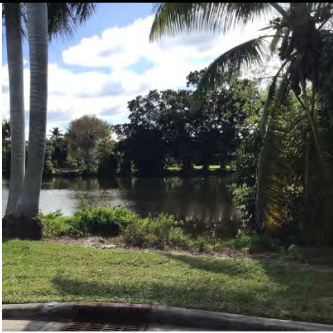
7. Lake 19: Curbside Inlet capturing runoff from 15 th Ave N. 24" reinforced concrete pipe discharging into Lake 19.
