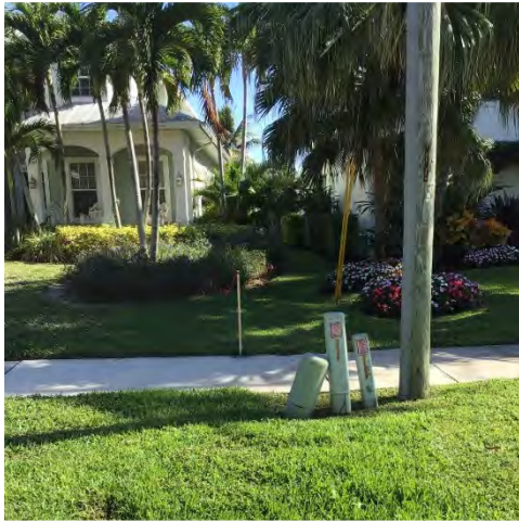
Lake 11: Stormwater inlet along W Lake Dr with 24" PVC pipe running between two residents along Lake 11 with concrete headwall
