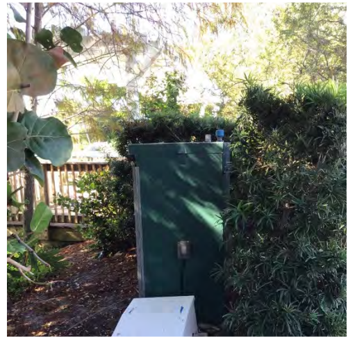
6. Lake 11: Diffuser and fountain compressor and pumps
