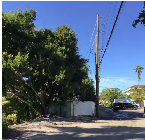
4. Lake 11: Overhead electric poles and lines, transformer, fire hydrant, and water valve and backflow assembly
