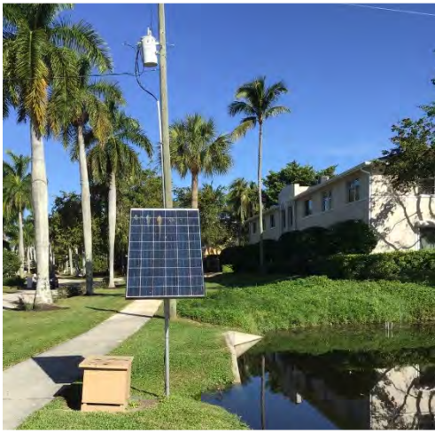
17. Lake 31: overhead electric poles and lines, diffuser compressor and solar panel, and culverts directly discharging into Lake 31 from Lake 11
