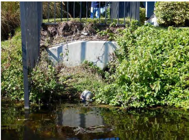
11. Lake 11: Culvert on west side of lake partially blocked by wedilia
