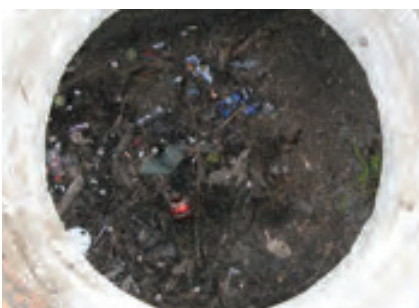
Easy maintenance access via top hatches / manholes without need for confined space entry.
