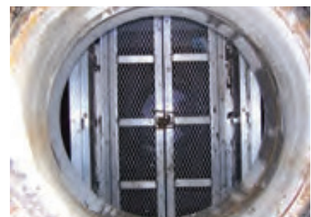
After cleaning sediment chambers, close and secure bottom screen doors to prevent debris loss.
