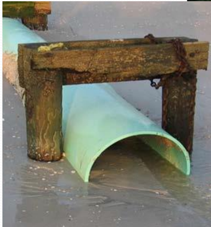
Blocked Discharge (Outfall 9)
