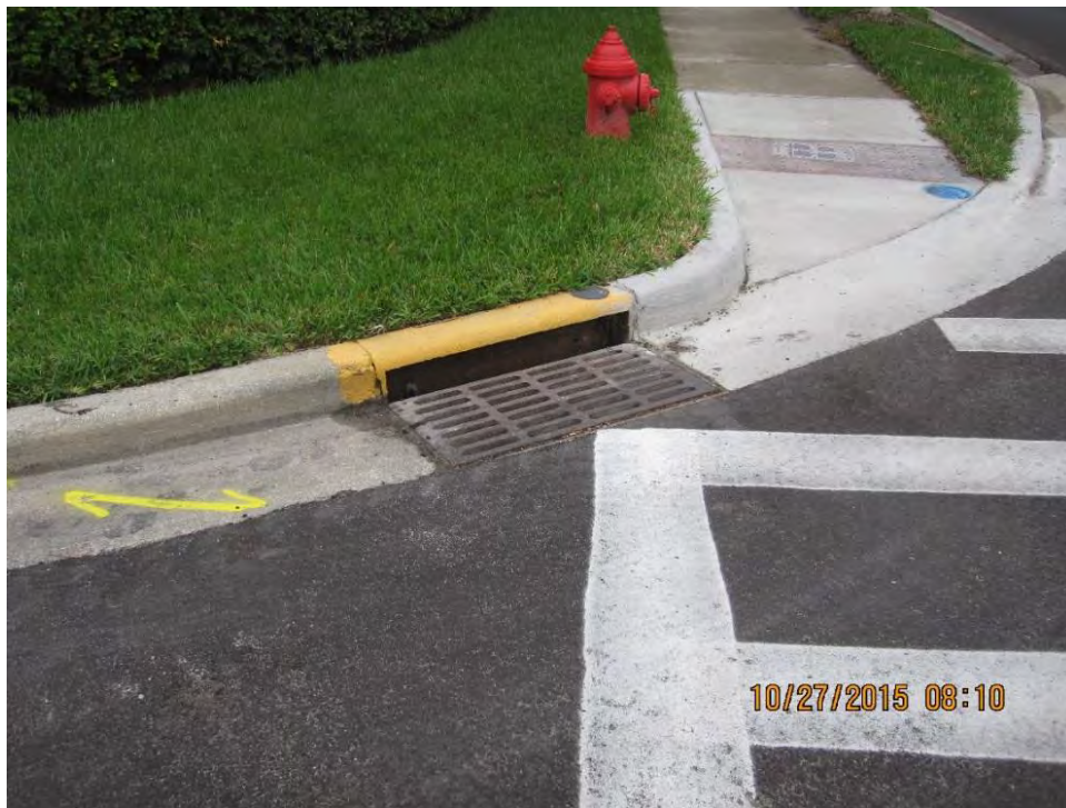
Figure 5-3. Typical Intersection with Utilities – Storm Drain in Foreground with Potable Water Line in Background
