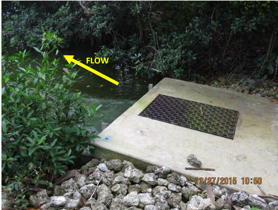
Figure 3-4. Alligator Lake Control Structure
