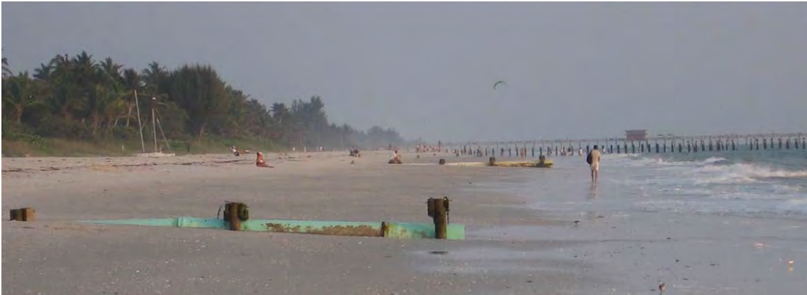
Figure 1-3. Typical Outfall Blockage (Outfall 9)
