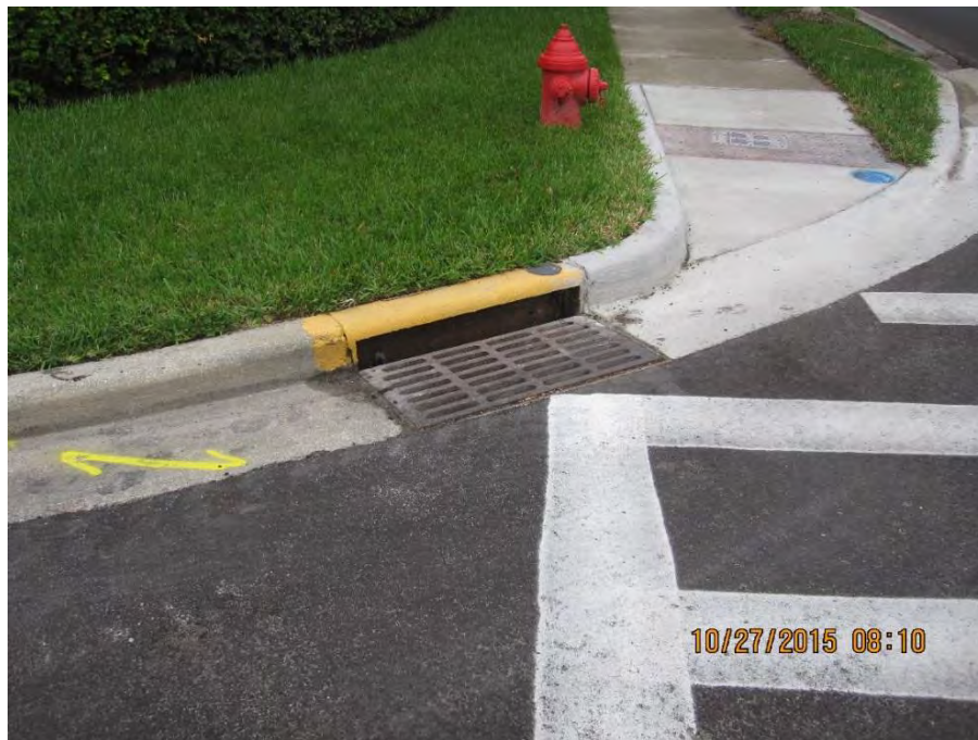
Figure 3-8. Typical Intersection with Utilities – Storm Drain in Foreground with Water Line in Background
