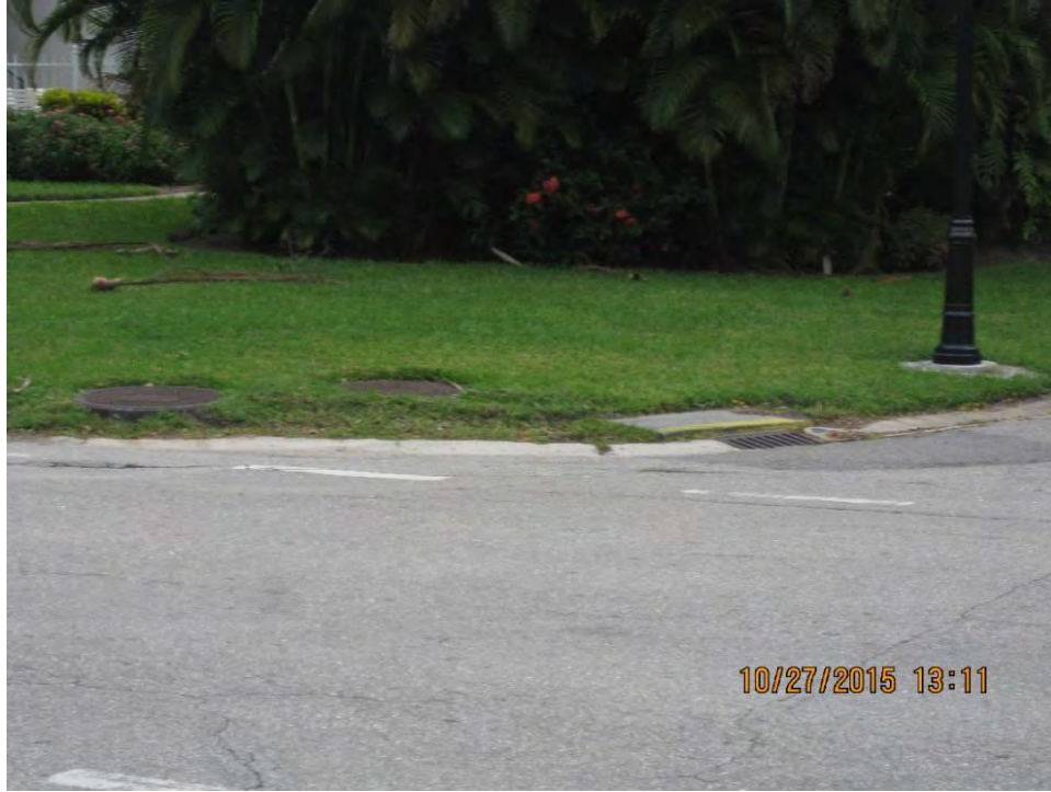
Figure 5-2. Typical Intersection with Utilities – Storm Drain with Adjacent Fiber Optic Cable Manholes
