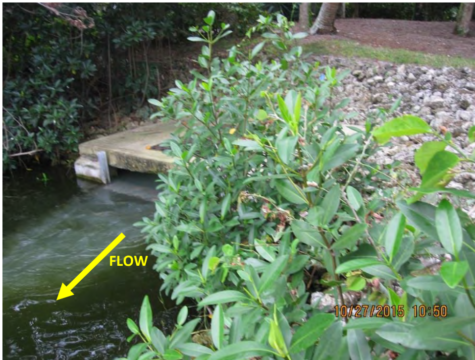
Figure 3-5. Alligator Lake Control Structure Weir
