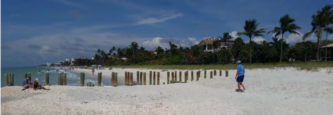
Figure 1-2. Impaired Lateral Access and Shoreline Offset (Scour Induced Erosion) (Outfall 6)
