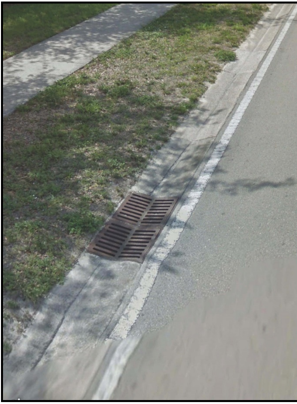
Figure 1: Depiction of a double valley gutter inlet directly over a 36-inch diameter storm sewer pipe.
