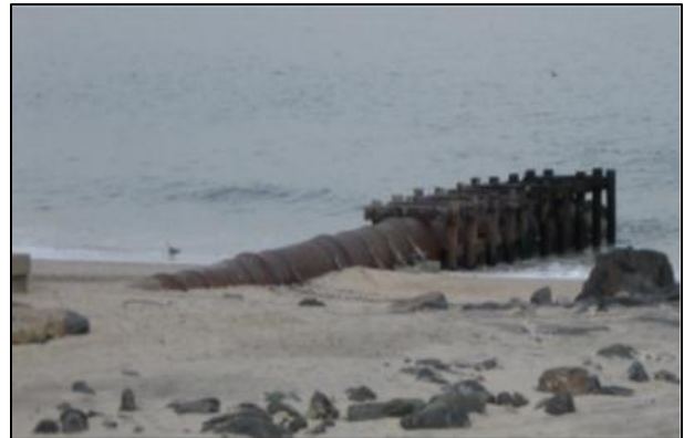
Photograph 2: Outfall at Long Branch, New Jersey on December 24, 2012 – months after Super storm Sandy. Structure is low and high surge may have carried waves over the top and not thru the structure.
